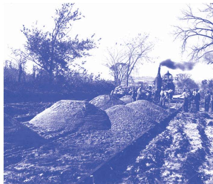
1918 Photo of construction in progress on Linn County Seedling Mile. Note use of steam-powered mixer. Photo Courtesy: Iowa Department of Transportation, Ames
