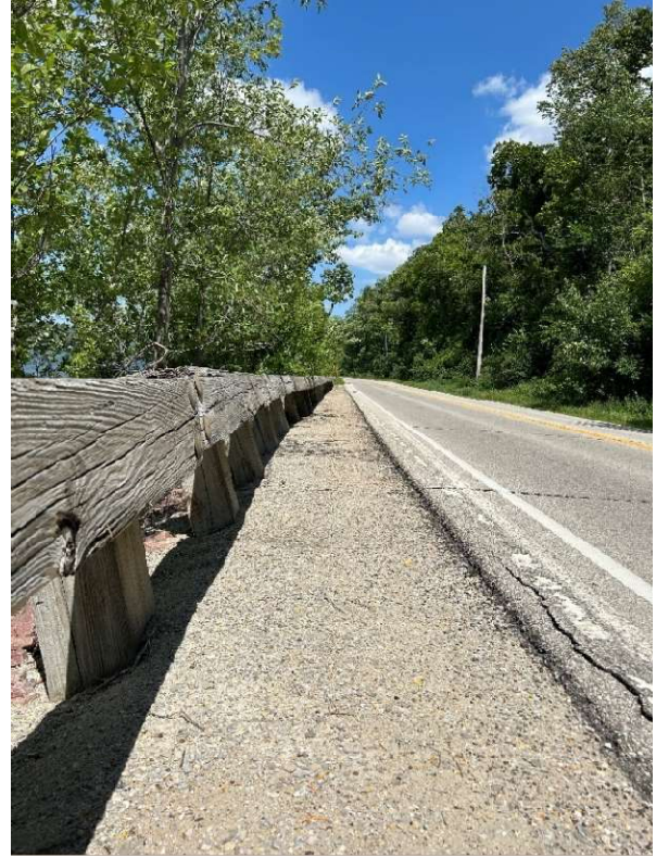
Figure 3: Showing riverward tilt of existing guardrail
