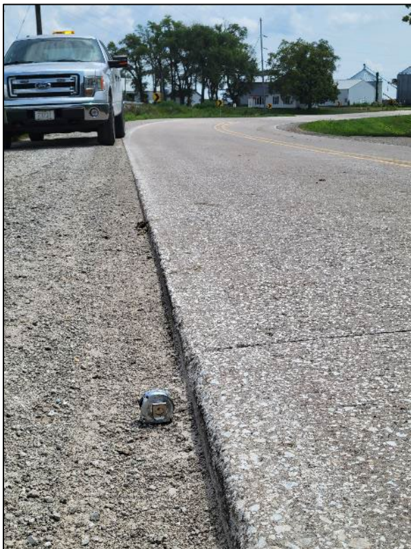
Photo 2: Typical edge rutting near curve.
