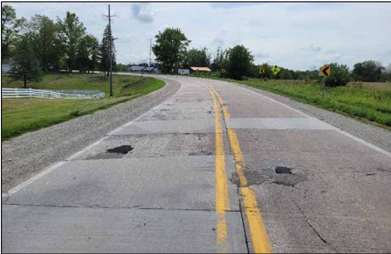
Photo 6: Project curve showing roadway deterioration.
