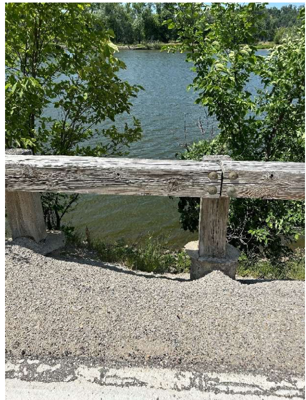
Figure 4: Conditions behind guardrail
