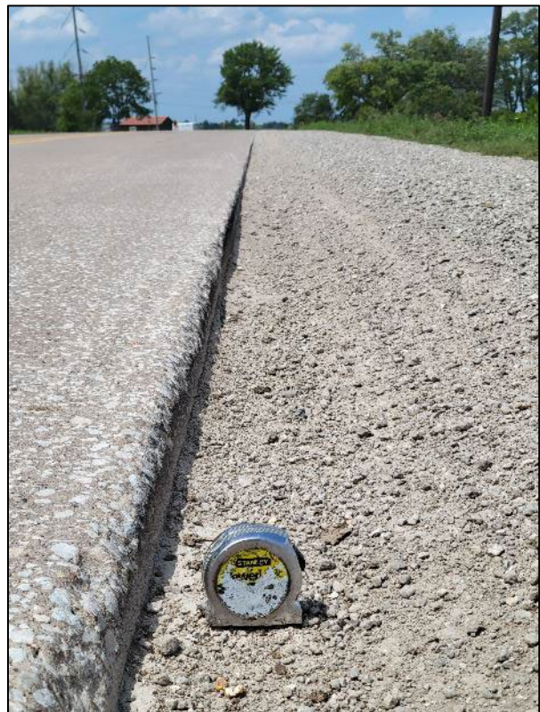
Photo 3: Edge rutting along straight section.
