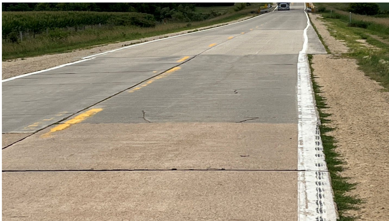
F1. Existing narrow pavement @ Cedar County Line
