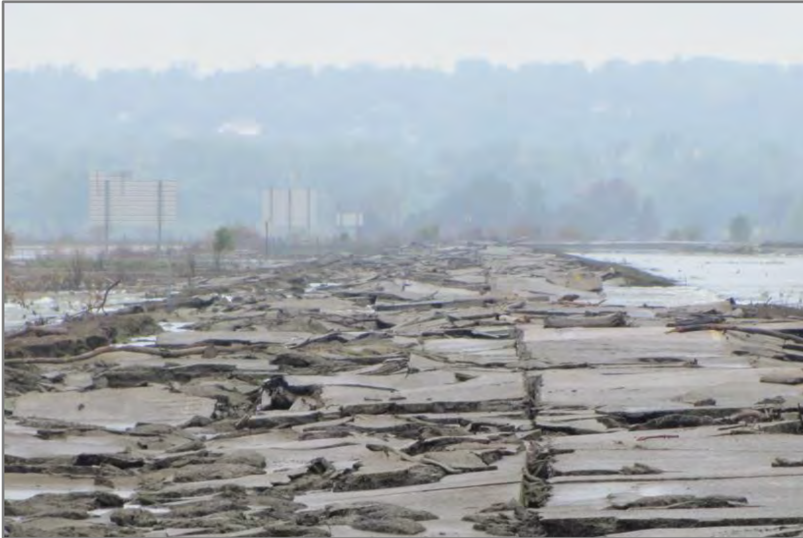
Receding water reveals damage
