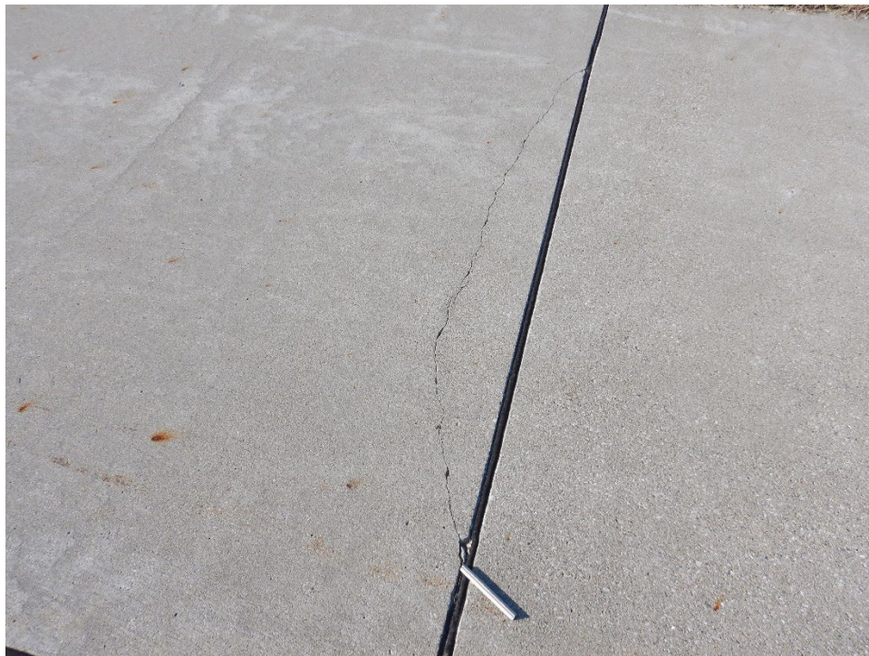
T05AM-02. Joint Spalling (Sample Unit No. 04).
