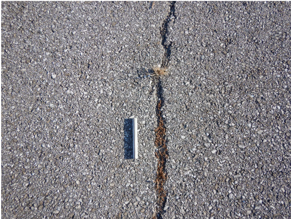
T01AM-03. L&T Cracking (Sample Unit No. 01).
