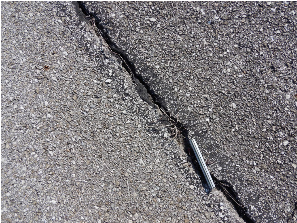
T04AM-01. L&T Cracking (Sample Unit No. 01).
