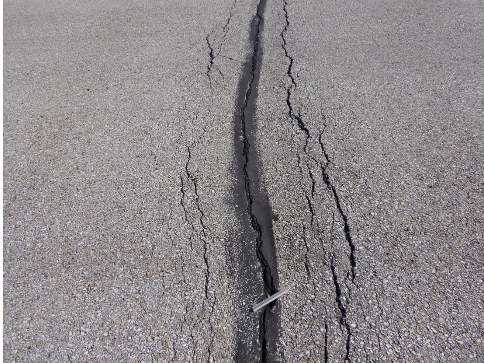
T01AM-02. L&T Cracking (Sample Unit No. 10).
