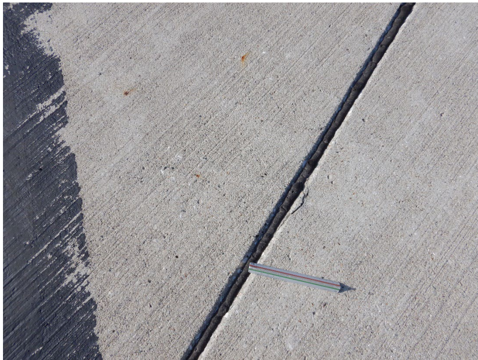
T05AM-04. Joint Seal Damage (Sample Unit No. 01).
