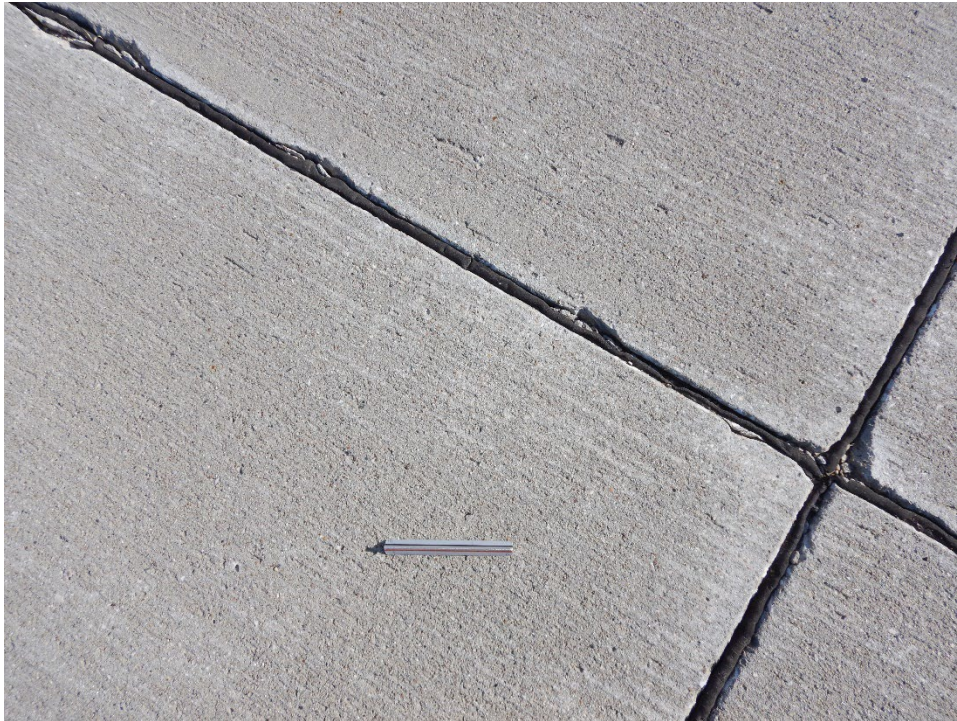
A01AM-02. Joint Seal Damage (Sample Unit No. 14).
