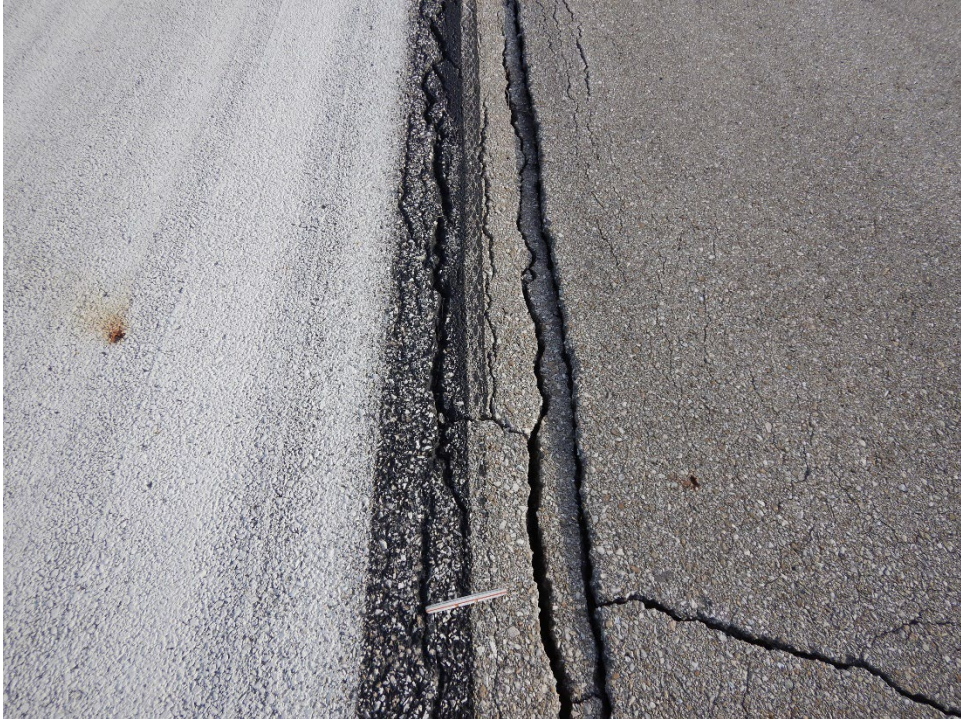
R13AM-02. L&T Cracking (Sample Unit No. 01).
