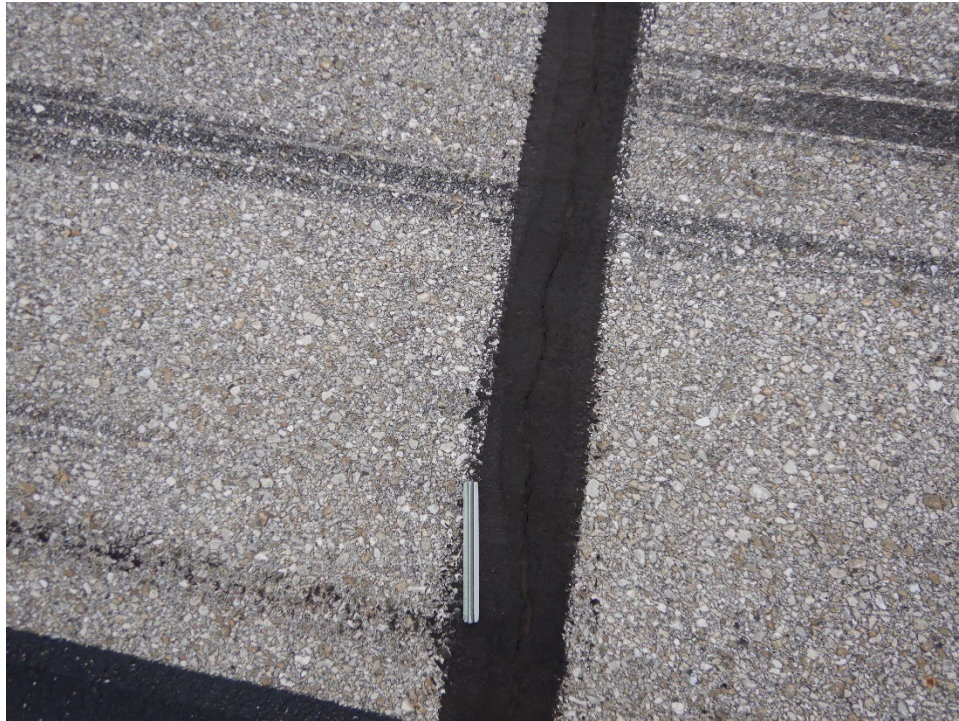
R01AM-01. L&T Cracking (Sample Unit No. 22).
