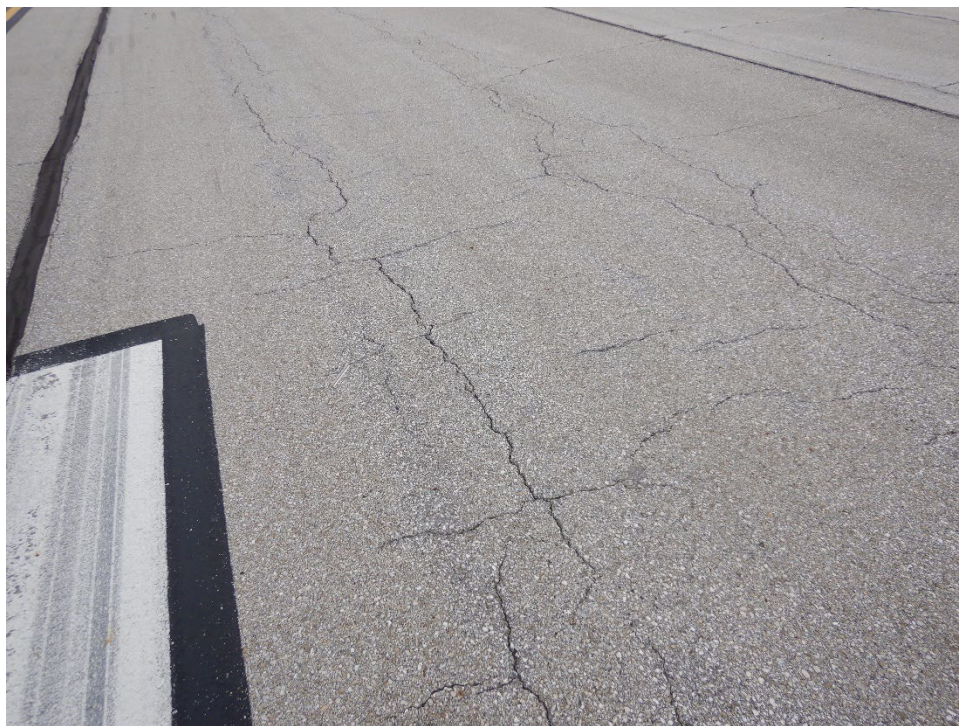
R01AM-01. Block Cracking (Sample Unit No. 58).
