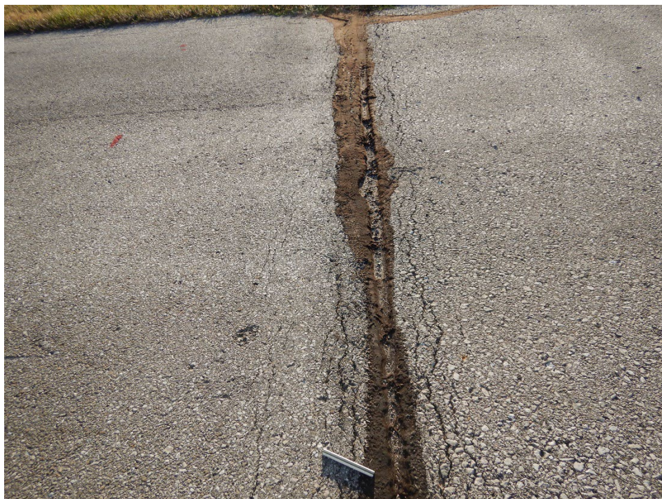
T02AM-02. L&T Cracking (Sample Unit No. 01) (2).
