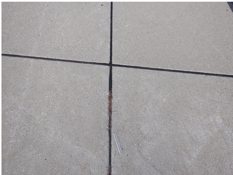
T06AM-02. Joint Seal Damage (Sample Unit No. 03).
