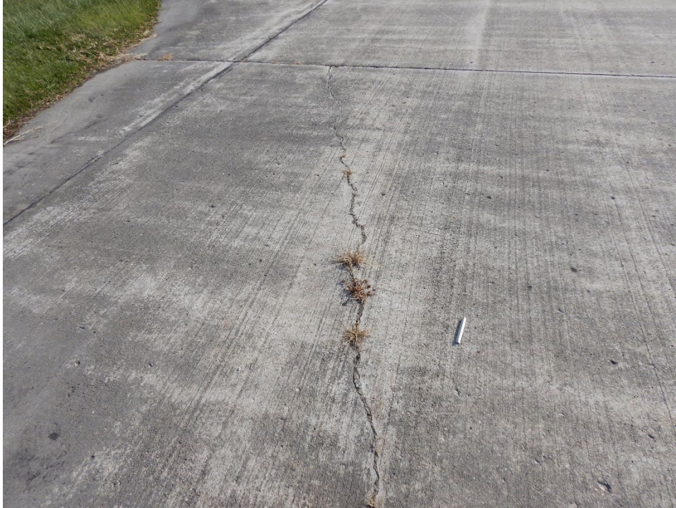
T11AM-01. LTD Cracking (Sample Unit No. 02).
