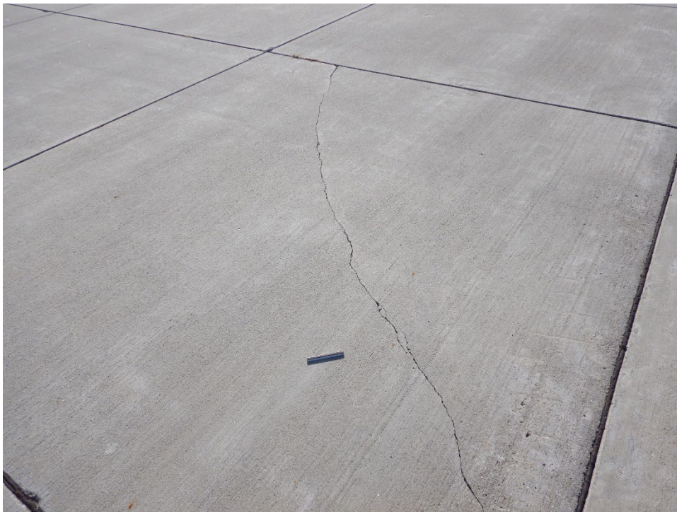
A01AM-02. LTD Cracking (Sample Unit No. 14).
