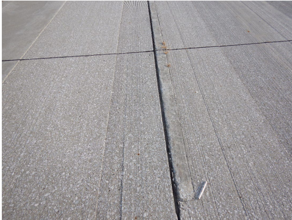
R13AM-01. Large Patching (Sample Unit No. 75).
