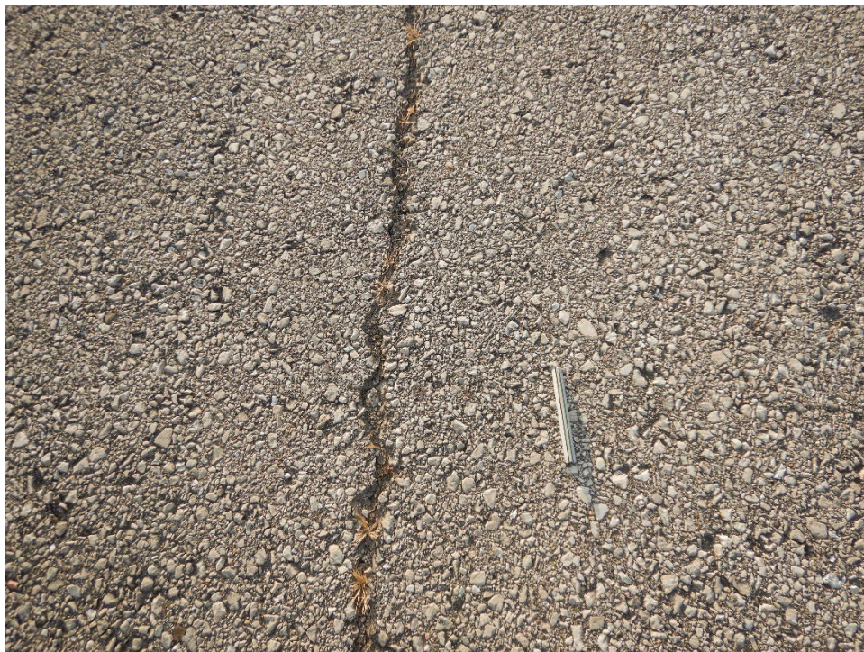
A01AM-01. L&T Cracking (Sample Unit No. 11).
