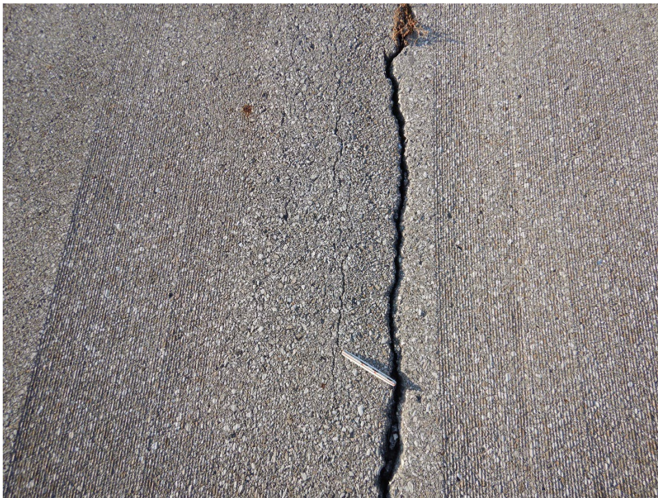
R13AM-03. L&T Cracking (Sample Unit No. 02).
