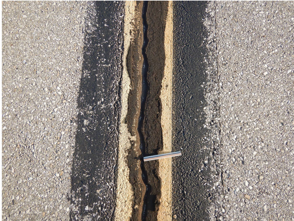
T02AM-02. L&T Cracking (Sample Unit No. 01) (1).
