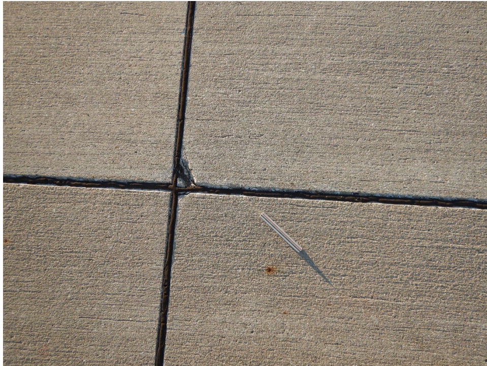
T01AM-07. Joint Seal Damage (Sample Unit No. 03).
