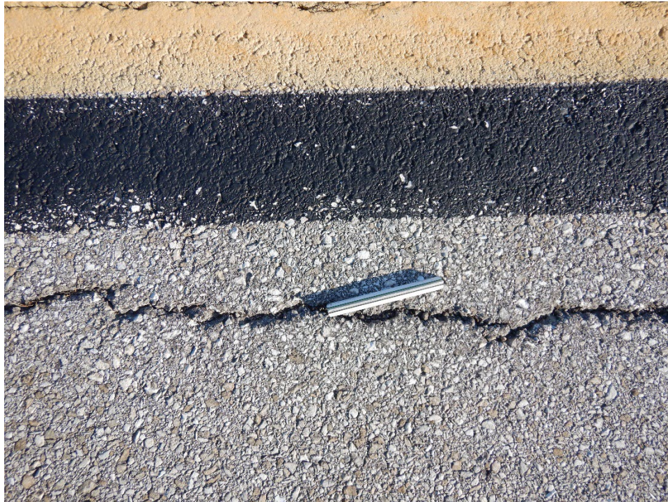
T01AM-04. L&T Cracking (Sample Unit No. 04) (1).
