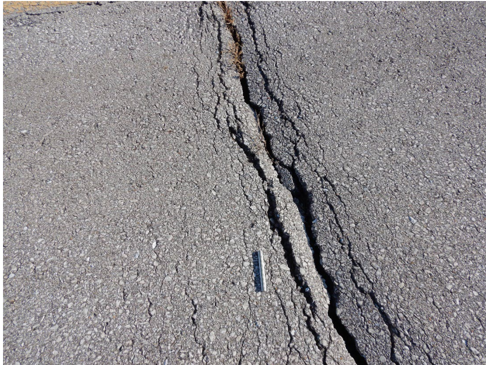
T13AM-02. L&T Cracking (Sample Unit No. 02).
