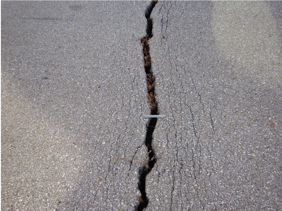
R13AM-02. L&T Cracking (Sample Unit No. 04).
