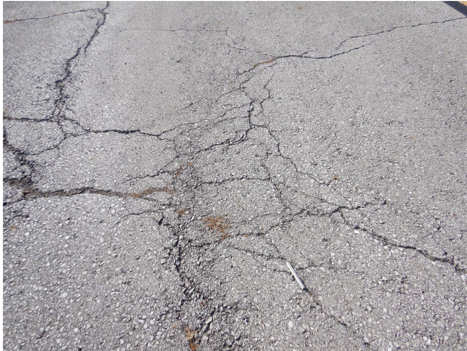
T05AM-01. Alligator Cracking (Sample Unit No. 01).
