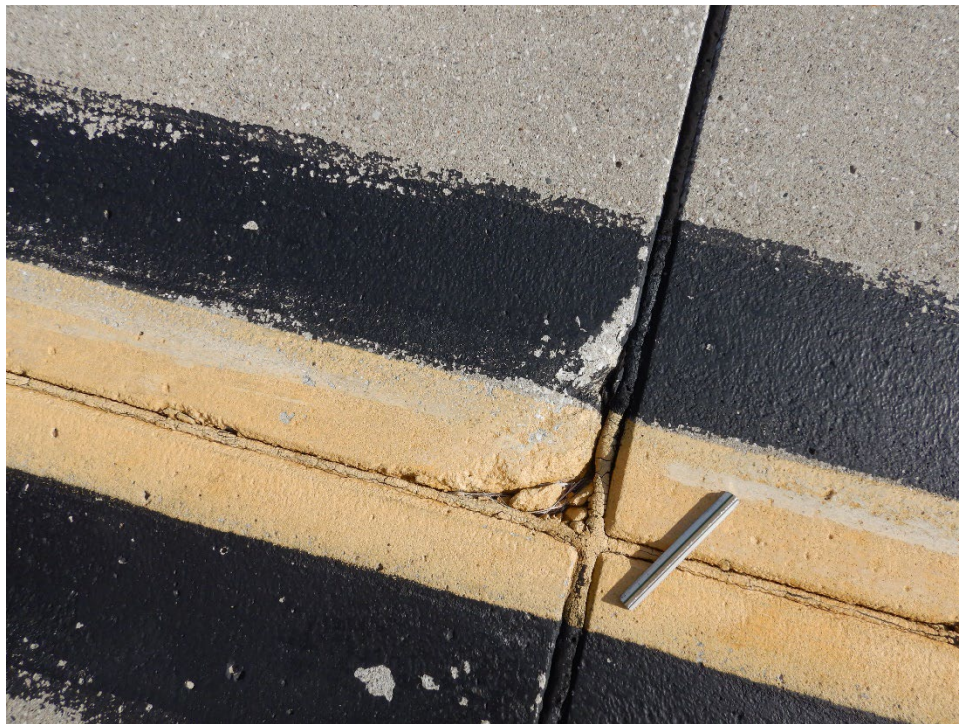
T01AM-05. Joint Seal Damage (Sample Unit No. 04).
