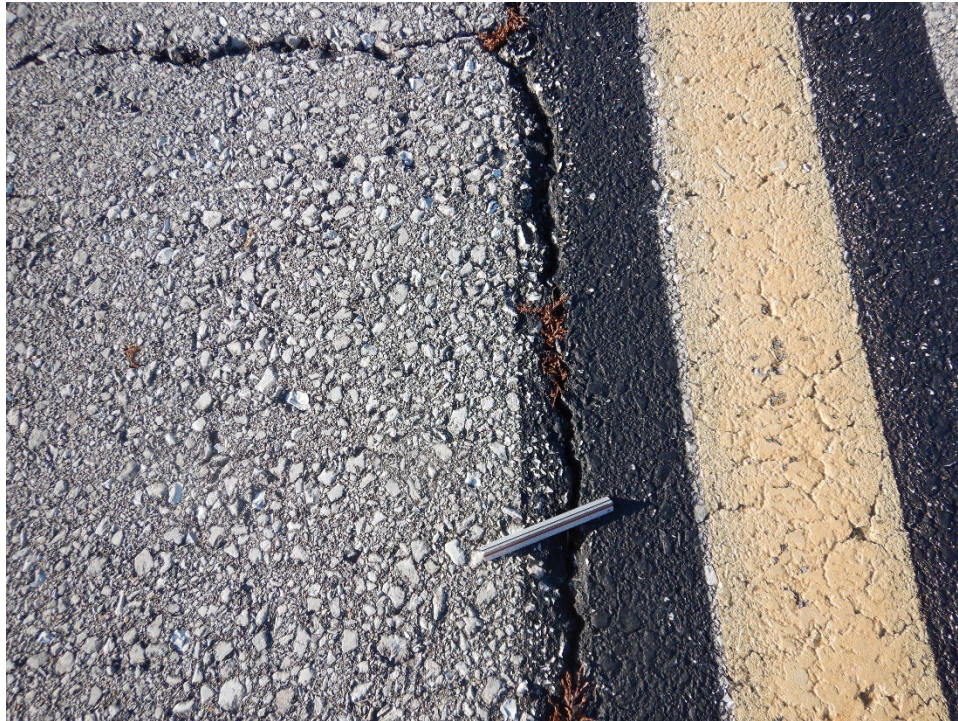
T02AM-04. L&T Cracking (Sample Unit No. 10).
