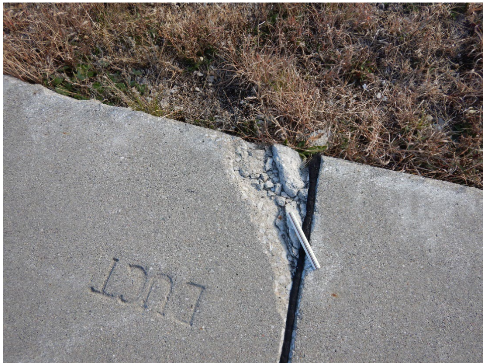
T05AM-03. Corner Spalling (Sample Unit No. 02).
