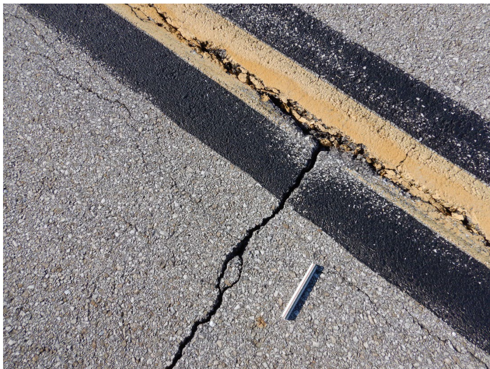
T01AM-02. L&T Cracking (Sample Unit No. 04).
