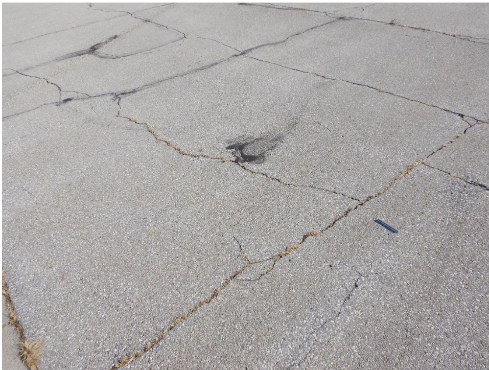
T12AM-02. Block Cracking (Sample Unit No. 01).
