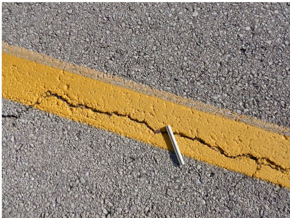
TH01AM-01. L&T Cracking (Sample Unit No. 07).
