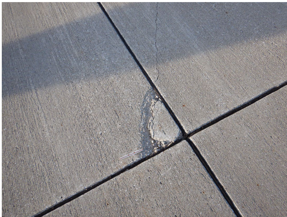
R13AM-04. Corner Spalling (Additional Sample Unit No. 05).
