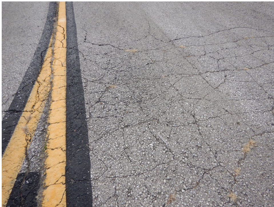
T06AM-01. Alligator Cracking (Sample Unit No. 01).
