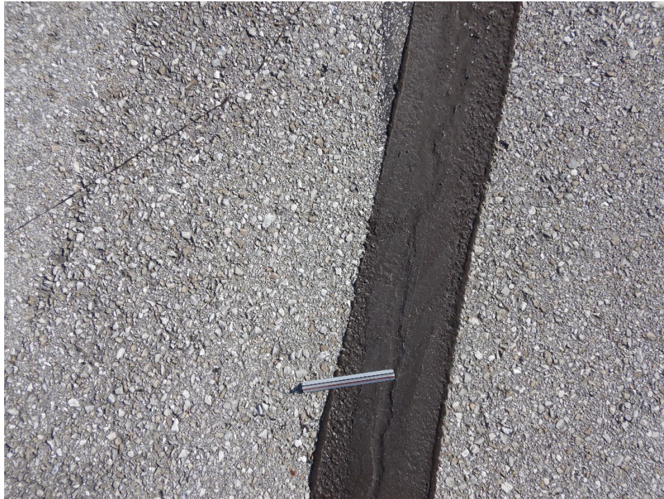
T03AM-02. L&T Cracking (Sample Unit No. 01).
