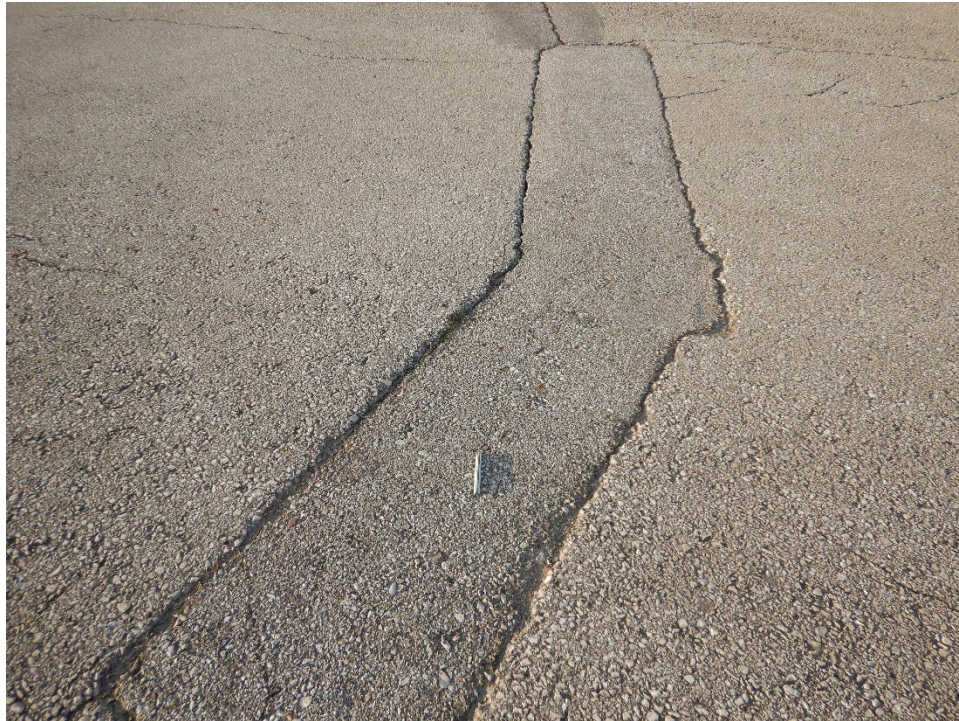
A01AM-01. Patching (Sample Unit No. 11).
