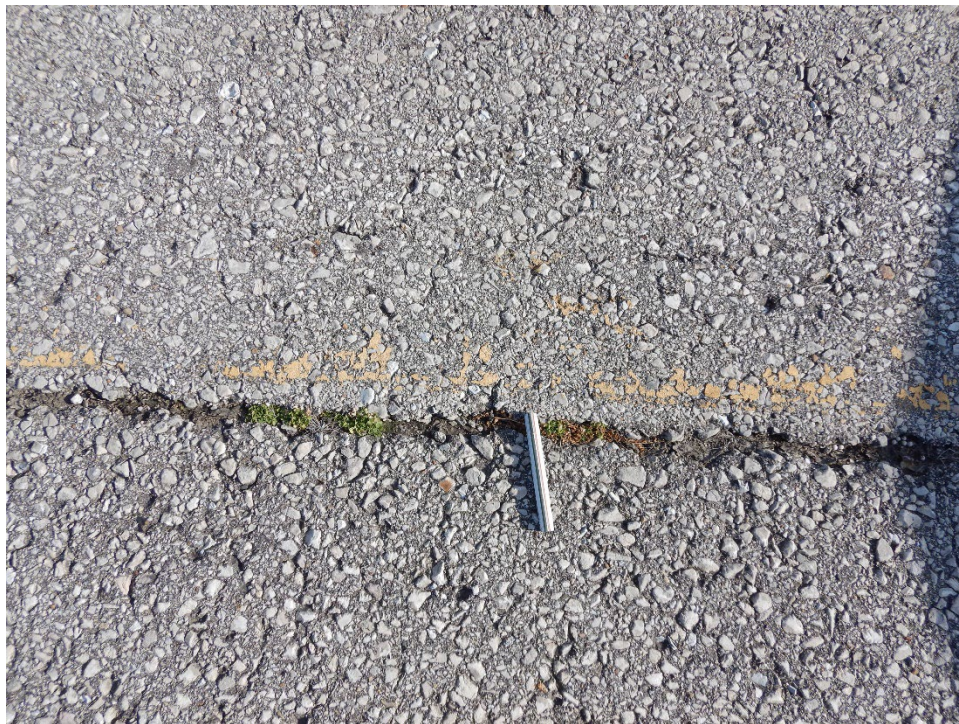
T13AM-02. L&T Cracking (Sample Unit No. 03).
