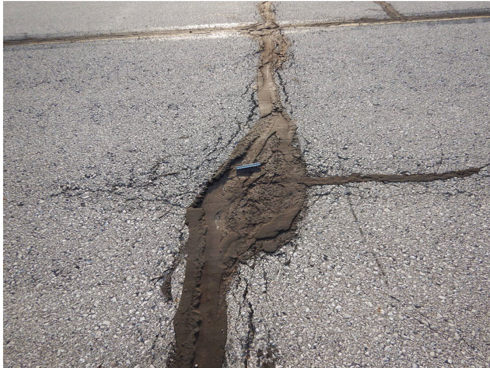
T02AM-01. L&T Cracking (Sample Unit No. 07) (2).
