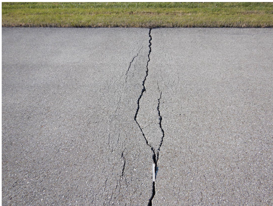
T01AM-04. L&T Cracking (Sample Unit No. 04) (2).
