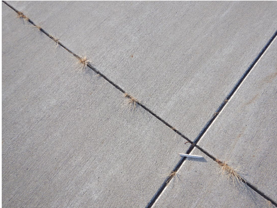
R13AM-04. Joint Seal Damage (Sample Unit No. 28).
