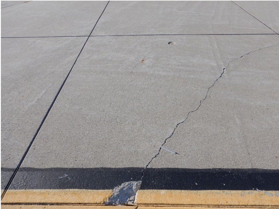
T01AM-06. LTD Cracking (Sample Unit No. 05).
