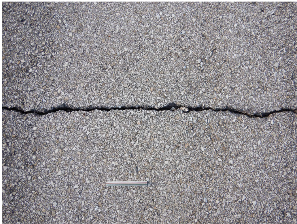
T02AM-03. L&T Cracking (Sample Unit No. 01).
