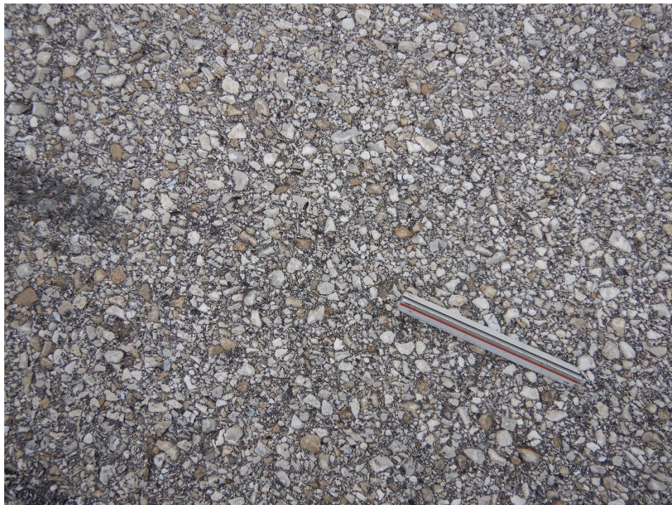
R01AM-01. Weathering (Sample Unit No. 22).
