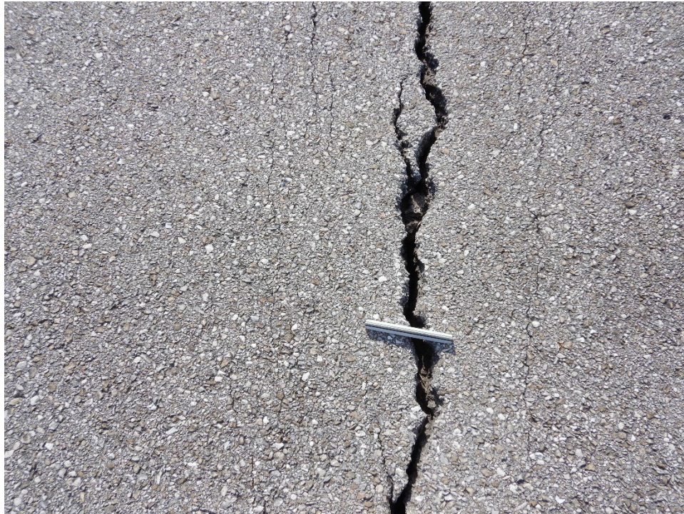
T04AM-02. L&T Cracking (Sample Unit No. 01).
