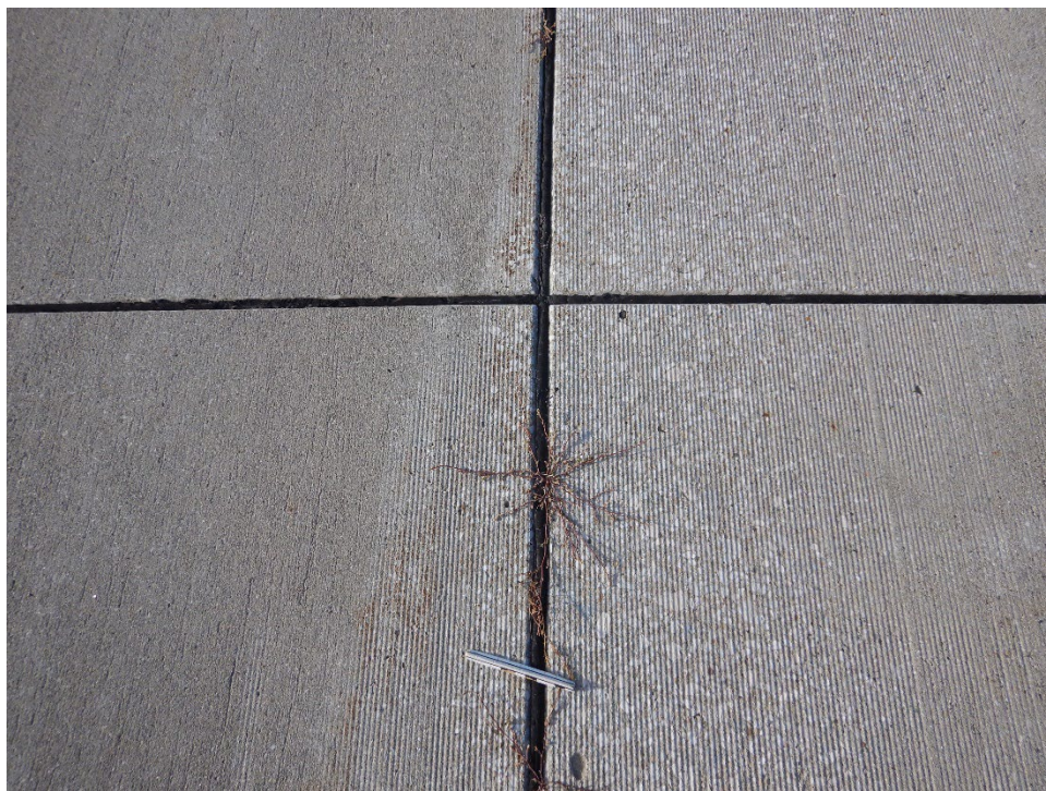
R13AM-01. Joint Seal Damage (Sample Unit No. 53).
