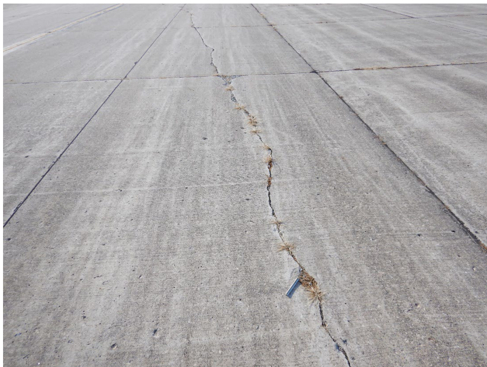
T10AM-01. LTD Cracking (Sample Unit No. 24).
