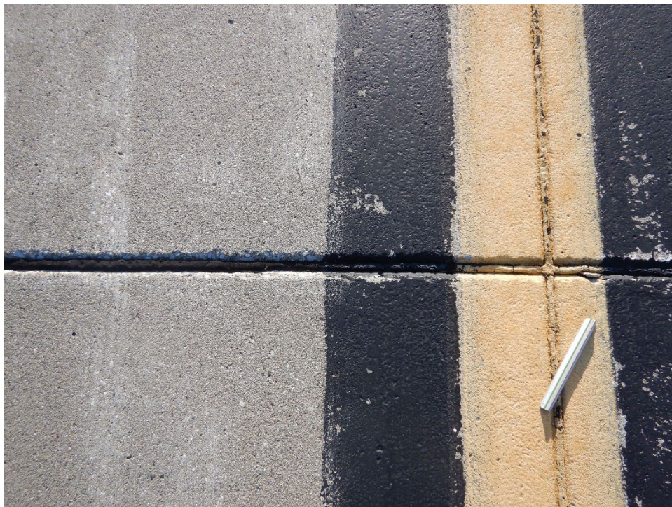
T07AM-01. Joint Seal Damage (Sample Unit No. 02).
