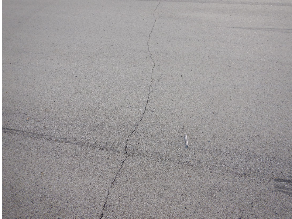
R12AT-01. L&T Cracking (Sample Unit No. 35).
