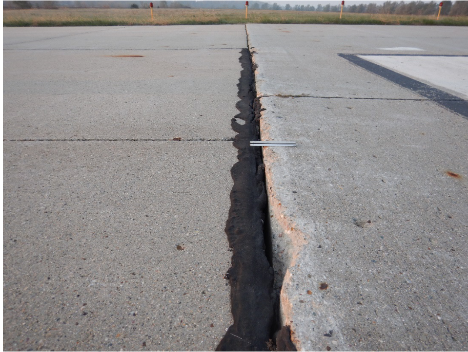
T03AT-01. Faulting (Additional Sample Unit No. 01).
