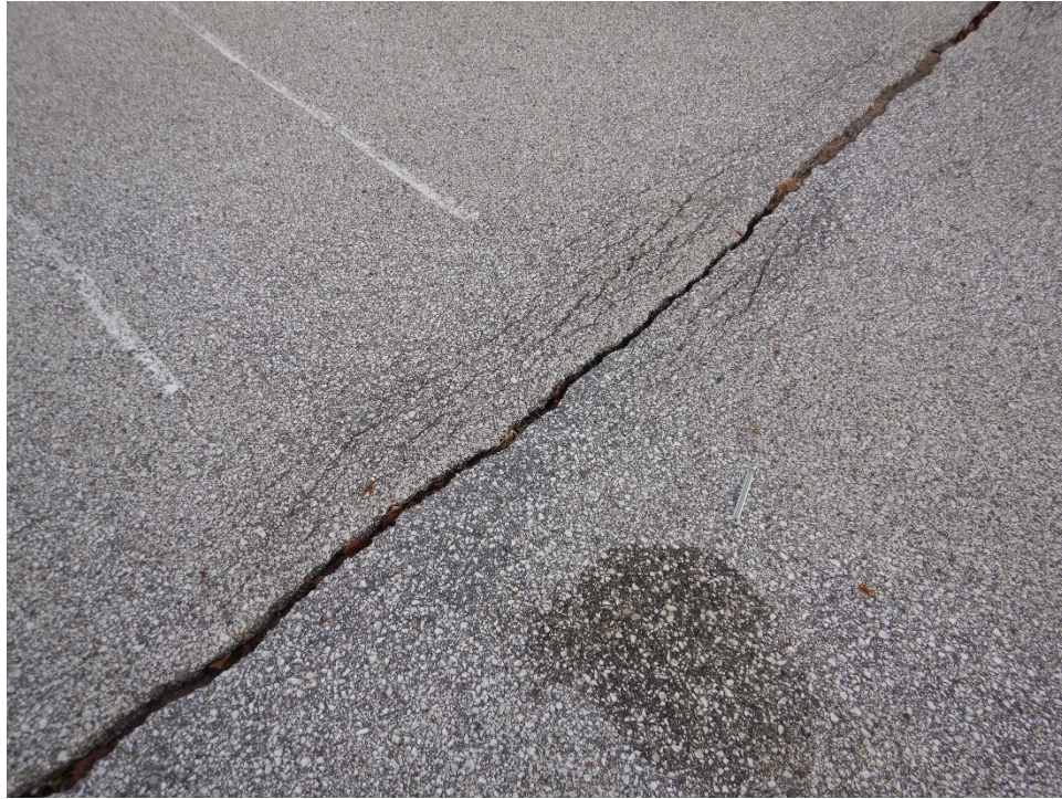
TH01AT-02. L&T Cracking (Sample Unit No. 01).
