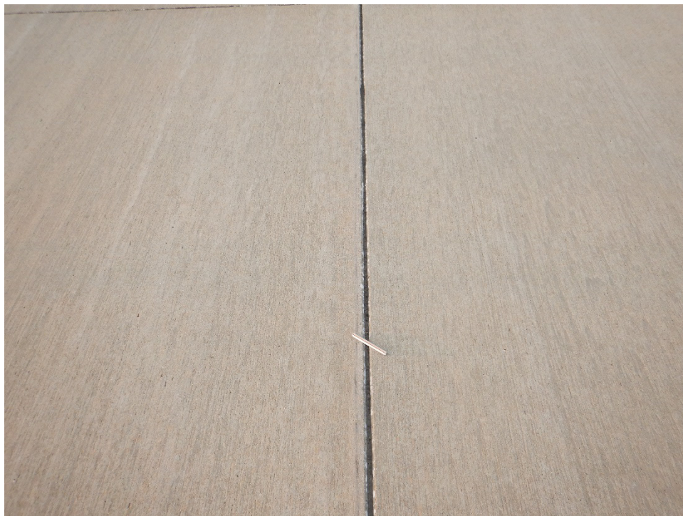
T04AT-01. Joint Seal Damage (Sample Unit No. 74).
