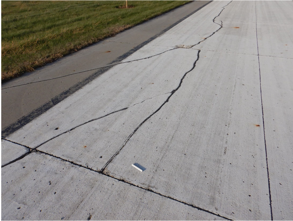
R02AT-01. Shattered Slab (Additional Sample Unit No. 81).
