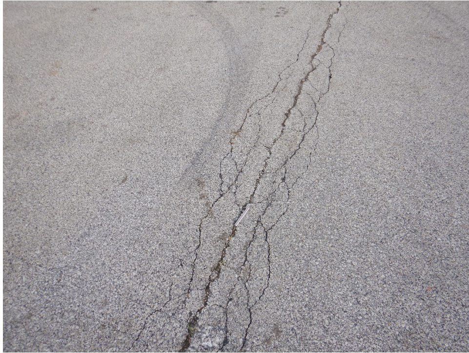
TH02AT-01. Alligator Cracking (Sample Unit No. 01).
