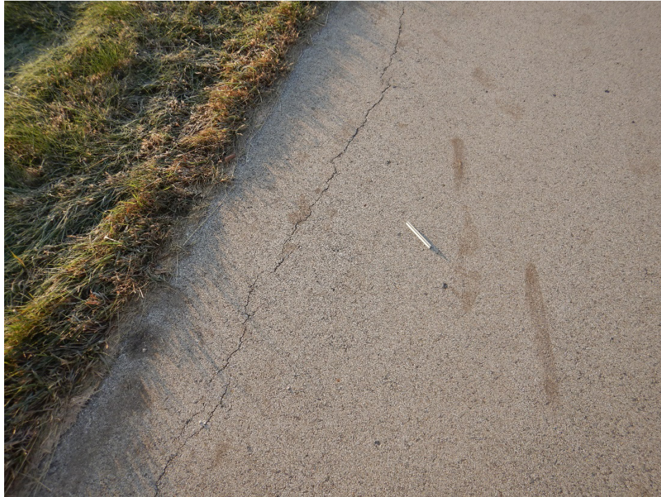
T01AT-01. L&T Cracking (Sample Unit No. 04).
