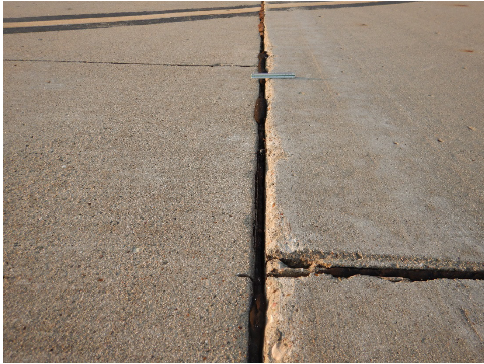
T02AT-01. Faulting (Sample Unit No. 03).
