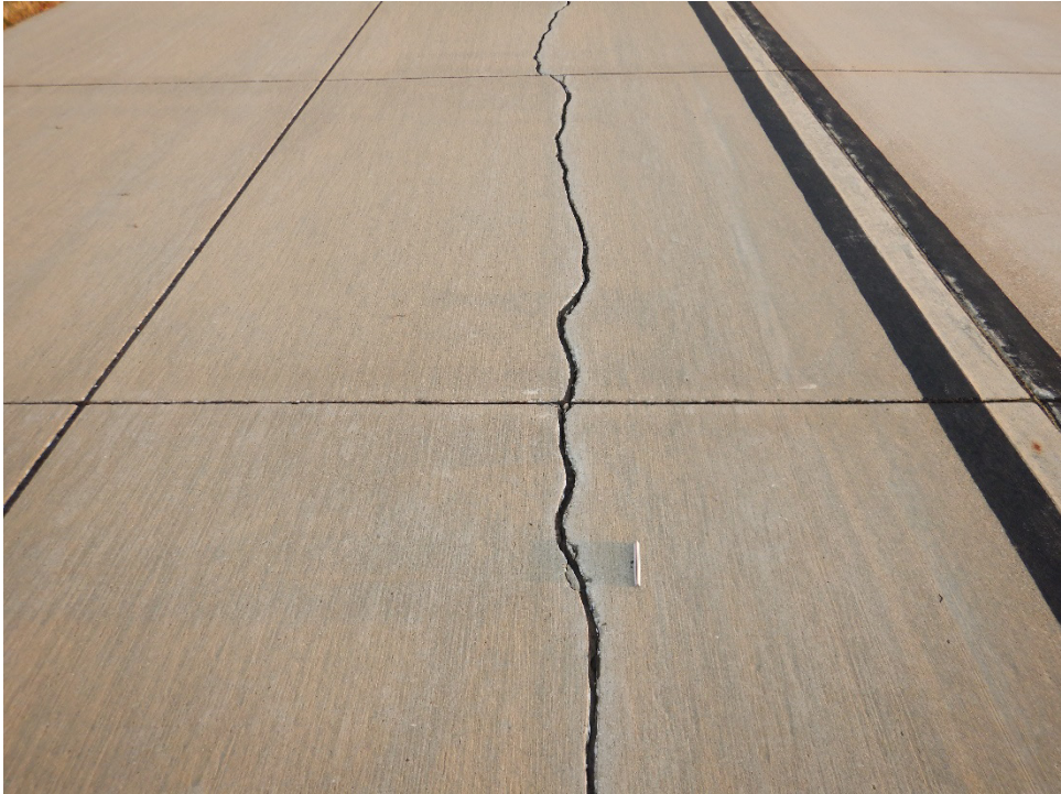
T04AT-01. LTD Cracking (Sample Unit No. 36).
