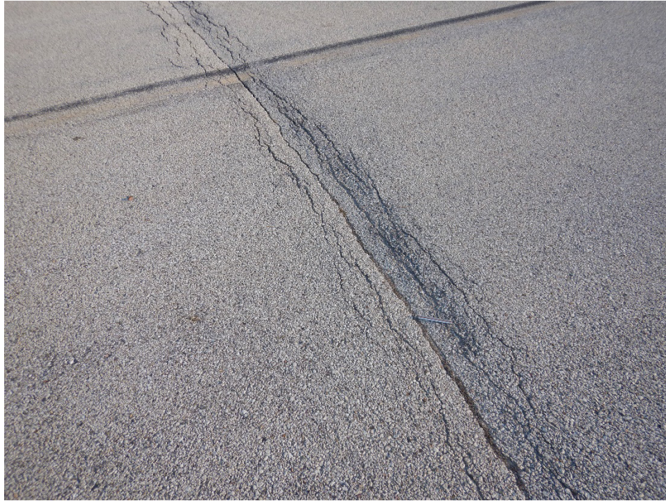
TH01AT-01. L&T Cracking (Sample Unit No. 01).
