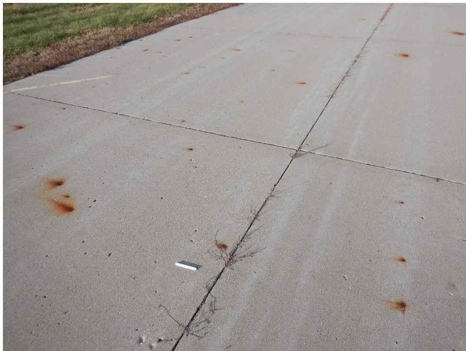
R02AT-01. Joint Seal Damage (Sample Unit No. 23).
