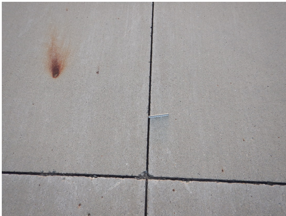
T03AT-01. Joint Seal Damage (Sample Unit No. 02).
