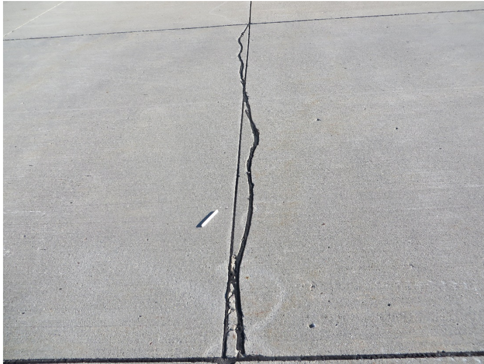
A02AU-02. Joint Spalling (Sample Unit No. 09).
