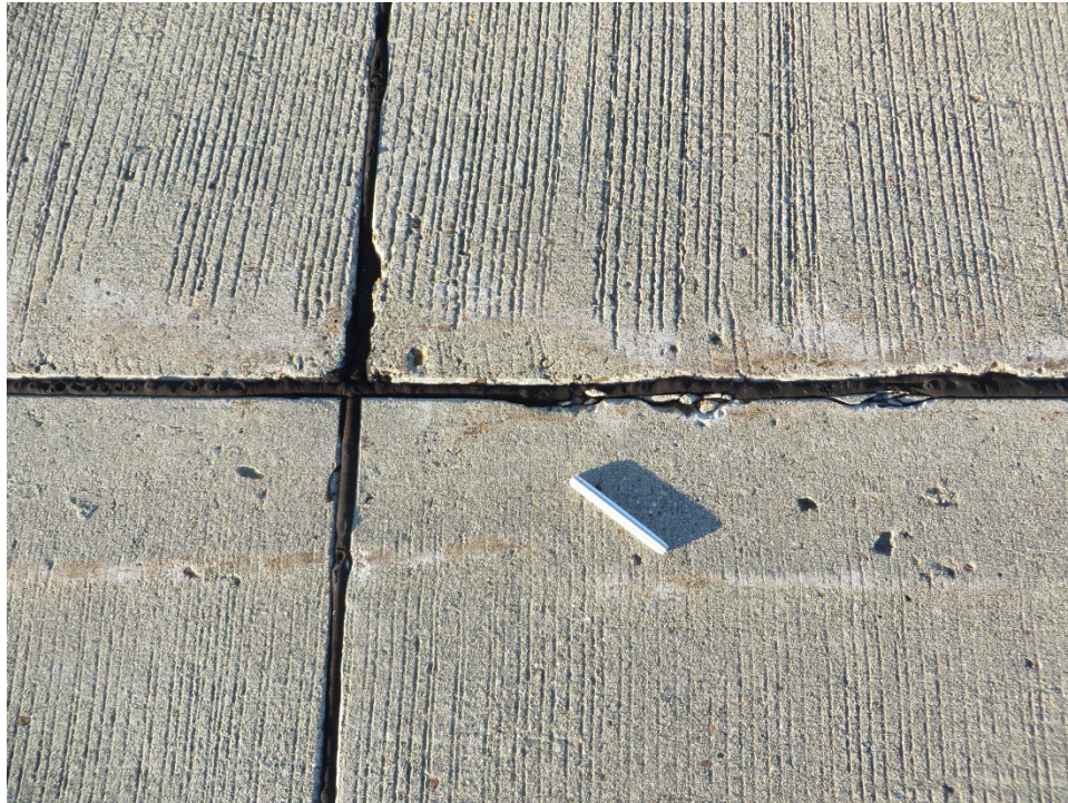
R14AU-02. Joint Seal Damage (Sample Unit No. 14).
