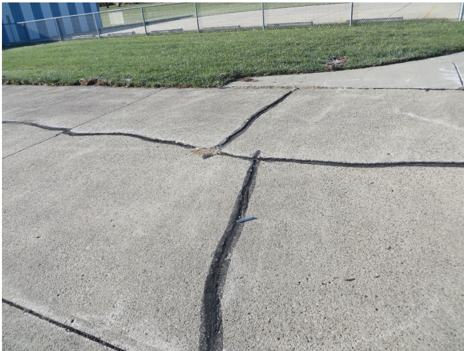
A01AU-01. Shattered Slab (Sample Unit No. 03).
