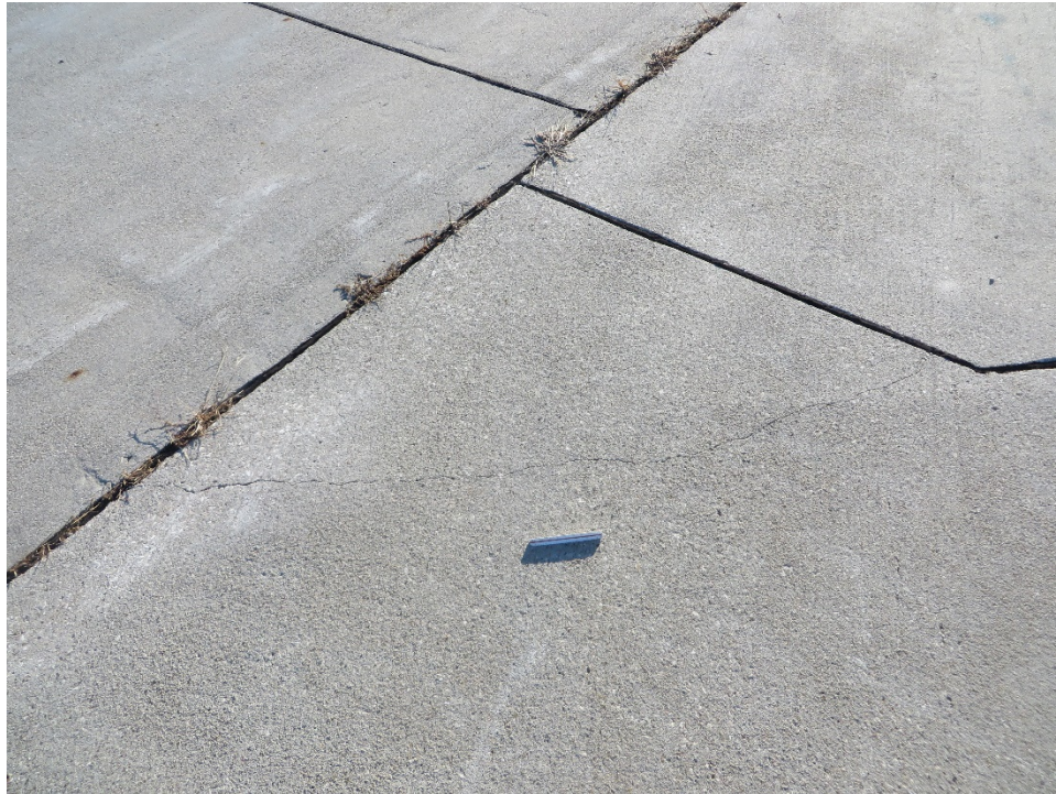
T01AU-03. Corner Break (Sample Unit No. 01).
