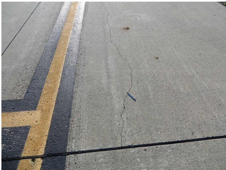
A02AU-02. LTD Cracking (Sample Unit No. 08).
