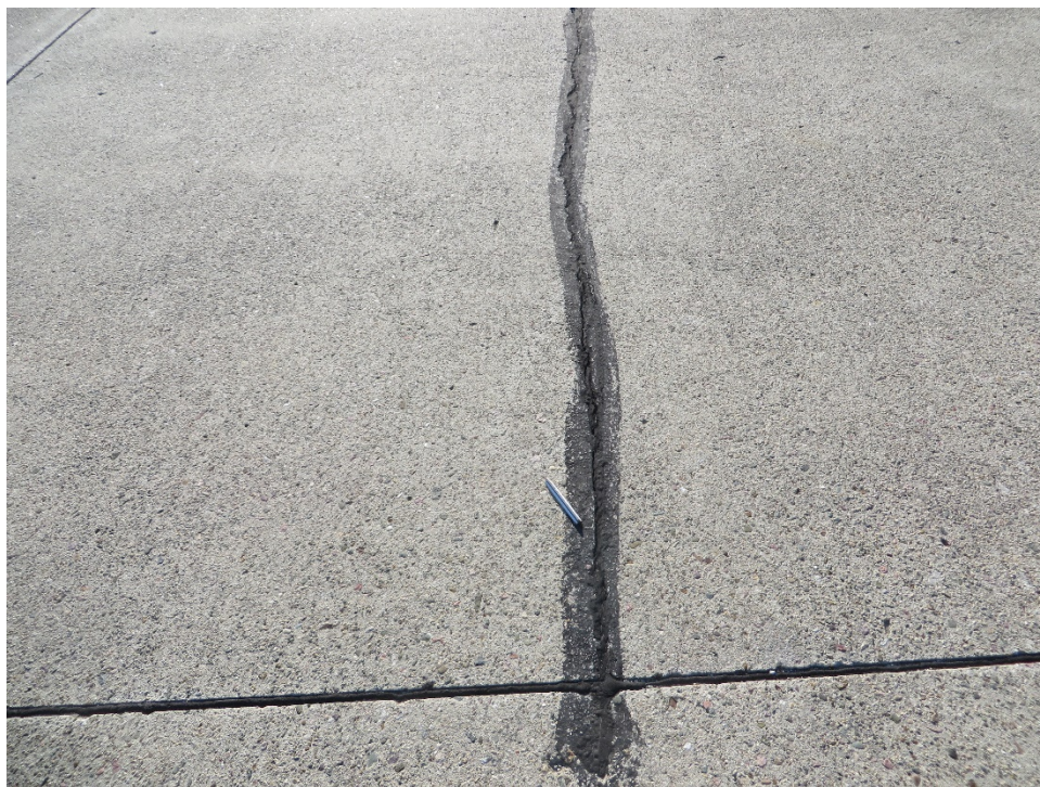
A01AU-01. LTD Cracking (Sample Unit No. 03).
