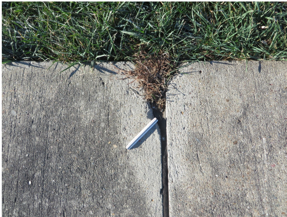
A02AU-01. Joint Spalling (Sample Unit No. 03).
