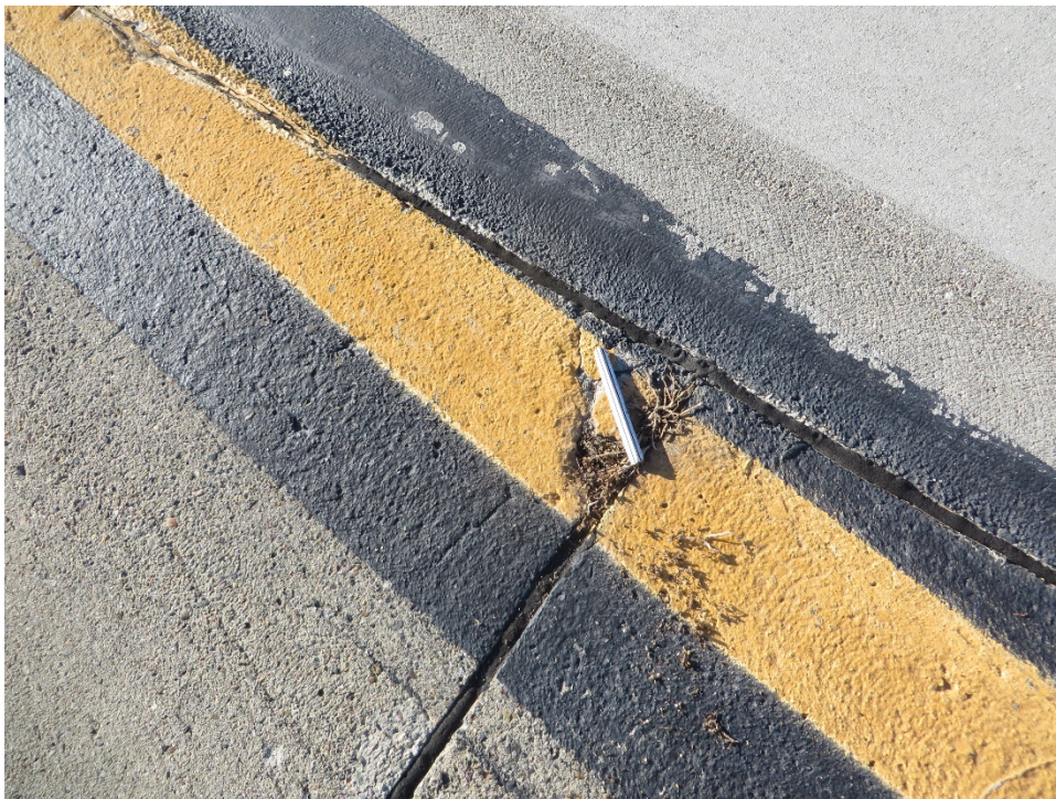
T01AU-02. Corner Spalling (Sample Unit No. 01).
