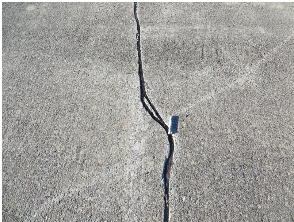
T01AU-01. LTD Cracking (Sample Unit No. 01).
