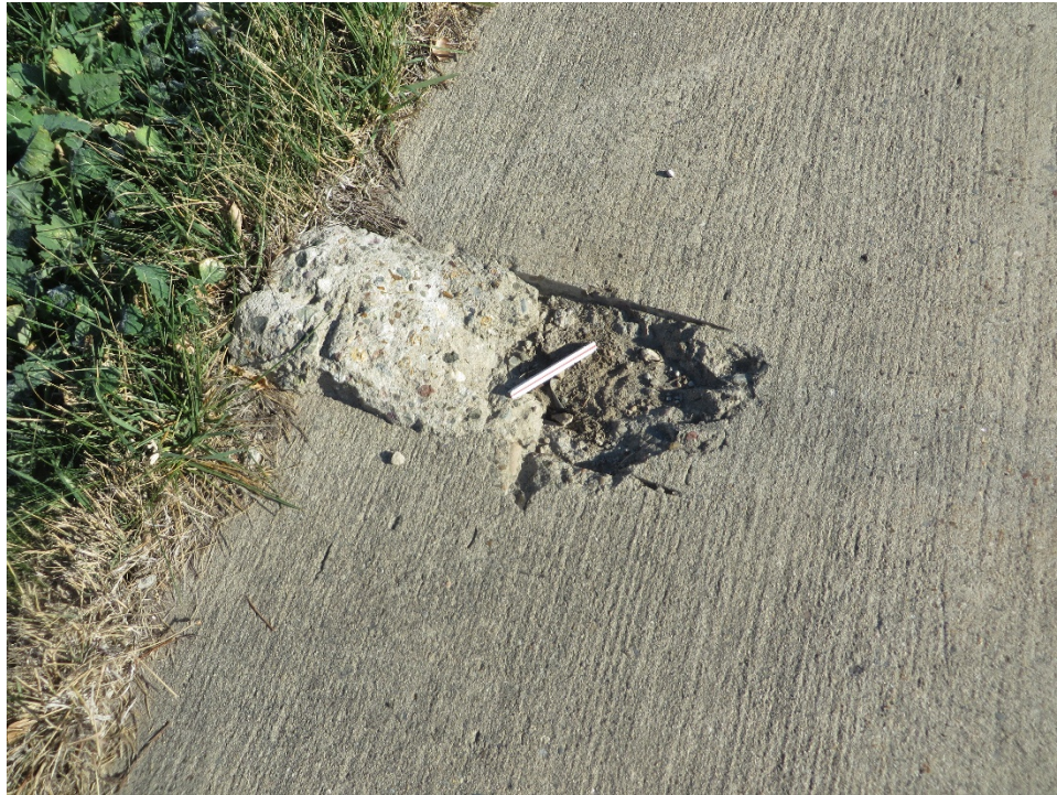
A02AU-01. Small Patching (Sample Unit No. 02).
