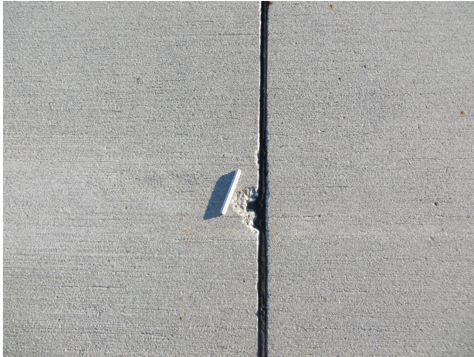
R14AU-01. Joint Spalling (Sample Unit No. 65).
