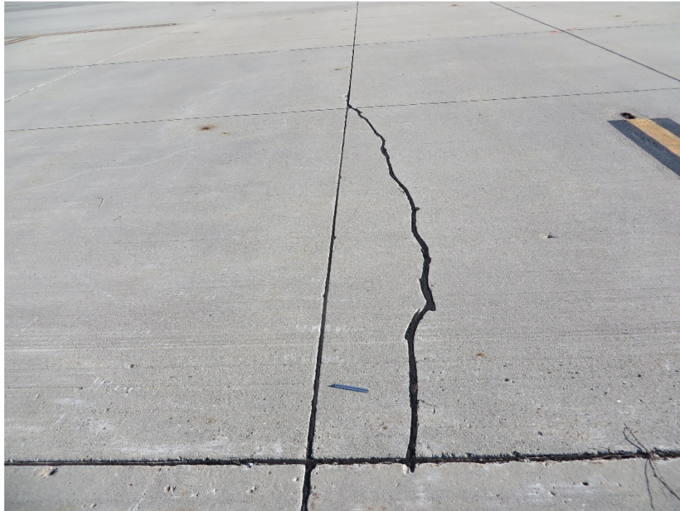
A02AU-02. LTD Cracking (Sample Unit No. 09).
