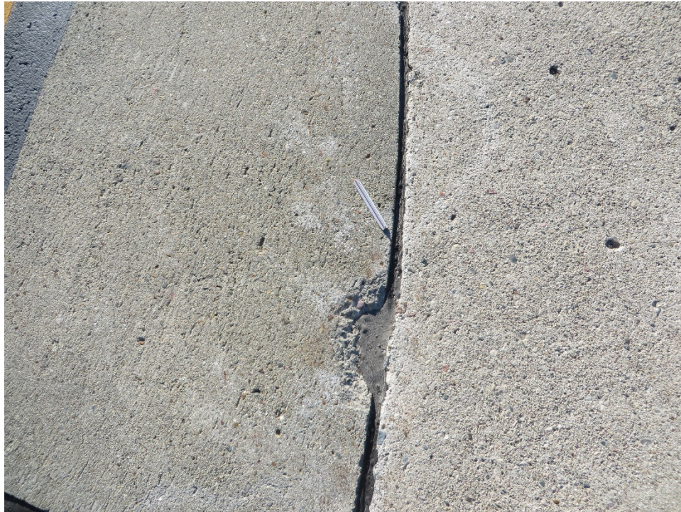
T01AU-02. Joint Spalling (Sample Unit No. 01).
