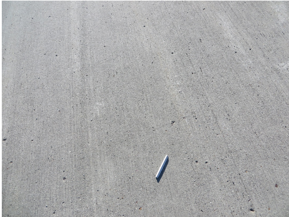
T02AU-01. Shrinkage Cracking (Sample Unit No. 12).
