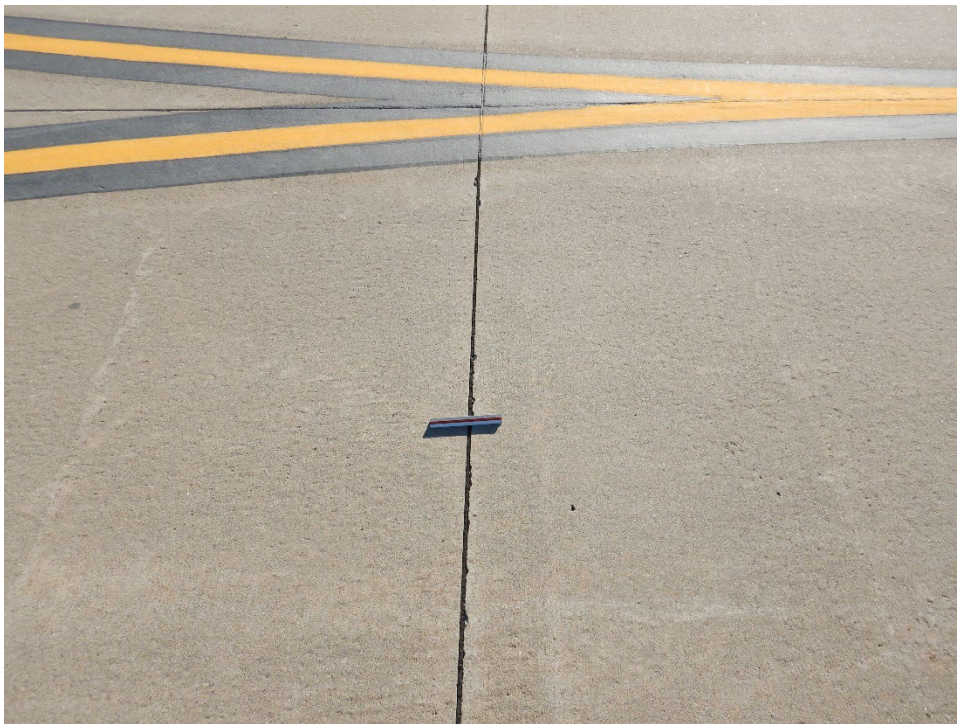
T01BL-01. Joint Seal Damage (Sample Unit No. 03).
