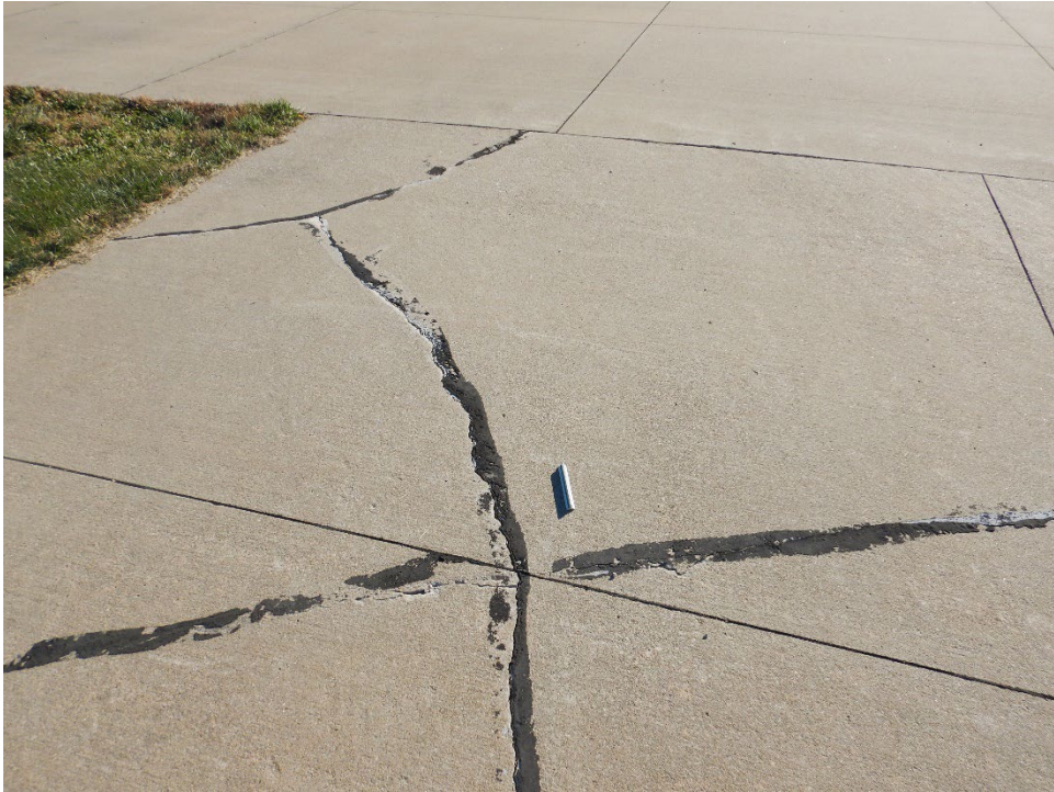
TH01BL-03. Shattered Slab (Sample Unit No. 01).
