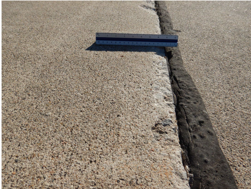
R18BL-03. Faulting (Sample Unit No. 09).
