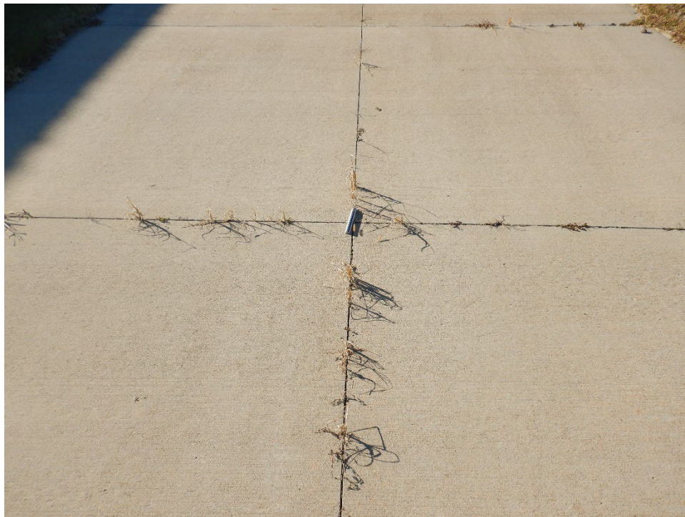
TH01BL-02. Joint Seal Damage (Sample Unit No. 01).
