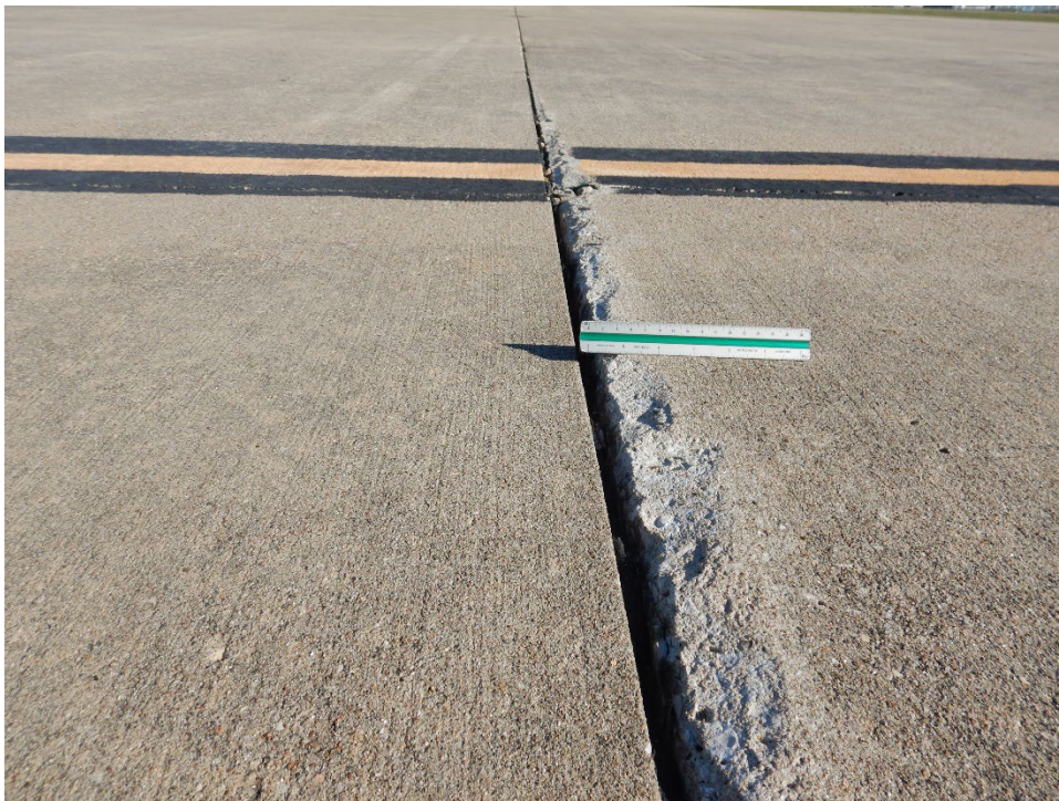
A01BL-02. Faulting (Sample Unit No. 02).
