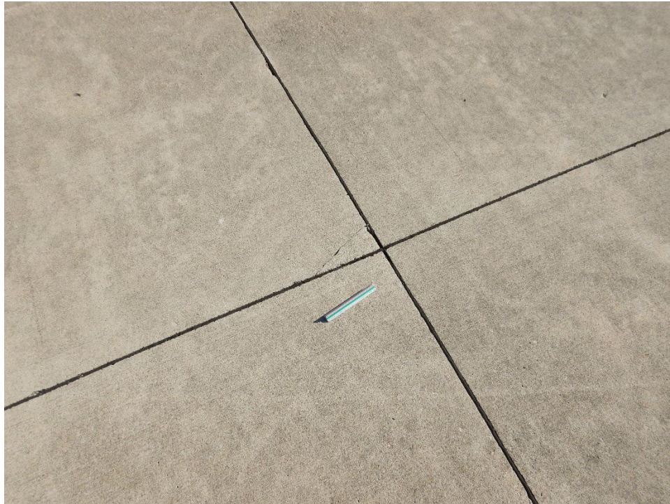
R18BL-01. Corner Spalling (Sample Unit No. 01).
