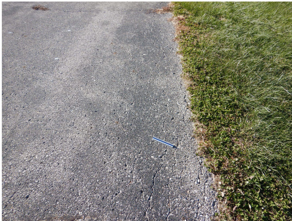
TH01BL-01. Alligator Cracking (Sample Unit No. 01).
