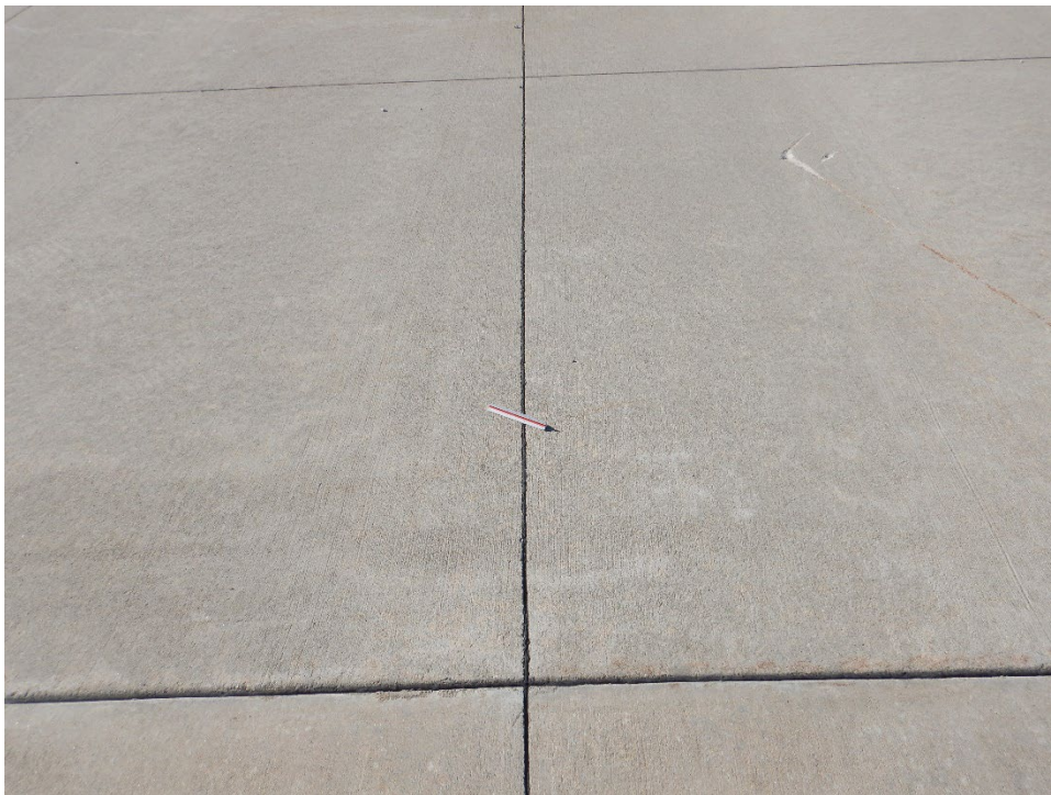
A01BL-01. Joint Seal Damage (Sample Unit No. 10).
