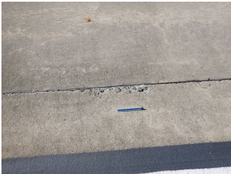
R18BL-03. Joint Spalling (Sample Unit No. 03).
