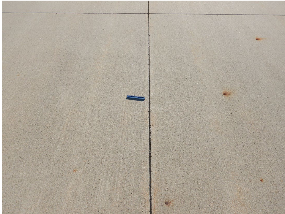
R18BL-02. Joint Seal Damage (Sample Unit No. 13).
