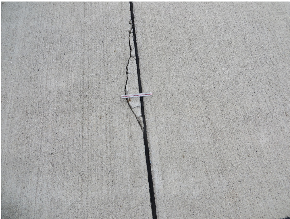
T01BO-04. Joint Spalling (Sample Unit No. 04).
