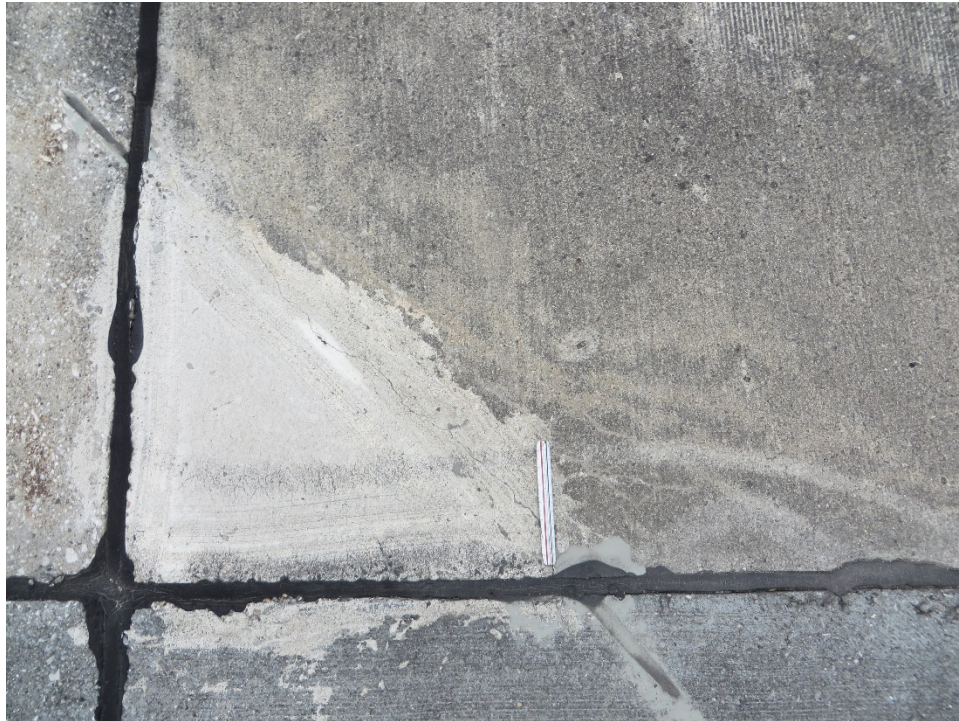
R15BO-02. Small Patching (Sample Unit No. 01).
