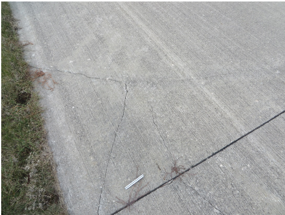
T01BO-02. Shattered Slab (Sample Unit No. 33).
