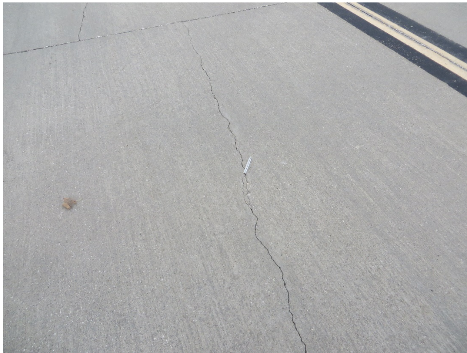
TH01BO-03. LTD Cracking (Sample Unit No. 10).
