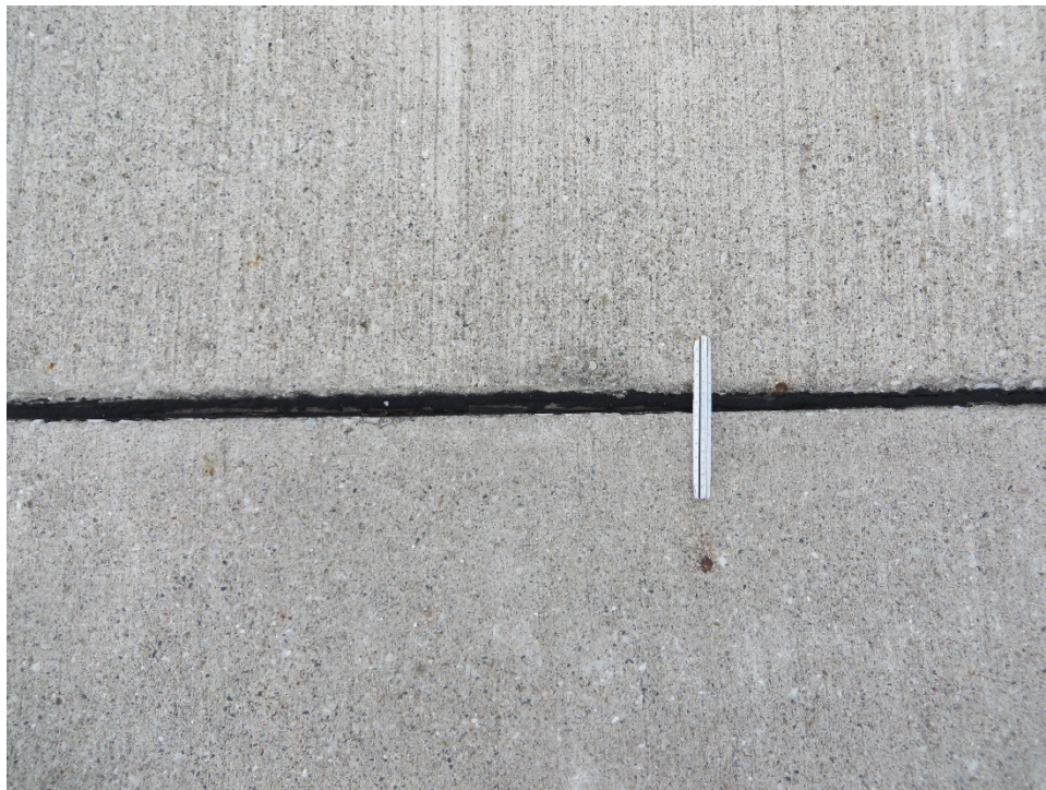
T01BO-05. Joint Seal Damage (Sample Unit No. 03).
