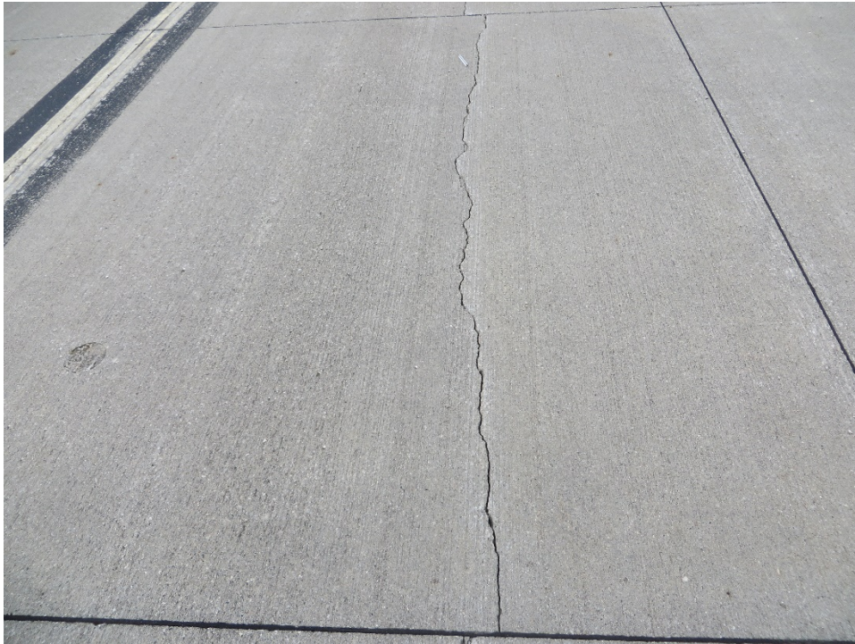
T01BO-02. LTD Cracking (Sample Unit No. 86).
