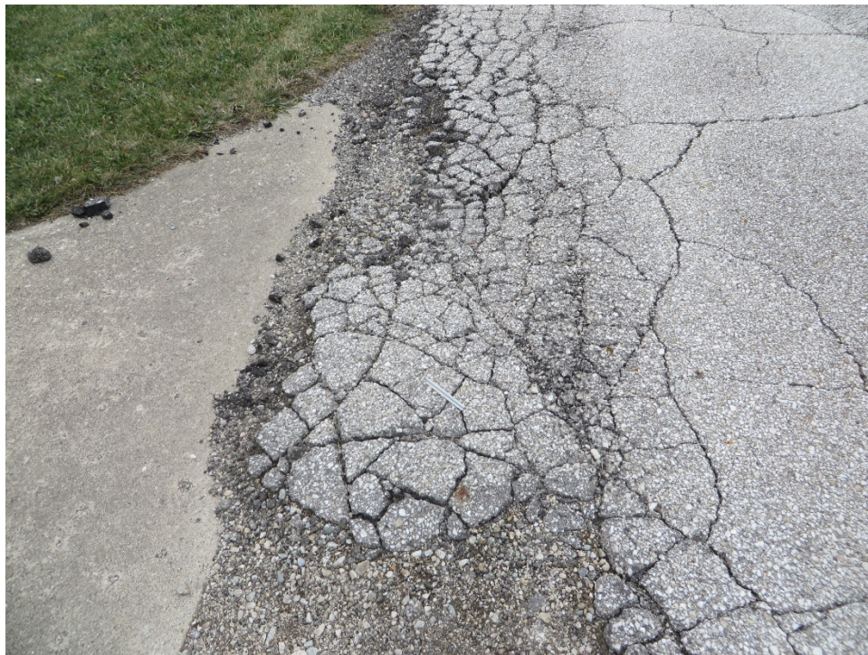
TH02BO-02. Alligator Cracking (Sample Unit No. 03) (2).
