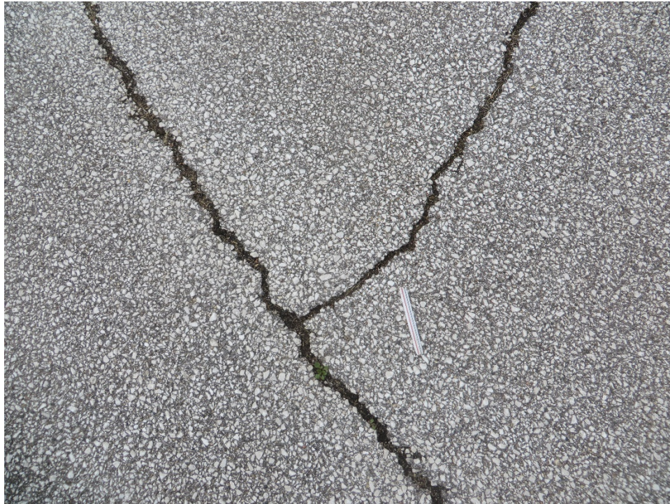
TH01BO-01. L&T Cracking (Sample Unit No. 02).
