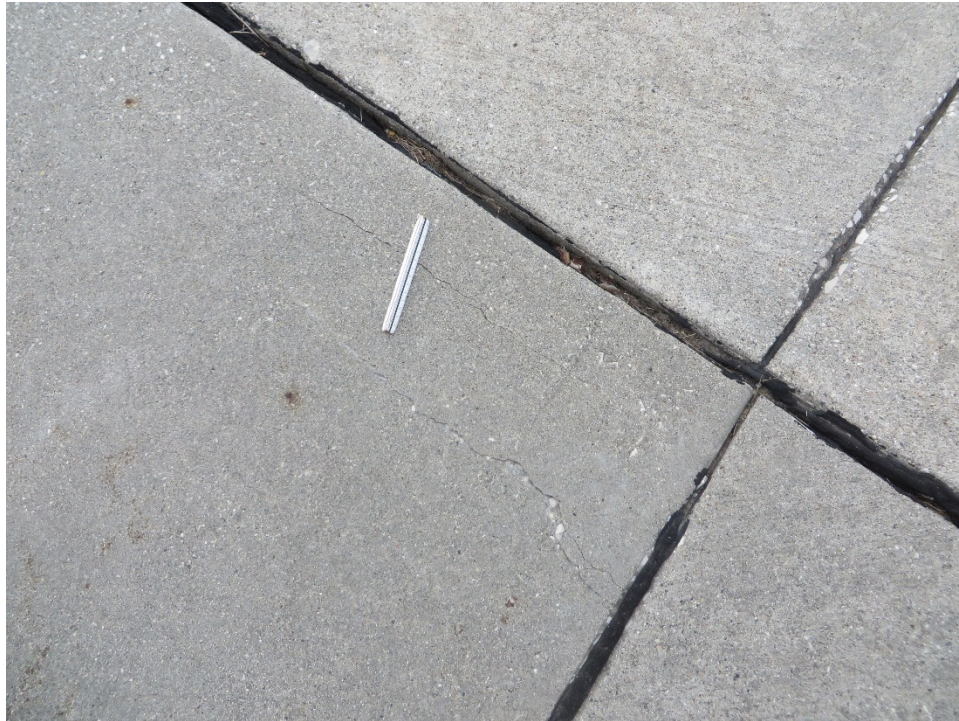
A01BO-03. Joint Spalling (Sample Unit No. 01).
