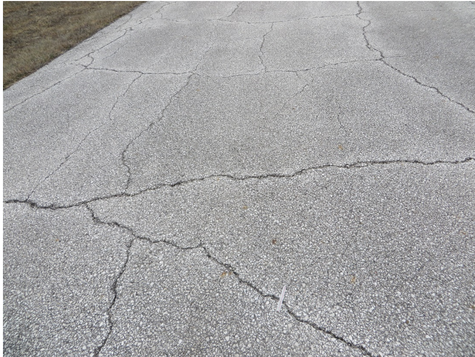
TH02BO-02. Block Cracking (Sample Unit No. 03).
