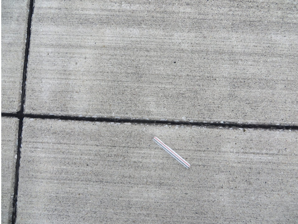
T01BO-06. Joint Seal Damage (Sample Unit No. 01).
