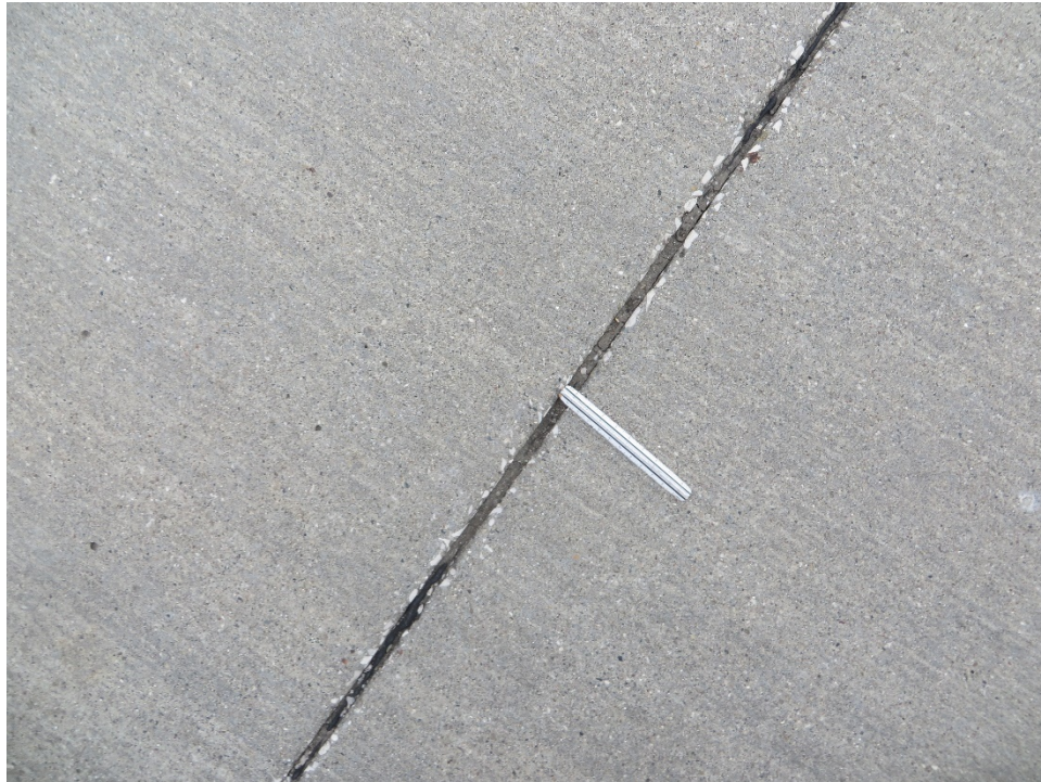
TH01BO-03. Joint Seal Damage (Sample Unit No. 10).
