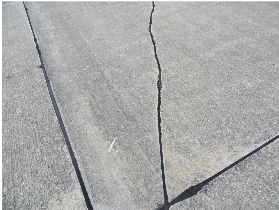
R15BO-02. LTD Cracking (Sample Unit No. 16).
