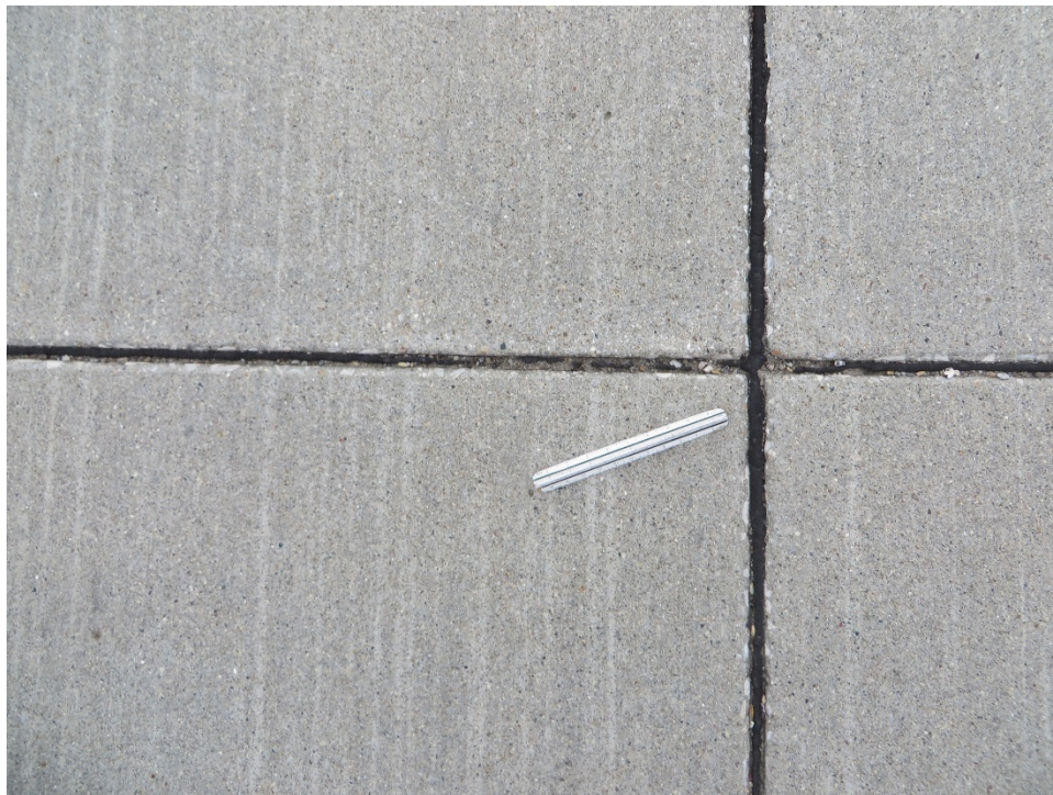
A01BO-01. Joint Seal Damage (Sample Unit No. 15).
