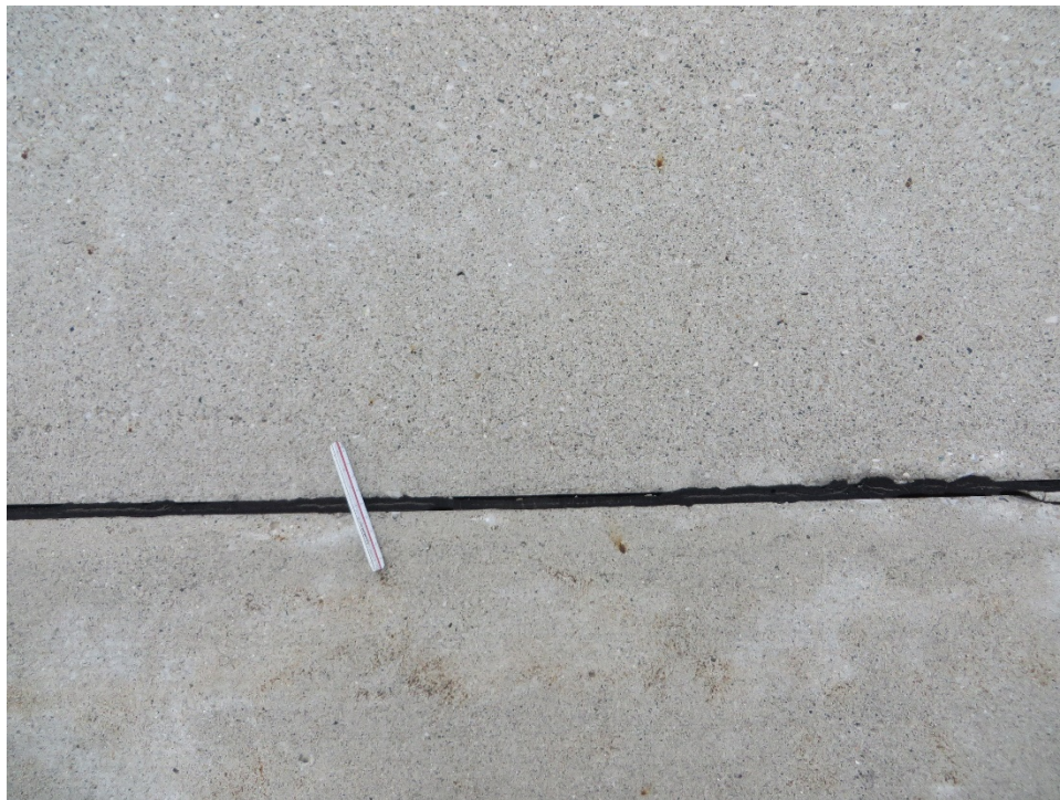
R15BO-01. Joint Seal Damage (Sample Unit No. 01).
