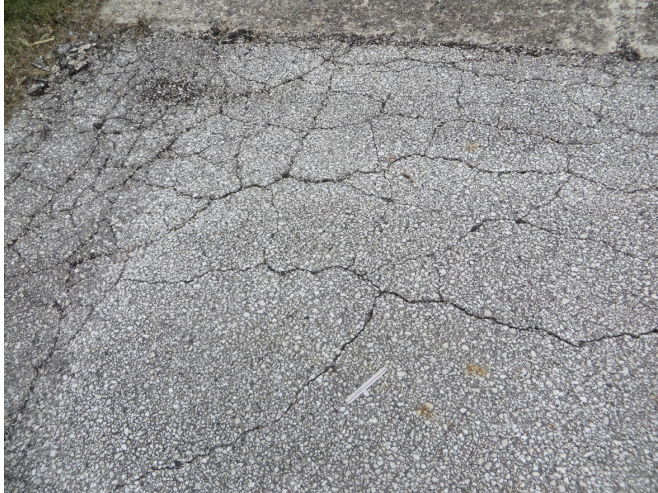
TH02BO-02. Alligator Cracking (Sample Unit No. 03) (1).
