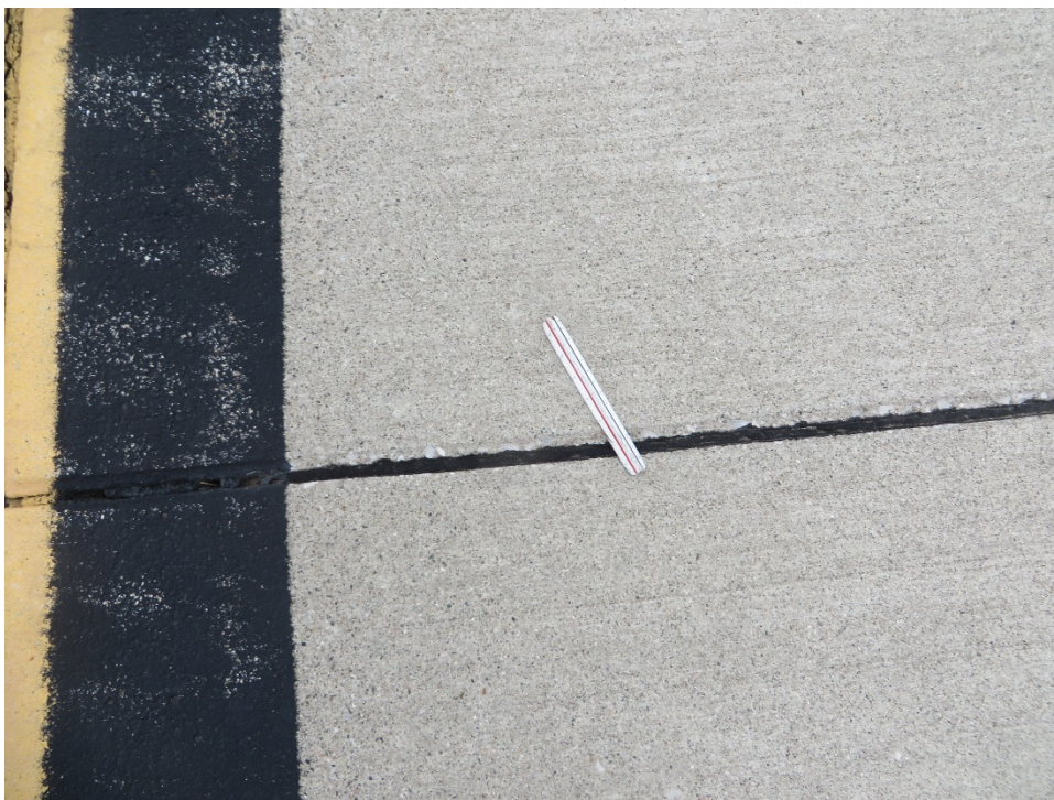
T01BO-03. Joint Seal Damage (Sample Unit No. 02).
