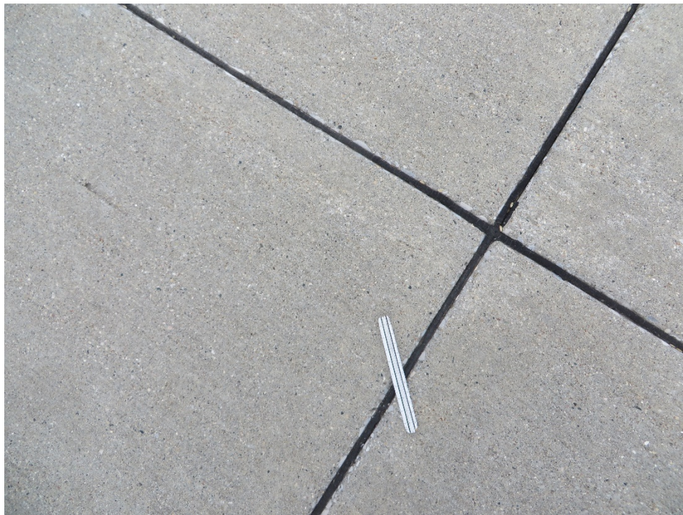
A01BO-02. Joint Seal Damage (Sample Unit No. 07).
