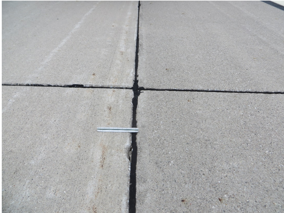
R15BO-01. Faulting (Sample Unit No. 30).
