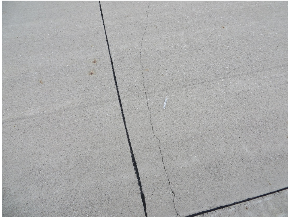
R15BO-01. LTD Cracking (Sample Unit No. 59).
