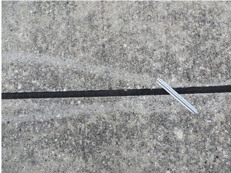
R15BO-02. Joint Seal Damage (Sample Unit No. 07).
