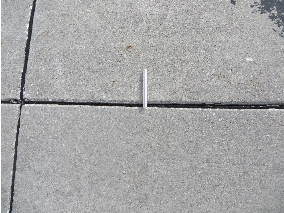
A01BO-03. Joint Seal Damage (Sample Unit No. 02).
