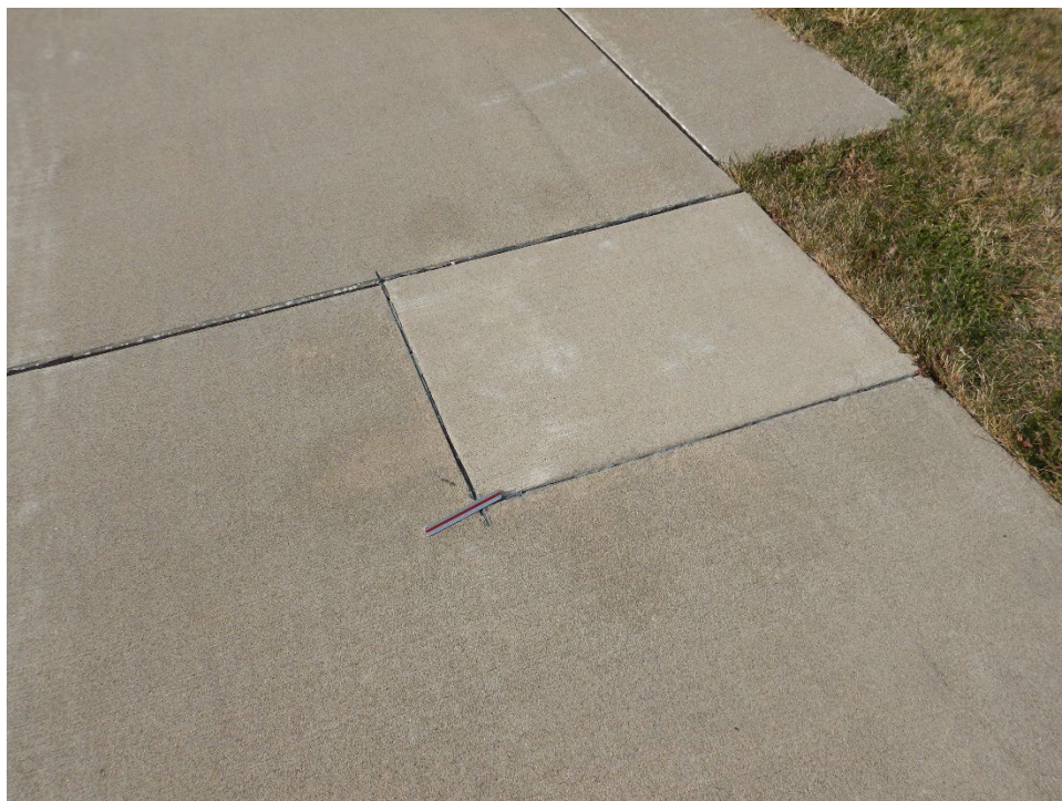
TH01BR-02. Large Patching (Sample Unit No. 14).
