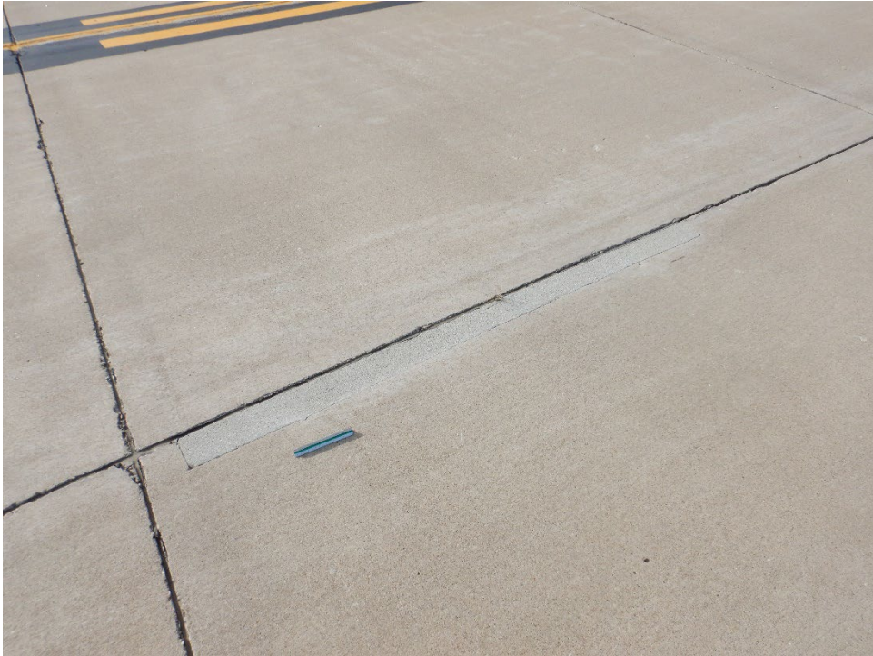
T01BR-02. Small Patching (Sample Unit No. 02).
