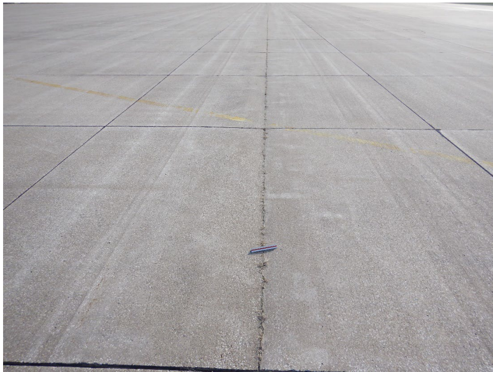
A01BR-02. LTD Cracking (Sample Unit No. 05).
