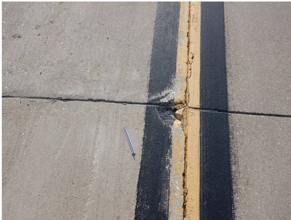
T02BR-02. Corner Spalling (Sample Unit No. 63).
