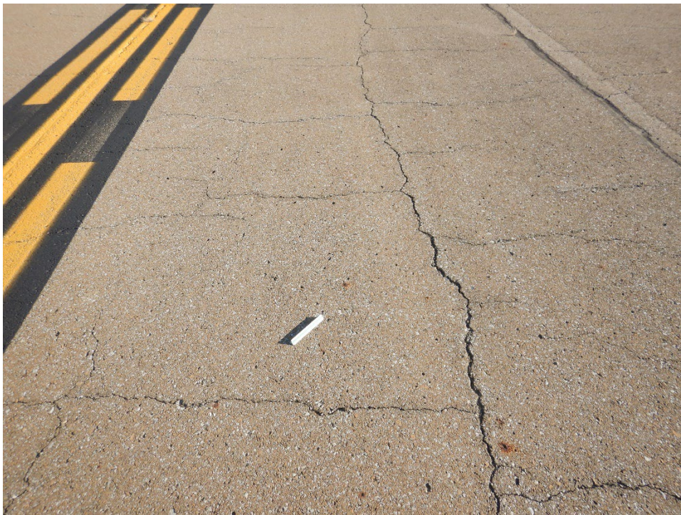
T01BR-01. Block Cracking (Sample Unit No. 27).
