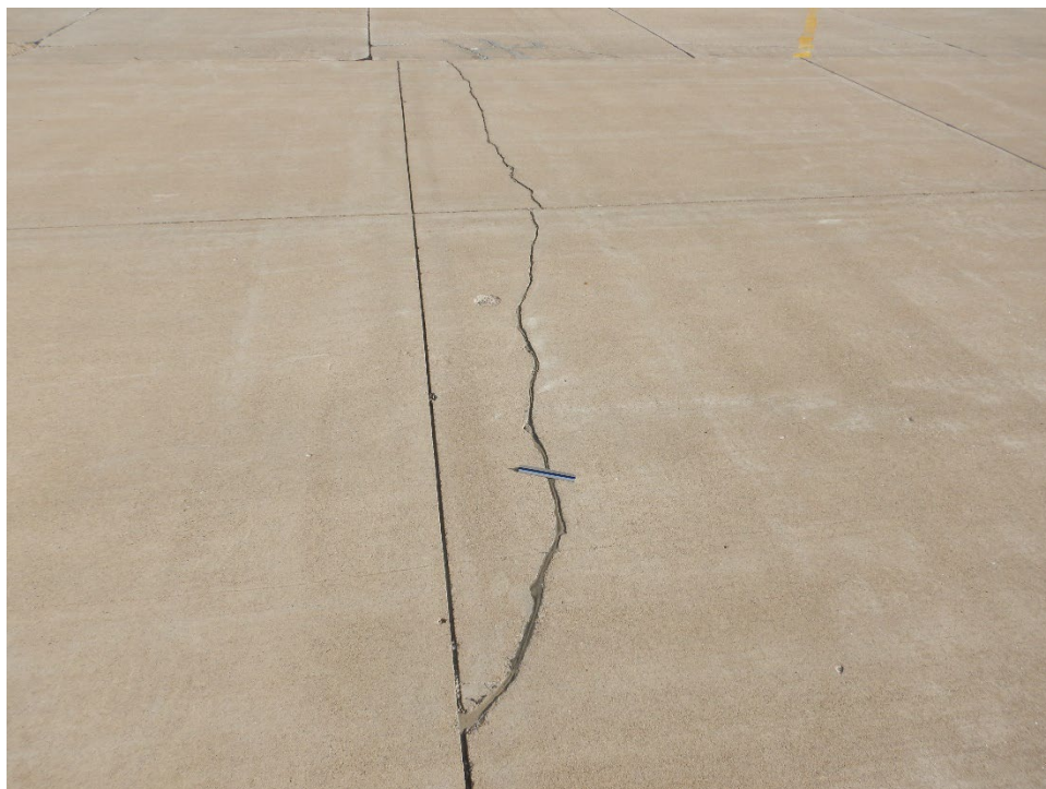
T03BR-03. LTD Cracking (Sample Unit No. 04).
