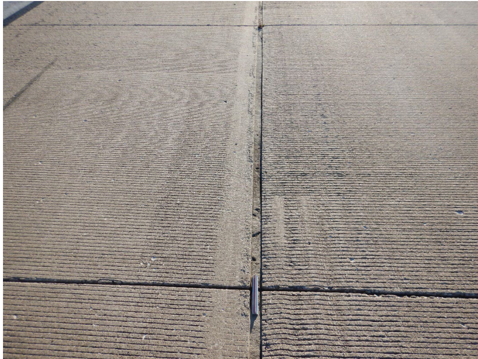
R12BR-01. Joint Seal Damage (Sample Unit No. 153).
