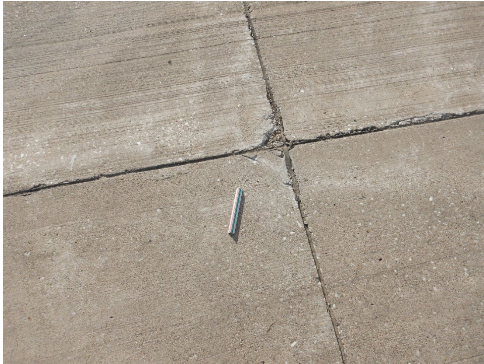
T06BR-01. Corner Spalling (Sample Unit No. 04).
