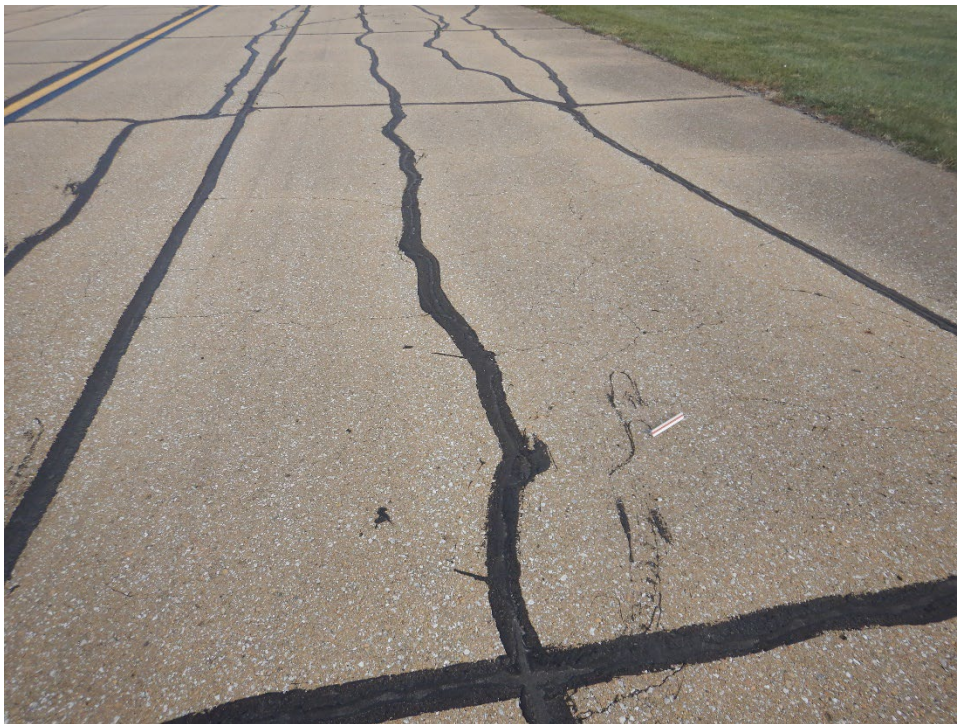
T03BR-04. Block Cracking (Sample Unit No. 02).
