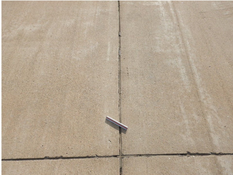
T03BR-03. Joint Seal Damage (Sample Unit No. 10).
