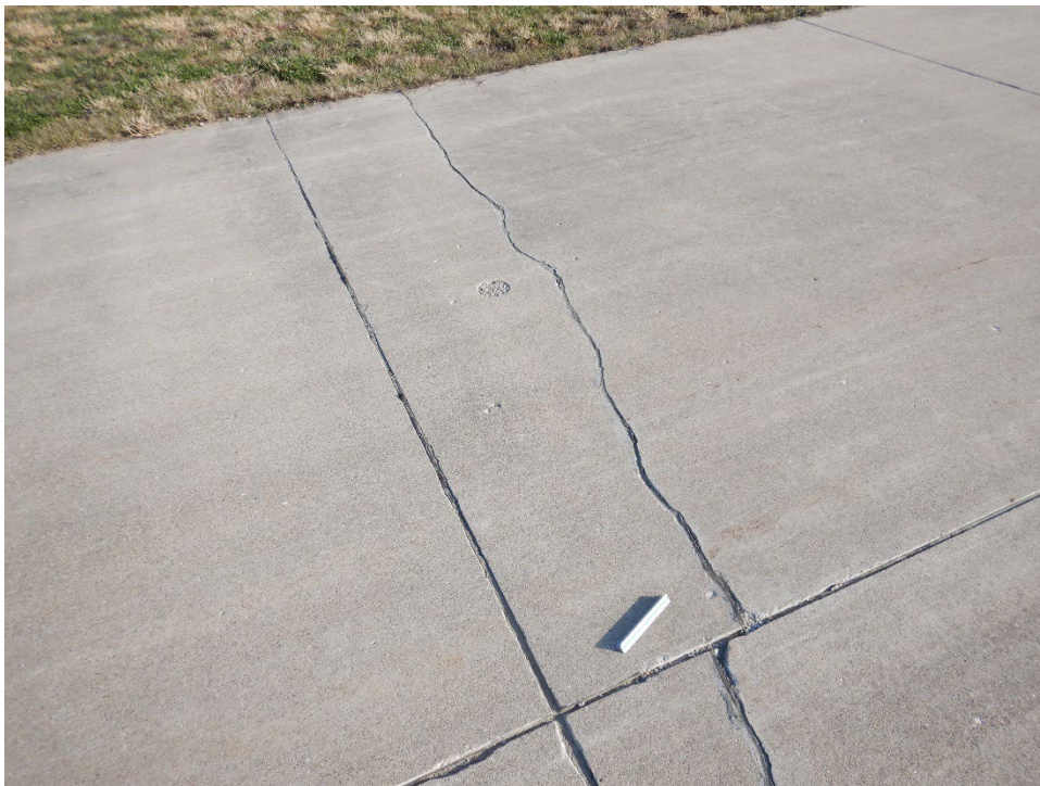
T02BR-01. LTD Cracking (Sample Unit No. 01).
