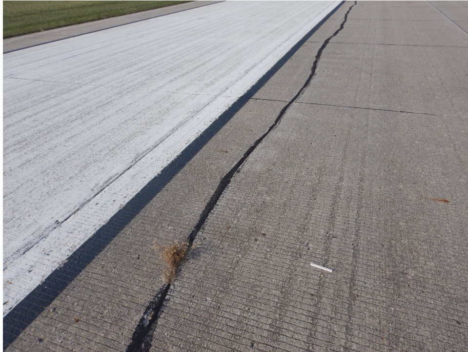
R13CA-03. LTD Cracking (Sample Unit No. 09).
