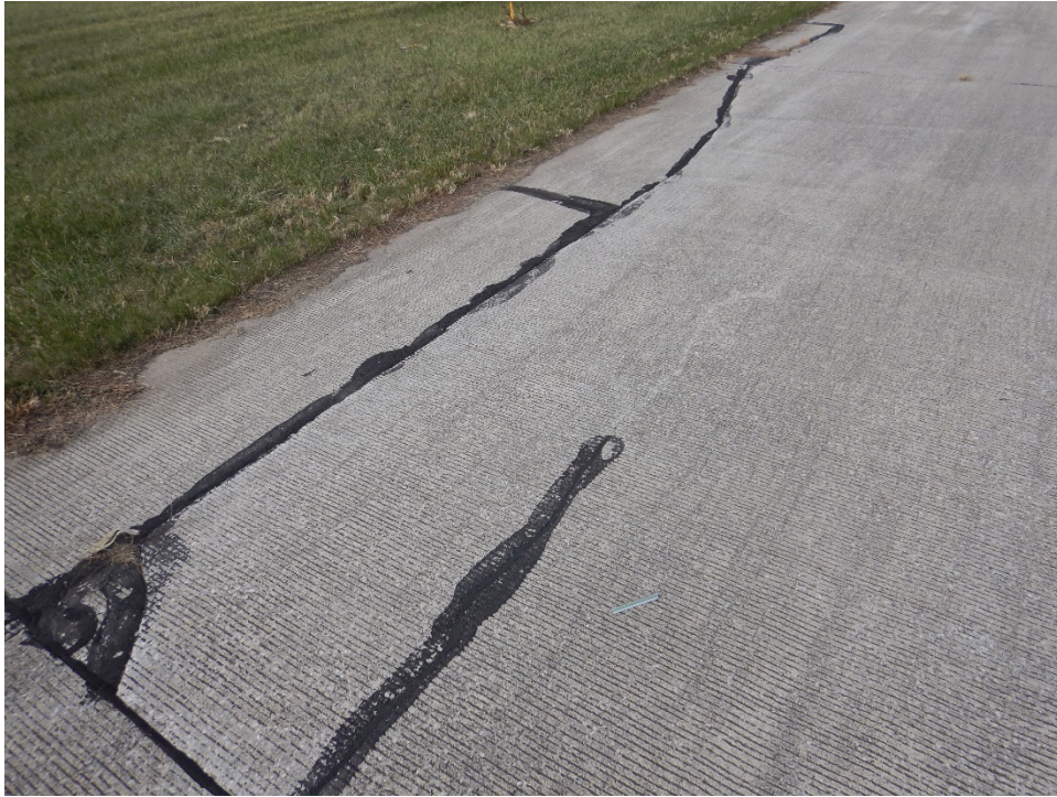
R13CA-05. LTD Cracking (Sample Unit No. 10).
