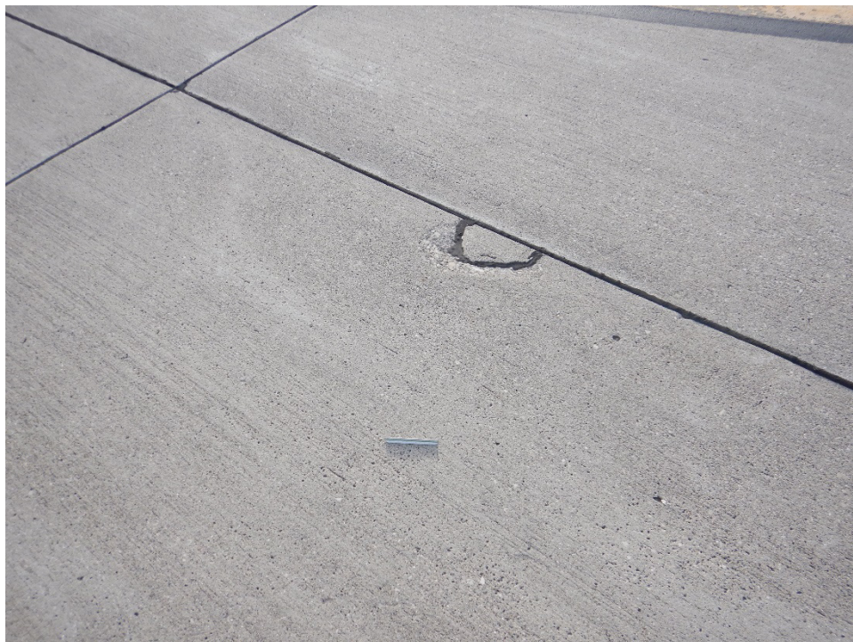
A01CA-01. Joint Spalling (Sample Unit No. 10).
