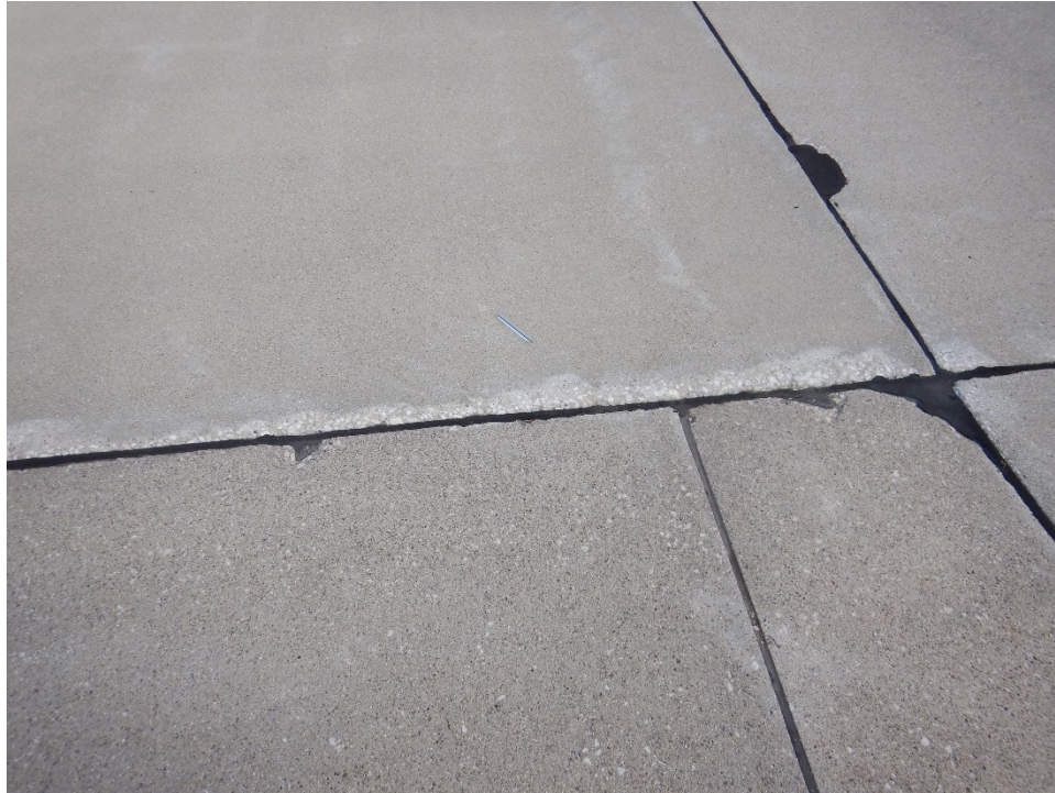
TH01CA-01. Faulting (Sample Unit No. 03).
