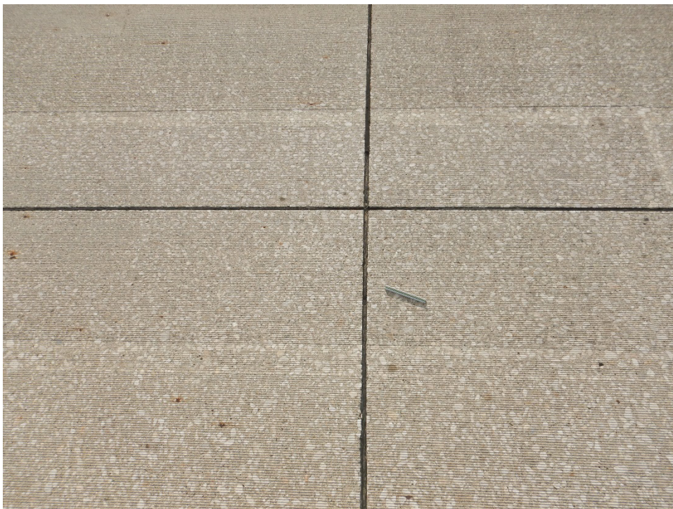
T06CA-01. Joint Seal Damage (Sample Unit No. 64).
