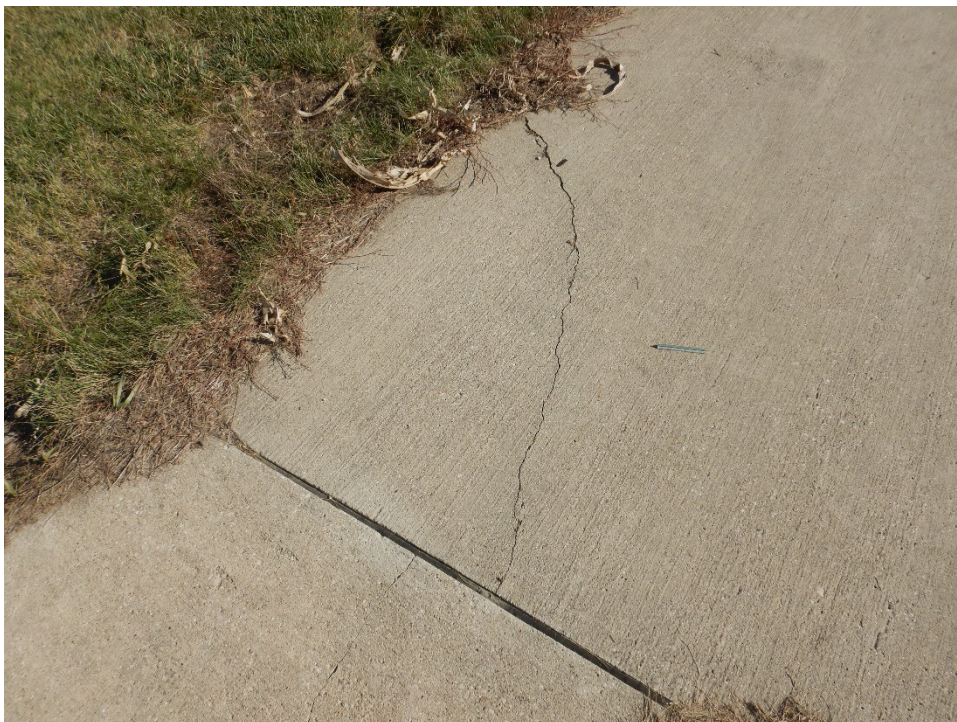
T05CA-01. Corner Break (Sample Unit No. 03).
