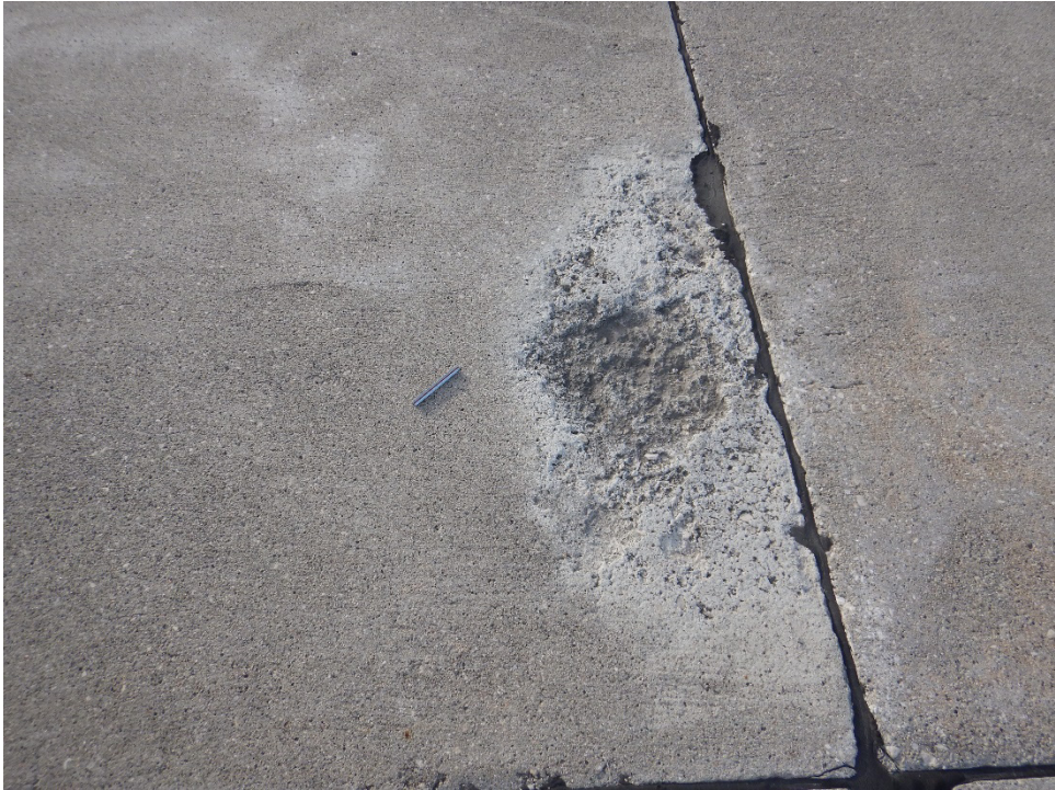
A01CA-01. Scaling (Additional Sample Unit No. 20).
