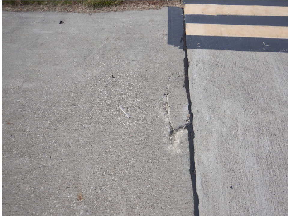
T06CA-01. Joint Spalling (Additional Sample Unit No. 01).
