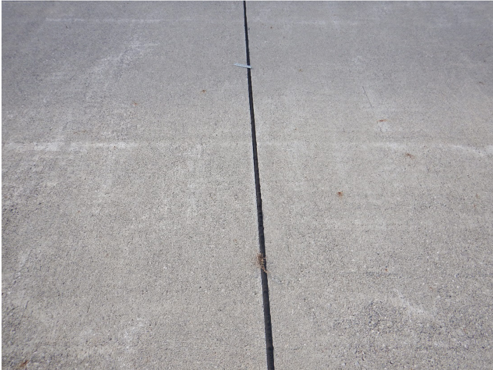
TH02CA-03. Joint Seal Damage (Sample Unit No. 01).
