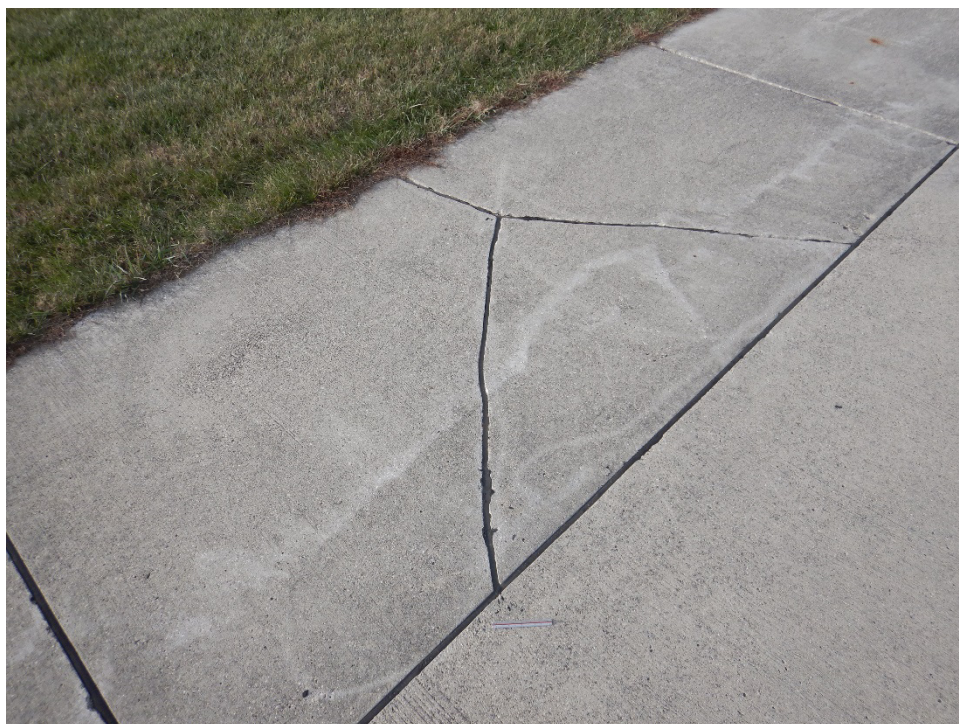
T04CA-01. LTD Cracking (Sample Unit No. 15).
