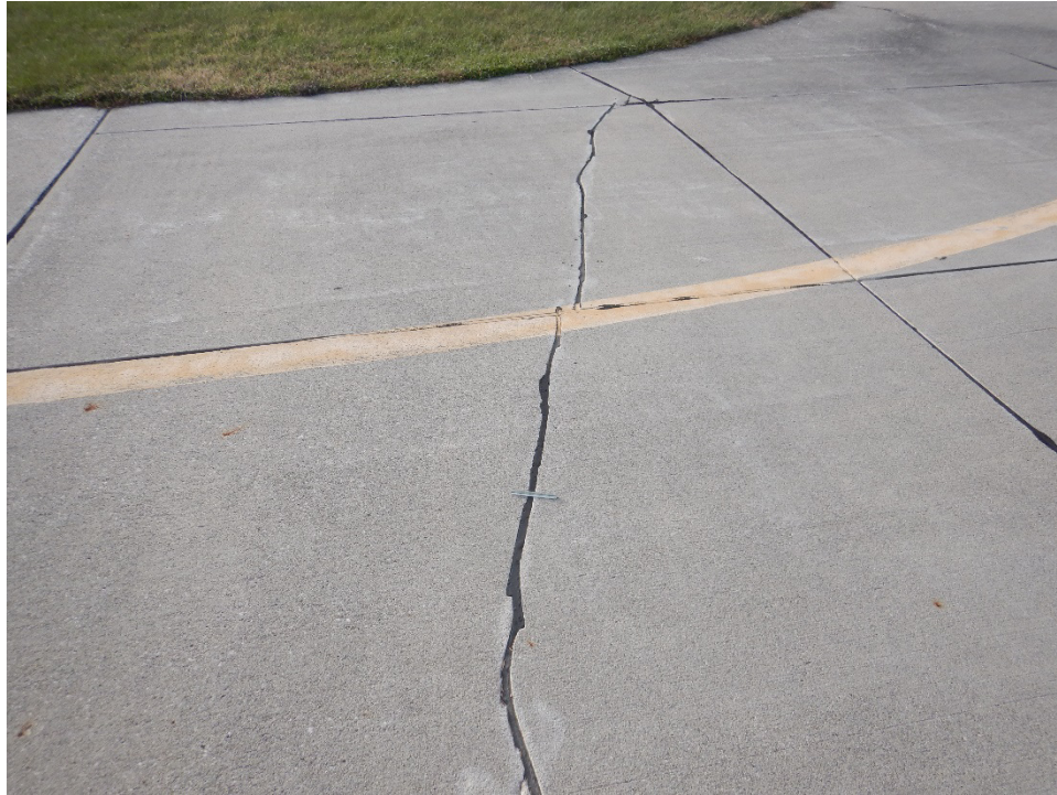
TH02CA-02. LTD Cracking (Sample Unit No. 01).
