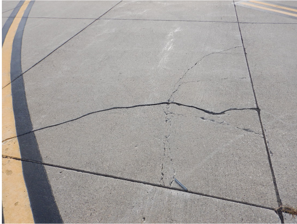
T02CA-01. Shattered Slab (Sample Unit No. 07).
