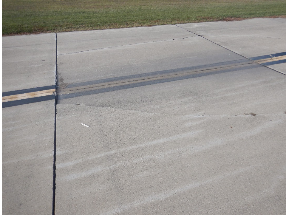
T04CA-01. Faulting (Additional Sample Unit No. 05).
