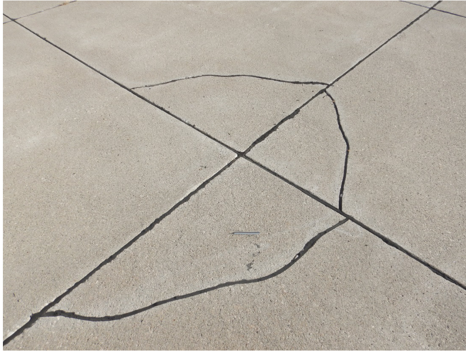
T01CA-01. Corner Break (Sample Unit No. 01).
