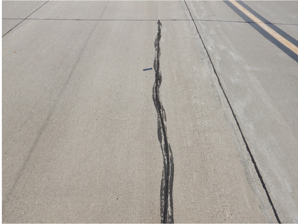
R03CA-02. LTD Cracking (Sample Unit No. 08).
