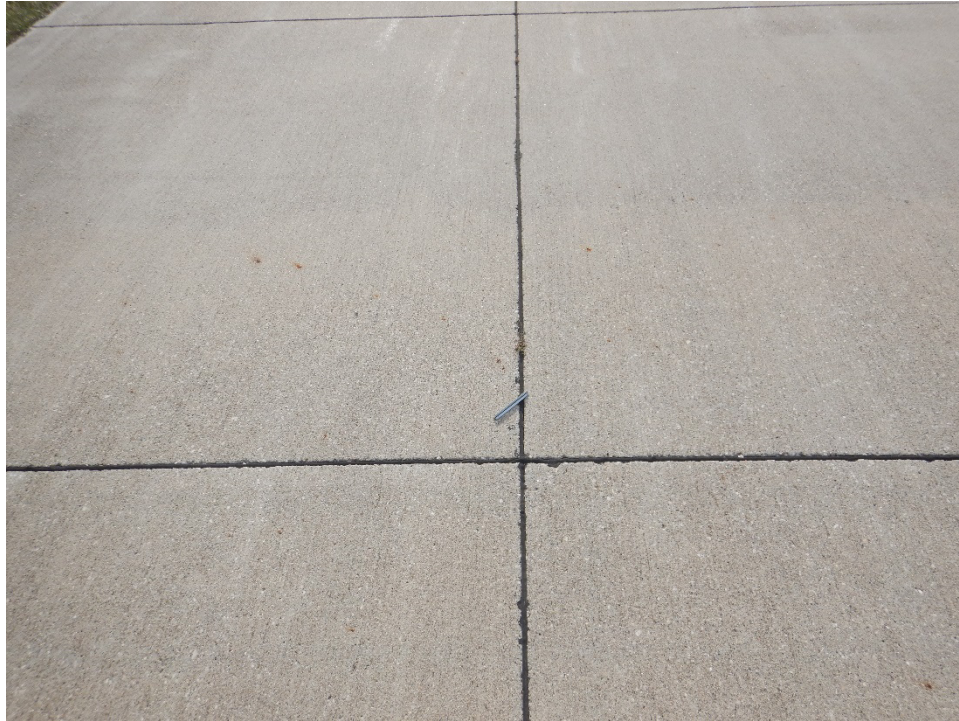
T01CA-02. Joint Seal Damage (Sample Unit No. 09).
