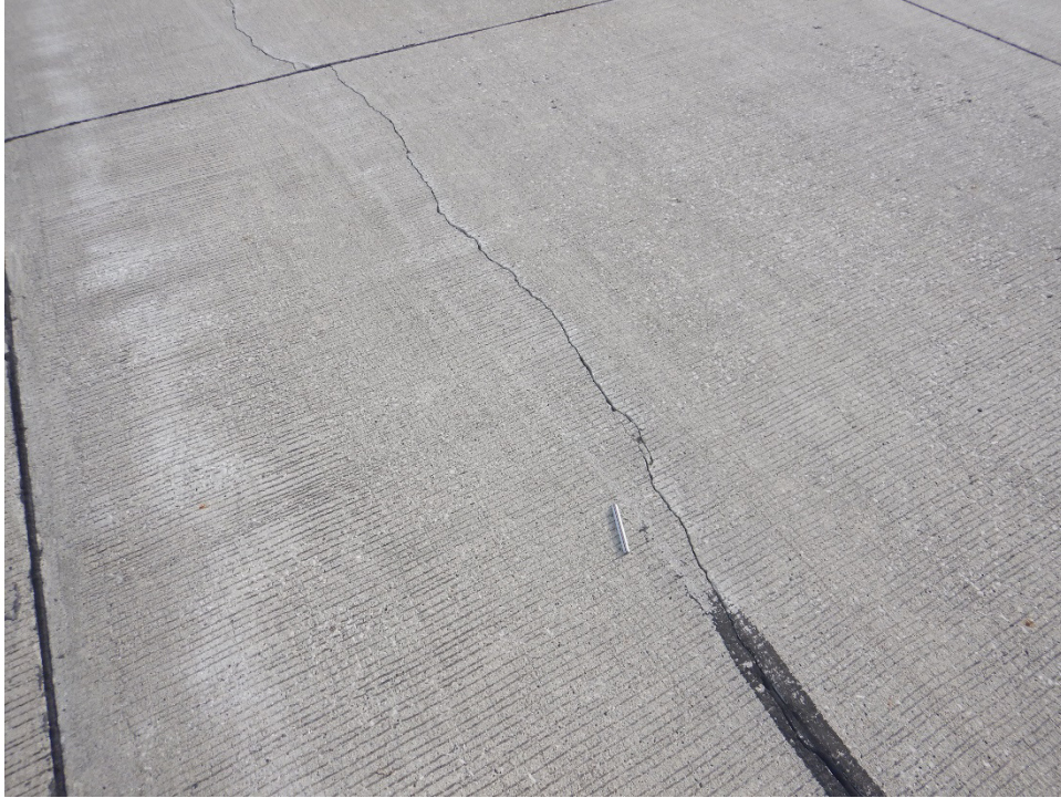
R13CA-04. LTD Cracking (Sample Unit No. 20).
