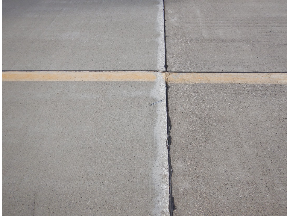
TH02CA-01. Faulting (Sample Unit No. 03).
