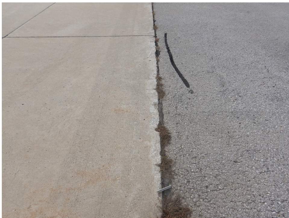
A01CL-05. Joint Spalling (Sample Unit No. 01).
