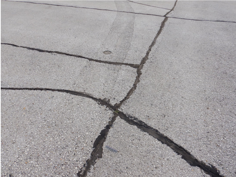
TACL-01. L&T Cracking (Sample Unit No. 01).
