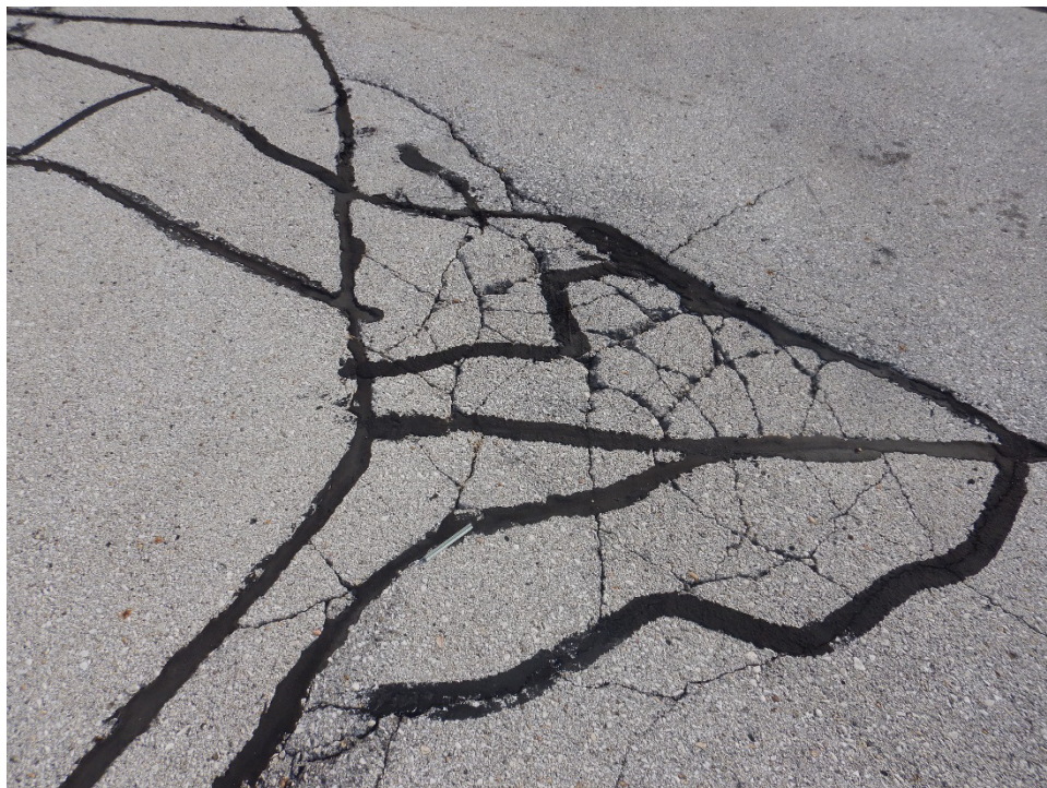
A01CL-01. Alligator Cracking (Sample Unit No. 01).
