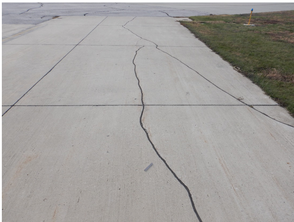
TH01CL-01. LTD Cracking (Sample Unit No. 01).
