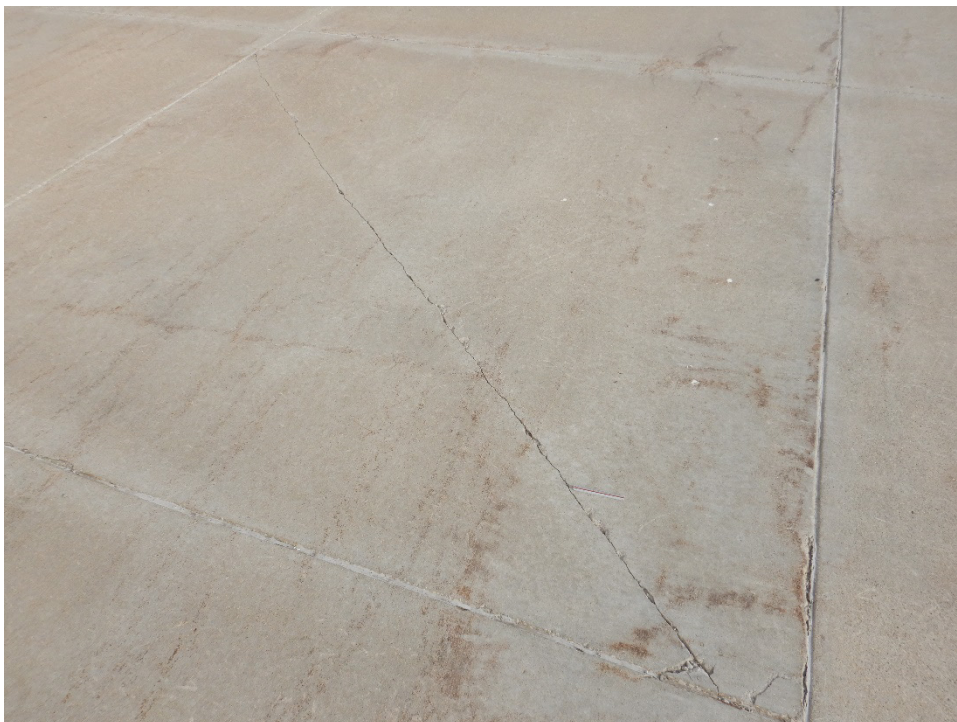
A01CL-06. LTD Cracking (Sample Unit No. 03).
