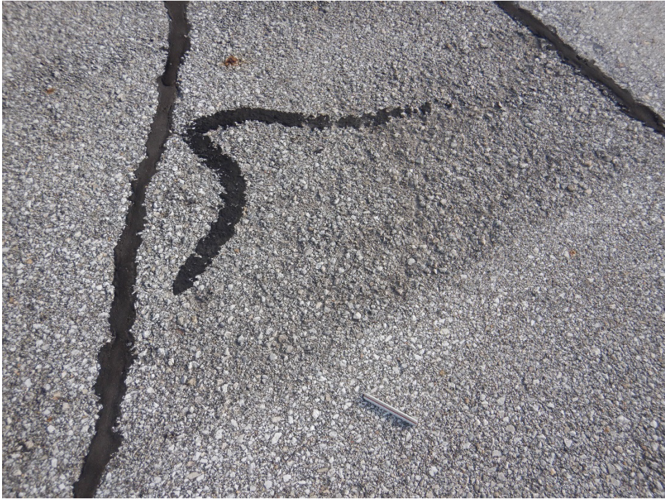
A01CL-02. Weathering (Sample Unit No. 02).
