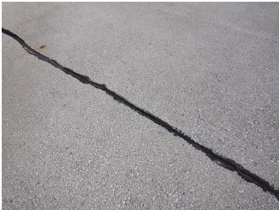
A01CL-04. L&T Cracking (Sample Unit No. 01).
