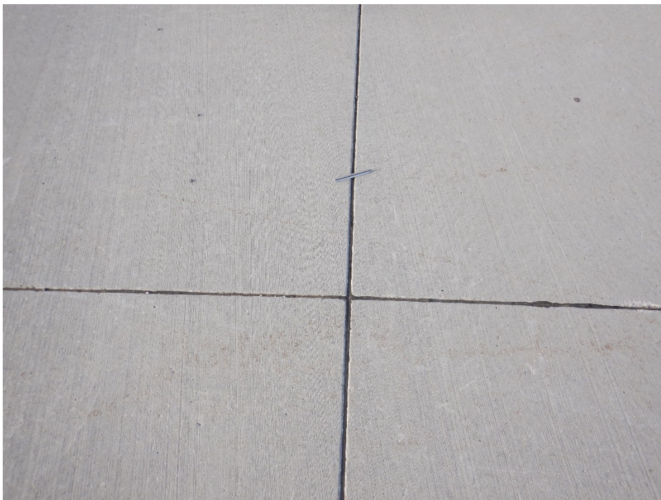
TACL-02. Joint Seal Damage (Sample Unit No. 01).
