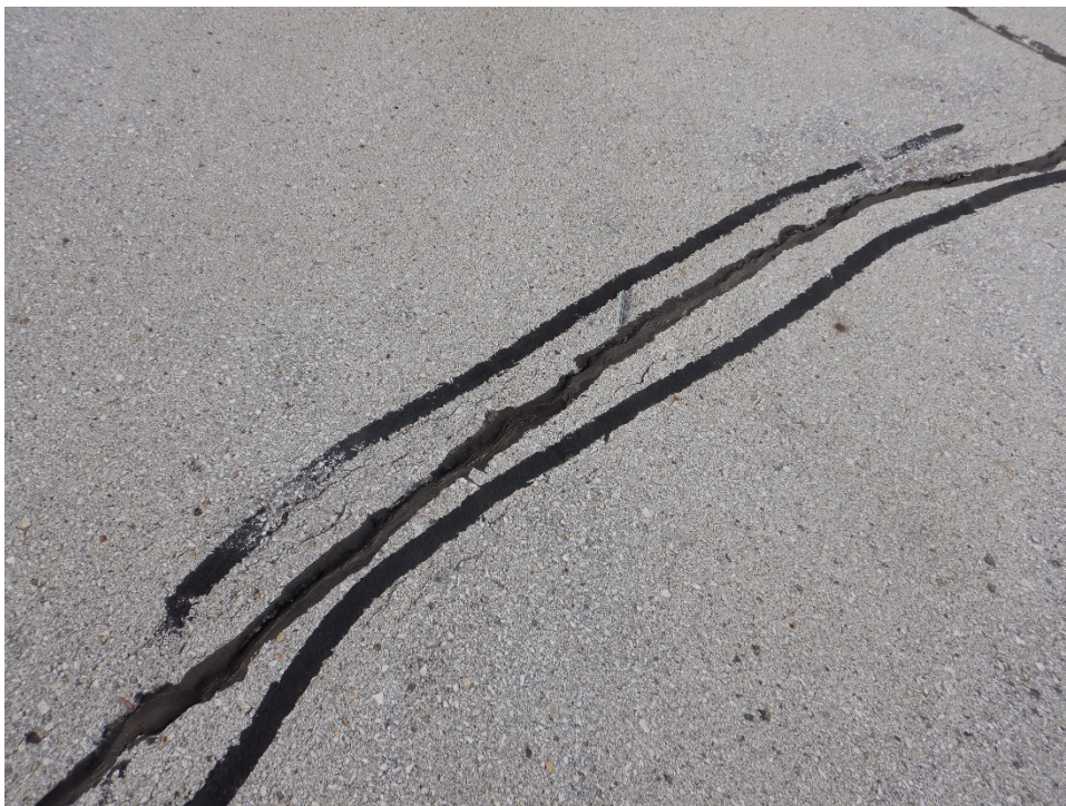
A01CL-03. L&T Cracking (Sample Unit No. 01).
