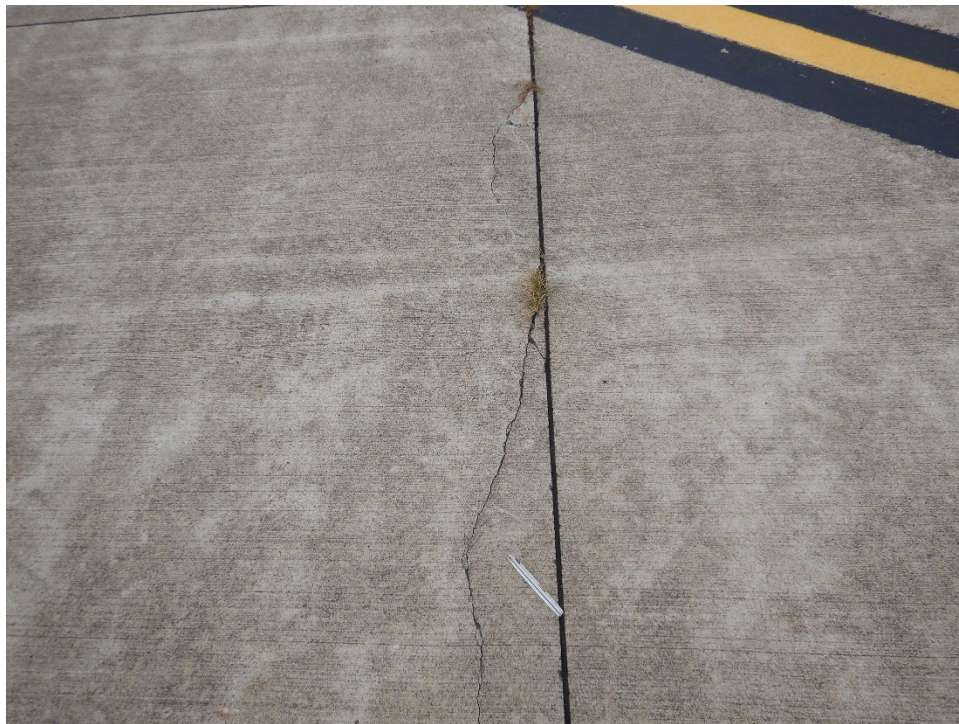
T06CN-01. Joint Spalling (Sample Unit No. 04).
