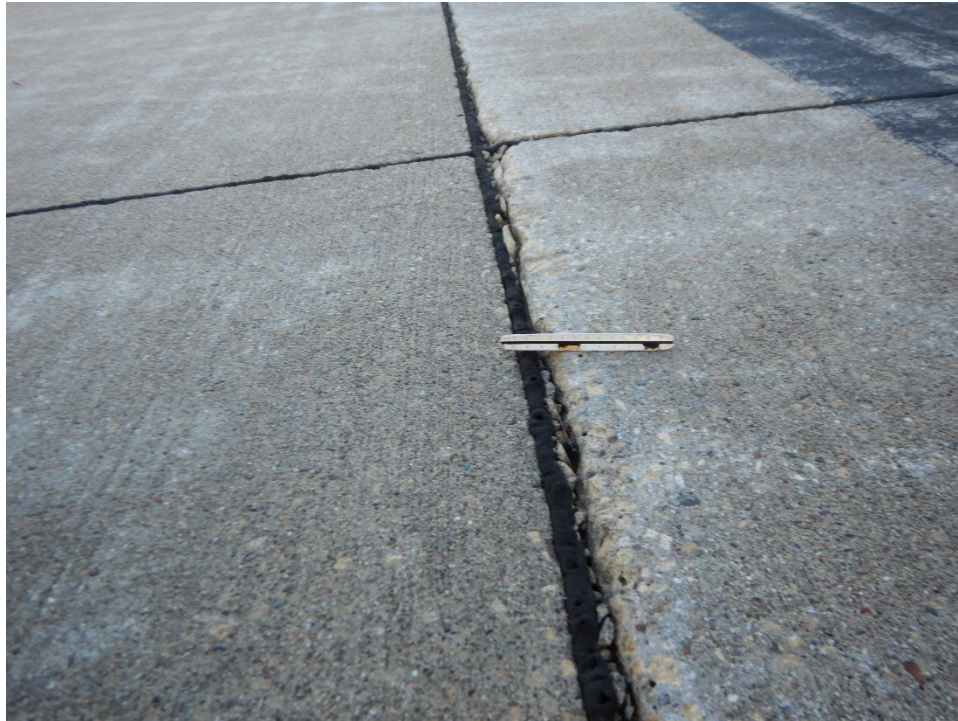
T07CN-01. Faulting (Sample Unit No. 04).
