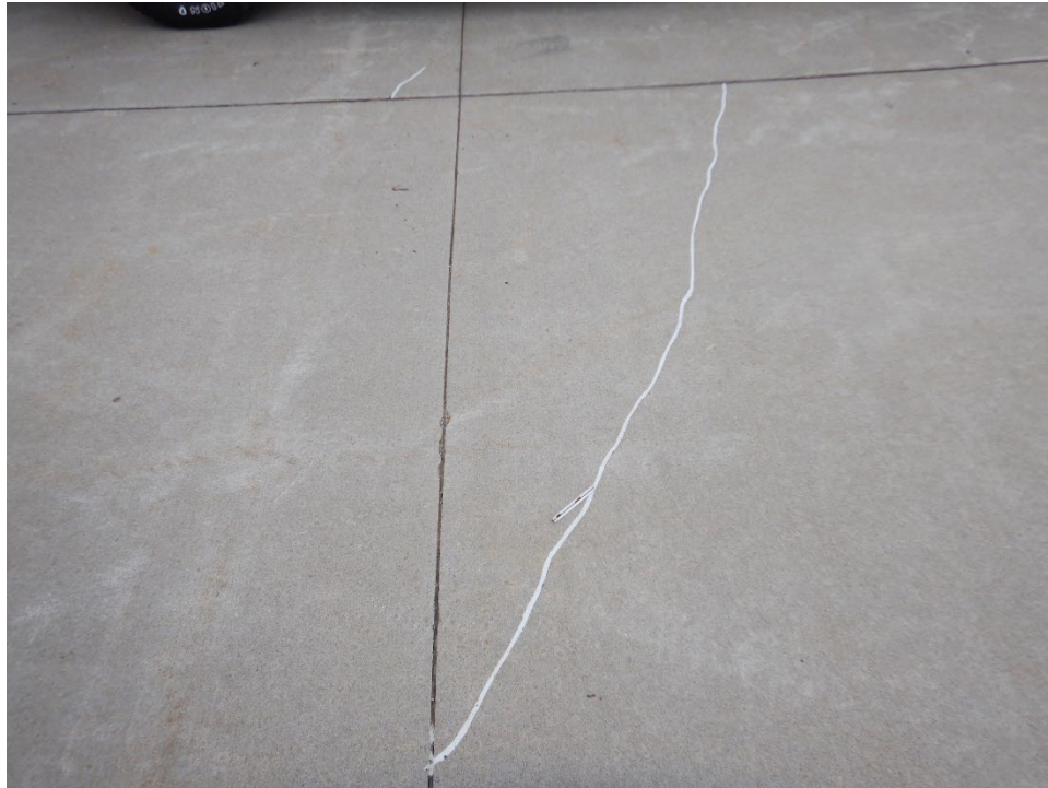
A01CN-02. LTD Cracking (Sample Unit No. 01).
