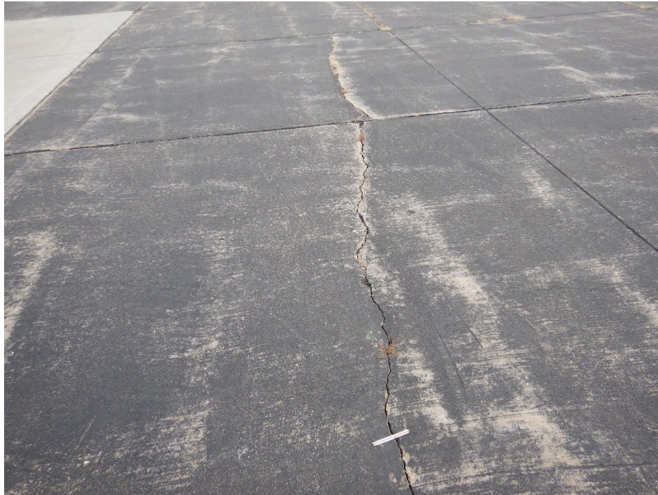
A01CN-01. LTD Cracking (Sample Unit No. 05).
