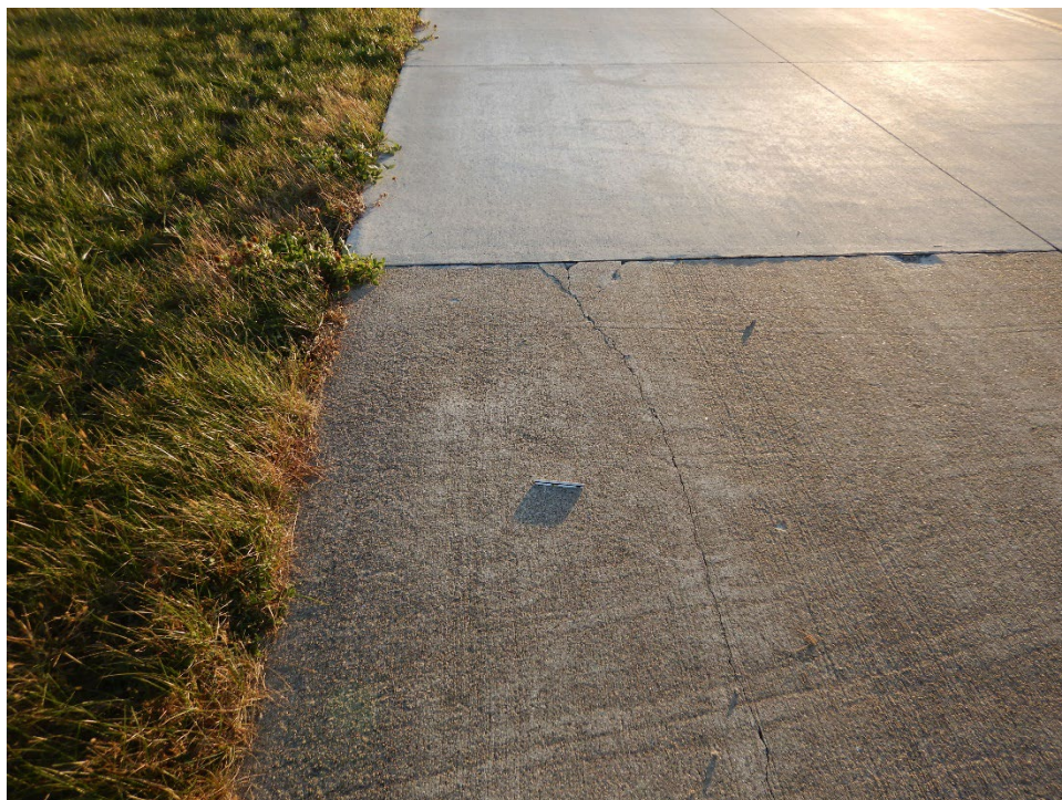
T03CN-03. LTD Cracking (Additional Sample Unit No. 42).
