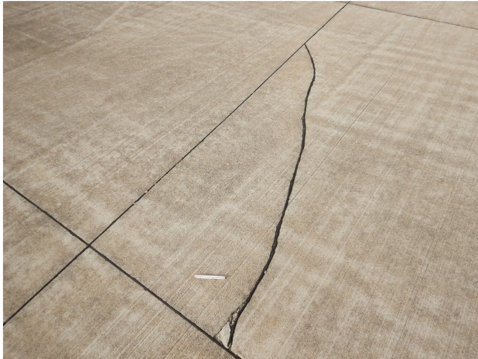
T05CN-01. LTD Cracking (Sample Unit No. 06).
