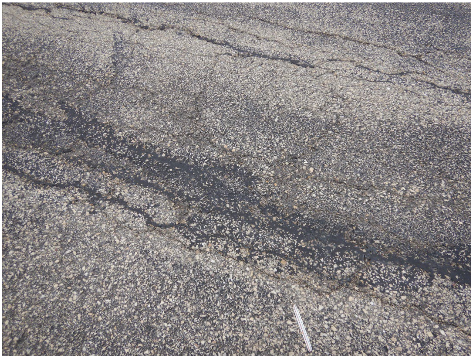
T04CN-01. Alligator Cracking (Sample Unit No. 05).
