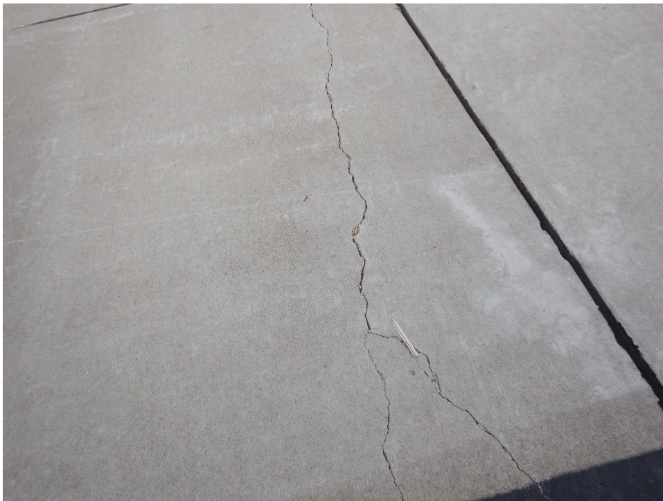
T01CN-03. LTD Cracking (Sample Unit No. 05).
