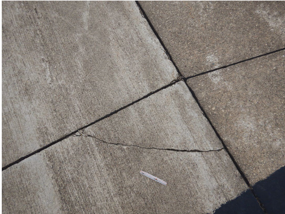
T03CN-02. Corner Spalling (Sample Unit No. 01).
