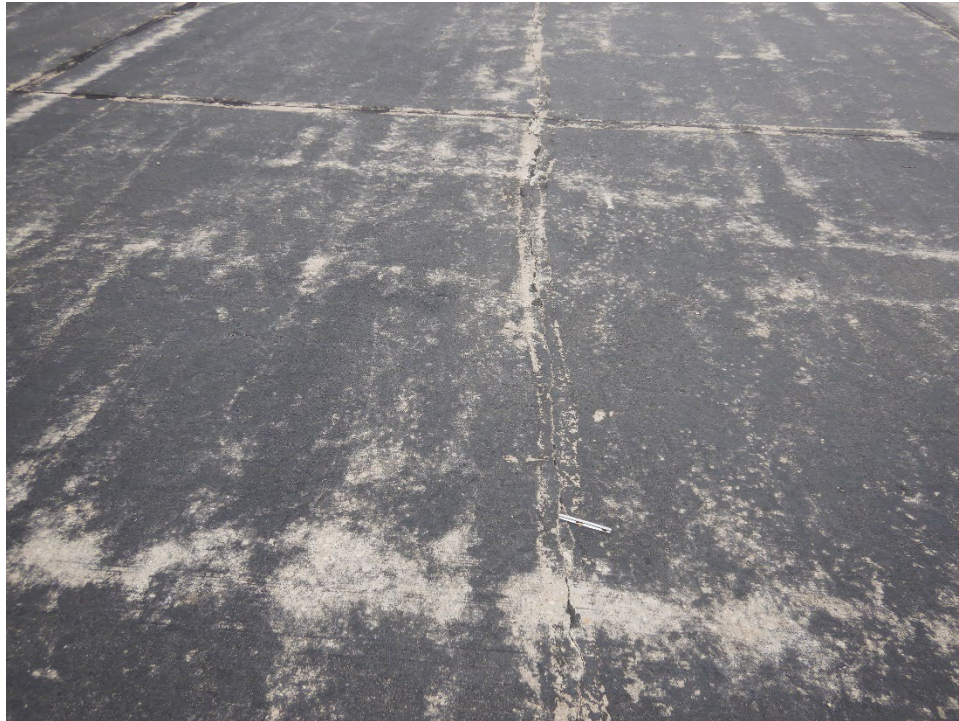
T04CN-02. LTD Cracking (Sample Unit No. 01).
