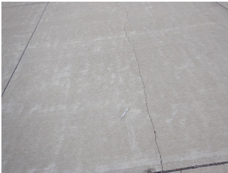
A01CN-04. LTD Cracking (Sample Unit No. 03).
