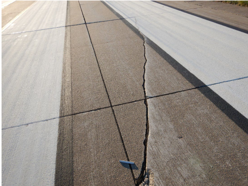
R14CN-01. LTD Cracking (Sample Unit No. 88).
