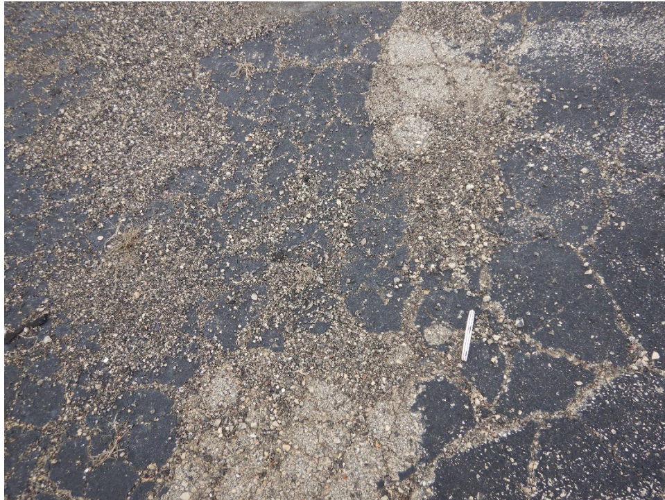
A01CN-03. Alligator Cracking (Sample Unit No. 03).
