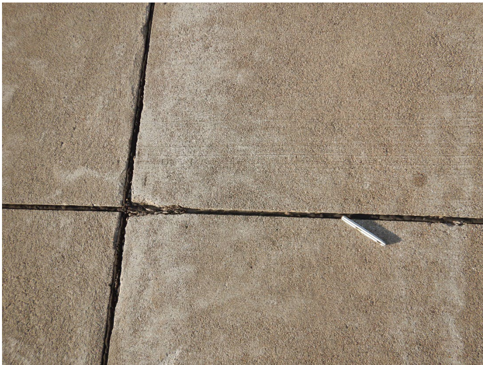
T02CN-01. Joint Seal Damage (Sample Unit No. 01).
