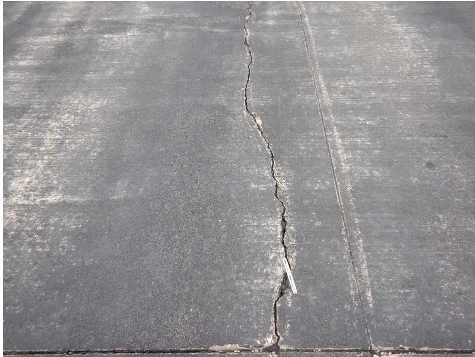
A02CN-01. LTD Cracking (Sample Unit No. 06).
