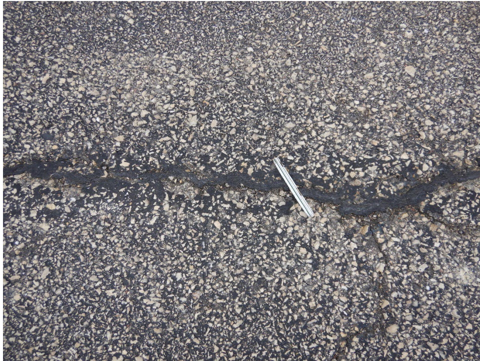
T04CN-01. L&T Cracking (Sample Unit No. 05).
