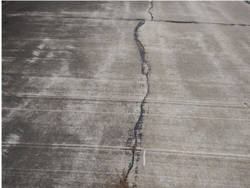
TH01CN-01. LTD Cracking (Sample Unit No. 07).
