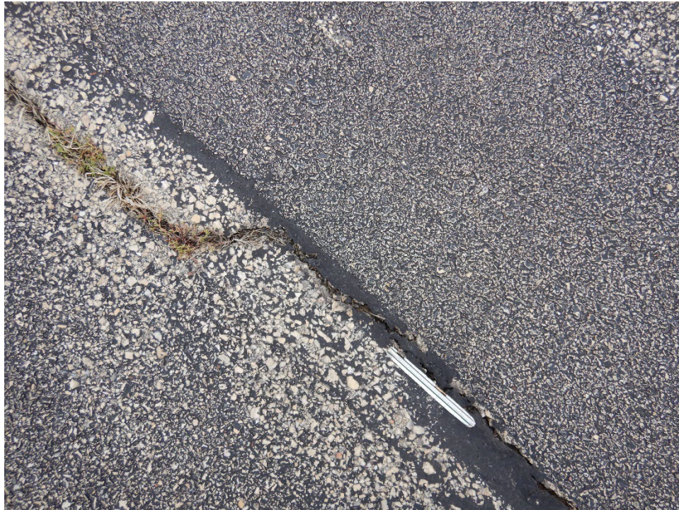
TH01CN-03. L&T Cracking (Sample Unit No. 02).
