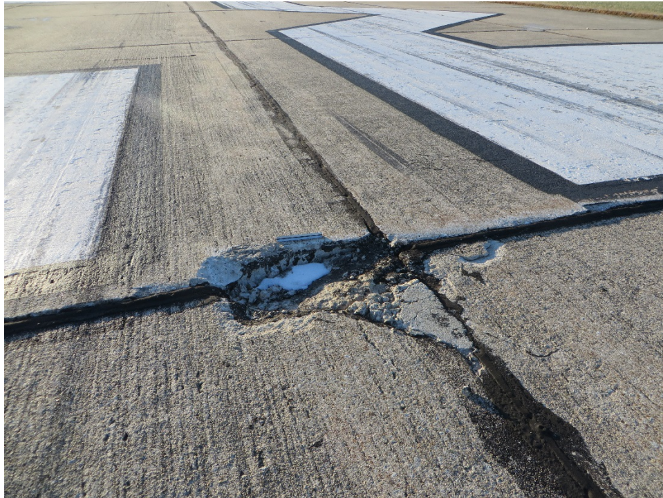
R15CR-01. Corner Spalling (Sample Unit No. 04).
