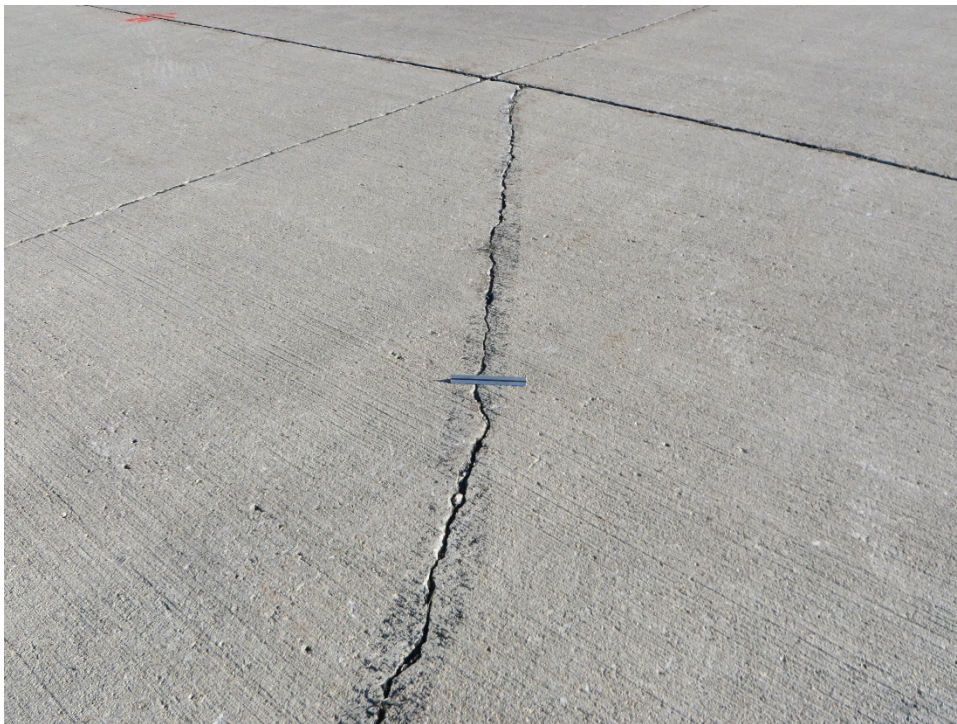
A02CR-01. LTD Cracking (Sample Unit No. 02).
