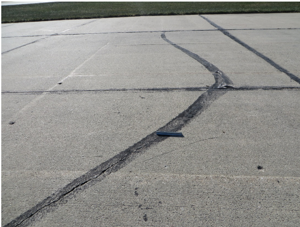
A02CR-02. LTD Cracking (Sample Unit No. 01).
