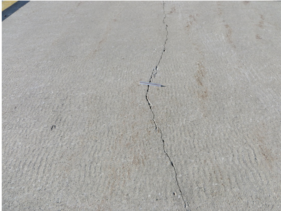
T01CR-01. LTD Cracking (Sample Unit No. 01).
