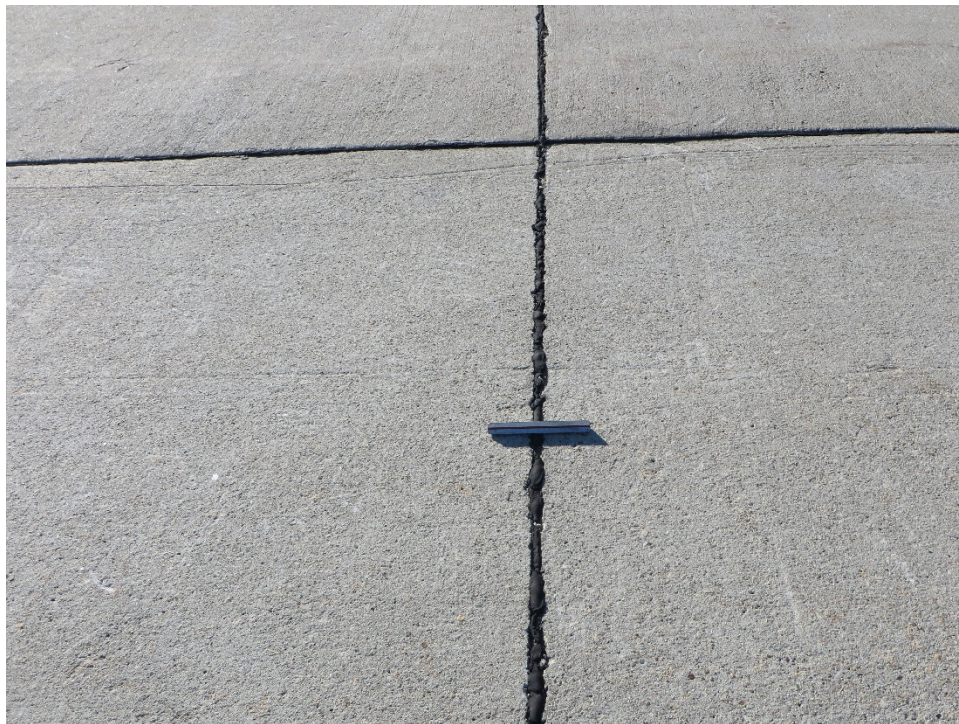
A01CR-01. Joint Seal Damage (Sample Unit No. 01).
