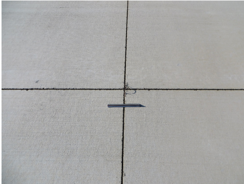
T04CR-01. Joint Seal Damage (Sample Unit No. 01).
