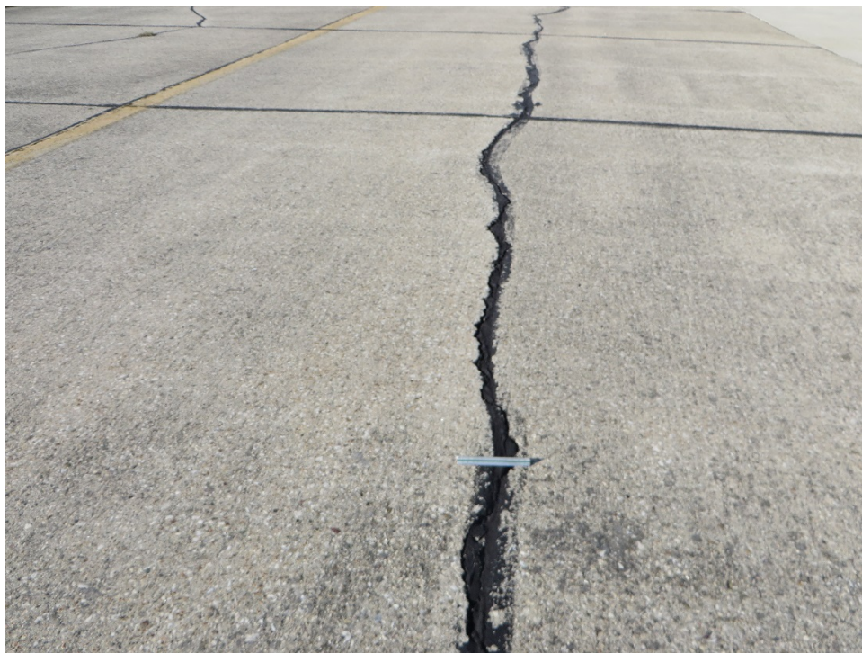
A01CR-03. LTD Cracking (Sample Unit No. 01).
