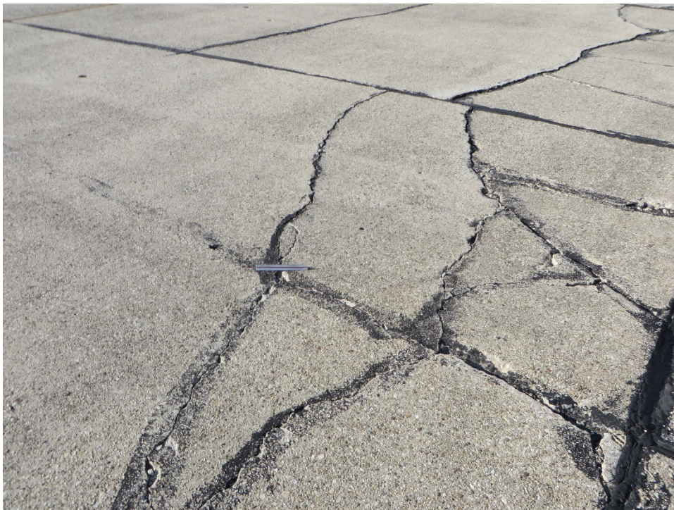
A01CR-02. Shattered Slab (Sample Unit No. 01).
