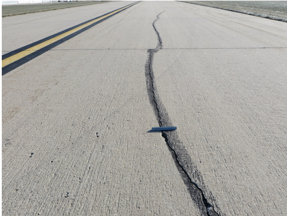
T03CR-01. LTD Cracking (Sample Unit No. 04).
