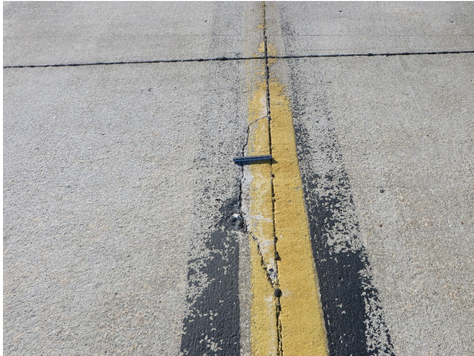
T02CR-01. Joint Spalling (Sample Unit No. 01).
