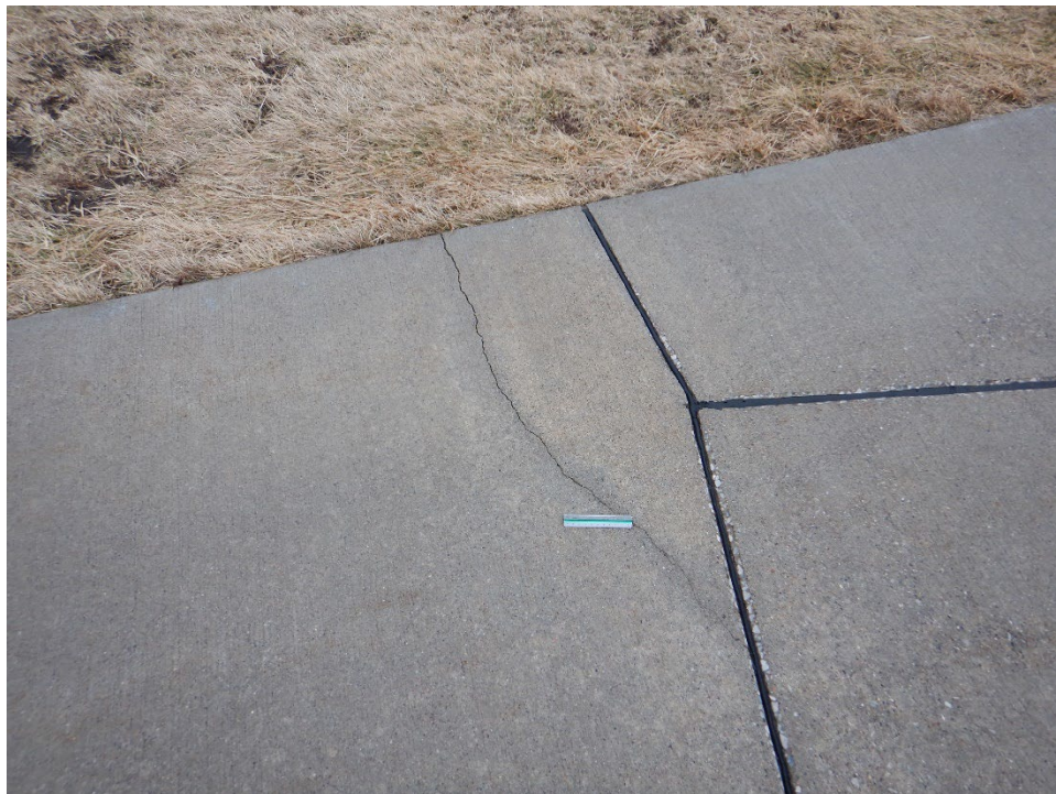
T01DA-05. Corner Break (Sample Unit No. 08).
