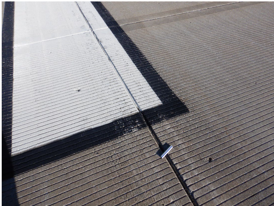
R15DA-03. Joint Seal Damage (Sample Unit No. 06).
