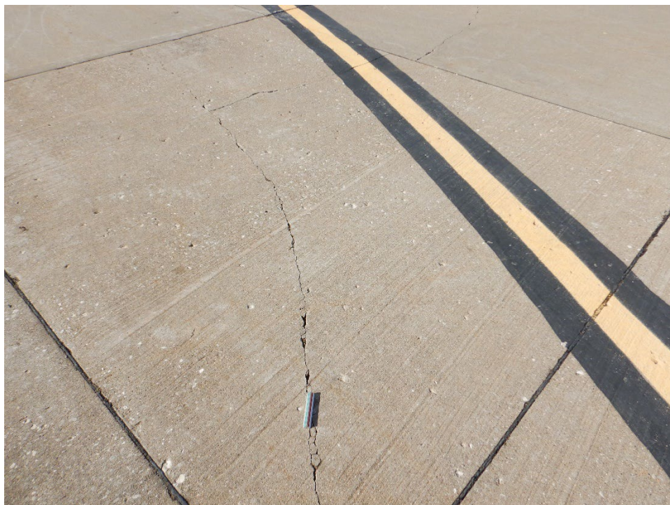
T02DA-02. LTD Cracking (Additional Sample Unit No. 04).
