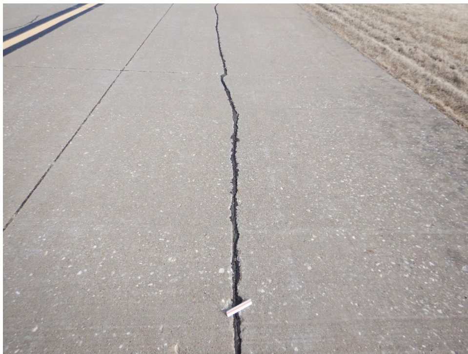
T02DA-03. LTD Cracking (Sample Unit No. 02).
