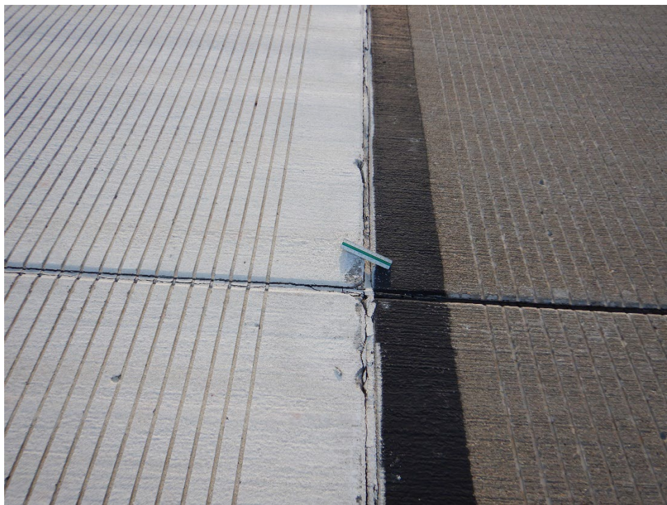
R03DA-01. Faulting (Sample Unit No. 07).
