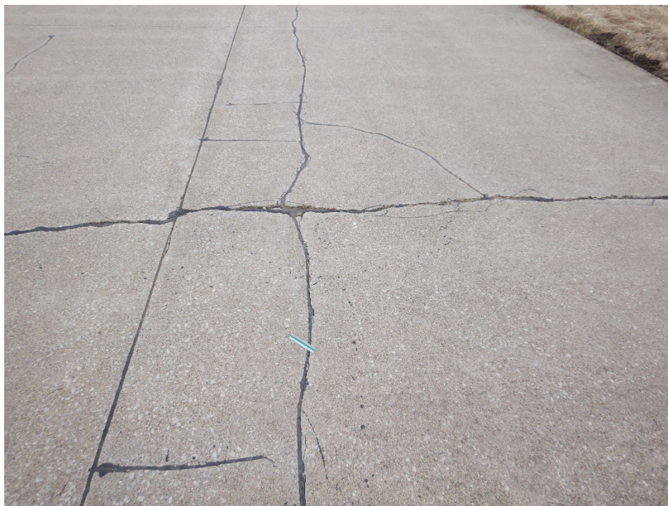
T03DA-01. Shattered Slab (Sample Unit No. 02).
