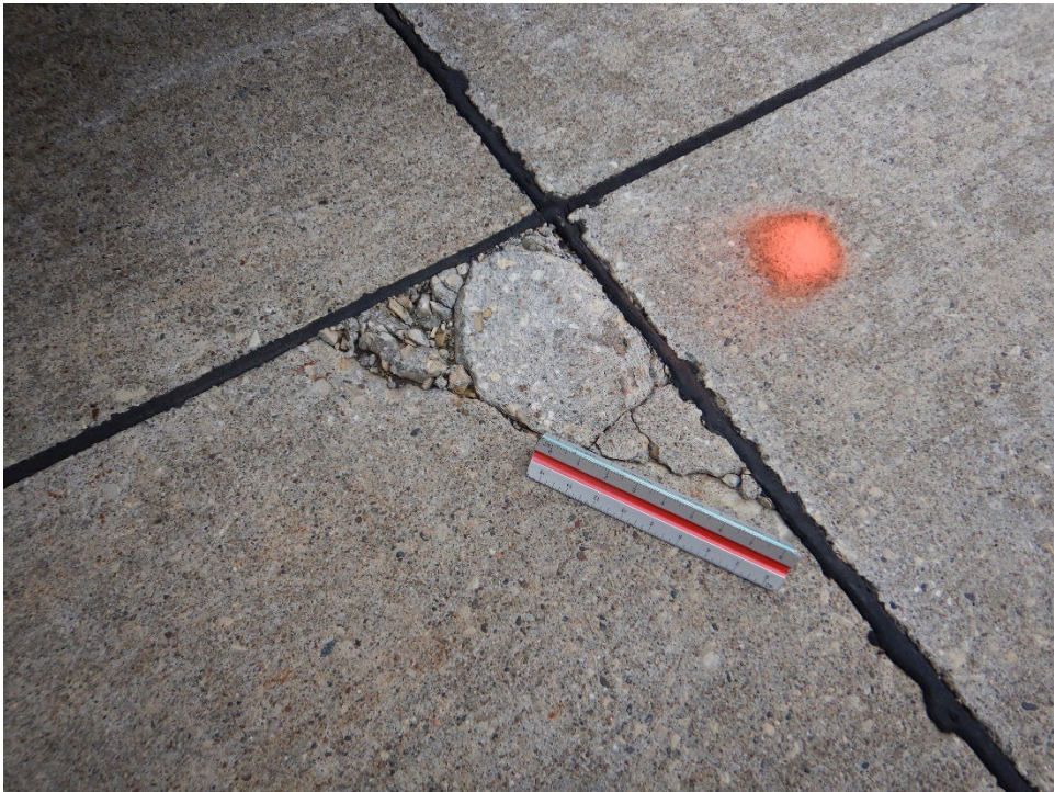
TH01DA-04. Corner Spalling (Sample Unit No. 09).
