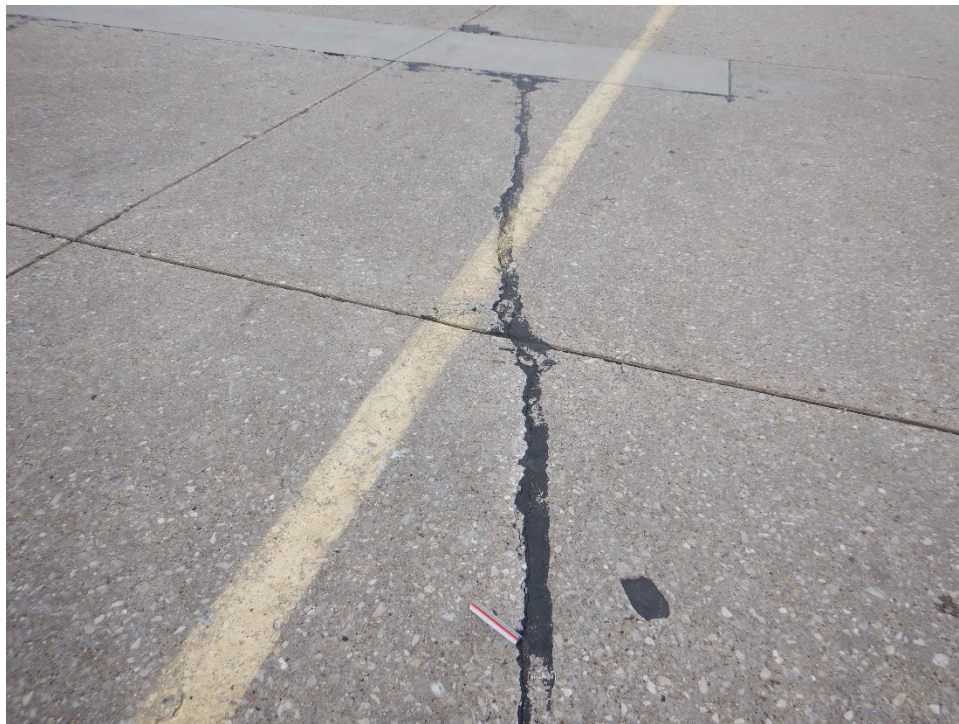
T04DA-01. LTD Cracking (Sample Unit No. 01).
