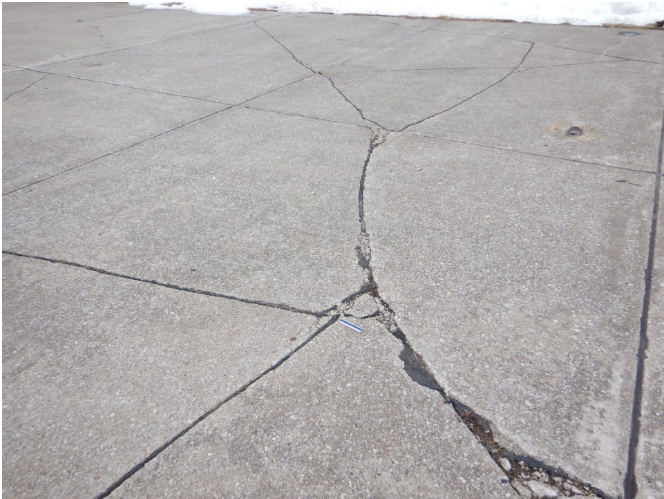
A02DA-01. Shattered Slab (Sample Unit No. 07).
