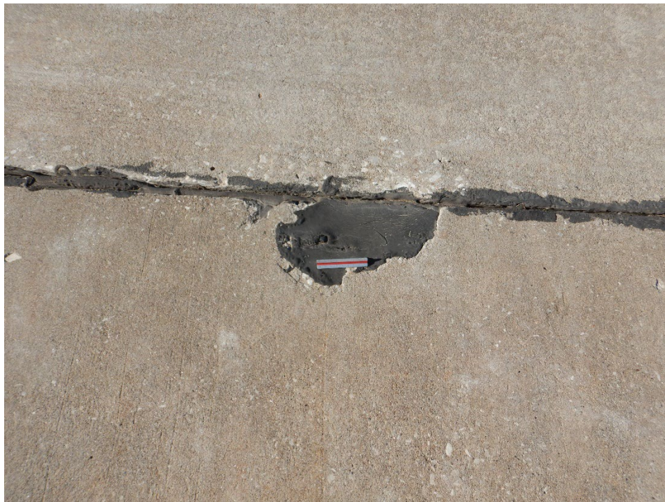
T07DA-01. Joint Spalling (Sample Unit No. 02).
