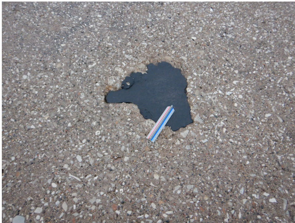
T01DA-02. Small Patching (Sample Unit No. 15).
