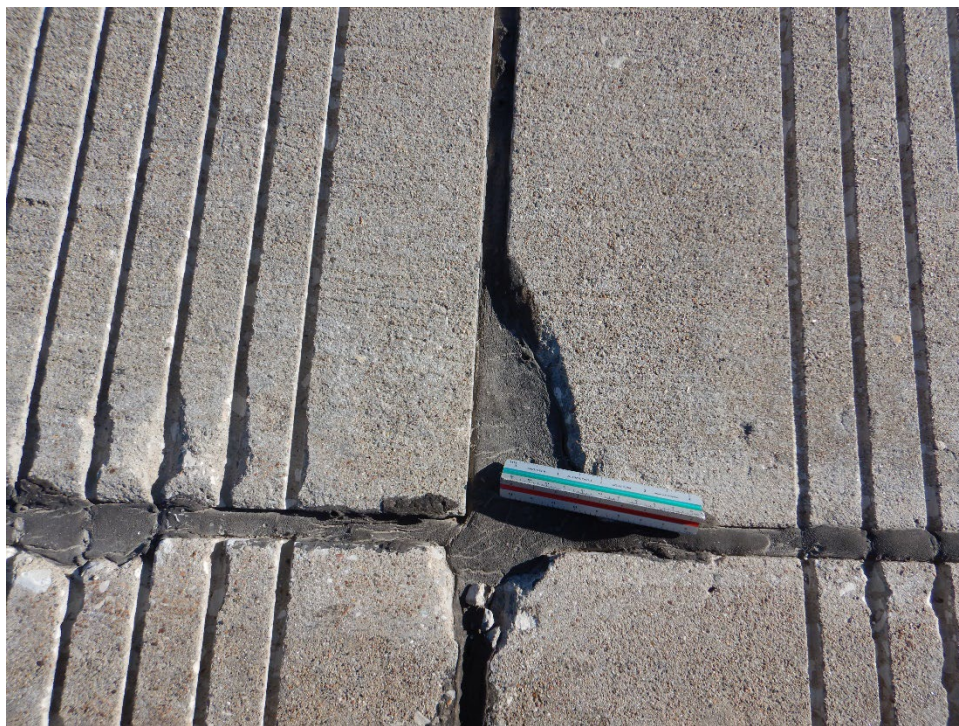
R15DA-02. Corner Spalling (Sample Unit No. 01).
