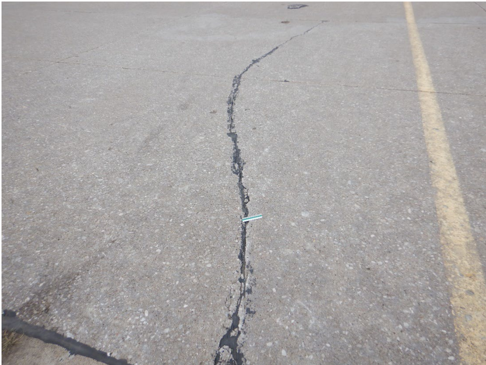
A01DA-01. LTD Cracking (Sample Unit No. 07).
