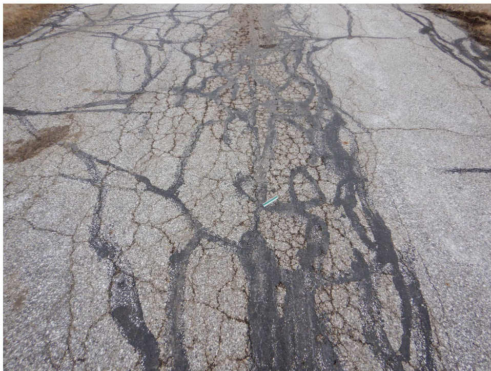
TH01DA-02. Alligator Cracking (Sample Unit No. 07).
