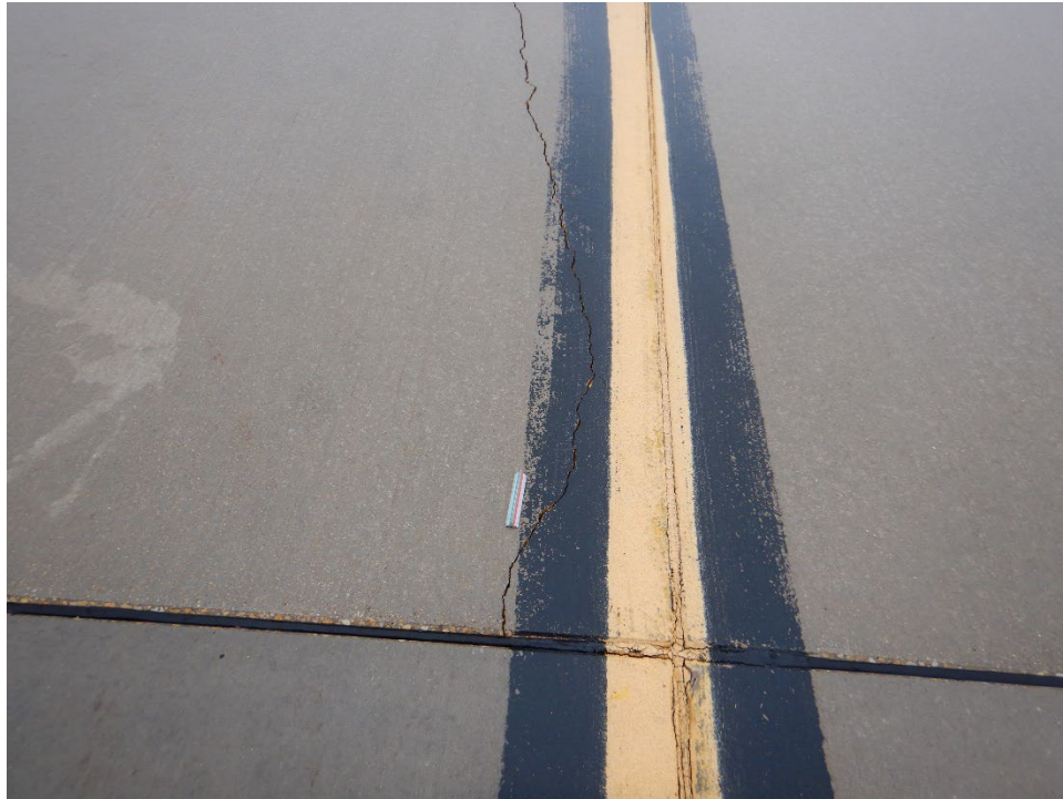
T01DA-06. LTD Cracking (Additional Sample Unit No. 08).
