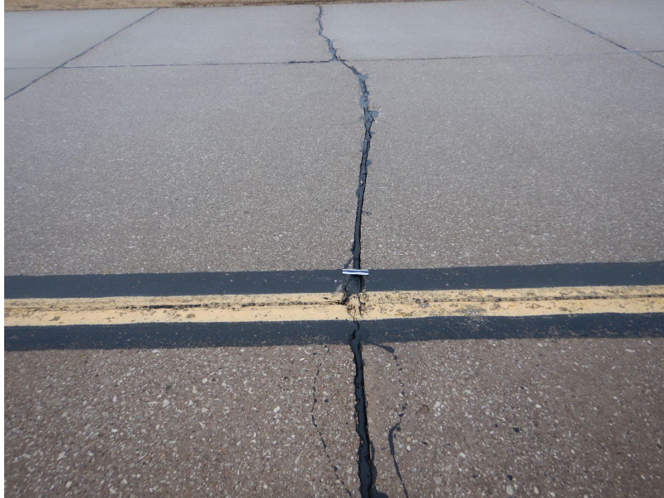
T01DA-01. LTD Cracking (Additional Sample Unit No. 04).
