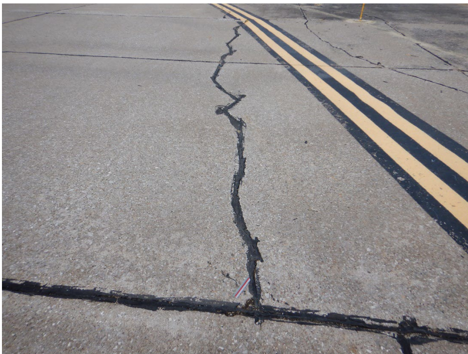
T01DA-03. LTD Cracking (Sample Unit No. 03).
