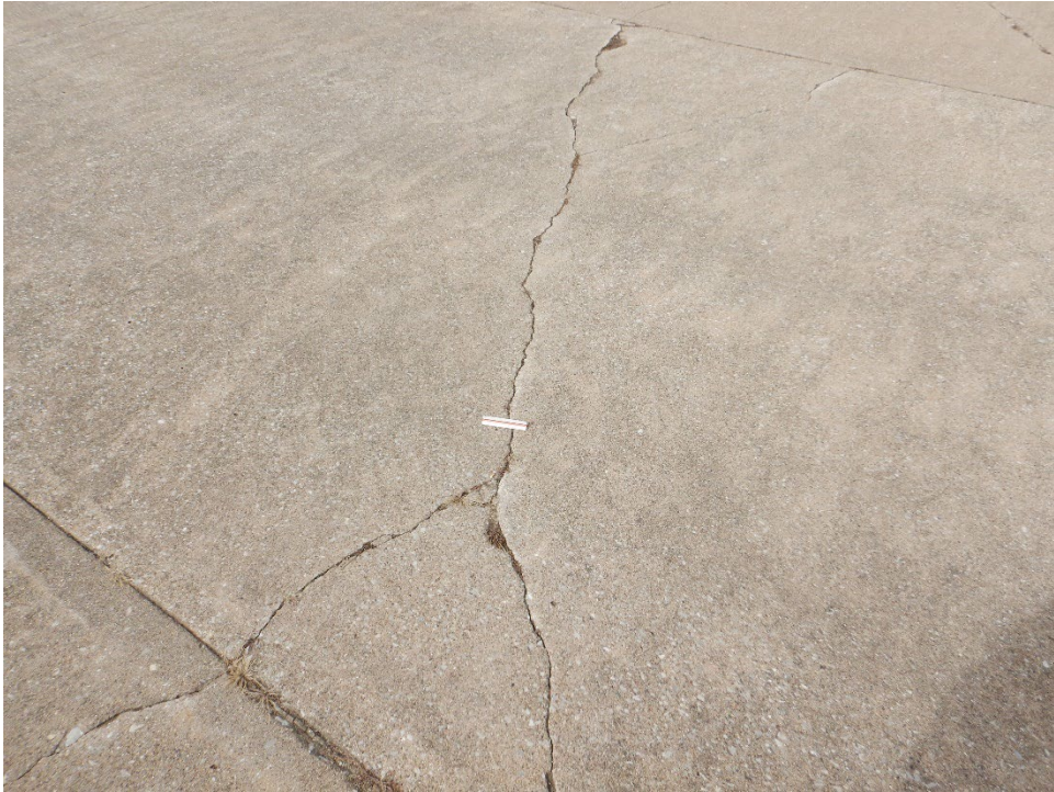
A04DA-01. Shattered Slab (Sample Unit No. 05).
