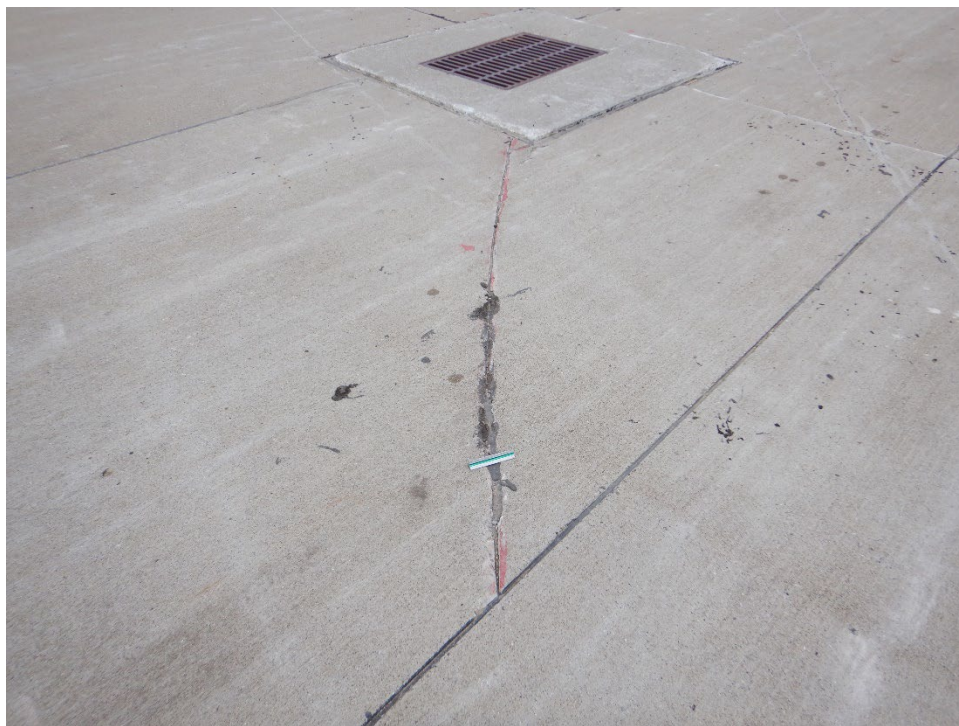
TH01DA-03. LTD Cracking (Sample Unit No. 07).
