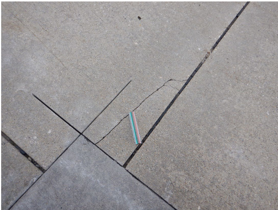
A02DA-02. Joint Spalling (Sample Unit No. 04).
