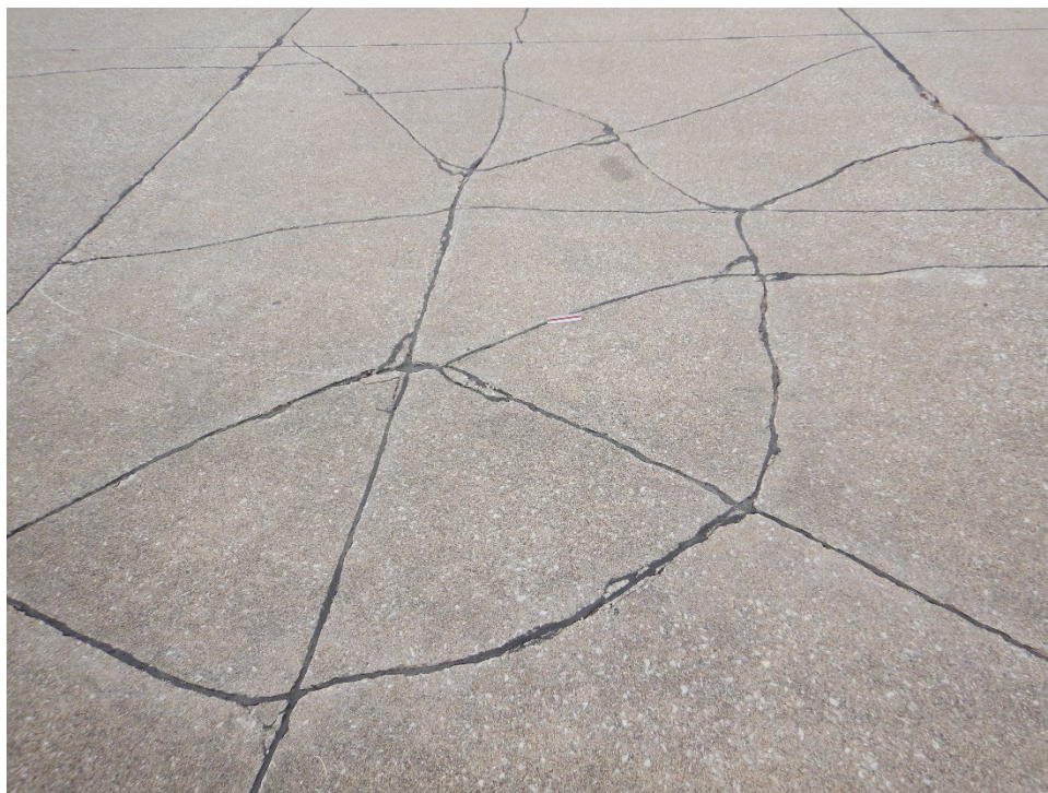
A03DA-01. Shattered Slab (Sample Unit No. 04).
