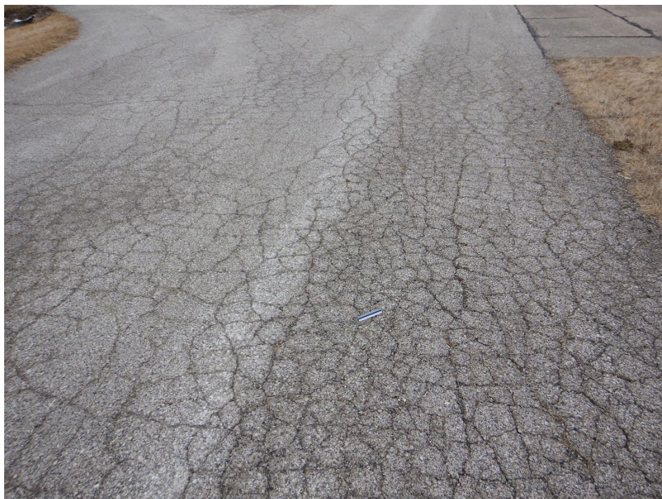
TH01DA-01. Alligator Cracking (Sample Unit No. 02).
