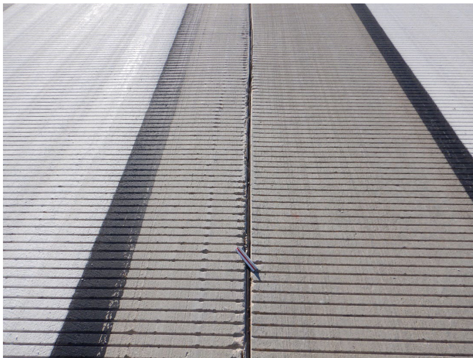
R15DA-01. Joint Seal Damage (Sample Unit No. 05).
