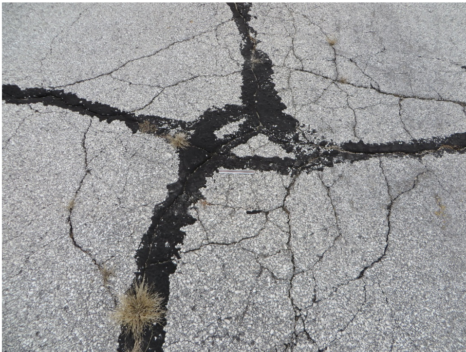
A01EG-01. Alligator Cracking (Sample Unit No. 01).
