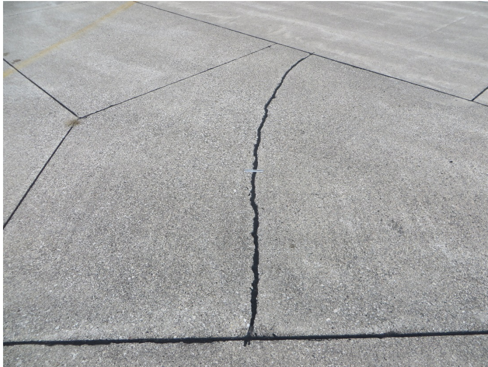
T01EG-01. LTD Cracking (Sample Unit No. 01).
