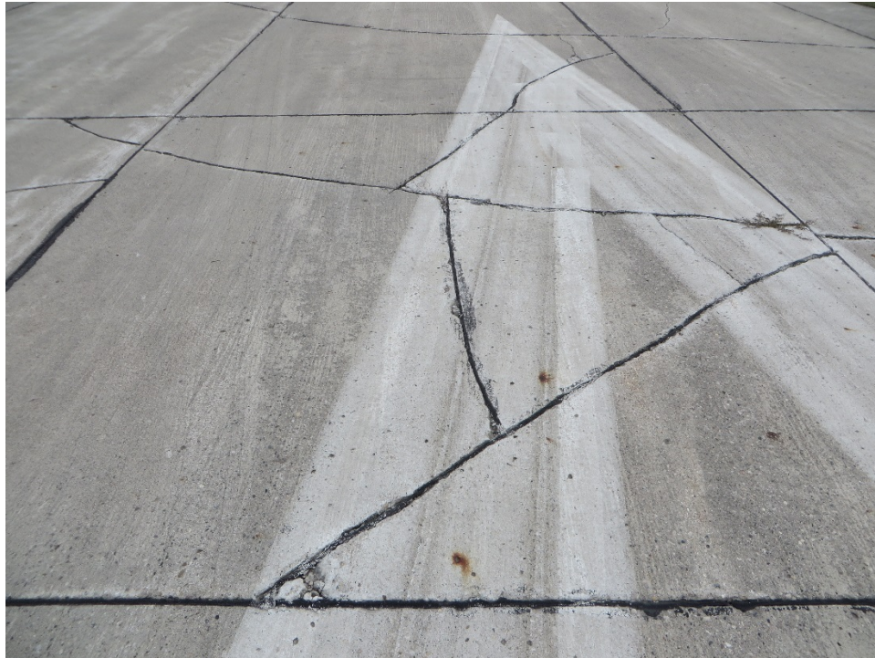
R13EG-01. Shattered Slab (Sample Unit No. 04).
