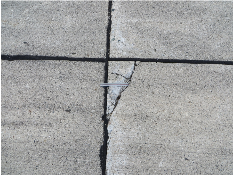
T01EG-02. Joint Spalling (Sample Unit No. 04).
