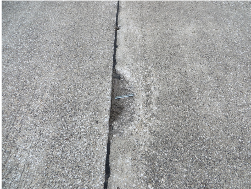
R13EG-02. Joint Spalling (Sample Unit No. 12).
