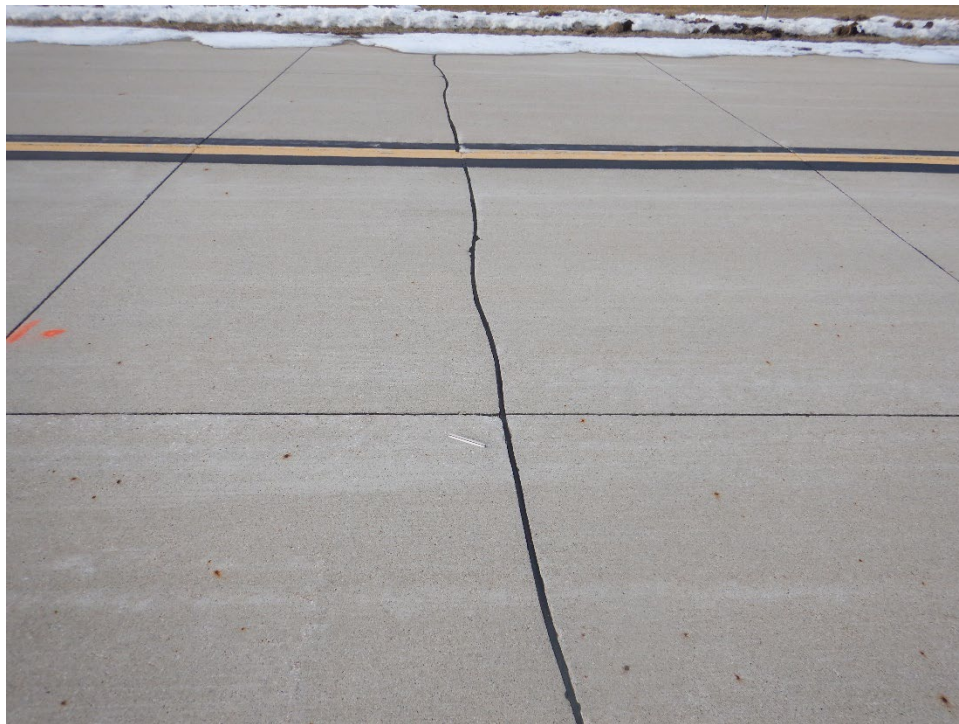
T01EM-01. LTD Cracking (Sample Unit No. 02).
