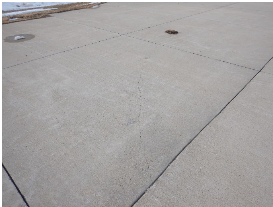
A01EM-01. LTD Cracking (Sample Unit No. 21).
