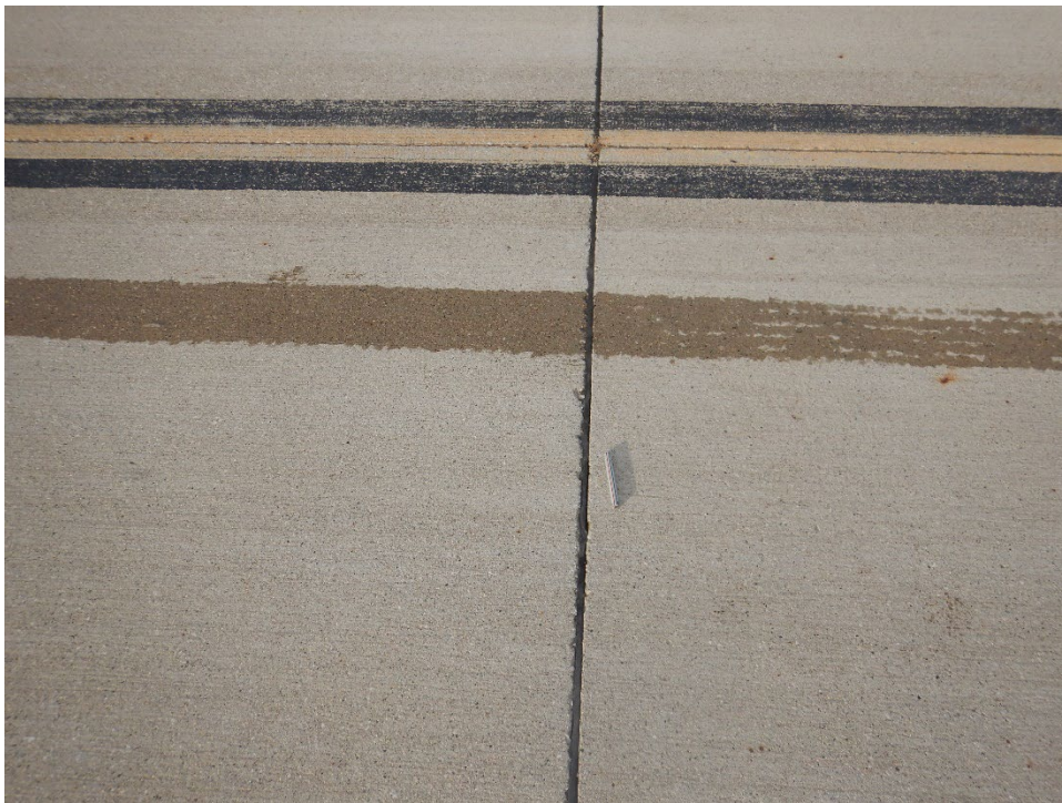
TH01EM-01. Joint Seal Damage (Sample Unit No. 05).
