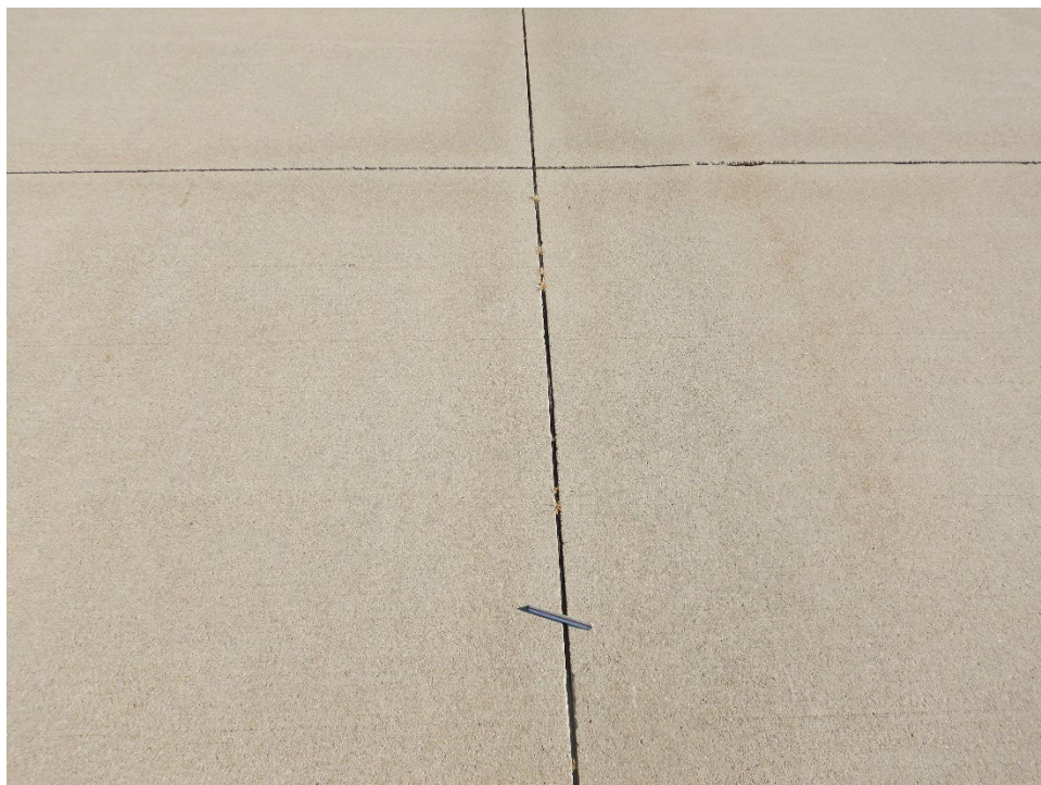
T01ES-01. Joint Seal Damage (Sample Unit No. 01).
