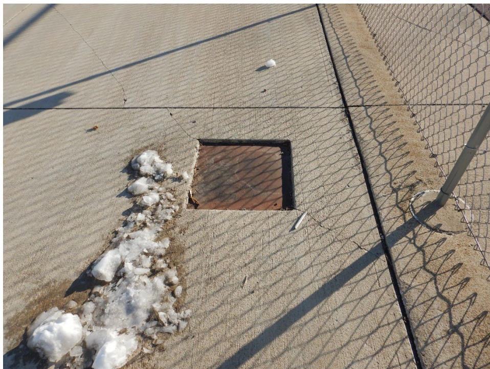
A01ES-01. Corner Break (Sample Unit No. 29).
