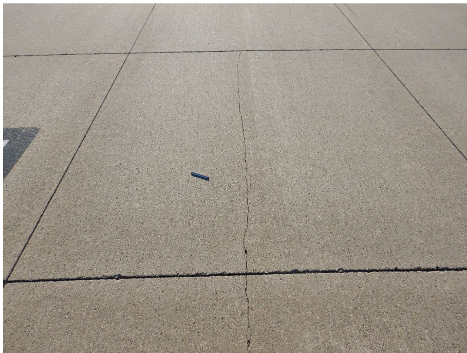
R16ES-01. LTD Cracking (Sample Unit No. 160).
