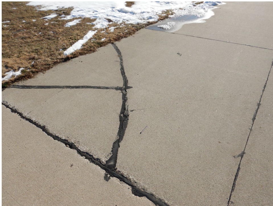
TH01ES-01. Shattered Slab (Sample Unit No. 05).
