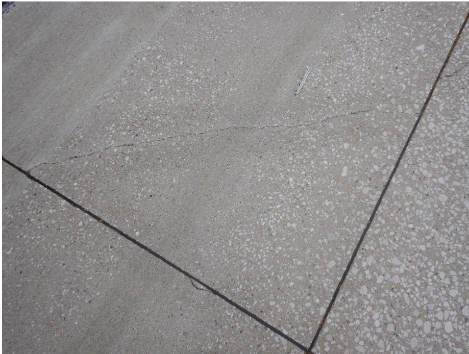
TFFD-02. Corner Break (Sample Unit No. 03).
