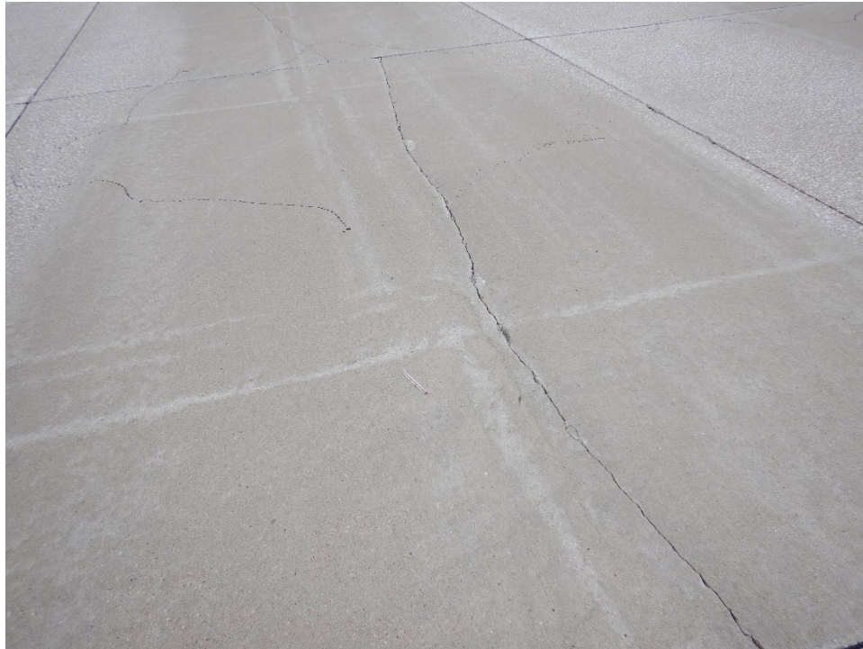
TDFD-03. LTD Cracking (Sample Unit No. 03).
