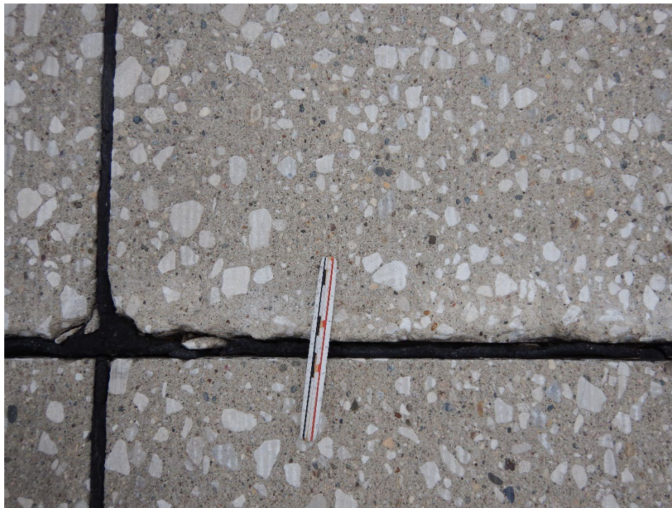
TDFD-03. Joint Seal Damage (Sample Unit No. 03).
