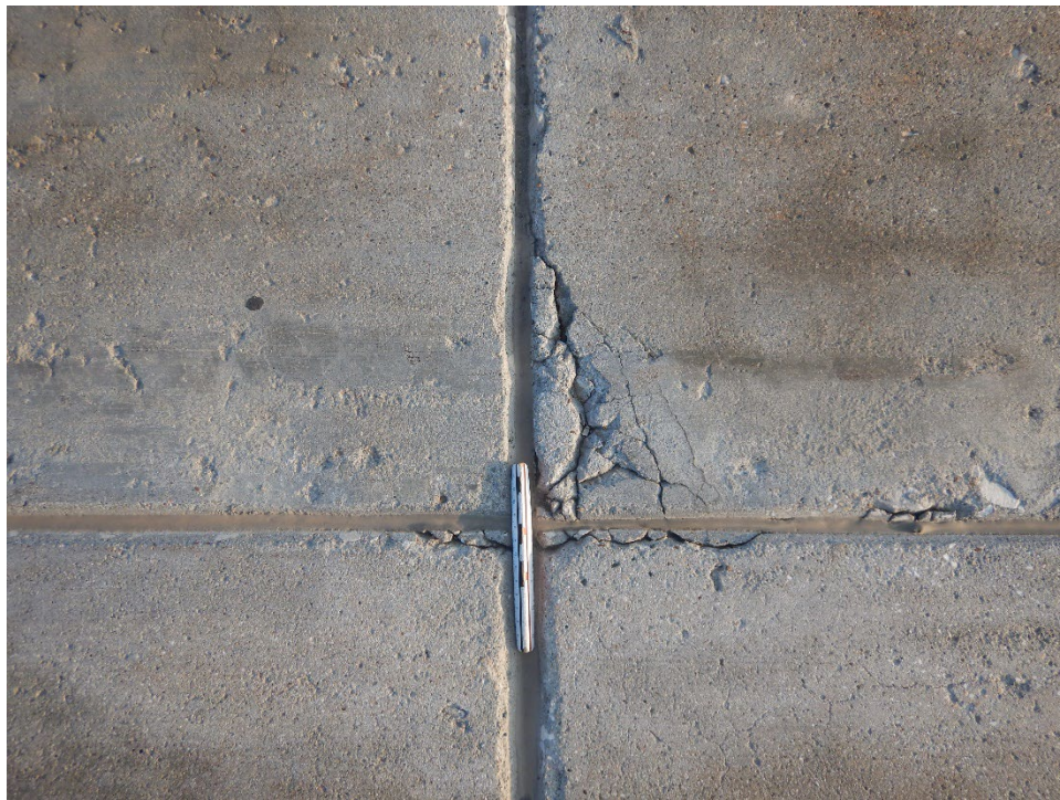
A02FD-02. Joint Spalling (Sample Unit No. 04).
