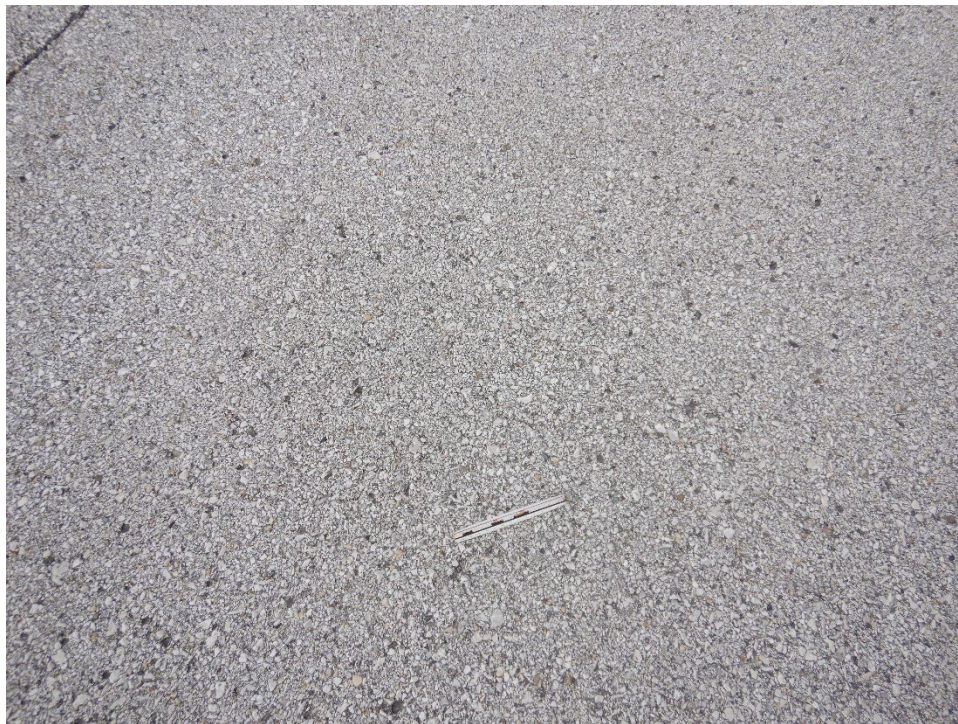
TBFD-01. Weathering (Sample Unit No. 11).
