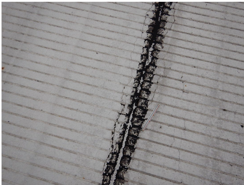
R06FD-01. L&T Cracking (Sample Unit No. 155).
