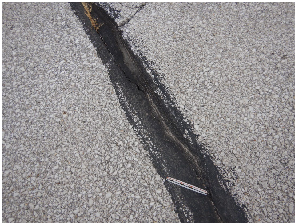
TH01FD-01. L&T Cracking (Sample Unit No. 09).
