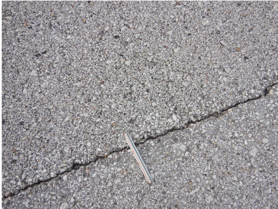
TBFD-01. L&T Cracking (Sample Unit No. 11).
