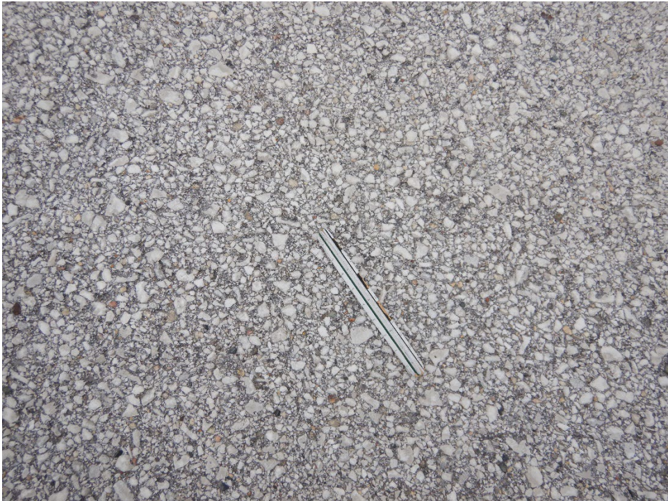
TBFD-02. Weathering (Sample Unit No. 09).
