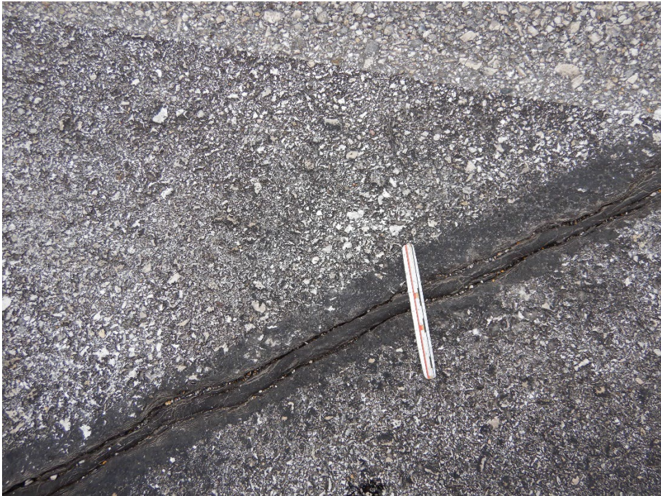
TBFD-05. L&T Cracking (Sample Unit No. 03).
