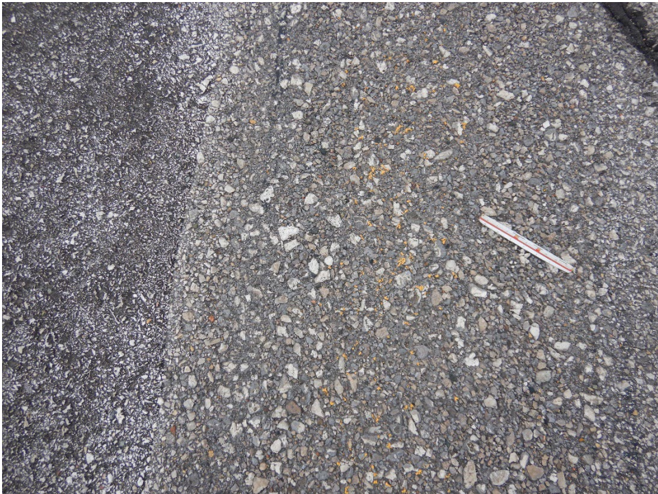
TBFD-05. Weathering (Sample Unit No. 03).
