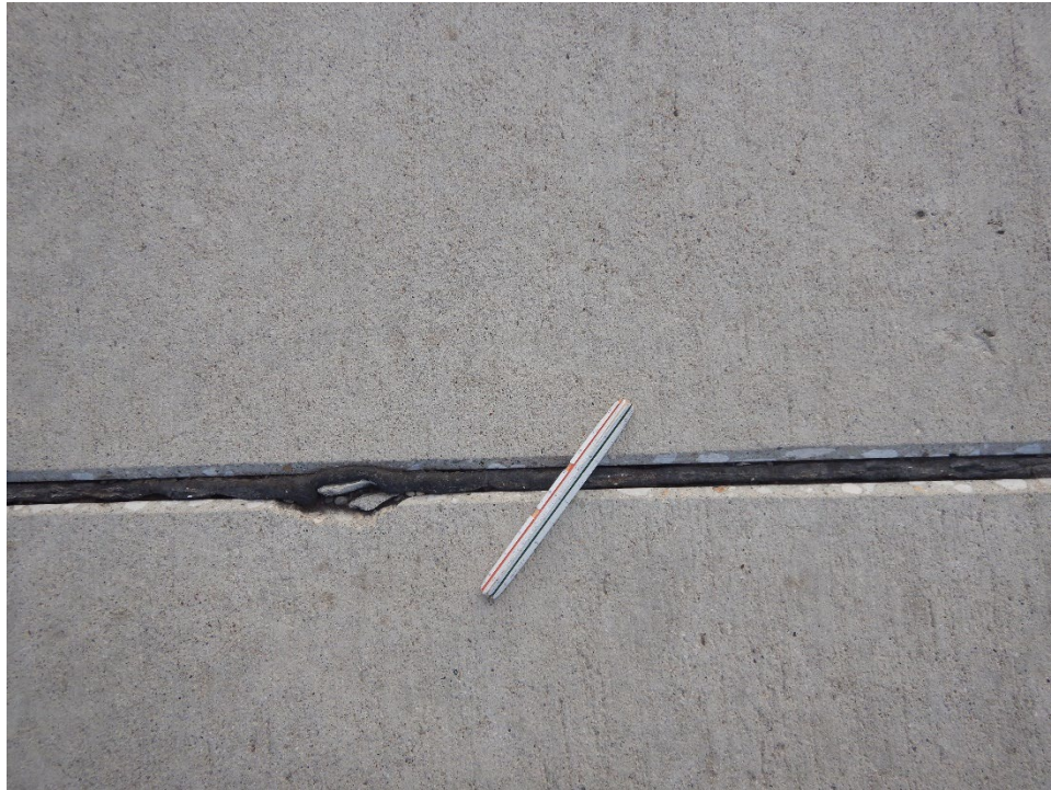
A02FD-01. Joint Seal Damage (Sample Unit No. 07).
