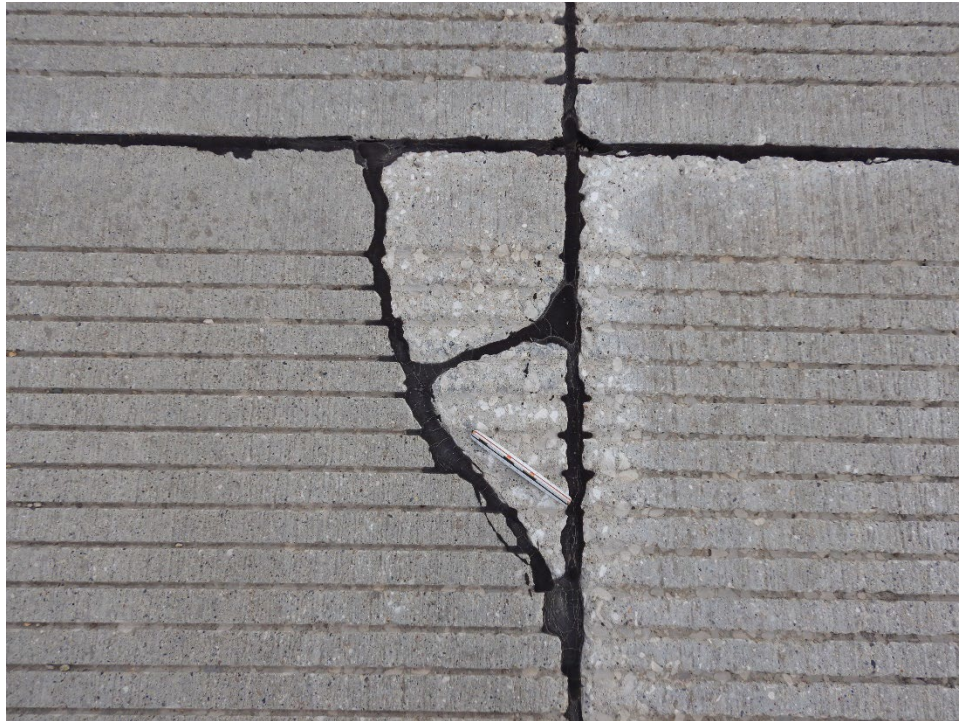
R12FD-04. Corner Spalling (Sample Unit No. 12).
