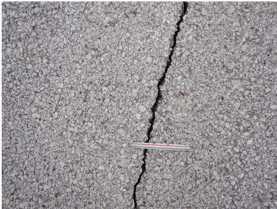
TBFD-02. L&T Cracking (Sample Unit No. 09).
