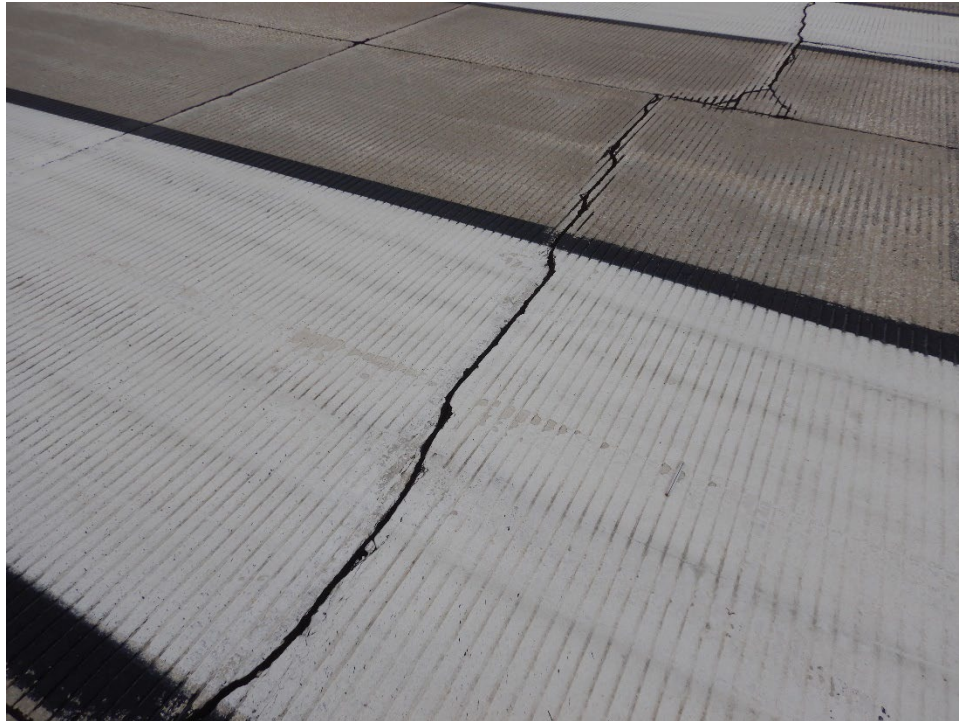
R12FD-03. LTD Cracking (Sample Unit No. 02).
