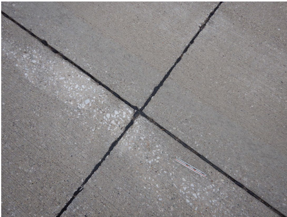
TCFD-01. Joint Seal Damage (Sample Unit No. 12).
