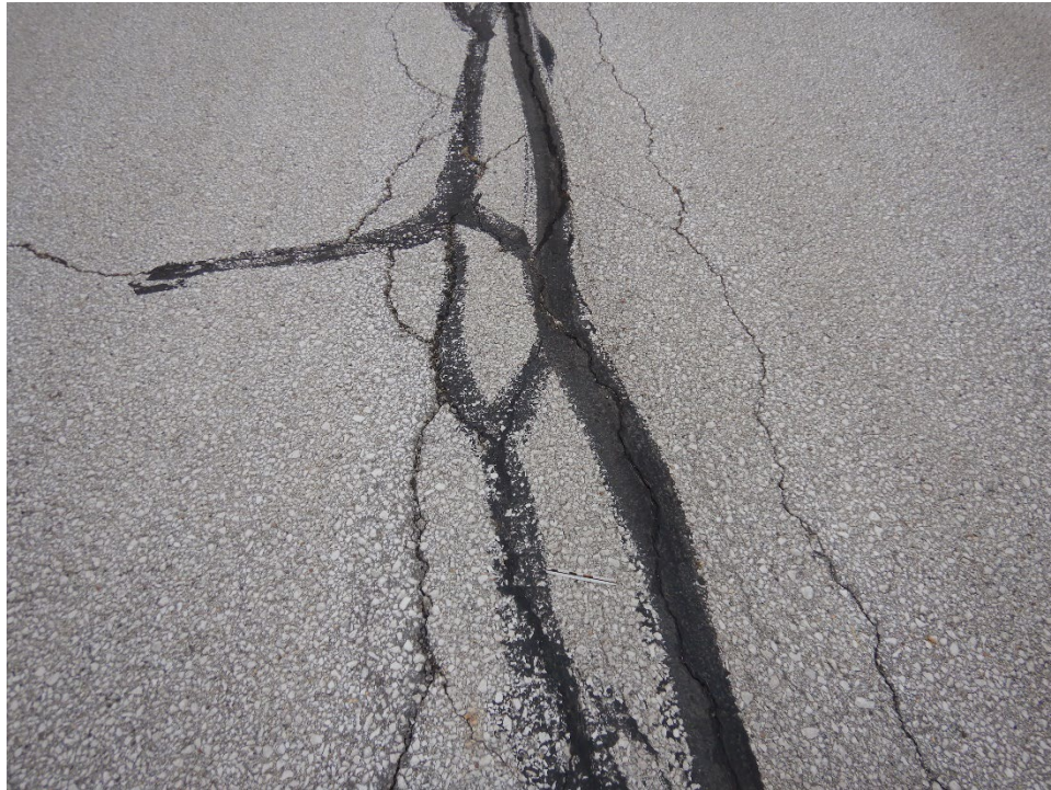
TH01FD-01. Alligator Cracking (Sample Unit No. 07).
