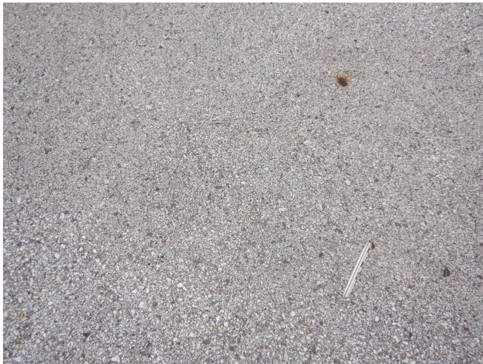
TBFD-06. Weathering (Sample Unit No. 01).
