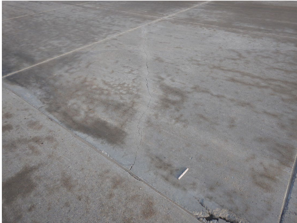
A02FD-02. LTD Cracking (Sample Unit No. 04).
