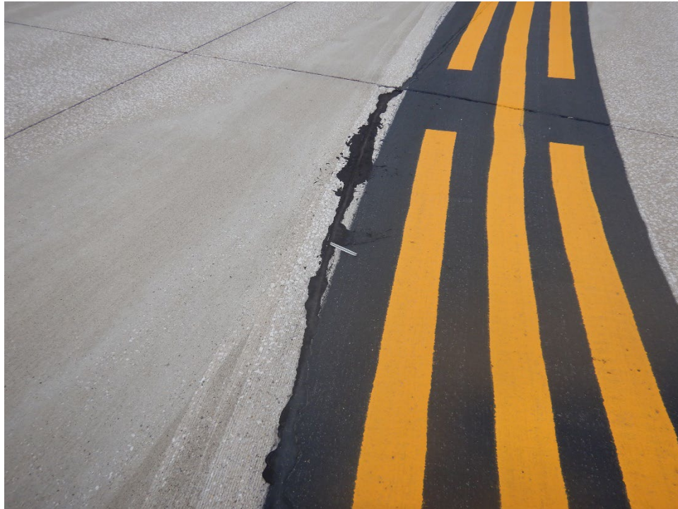
TFFD-02. LTD Cracking (Sample Unit No. 12).
