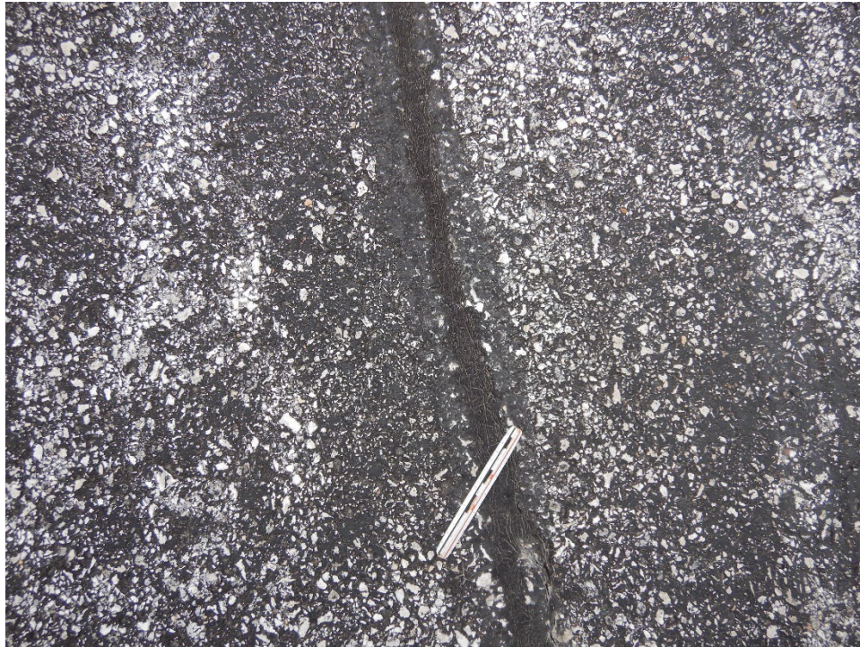
TBFD-04. L&T Cracking (Sample Unit No. 03).
