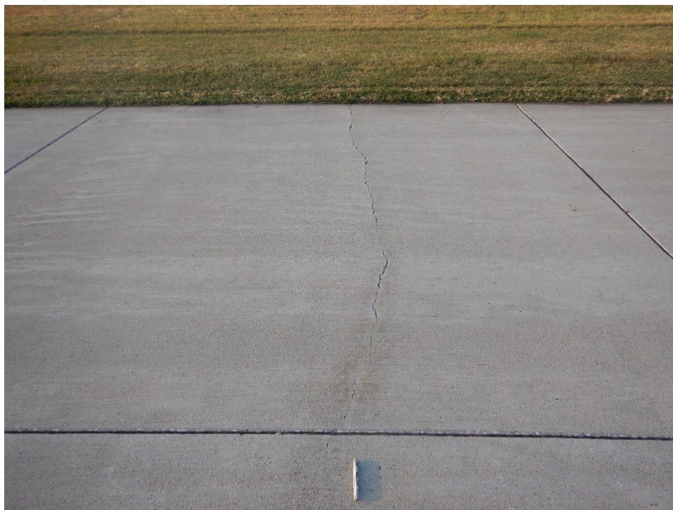
A02FD-01. LTD Cracking (Additional Sample Unit No. 14).
