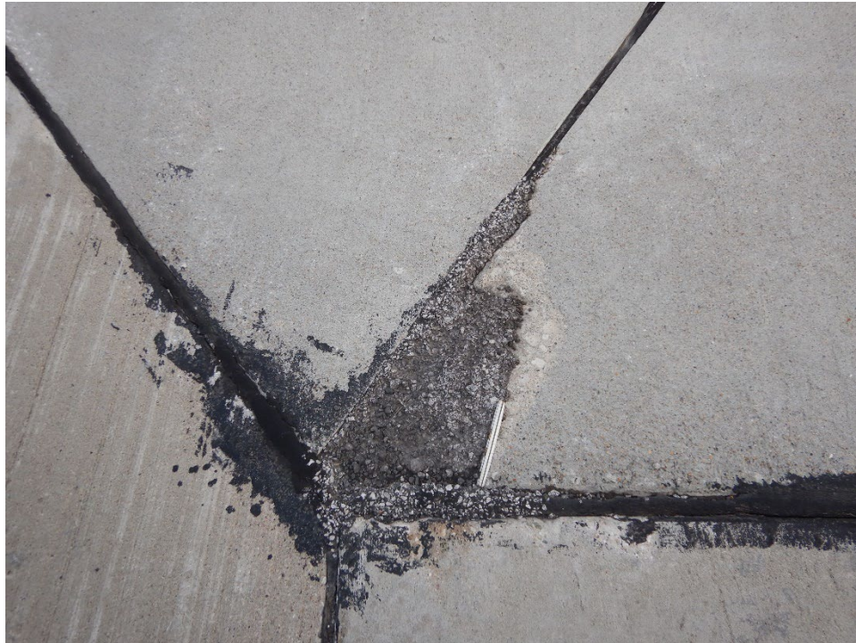
A01FD-02. Corner Spalling (Additional Sample Unit No. 15).
