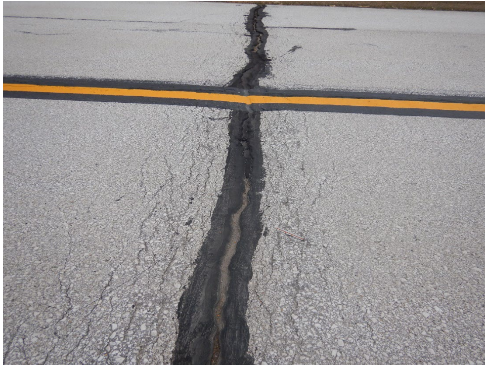
TFFD-01. L&T Cracking (Sample Unit. 05).
