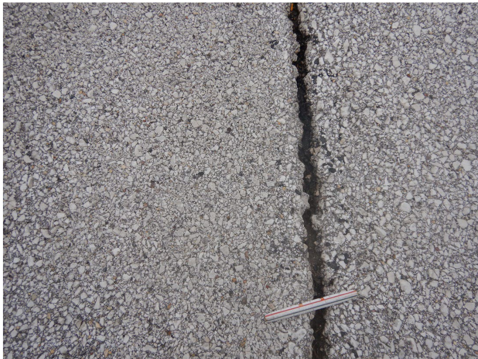
TDFD-01. L&T Cracking (Sample Unit No. 05).
