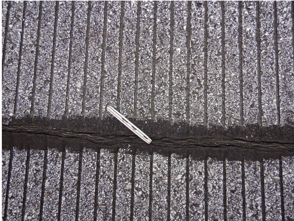
R06FD-01. L&T Cracking (Sample Unit No. 96).
