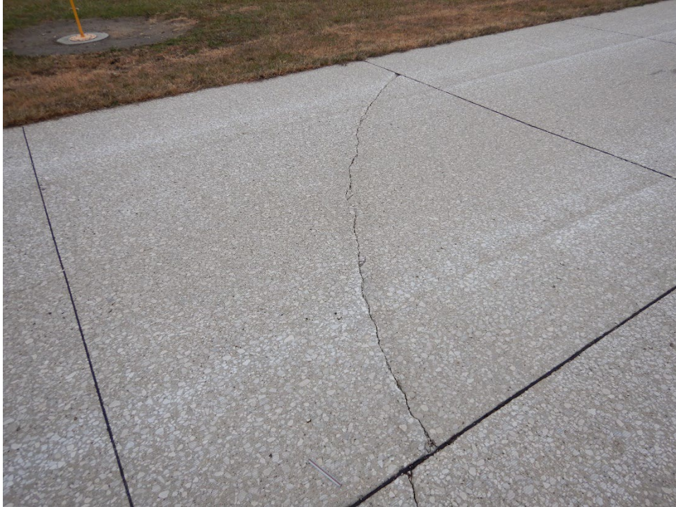
TAFD-01. LTD Cracking (Sample Unit No. 10).
