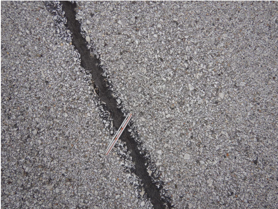
TDFD-02. L&T Cracking (Sample Unit No. 04).
