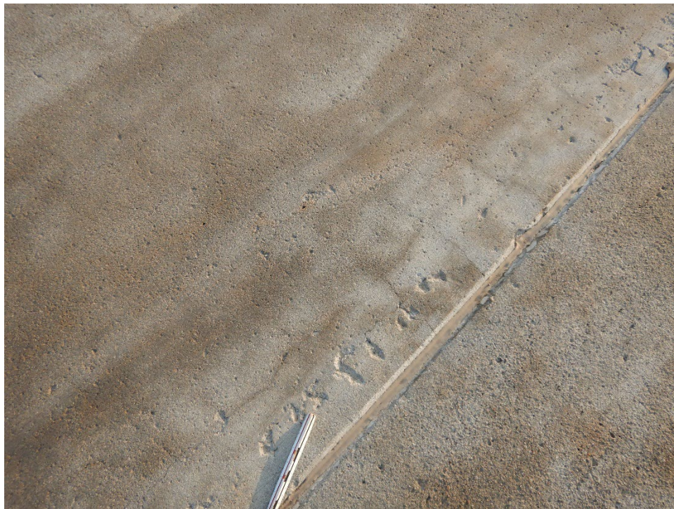
A02FD-02. Shrinkage Cracking (Sample Unit No. 04).
