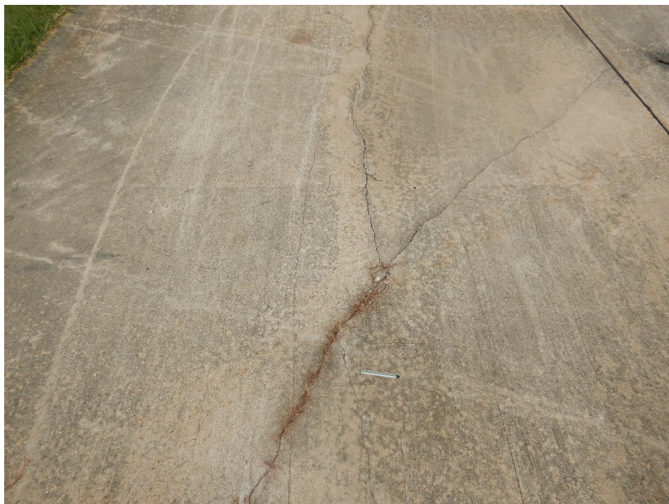
A01FM-01. Shattered Slab (Sample Unit No. 08).
