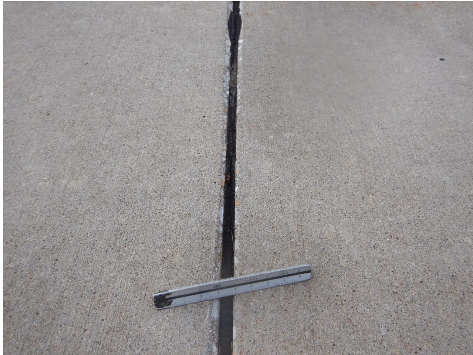
T01FM-02. Joint Seal Damage (Sample Unit No. 02).
