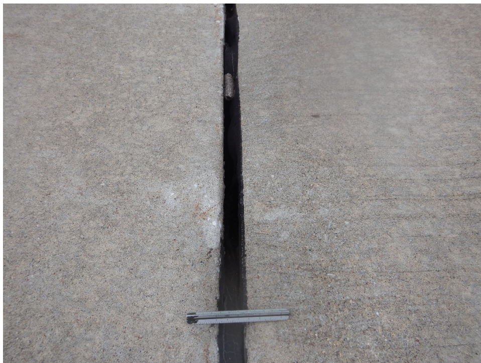
TH01FM-01. Joint Seal Damage (Sample Unit No. 04).
