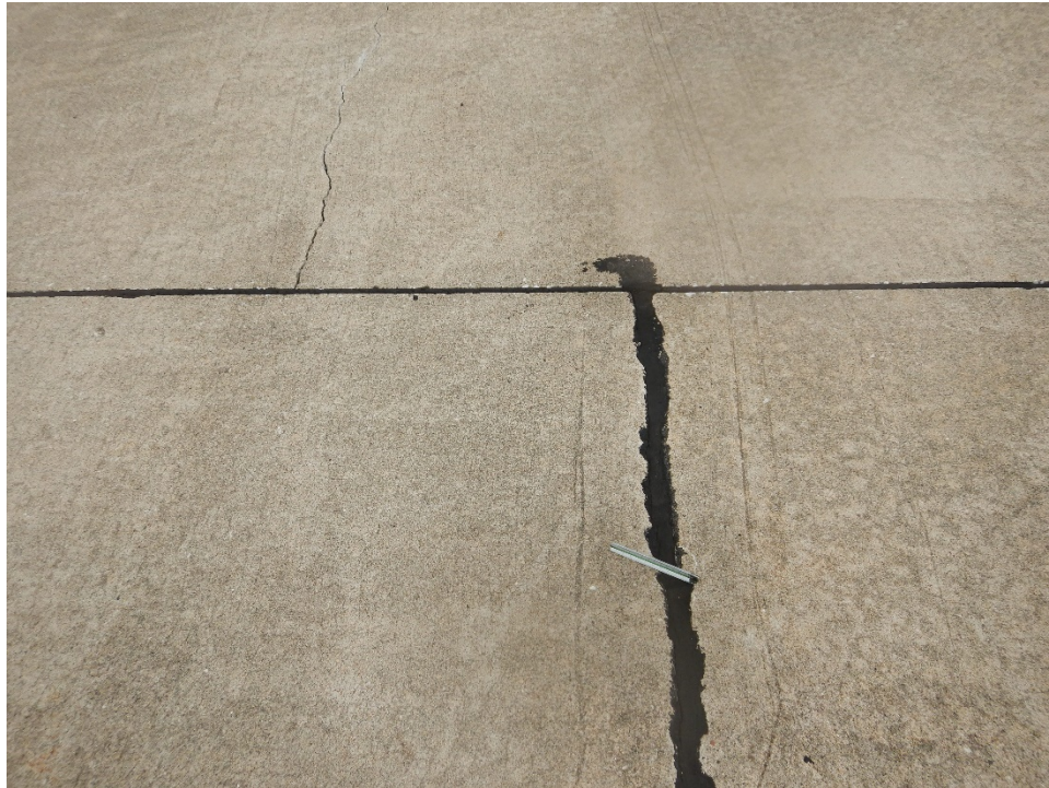
A01FM-02. LTD Cracking (Sample Unit No. 01).
