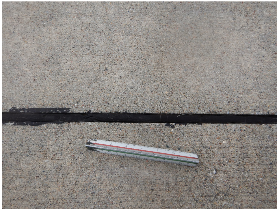
T05FM-01. Joint Seal Damage (Sample Unit No. 03).
