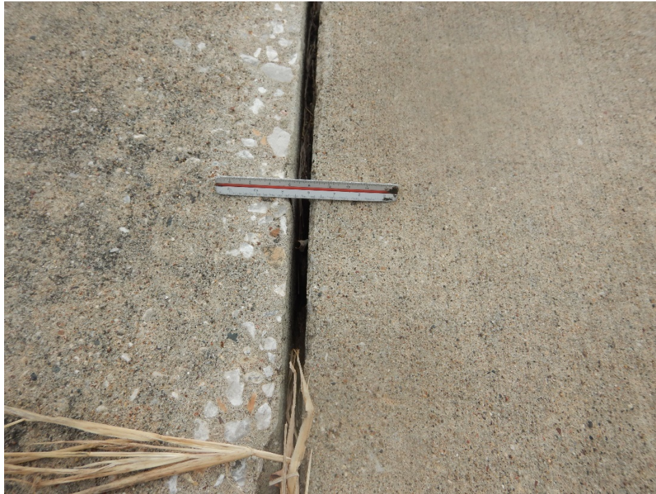
T06FM-01. Joint Seal Damage (Sample Unit No. 03).
