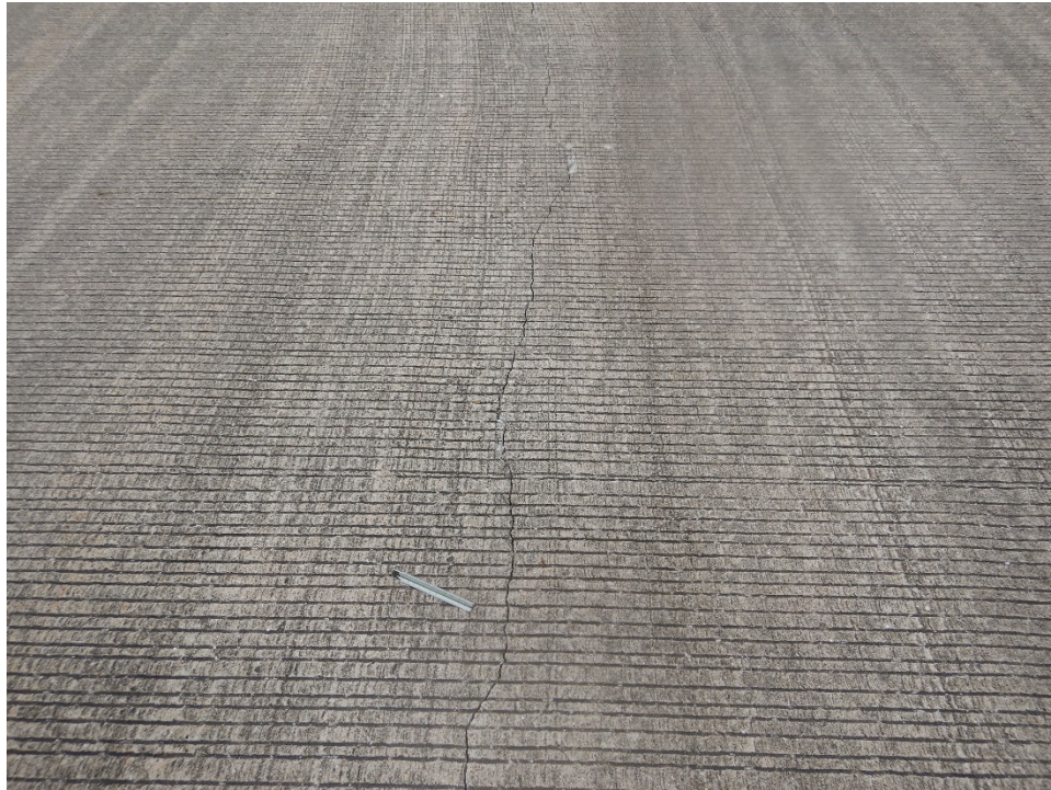
R17FM-01. LTD Cracking (Sample Unit No. 08).
