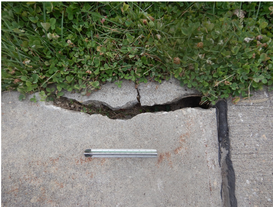
TH02FM-01. Joint Spalling (Sample Unit No. 05).
