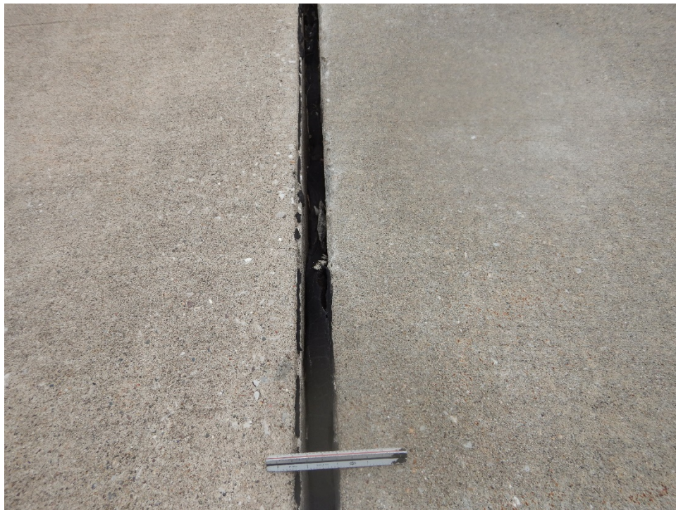
A01FM-02. Joint Seal Damage (Sample Unit No. 01).
