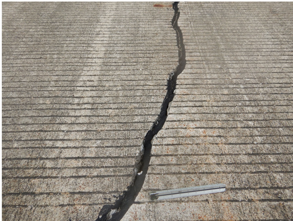
R17FM-01. LTD Cracking (Sample Unit No. 48).
