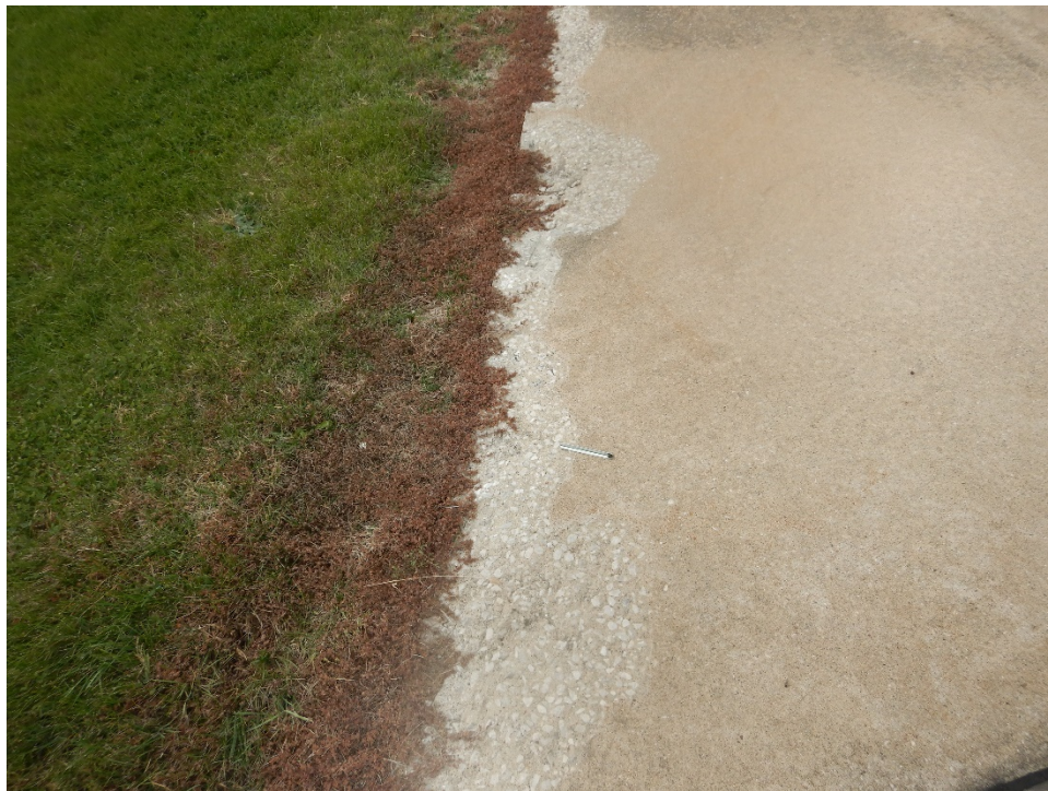
T01FM-01. Joint Spalling (Sample Unit No. 01).
