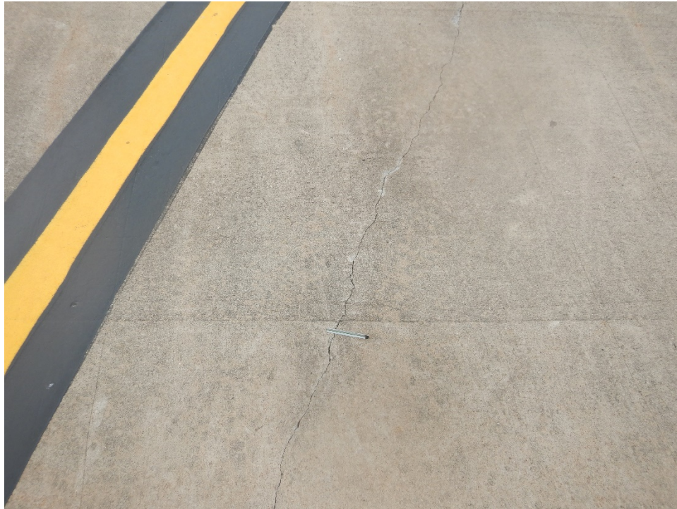
T01FM-01. LTD Cracking (Sample Unit No. 02).
