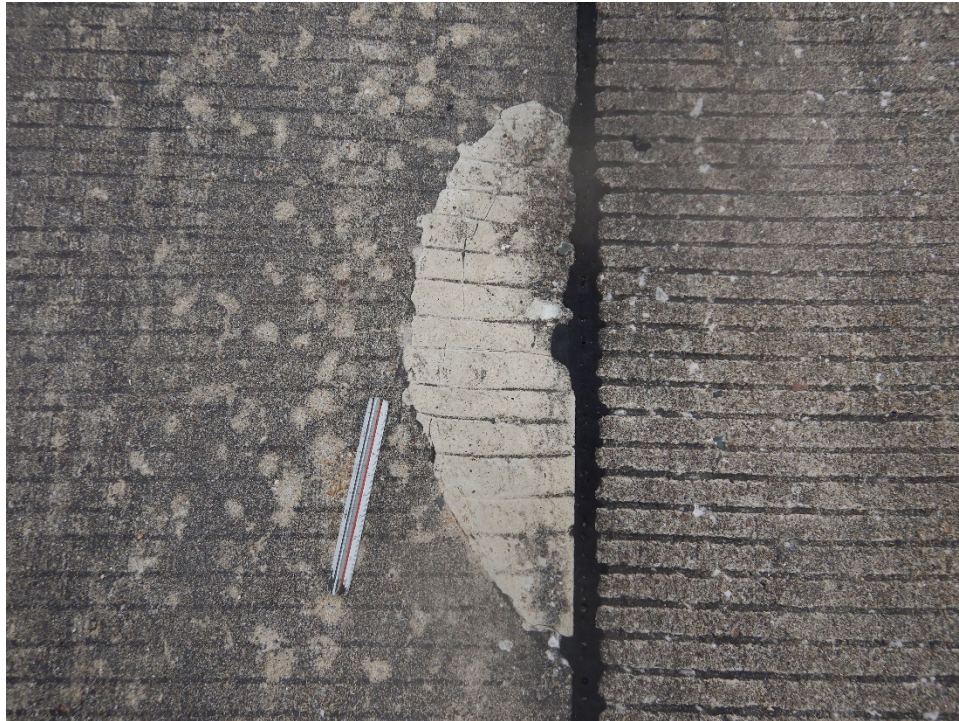
R17FM-01. Small Patching (Sample Unit No. 08).
