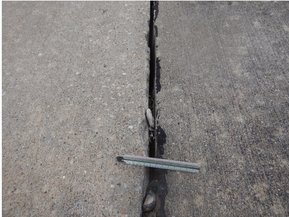
T05FM-01. Joint Seal Damage (Sample Unit No. 02).
