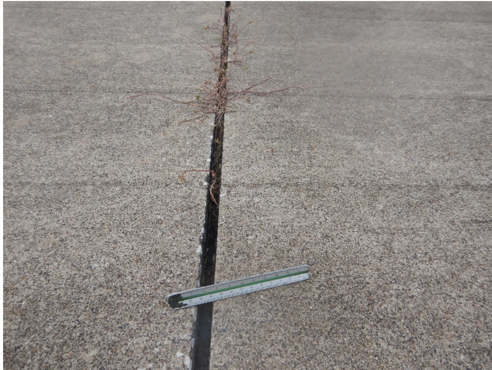
A01FM-01. Joint Seal Damage (Sample Unit No. 05).
