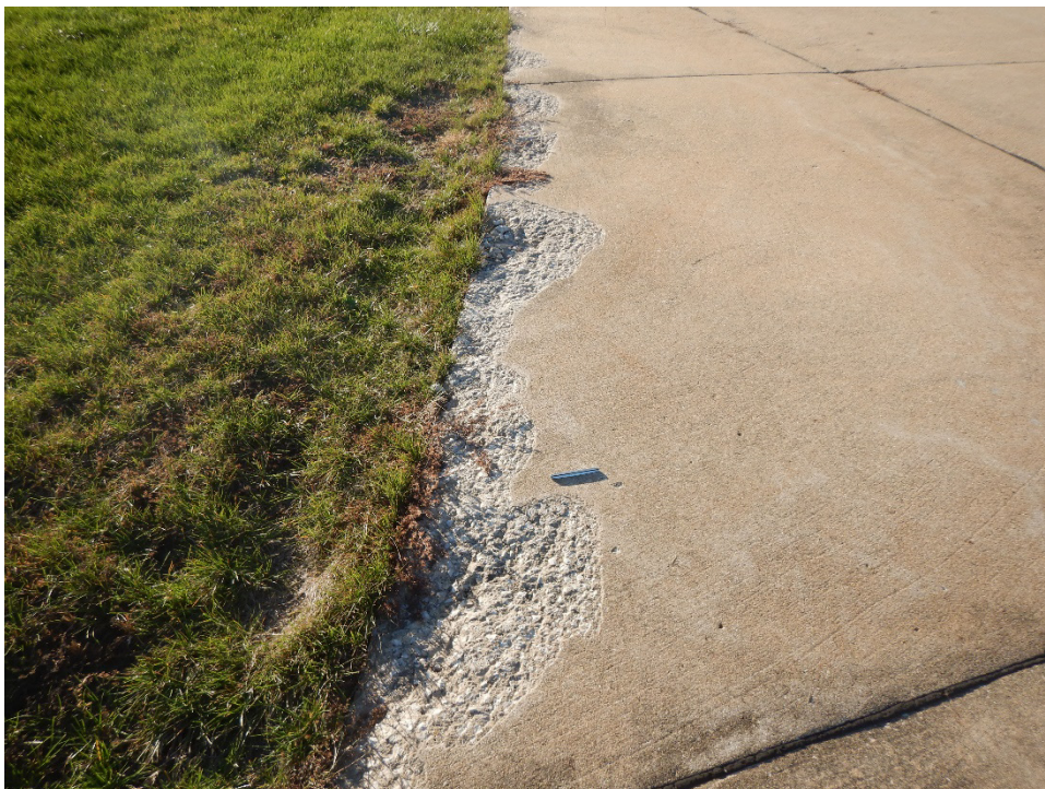
T01FM-01. Joint Spalling (Sample Unit No. 01).
