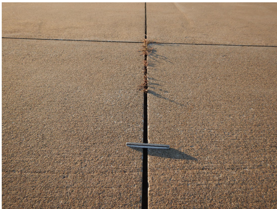
A01FM-01. Joint Seal Damage (Sample Unit No. 05).
