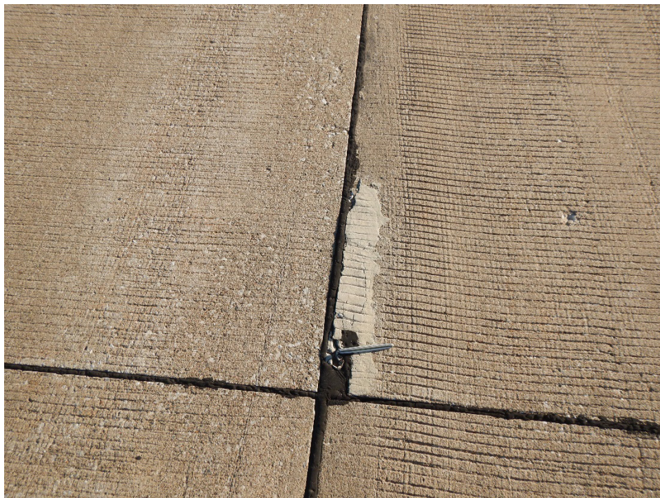
R17FM-01. Small Patching (Sample Unit No. 71).
