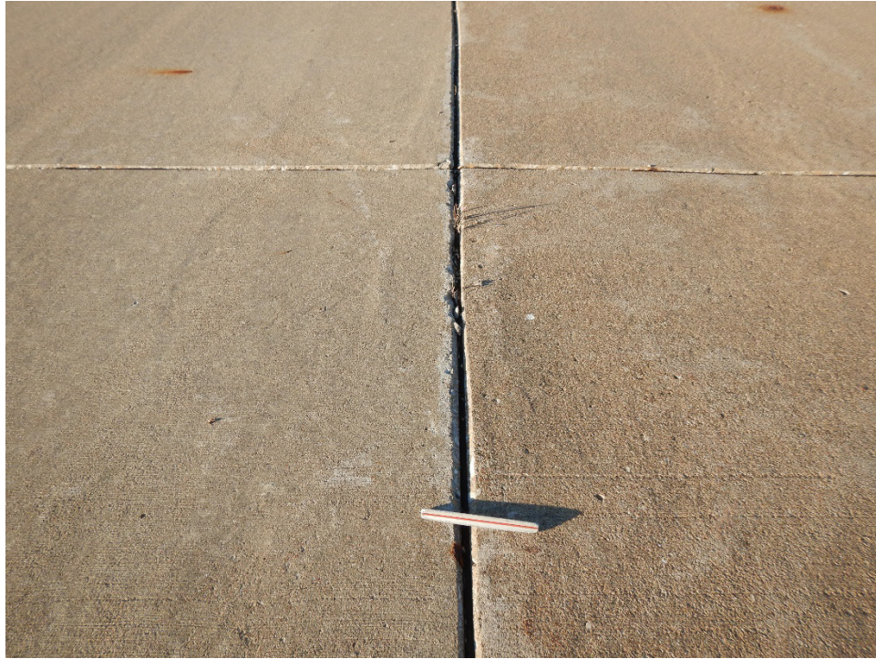
T01FM-02. Joint Seal Damage (Sample Unit No. 01).
