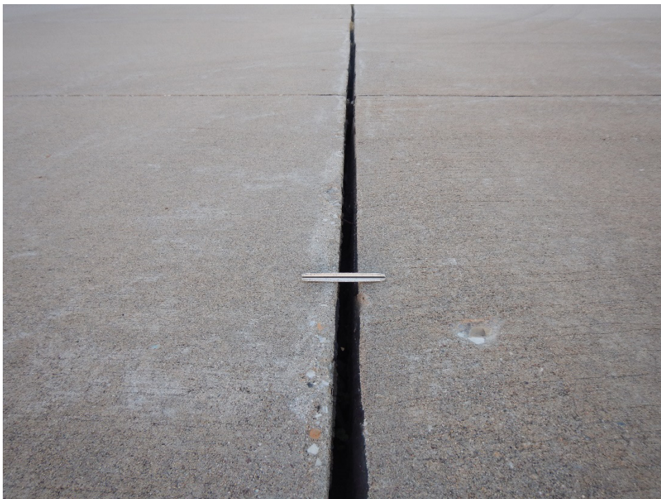
TH01FM-01. Joint Seal Damage (Sample Unit No. 04).
