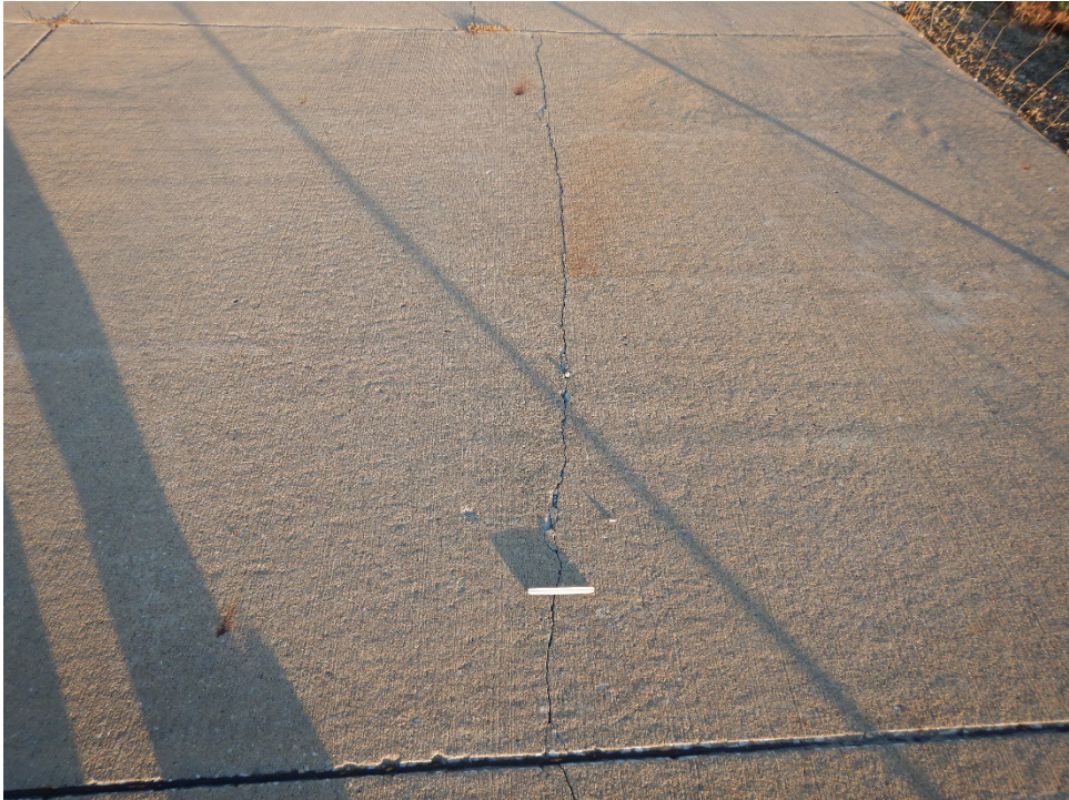
TH01FM-01. LTD Cracking (Sample Unit No. 05).
