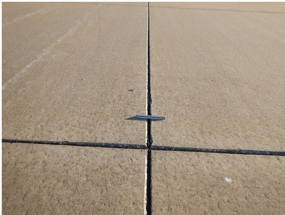
TH02FM-01. Joint Seal Damage (Sample Unit No. 02).
