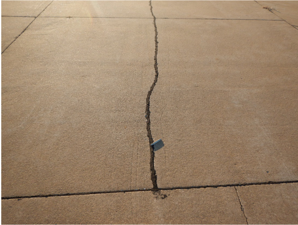
A01FM-02. LTD Cracking (Sample Unit No. 01).
