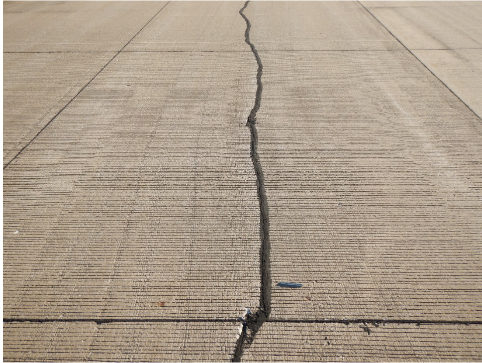
R17FM-01. LTD Cracking (Sample Unit No. 08).
