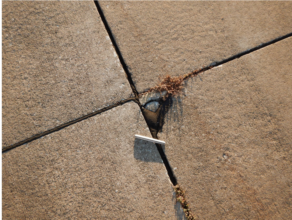
A01FM-01. Corner Spalling (Sample Unit No. 01).
