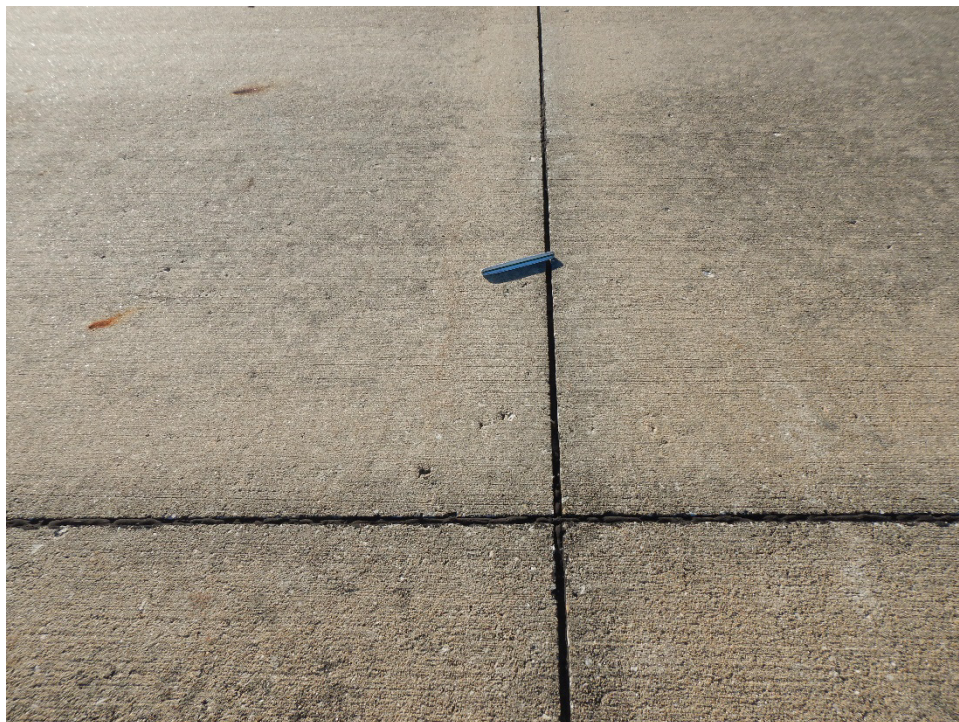
T05FM-01. Joint Seal Damage (Sample Unit No. 03).
