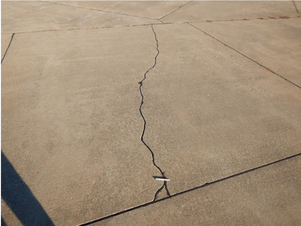
T01FM-01. LTD Cracking (Sample Unit No. 02).
