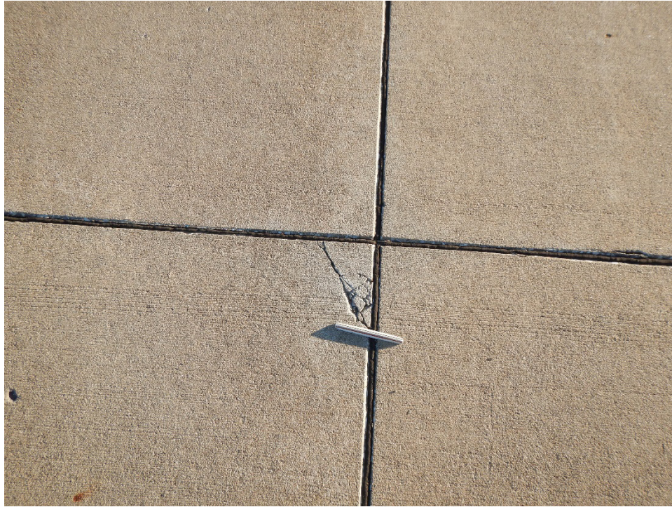
TH02FM-01. Corner Spalling (Sample Unit No. 01).
