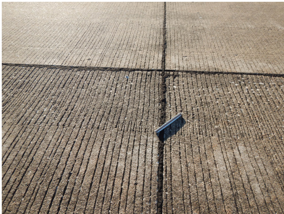
R17FM-01. Joint Seal Damage (Sample Unit No. 62).
