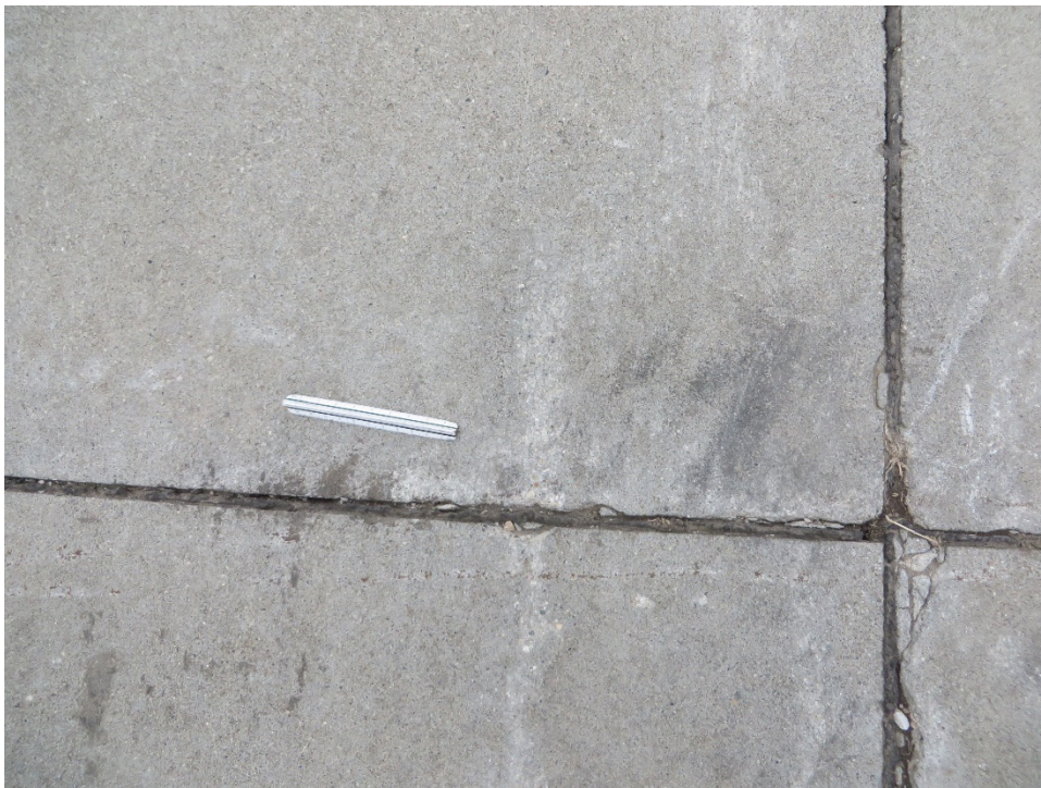
T02GC-01. Joint Seal Damage (Sample Unit No. 02).
