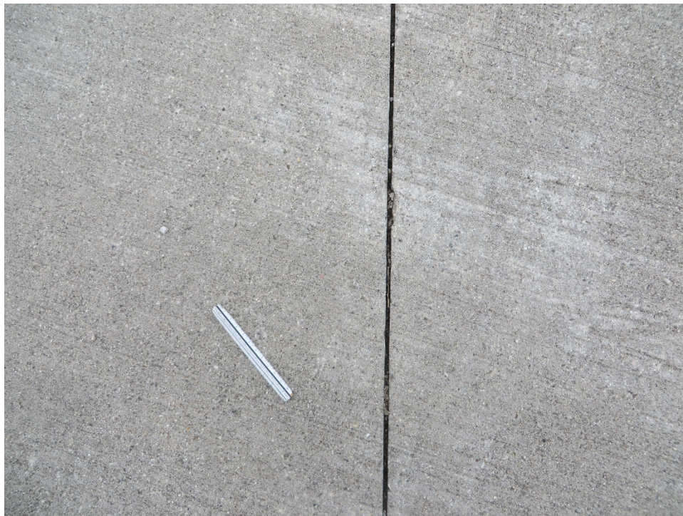
TH01GC-01. Joint Seal Damage (Sample Unit No. 02).
