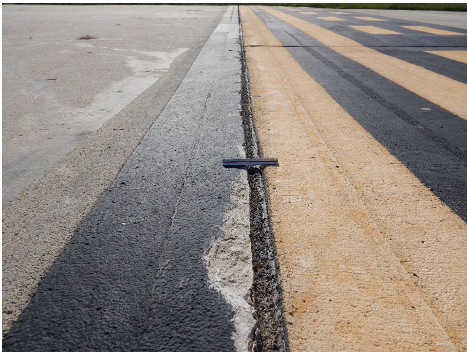
TA2GC-01. Faulting (Sample Unit No. 01).
