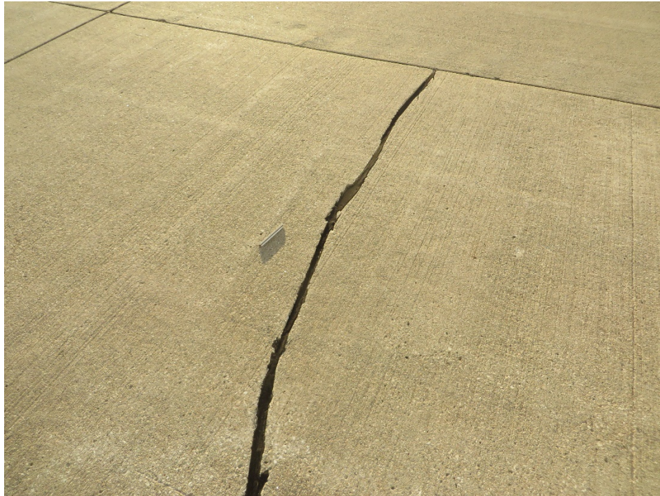
A01HA-01. LTD Cracking (Sample Unit No. 26).
