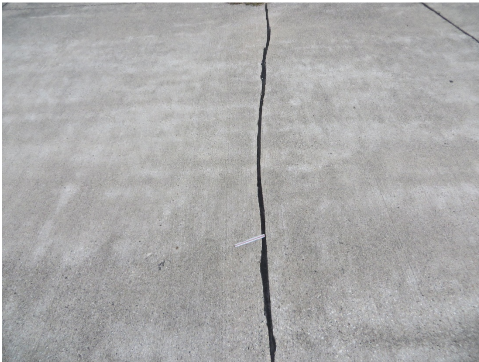
T01HA-01. LTD Cracking (Sample Unit No. 04).
