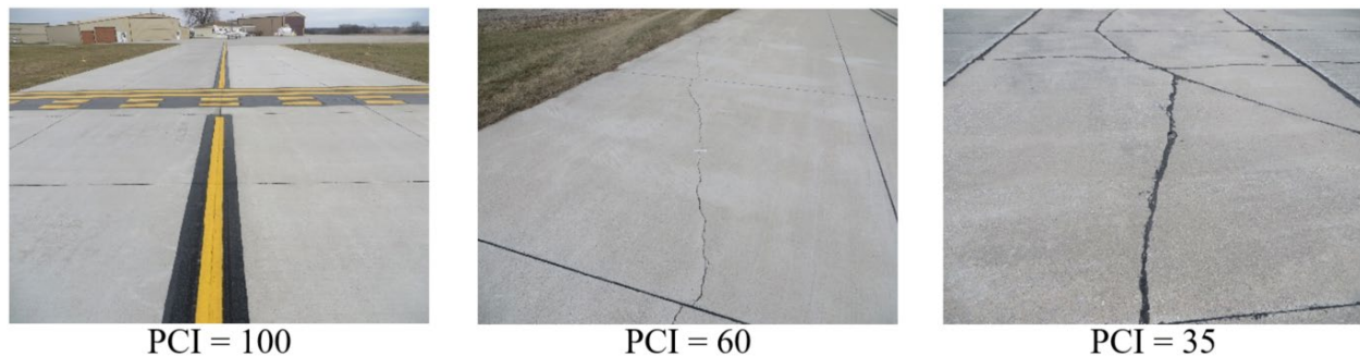
Figure 4. Visual representation of PCI scale on typical pavement surfaces.
