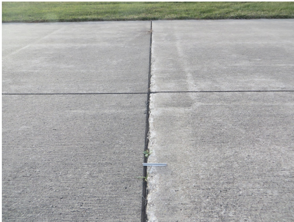
A01HA-01. Faulting (Sample Unit No. 14).
