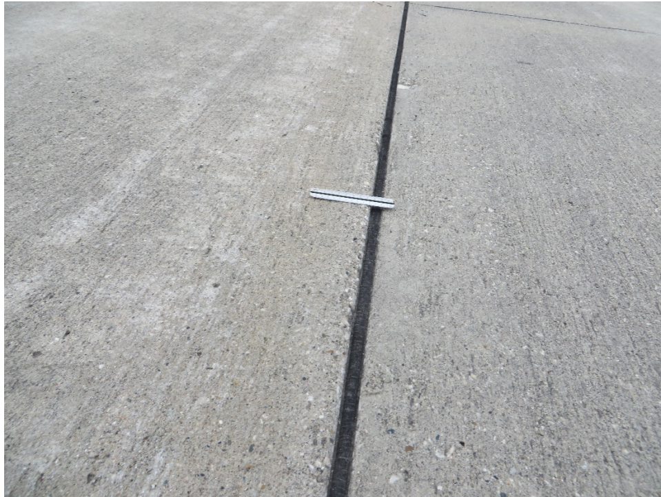
R17HA-01. Faulting (Sample Unit No. 35).
