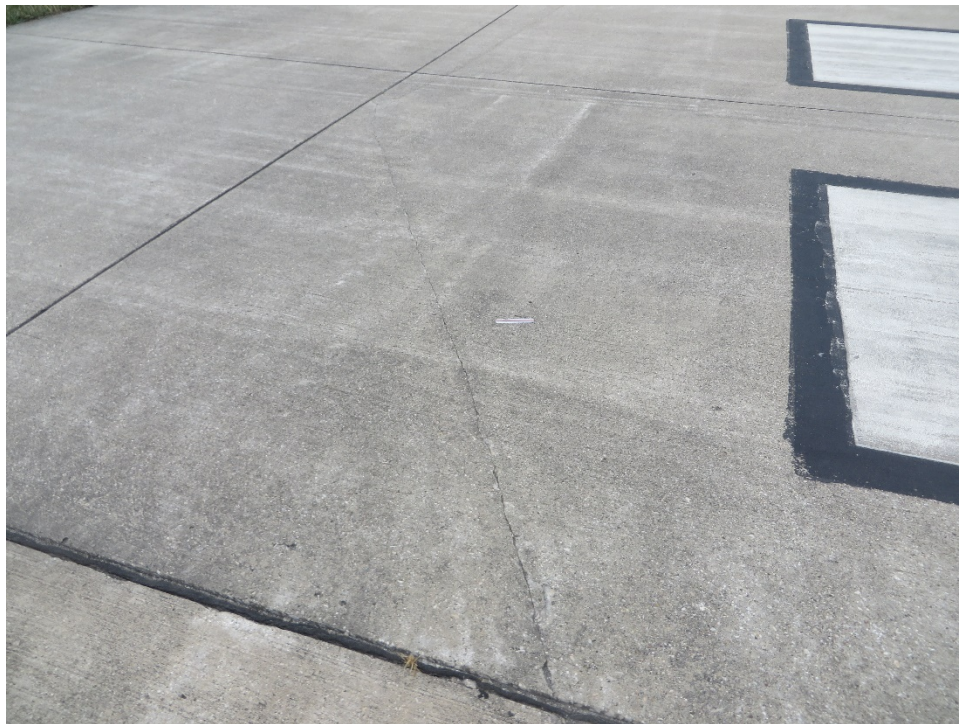
R17HA-01. LTD Cracking (Sample Unit No. 05).
