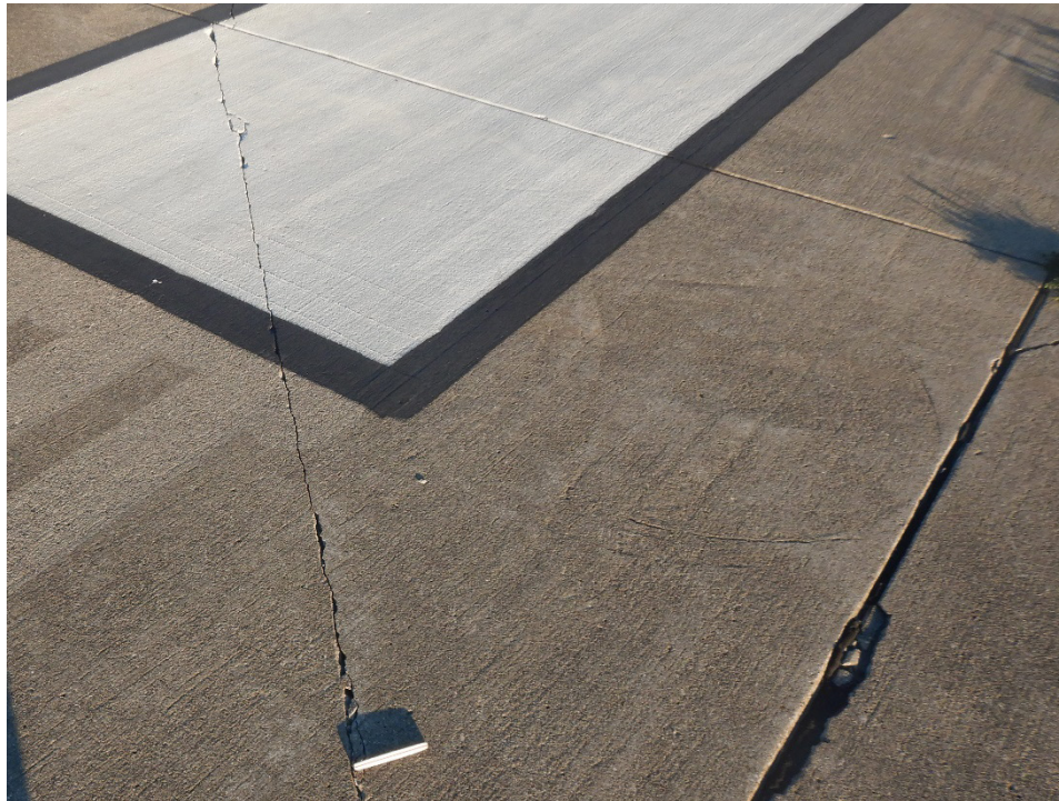
R17HA-01. LTD Cracking (Sample Unit No. 05).
