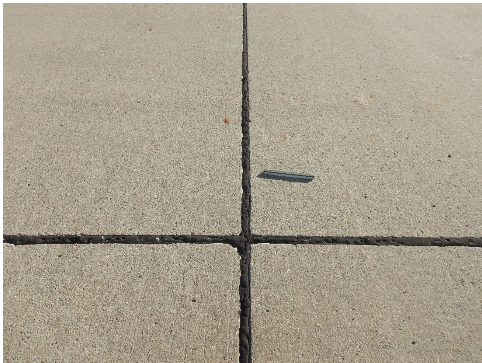
TH01HA-01. Joint Seal Damage (Sample Unit No. 07).
