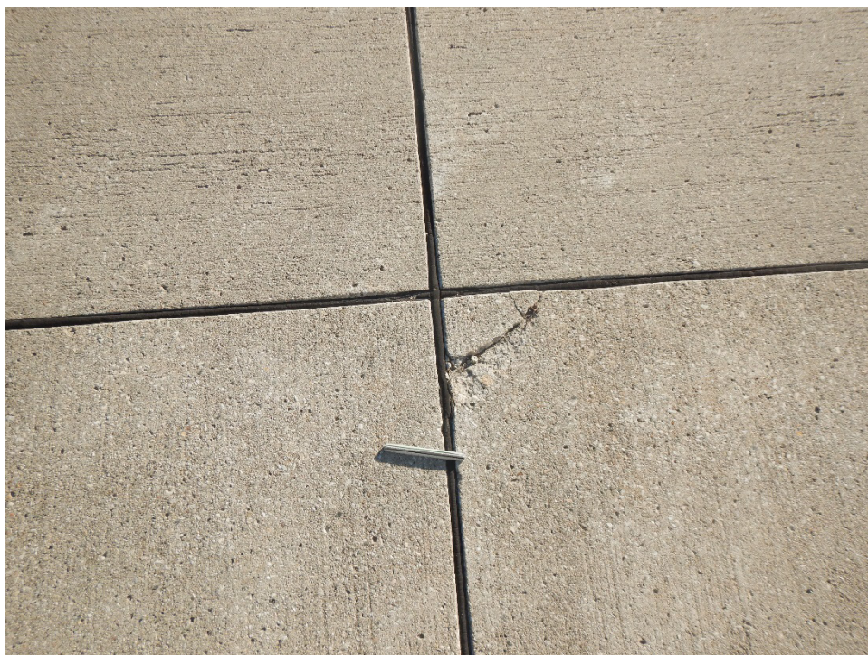
A01HA-01. Corner Spalling (Sample Unit No. 39).
