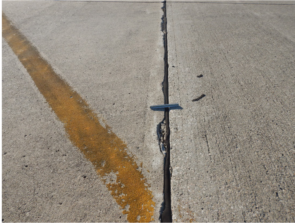
A01HA-01. Joint Seal Damage (Sample Unit No. 10).
