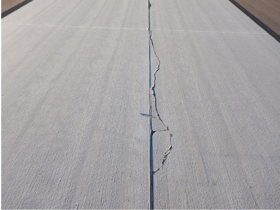
R17HA-01. Joint Spalling (Sample Unit No. 25).
