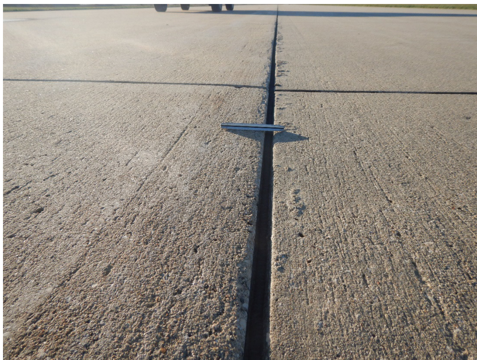
R17HA-01. Faulting (Sample Unit No. 35).
