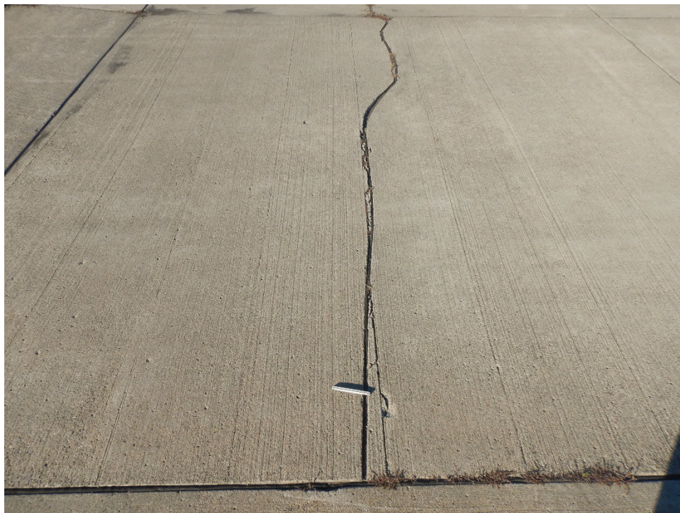
A01HA-01. LTD Cracking (Additional Sample Unit No. 18).
