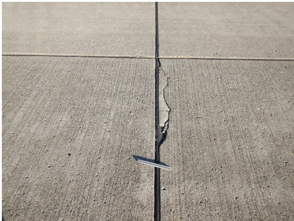
TAHA-01. Joint Seal Damage (Sample Unit No. 03).
