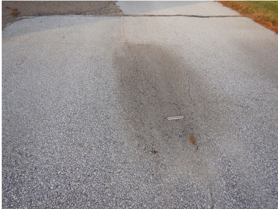
TH01HL-03. Rutting (Sample Unit No. 01).
