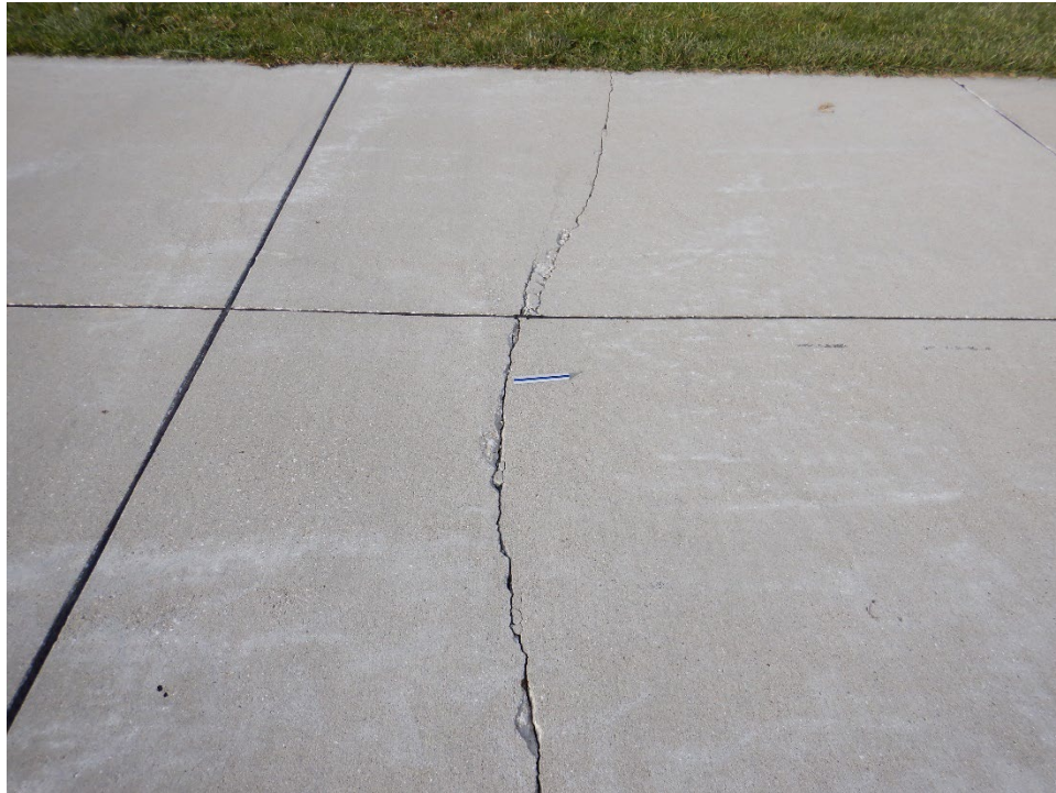
T01HL-01. LTD Cracking (Sample Unit No. 03).
