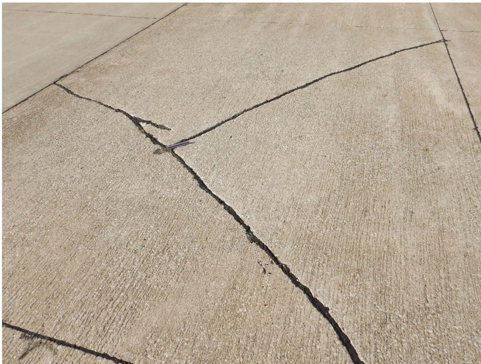
A01HL-01. LTD Cracking (Sample Unit No. 02)
