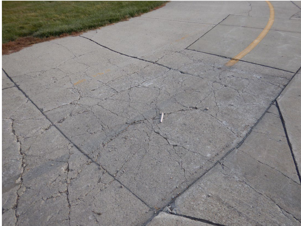
TH01HL-01. Shattered Slab (Sample Unit No. 01).
