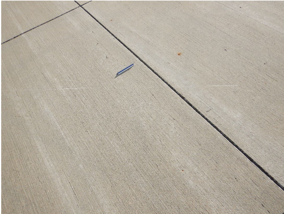
T02HL-01. LTD Cracking (Sample Unit No. 14).
