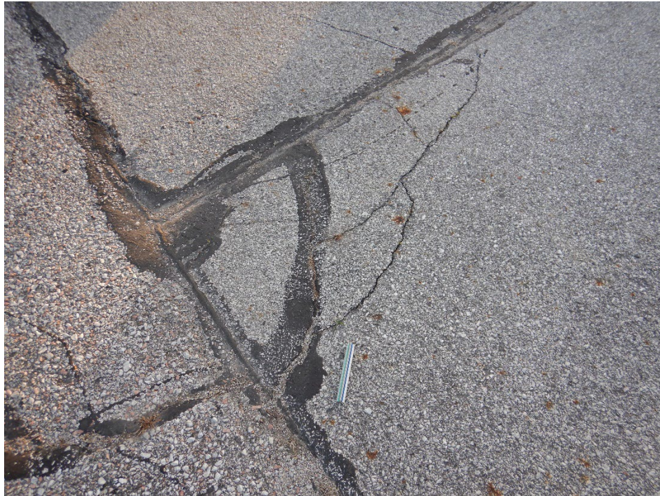
TH01HL-04. Alligator Cracking (Sample Unit No. 01).
