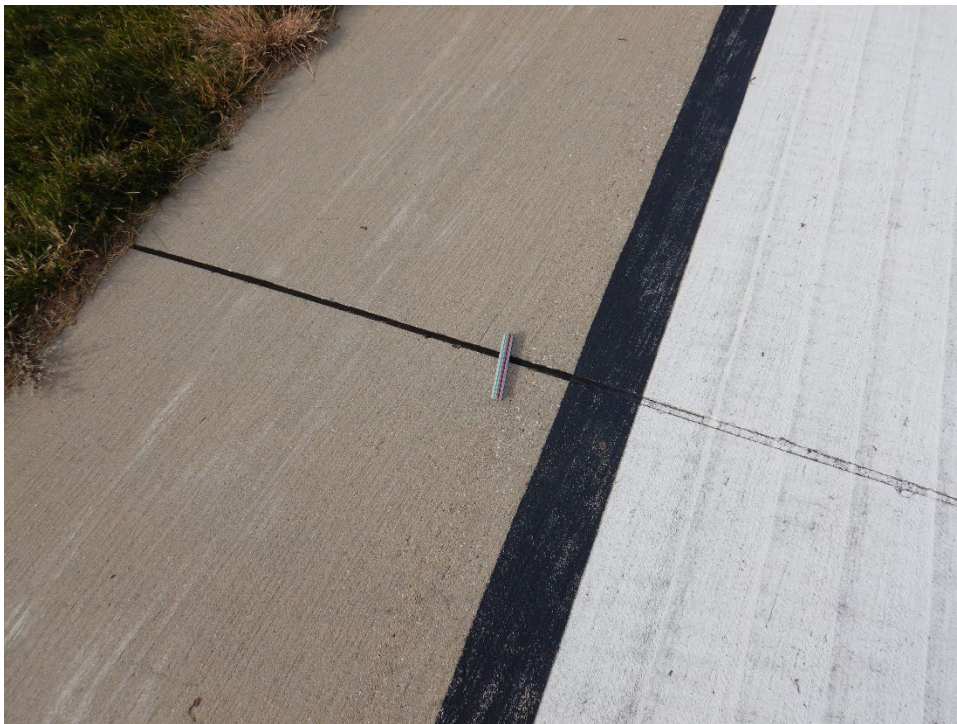
R15HL-02. Joint Seal Damage (Sample Unit No. 10).
