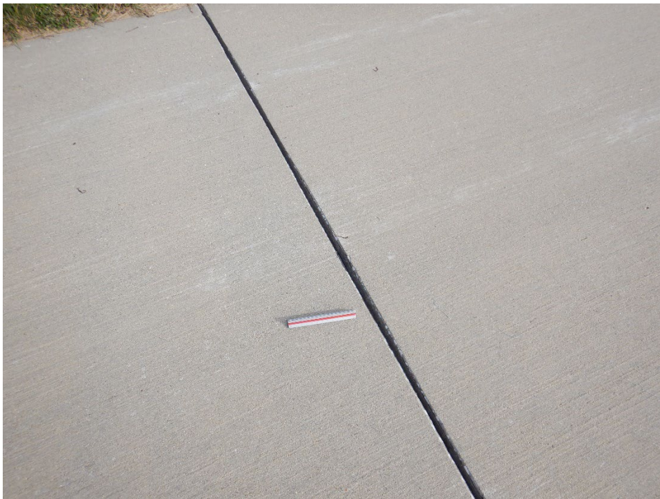
R15HL-04. Joint Seal Damage (Sample Unit No. 12).
