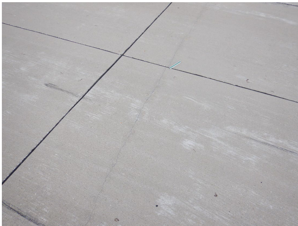
R15HL-01. LTD Cracking (Sample Unit No. 15).
