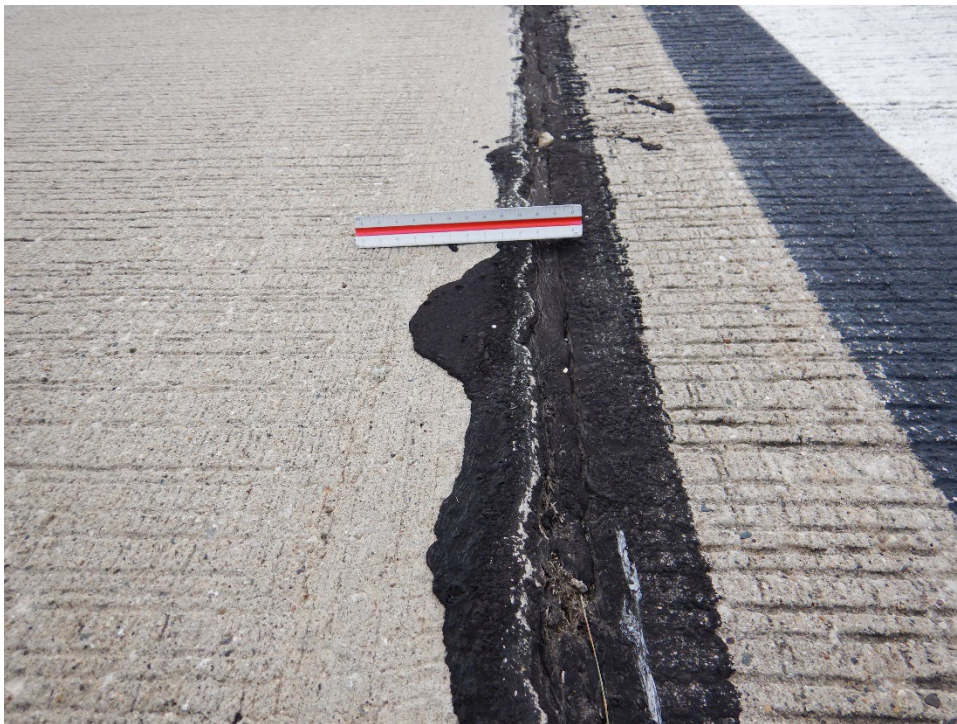
R15HL-03. Faulting (Sample Unit No. 11).
