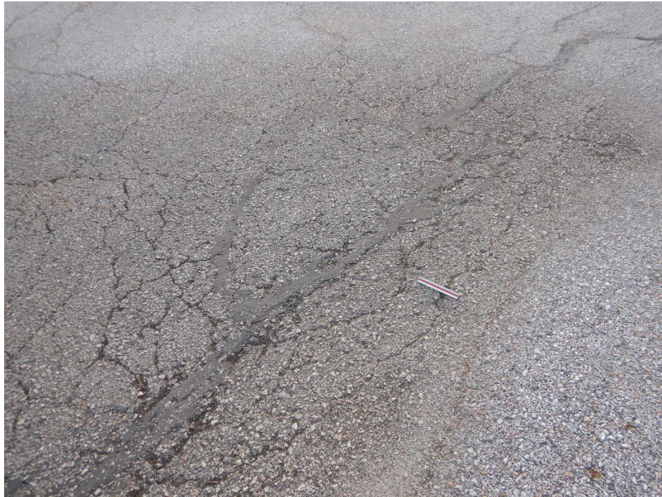
TH01HL-02. Alligator Cracking (Sample Unit No. 05).
