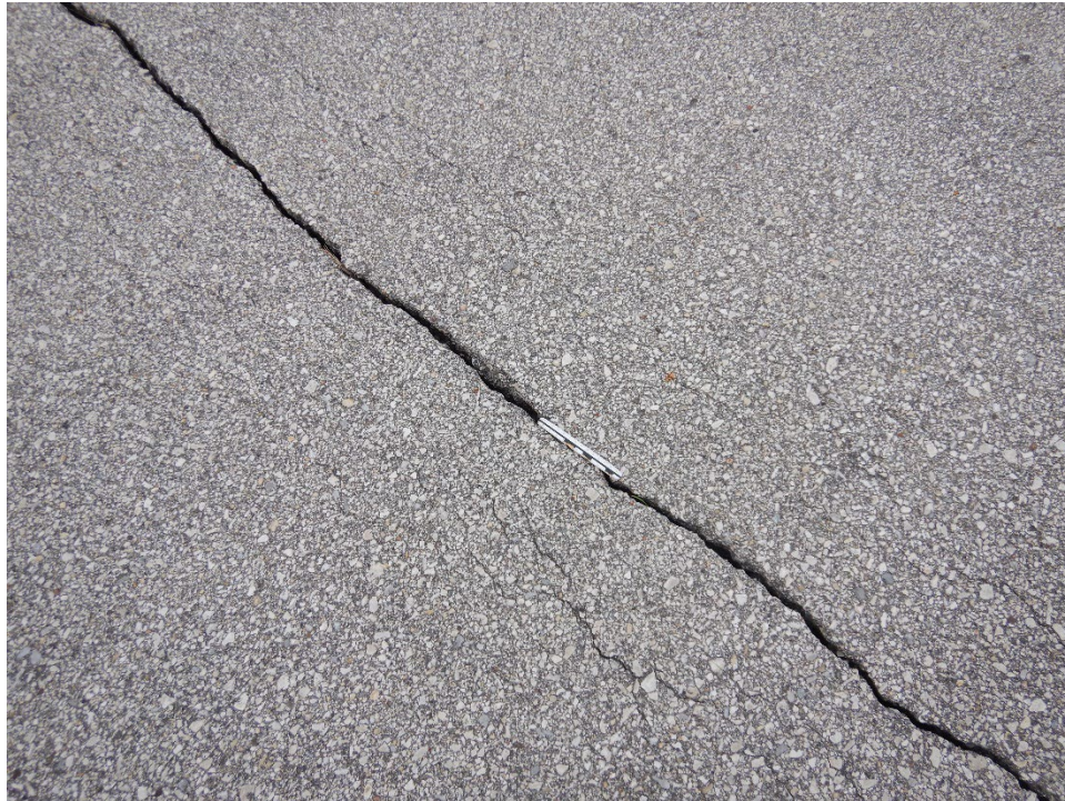
TH01HU-01. L&T Cracking (Sample Unit No. 01).
