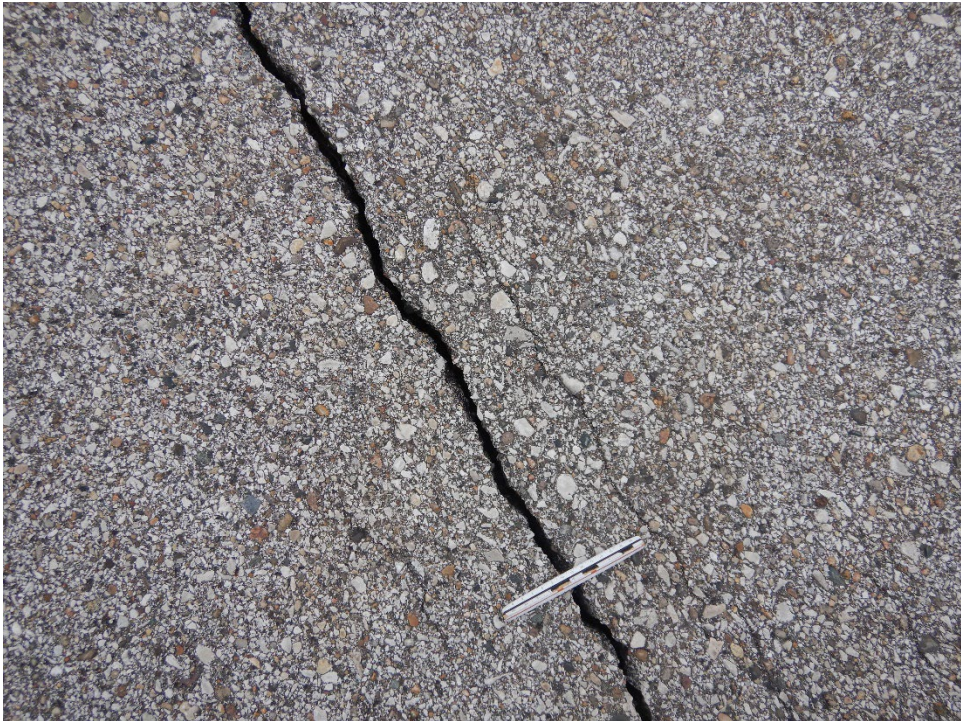
T01HU-01. L&T Cracking (Sample Unit No. 01).
