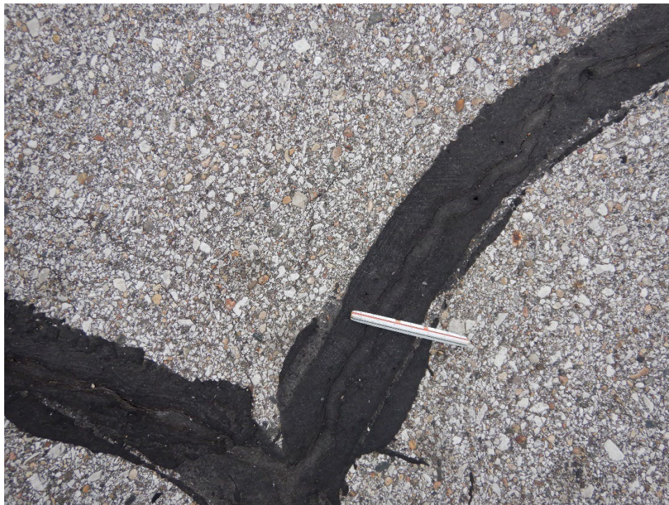
A01HU-01. L&T Cracking (Sample Unit No. 01).
