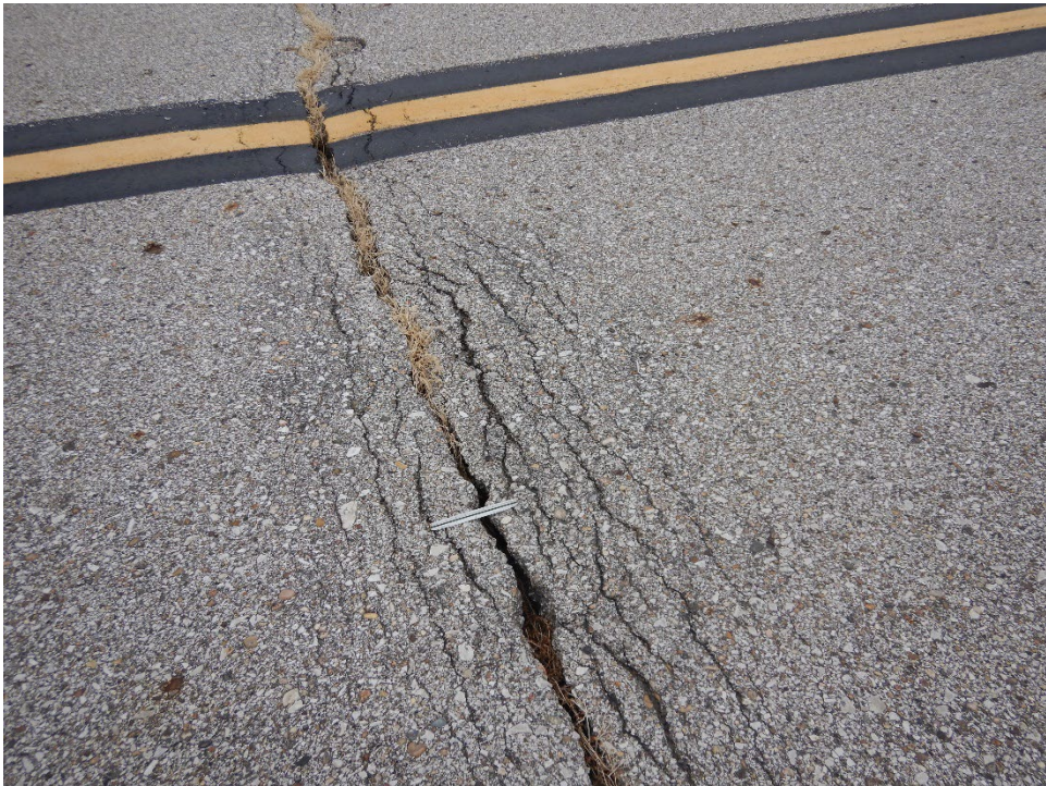
T01HU-01. L&T Cracking (Sample Unit No. 02).
