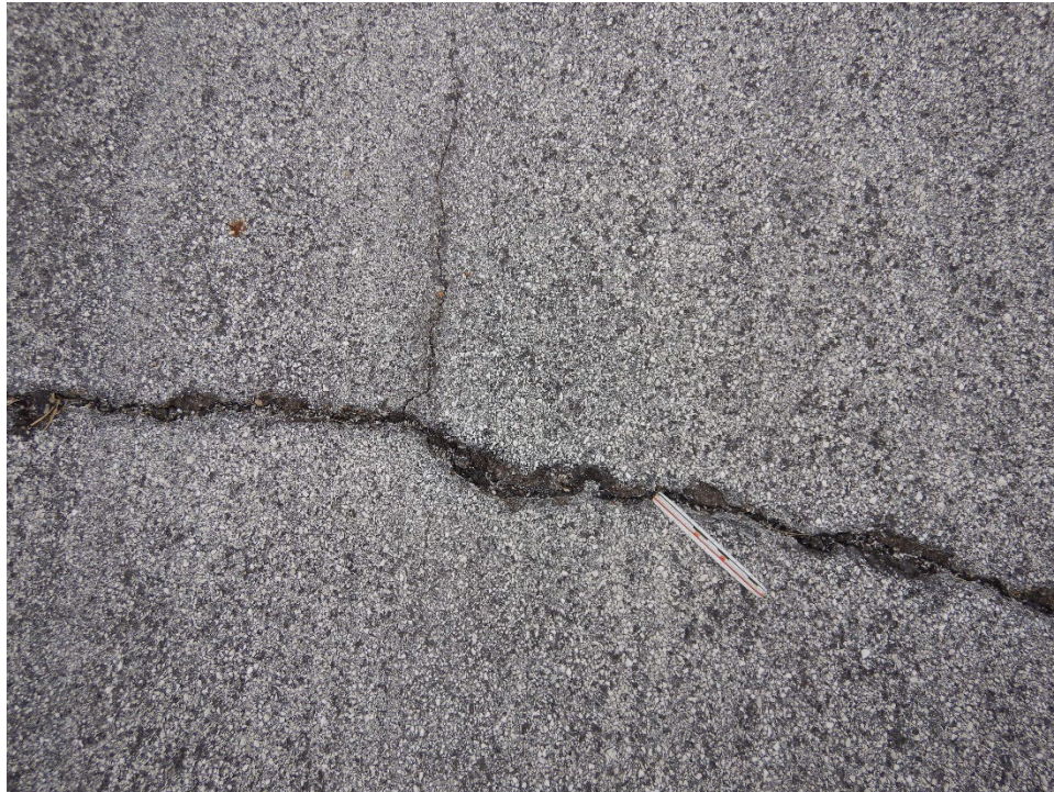
R12HU-02. L&T Cracking (Sample Unit No. 02).
