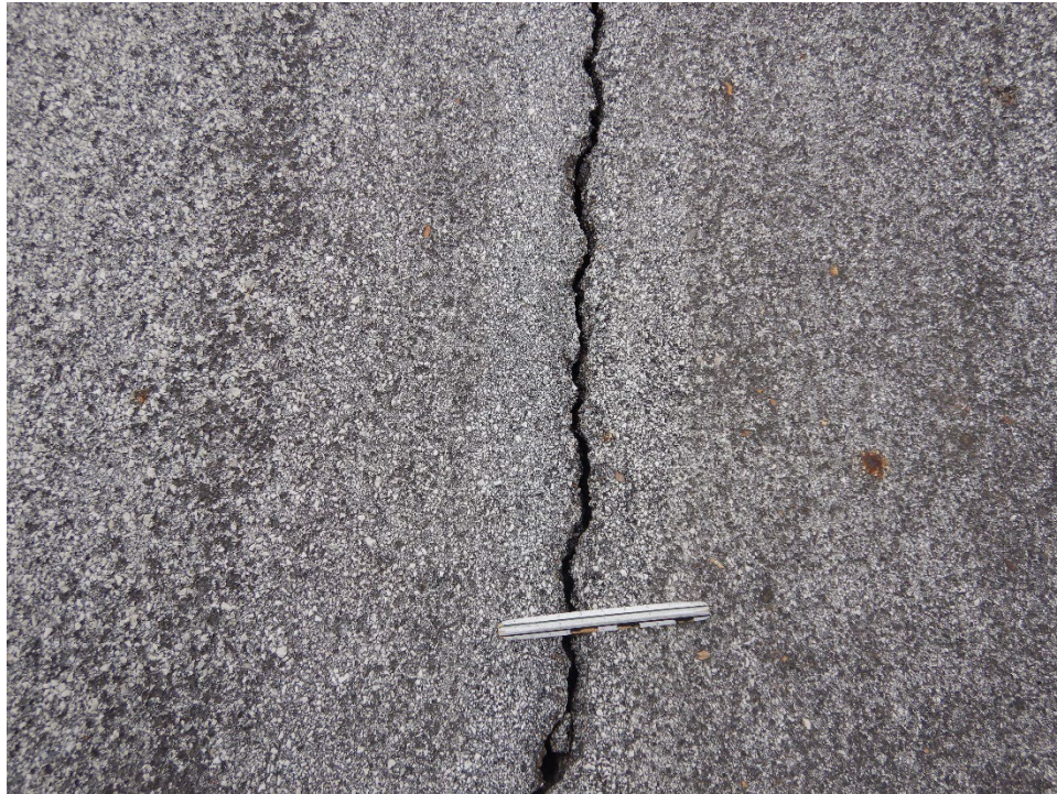
R12HU-01. L&T Cracking (Sample Unit No. 04).
