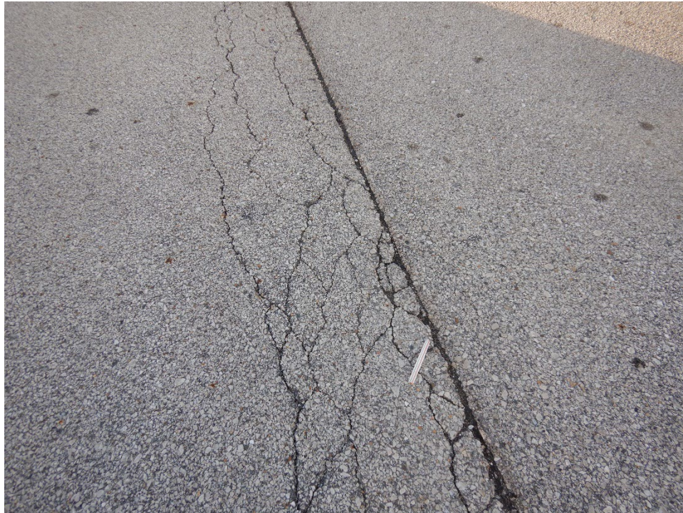
TH02IC-01. Alligator Cracking (Sample Unit No. 03) (2).
