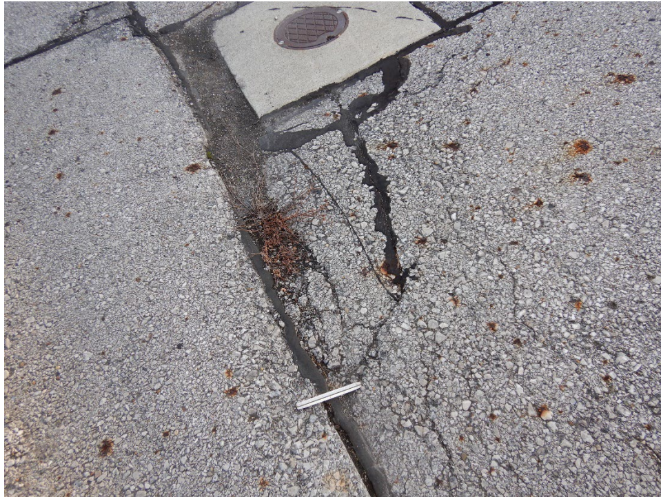
TH01IC-02. Alligator Cracking (Sample Unit No. 02).
