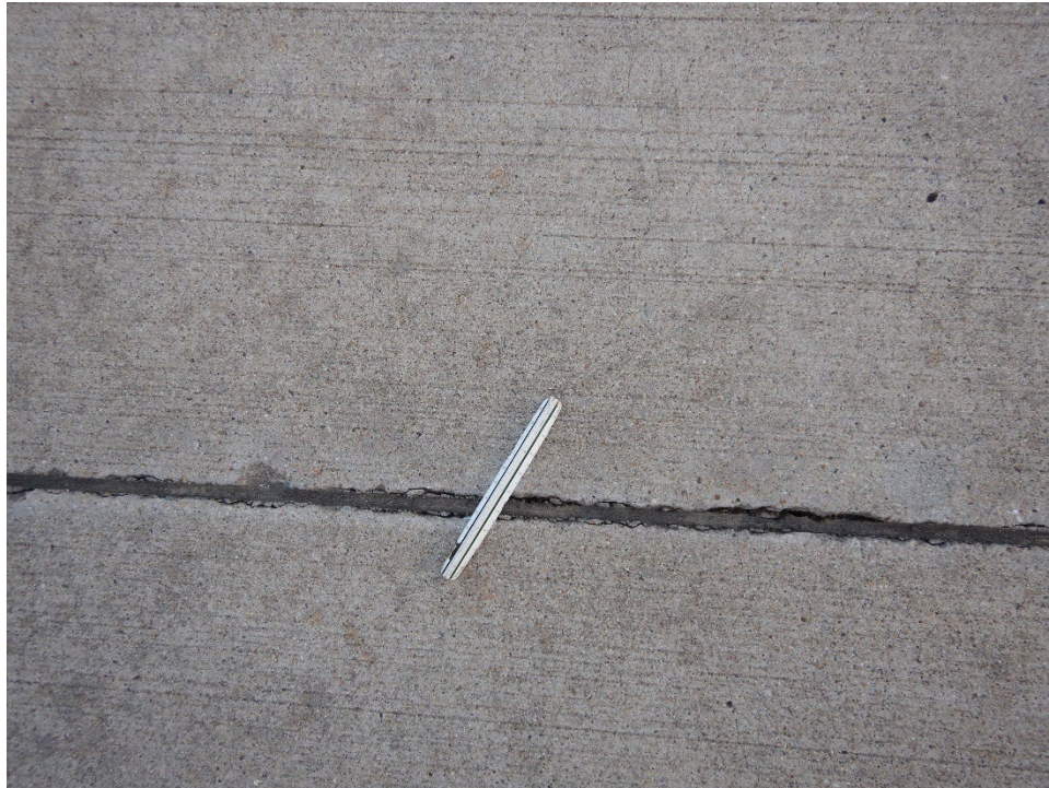
TH02IC-03. Joint Seal Damage (Sample Unit No. 01).
