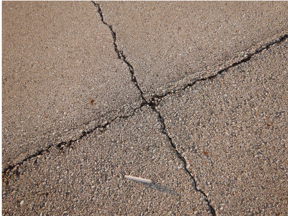
T01IC-01. Joint Reflection Cracking (Sample Unit No. 06).
