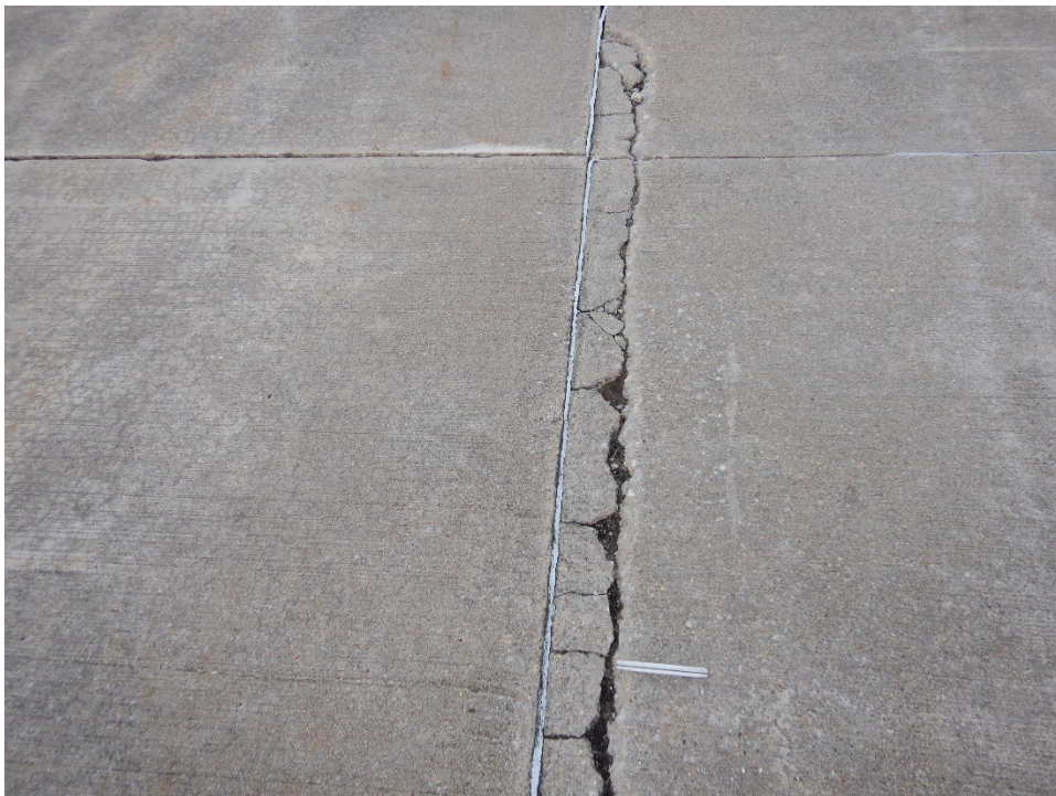
TH02IC-02. Joint Spalling (Sample Unit No. 17).
