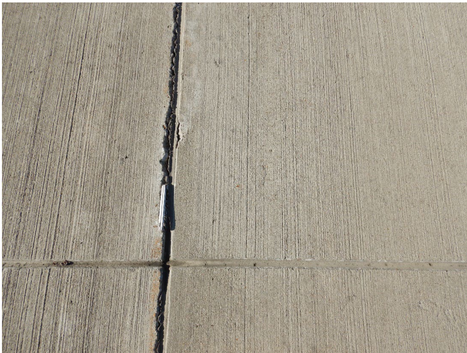
R12IC-01. Joint Seal Damage (Sample Unit No. 11).
