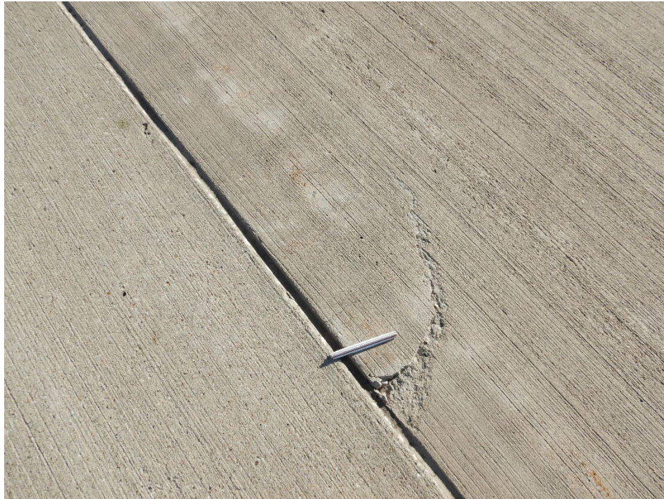
R12IC-01. Joint Spalling (Sample Unit No. 35).
