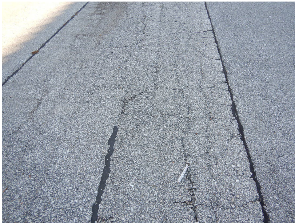
TH01IC-04. Alligator Cracking (Sample Unit No. 17).
