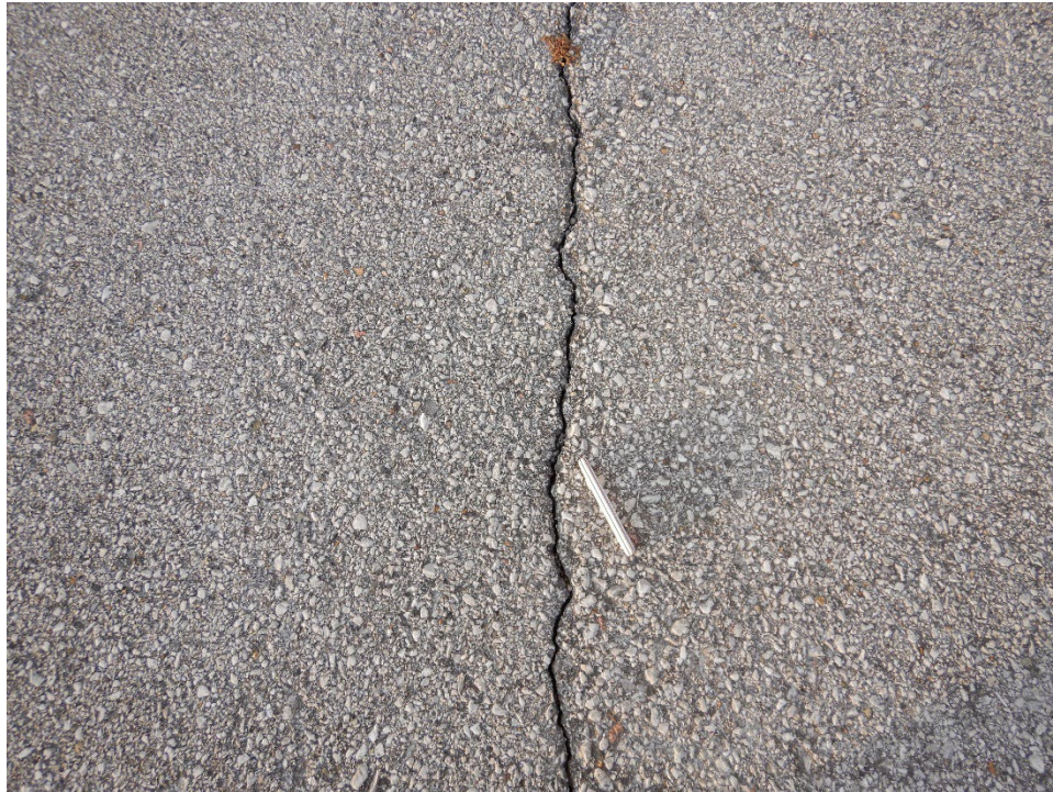
T01IC-04. L&T Cracking (Sample Unit No. 02).
