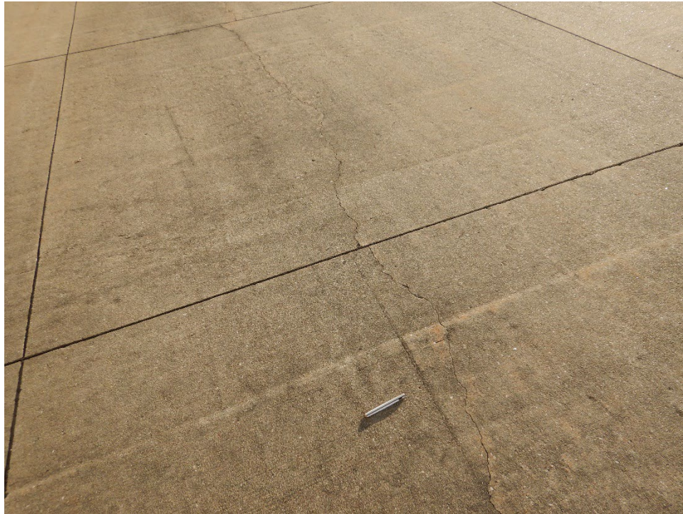
TH02IC-02. LTD Cracking (Sample Unit No. 02).
