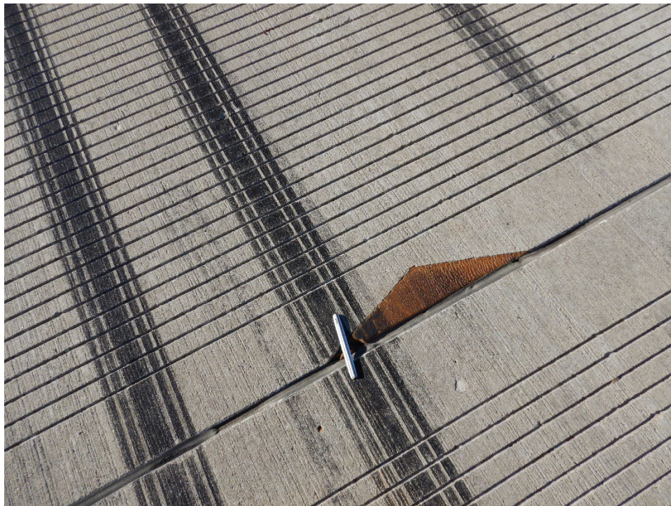
R07IC-02. Small Patching (Sample Unit No. 08).
