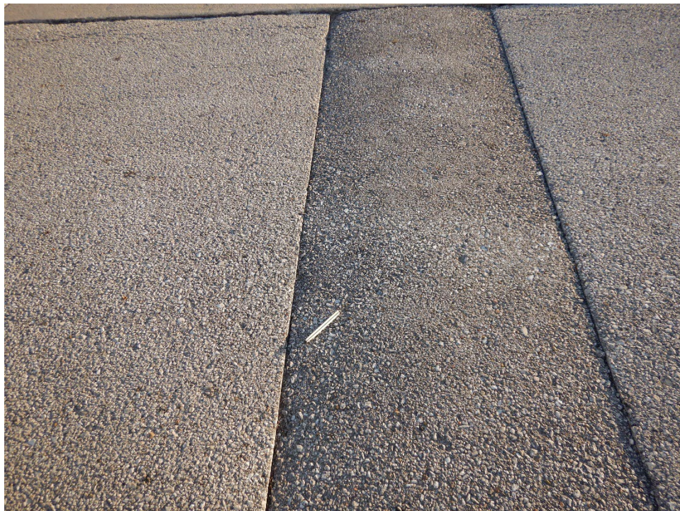
TH02IC-01. Patching (Sample Unit No. 02).
