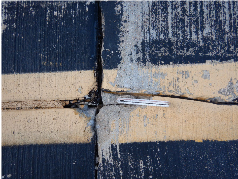
T01IC-06. Corner Spalling (Sample Unit No. 01).
