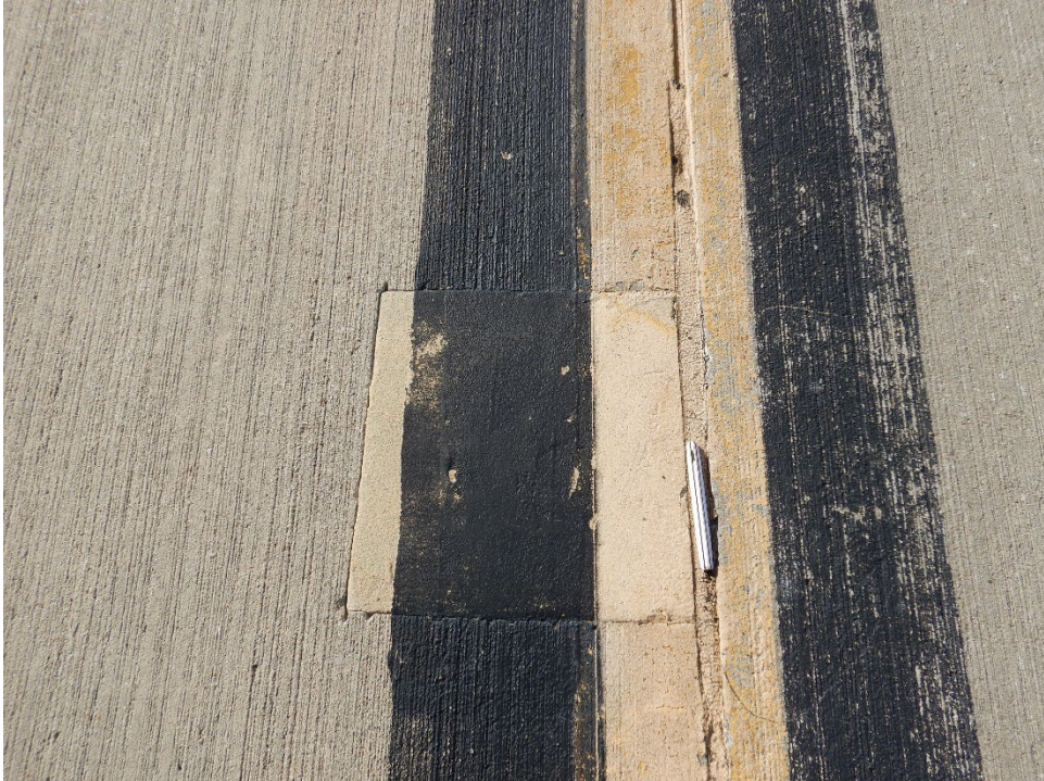
T02IC-02. Small Patching (Sample Unit No. 25).
