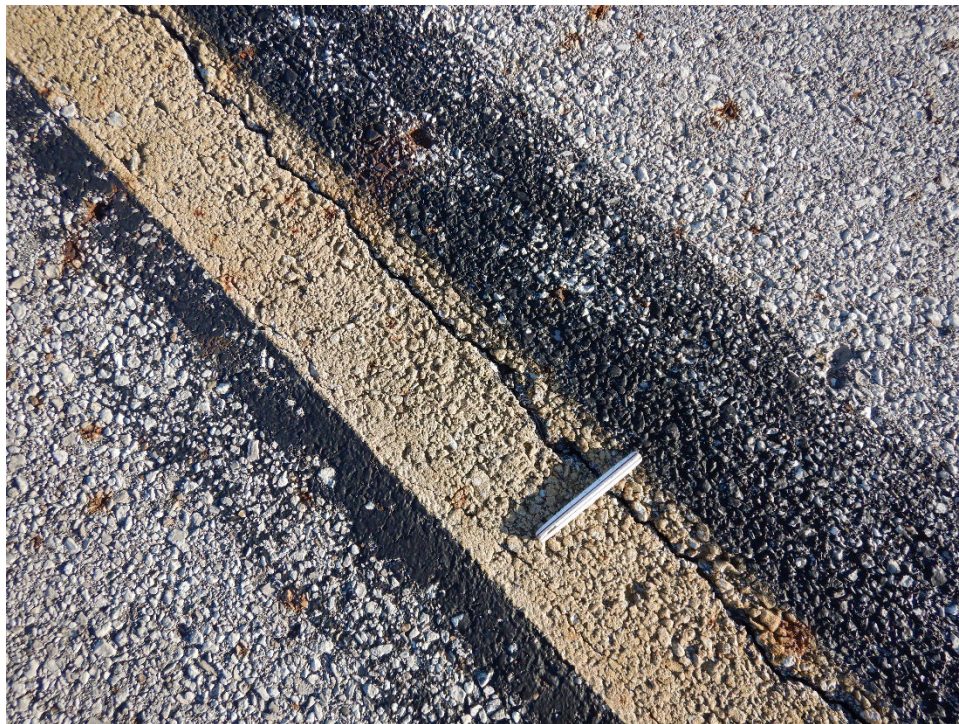
TH01IC-02. L&T Cracking (Sample Unit No. 01).
