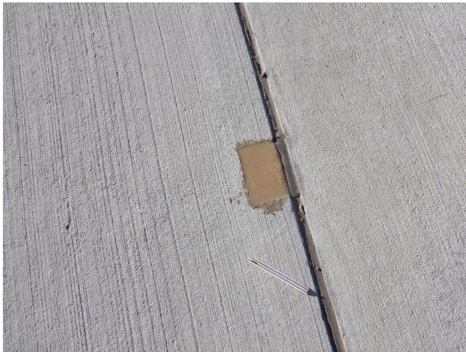
A01IC-01. Small Patching (Sample Unit No. 06).
