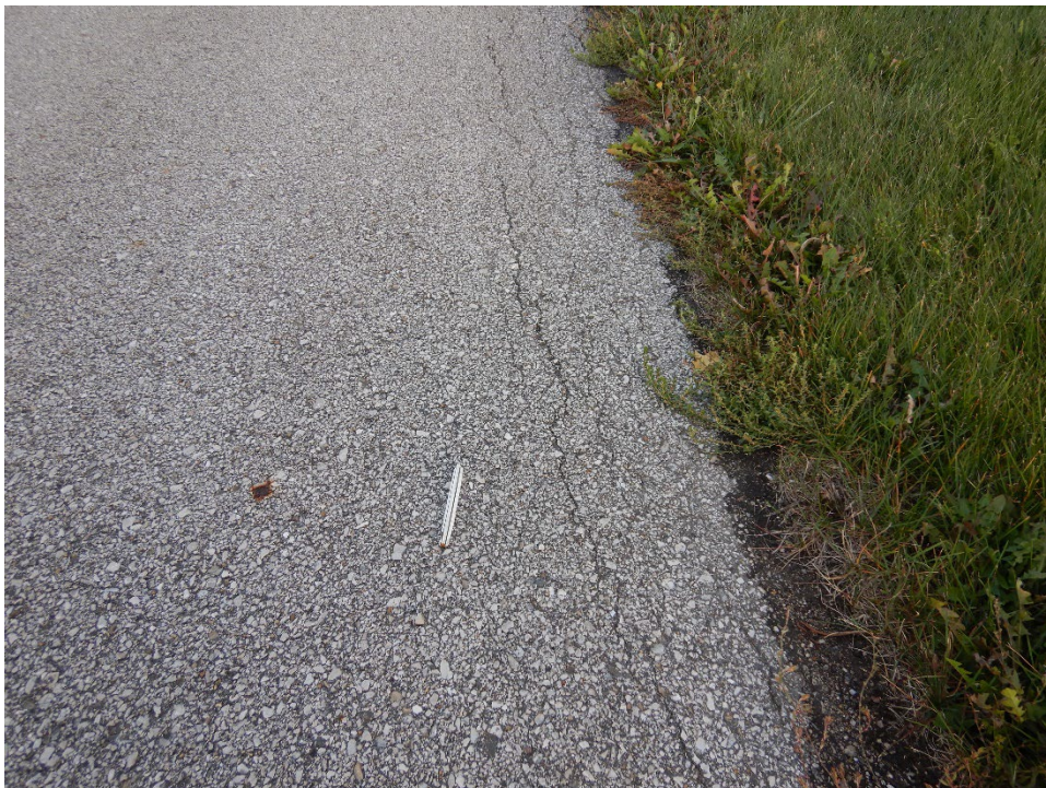
TH02IC-01. Alligator Cracking (Sample Unit No. 03) (1).
