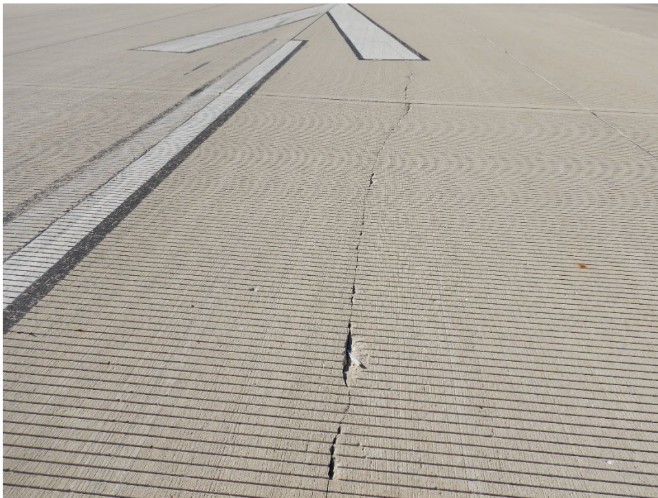
R07IC-01. LTD Cracking (Sample Unit No. 53).
