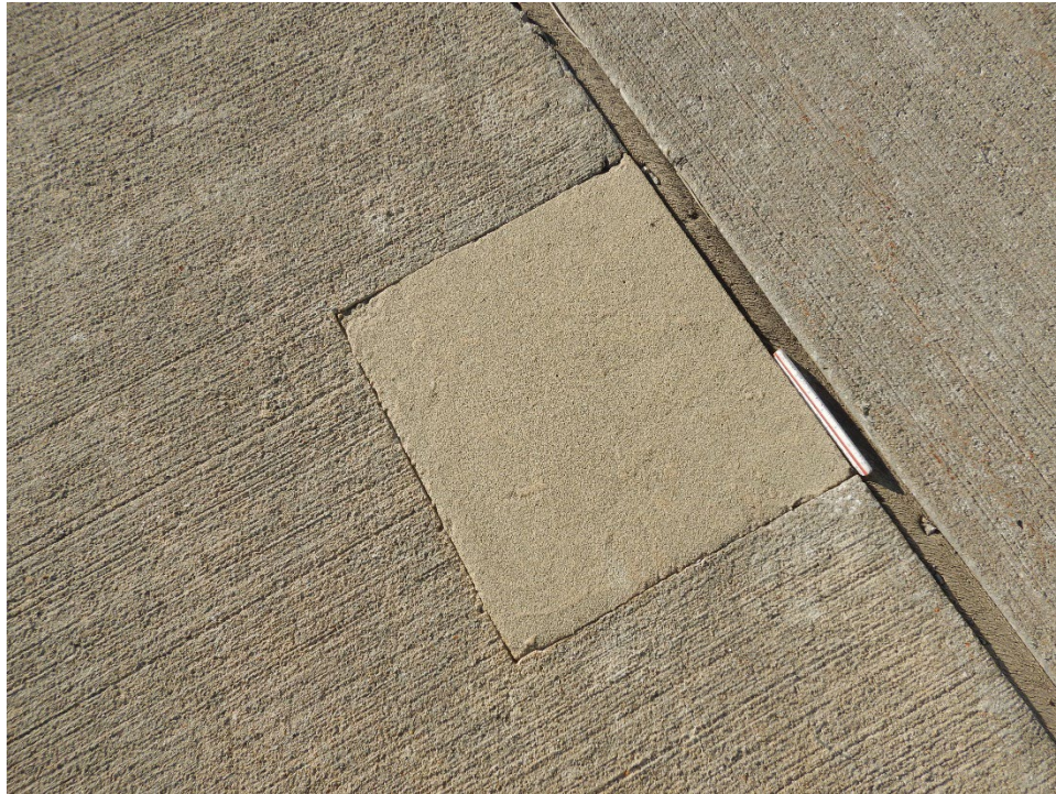
TH01IC-01. Small Patching (Sample Unit No. 04).
