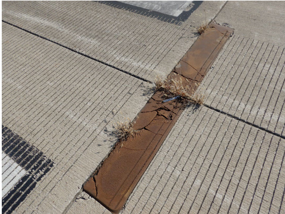
R07IC-01. Small Patching (Additional Sample Unit No. 36).
