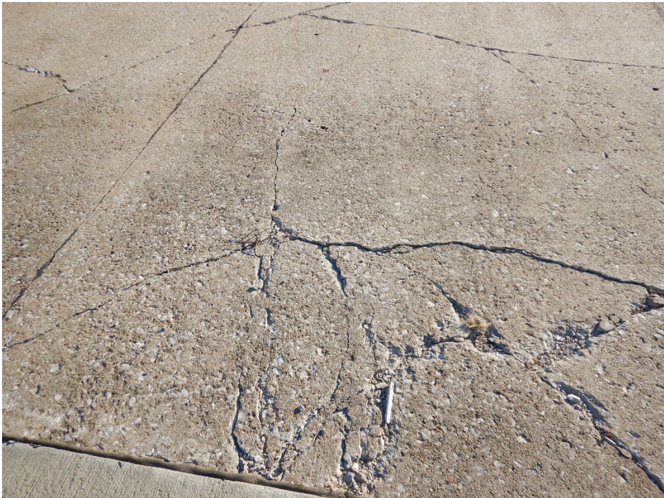
TH01IC-03. Shattered Slab (Sample Unit No. 02).
