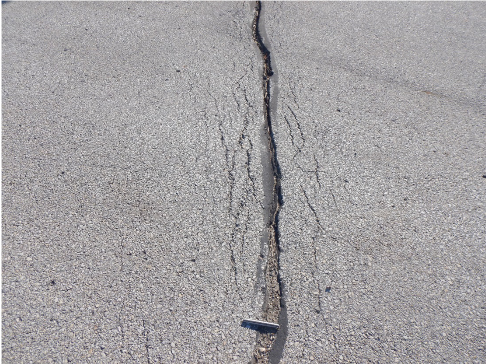
TH01IF-01. L&T Cracking (Sample Unit No. 01).
