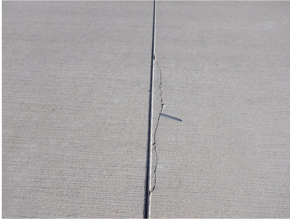
R13IF-01. Joint Spalling (Sample Unit No. 56).
