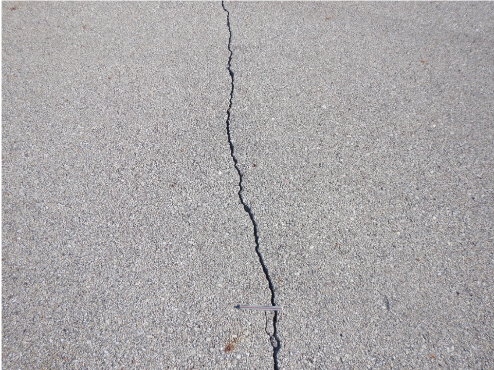
TH01IF-02. L&T Cracking (Sample Unit No. 01).
