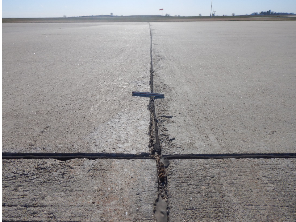
A01IF-02. Faulting (Sample Unit No. 08).
