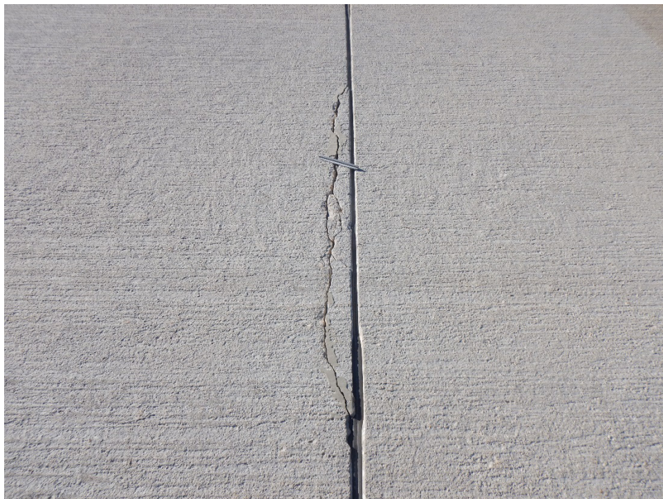
R13IF-02. Joint Spalling (Sample Unit No. 04).
