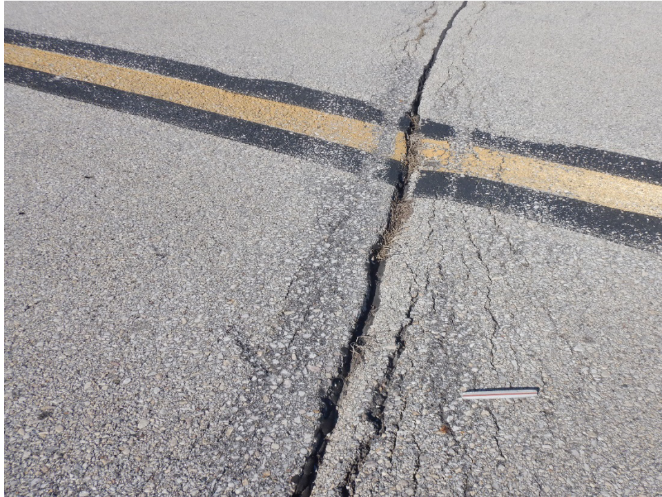
TAIF-01. L&T Cracking (Sample Unit No. 01).
