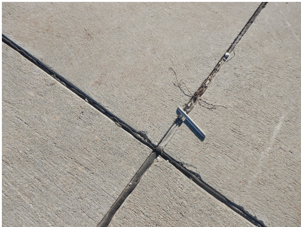
A01IF-02. Joint Seal Damage (Sample Unit No. 05).
