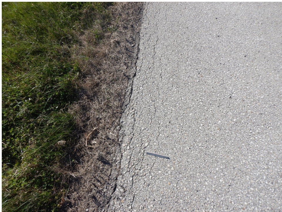
TAIF-01. Alligator Cracking (Sample Unit No. 03).
