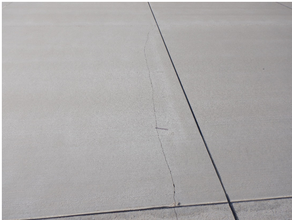
R13IF-01. LTD Cracking (Sample Unit No. 65).
