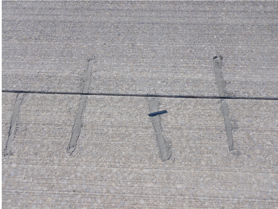
TBIF-01. Shrinkage Cracking (Sample Unit No. 70).
