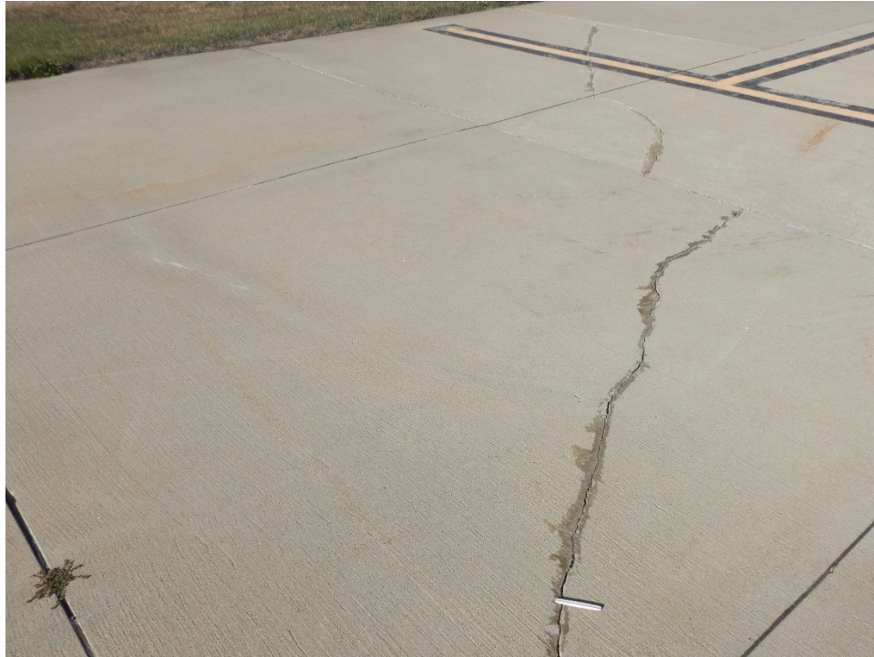
A01IF-02. LTD Cracking (Additional Sample Unit No. 06).
