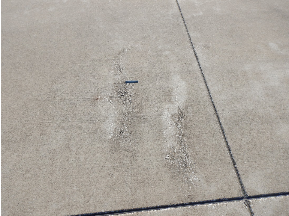
TCKE-01. Scaling (Sample Unit No. 02).
