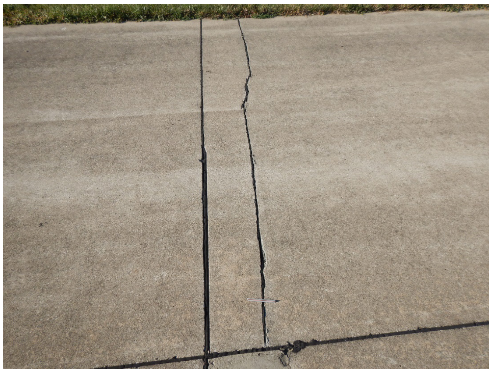
R14KE-02. LTD Cracking (Sample Unit No. 05).
