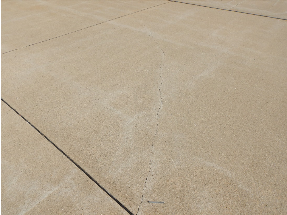
A01KE-04. LTD Cracking (Sample Unit No. 01).
