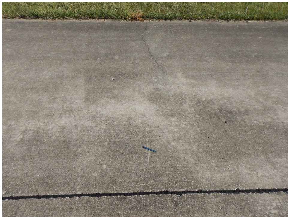
TCKE-02. LTD Cracking (Sample Unit No. 06).
