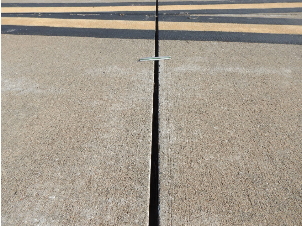
TDKE-01. Joint Seal Damage (Sample Unit No. 05).
