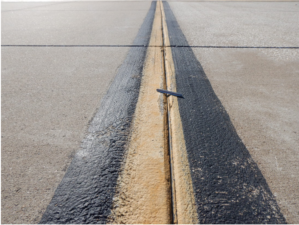
TBKE-04. Joint Seal Damage (Sample Unit No. 01).
