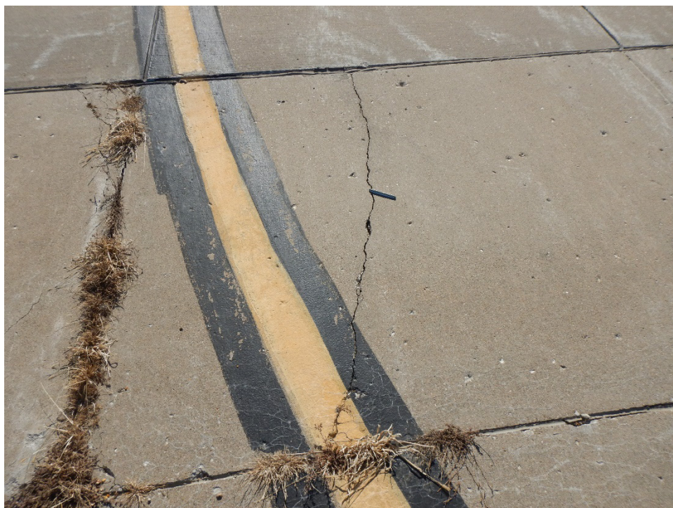
TAKE-05. LTD Cracking (Sample Unit No. 03).
