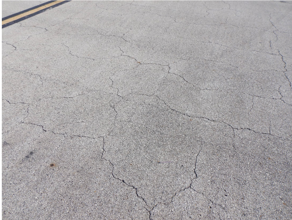
A01KE-02. Block Cracking (Sample Unit No. 02).
