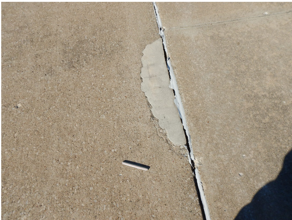
TBKE-01. Small Patching (Sample Unit No. 02).
