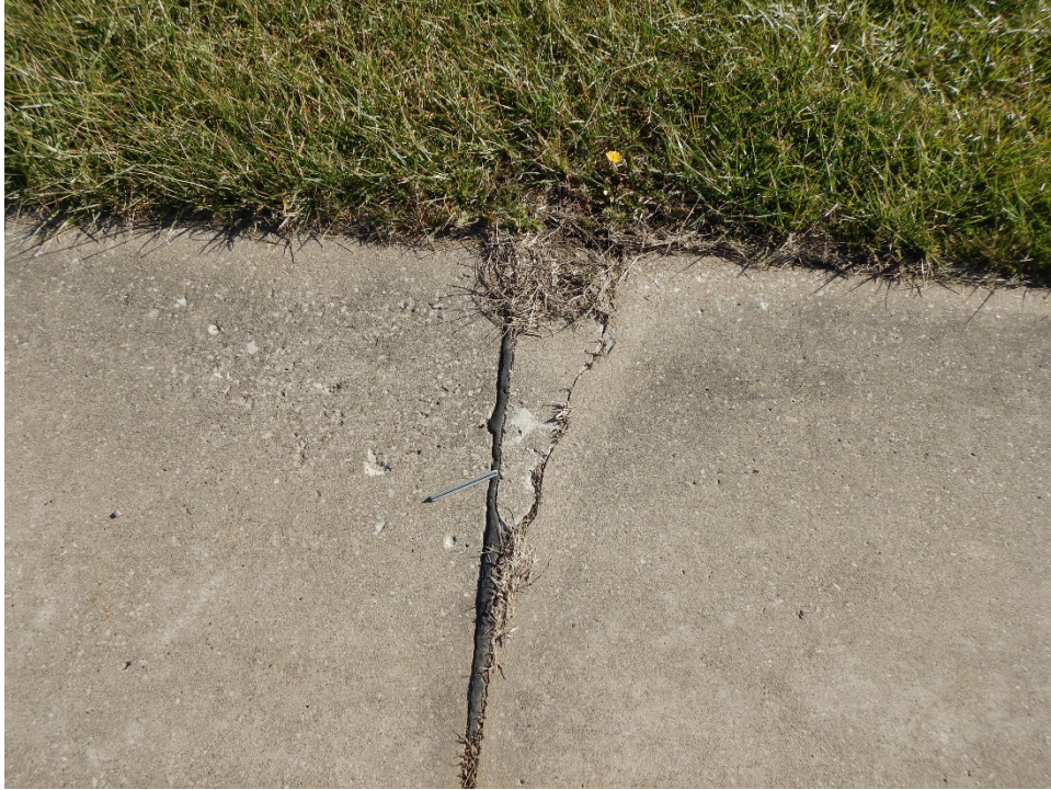
TBKE-02. Joint Spalling (Sample Unit No. 04).
