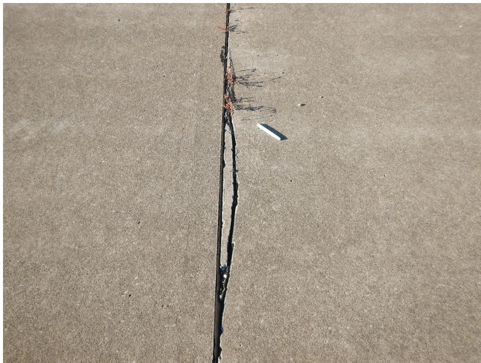
R14KE-01. Joint Spalling (Sample Unit No. 25).
