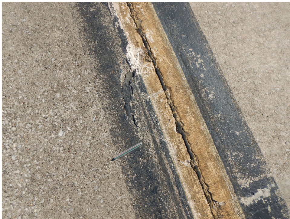
TBKE-01. Joint Spalling (Sample Unit No. 05).
