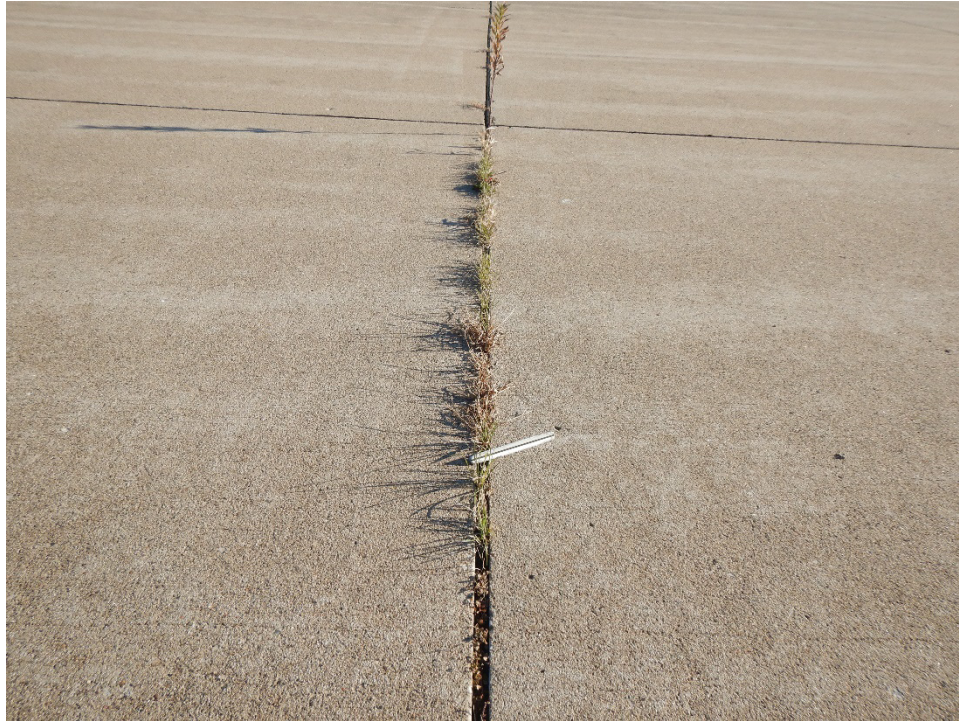
R14KE-01. Joint Seal Damage (Sample Unit No. 18).
