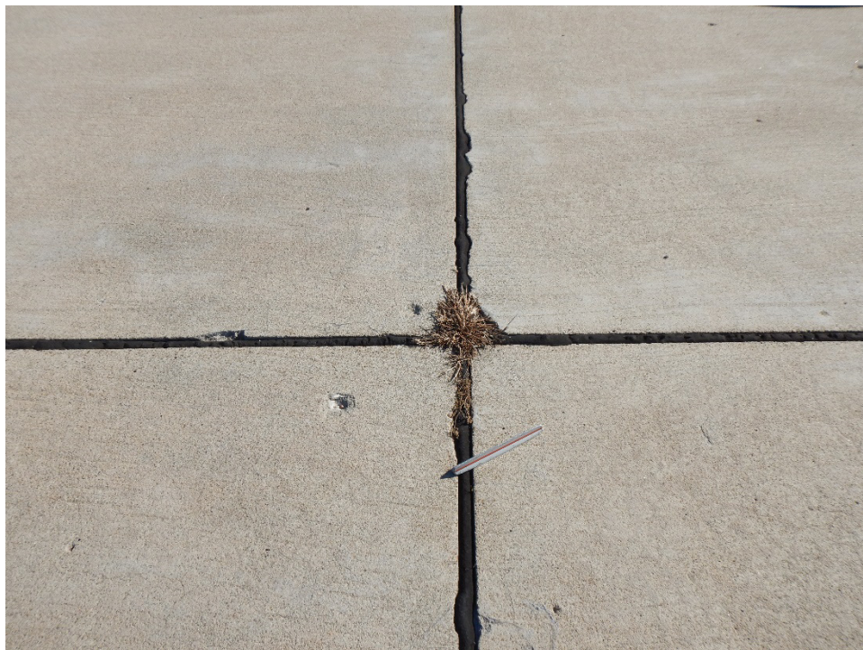
TBKE-03. Joint Seal Damage (Sample Unit No. 01).
