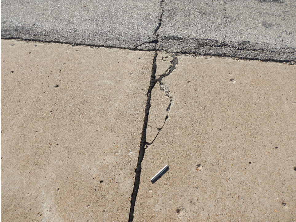
A01KE-03. Joint Spalling (Sample Unit No. 01).
