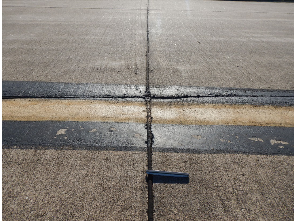
TCKE-03. Joint Seal Damage (Sample Unit No. 03).
