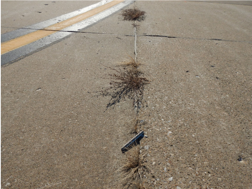
TAKE-02. Joint Seal Damage (Sample Unit No. 01).
