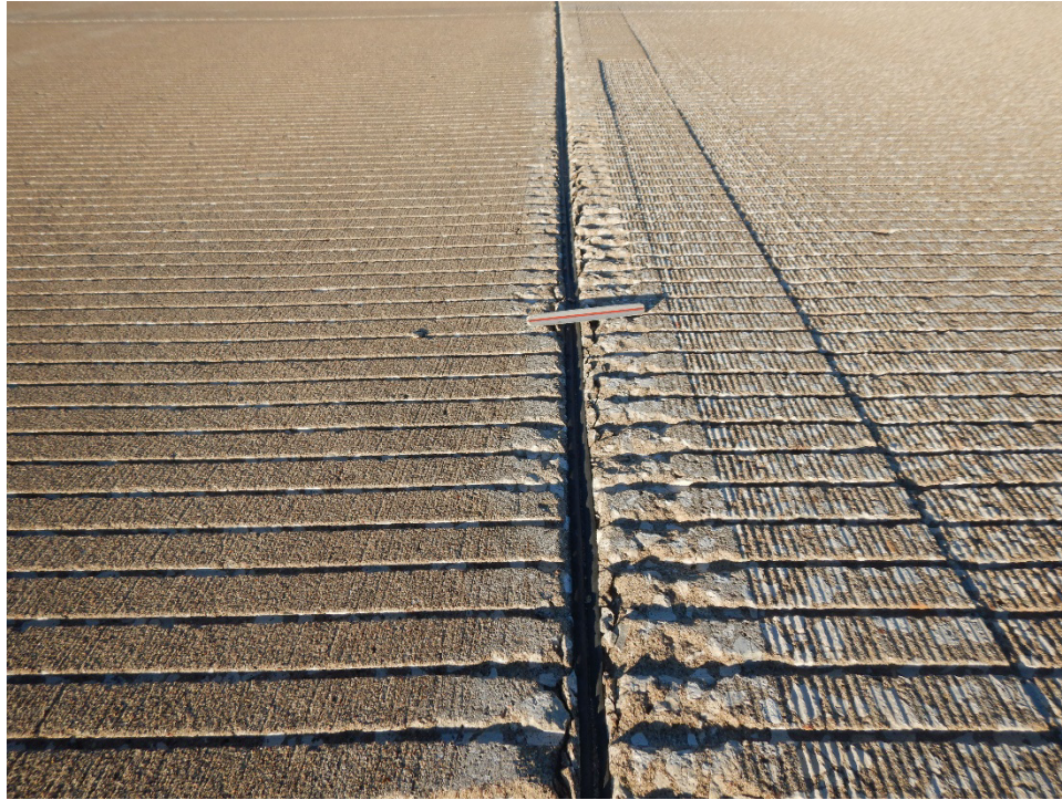
R08KE-01. Joint Seal Damage (Sample Unit No. 036).
