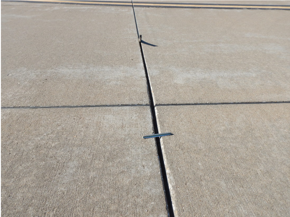
TAKE-06. Joint Seal Damage (Sample Unit No. 03).
