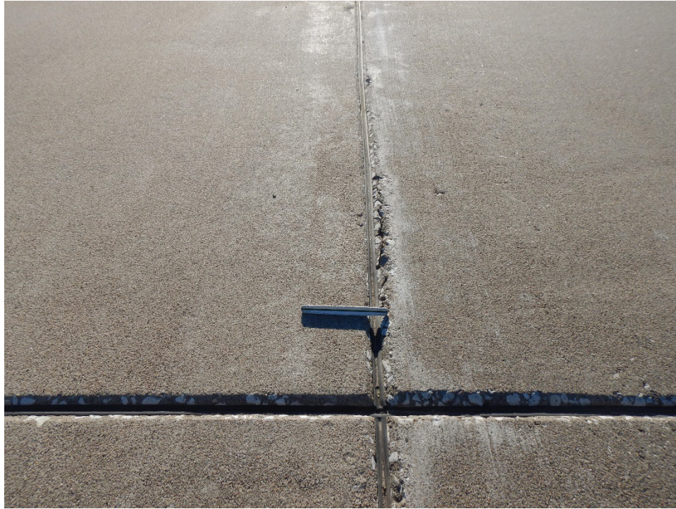
R14KE-04. Joint Seal Damage (Sample Unit No. 04).
