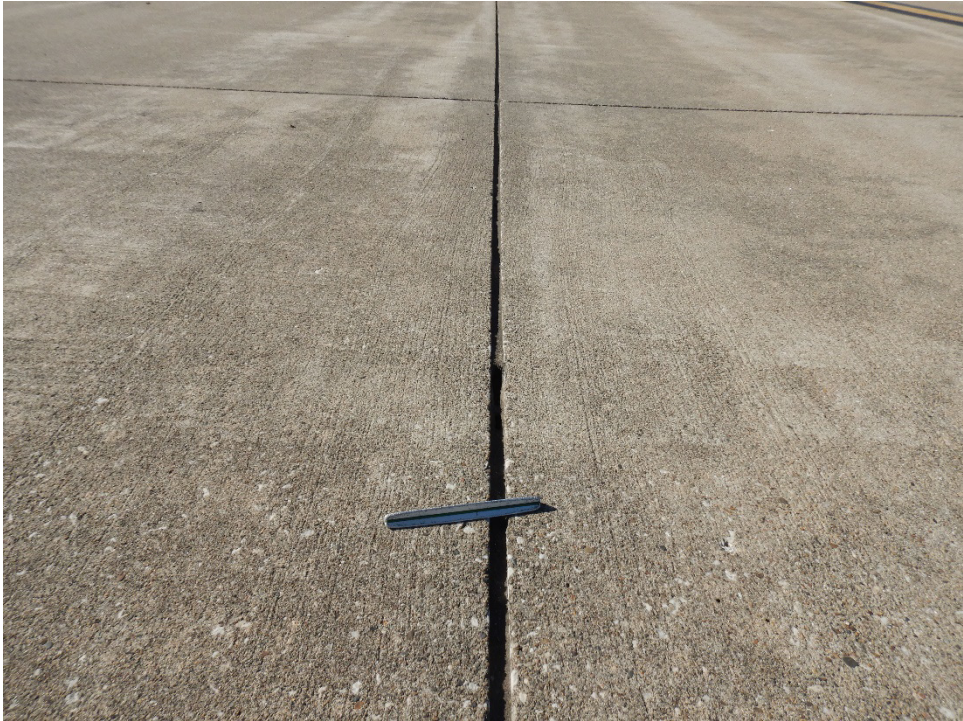
TAKE-04. Joint Seal Damage (Sample Unit No. 82).
