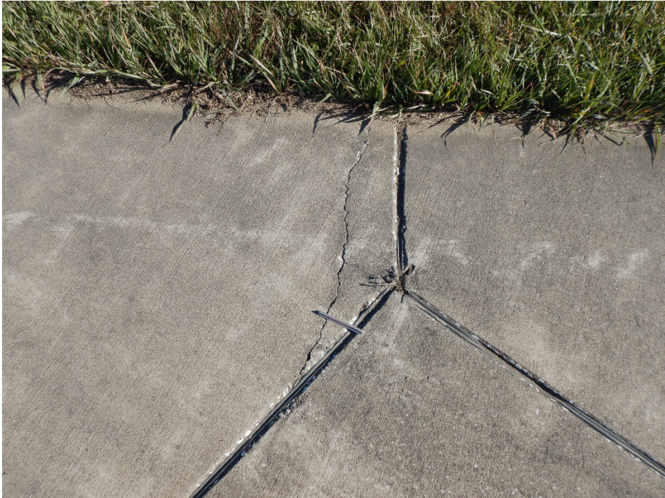
TBKE-04. Joint Spalling (Sample Unit No. 08).
