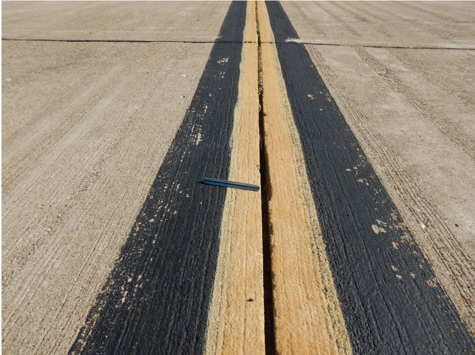
TAKE-03. Joint Seal Damage (Sample Unit No. 07).
