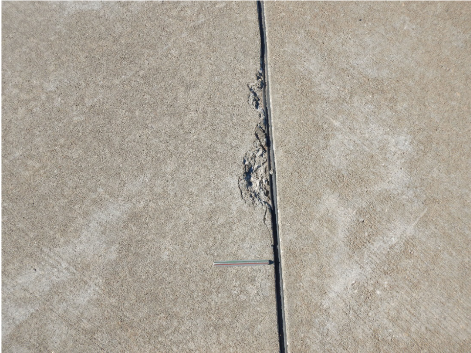
TDKE-01. Joint Spalling (Sample Unit No. 08).
