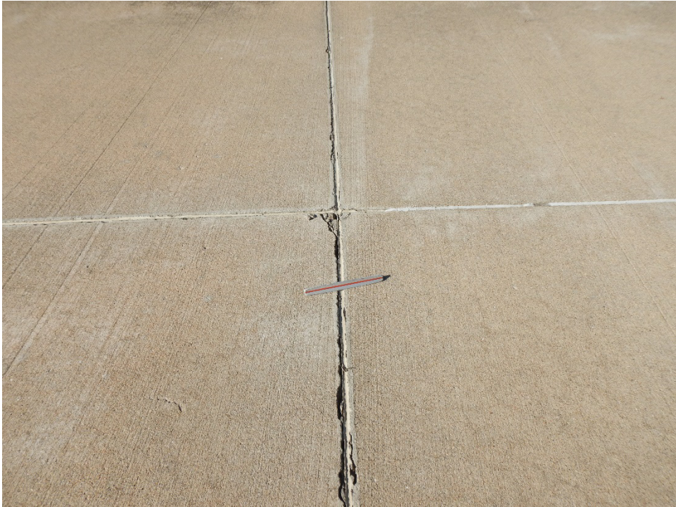
TH01KE-01. Joint Seal Damage (Sample Unit No. 18).
