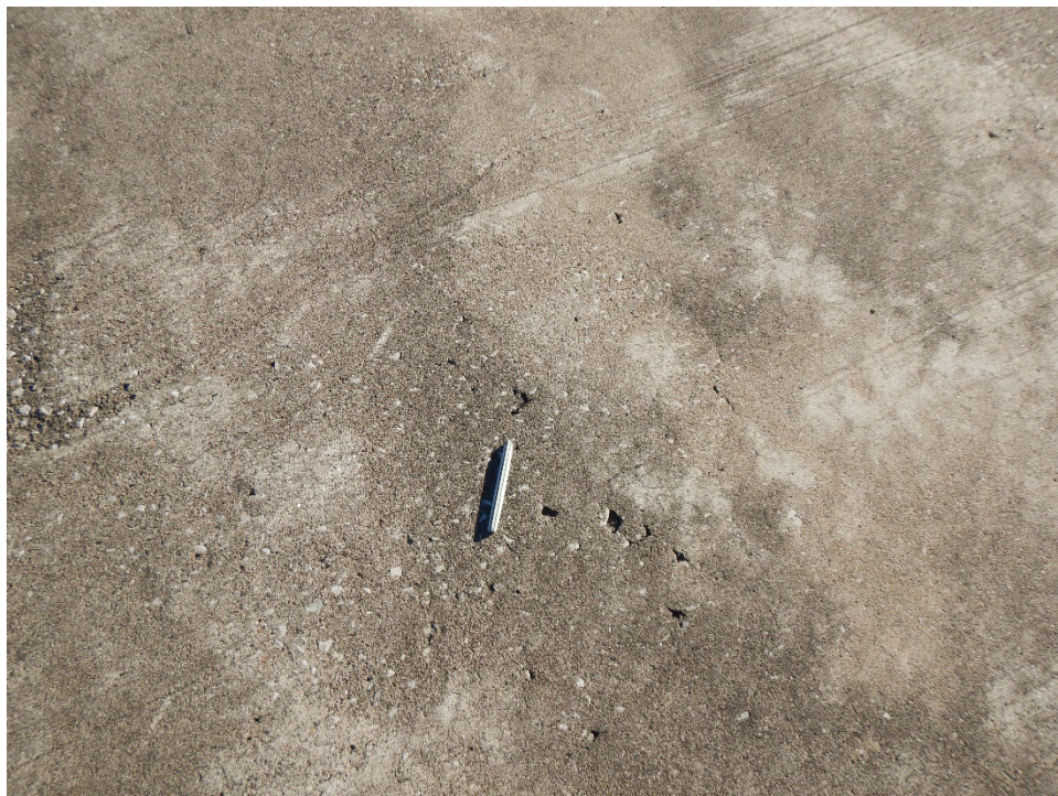
TCKE-03. Scaling (Sample Unit No. 02).
