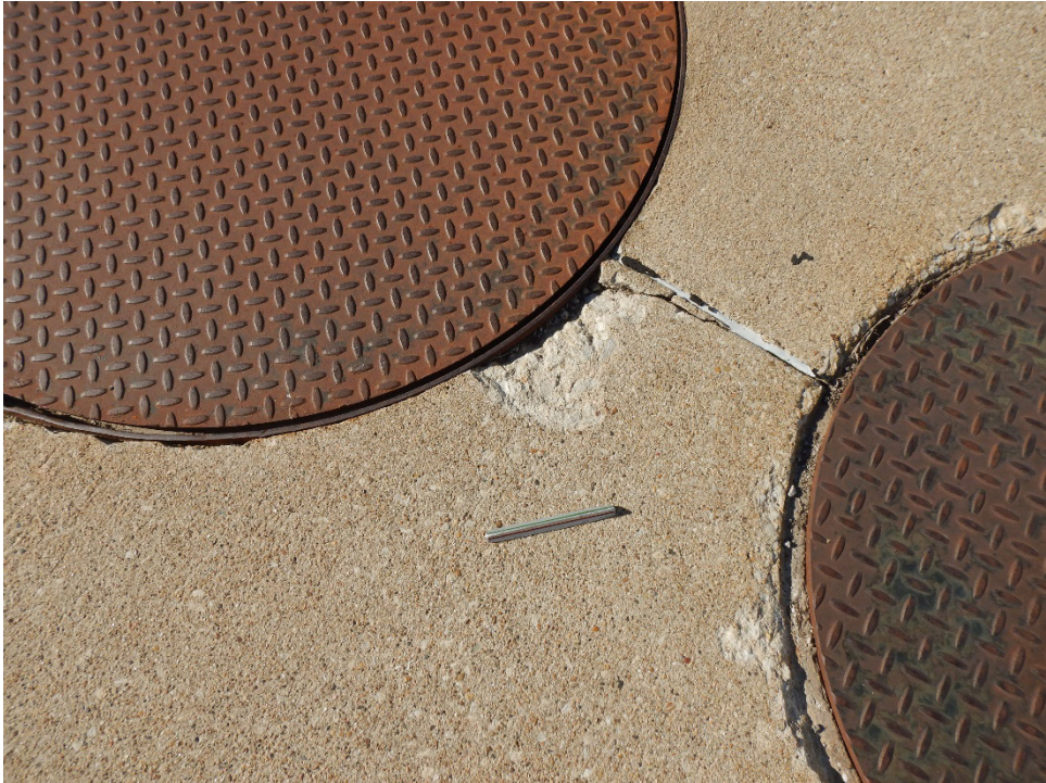
A01KE-04. Joint Spalling (Sample Unit No. 01).
