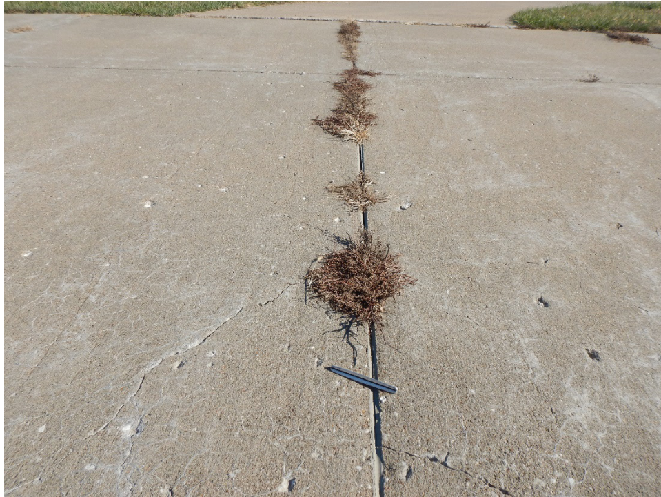
TAKE-05. Joint Seal Damage (Sample Unit No. 02).
