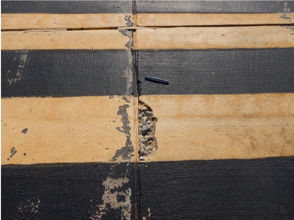
TAKE-06. Joint Spalling (Sample Unit No. 01).
