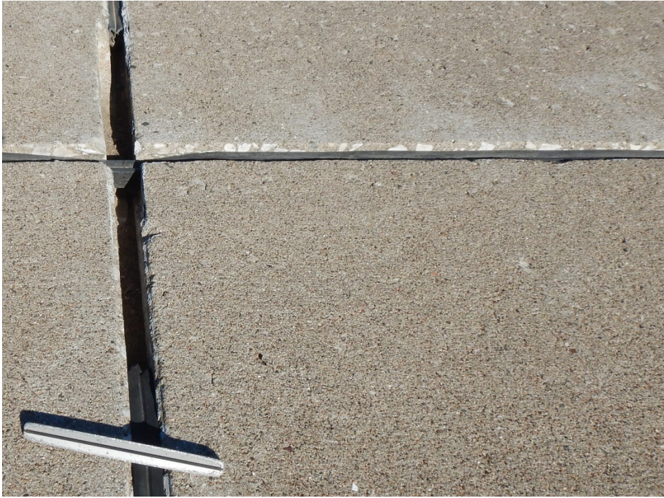
TAKE-01. Joint Seal Damage (Sample Unit No. 03).
