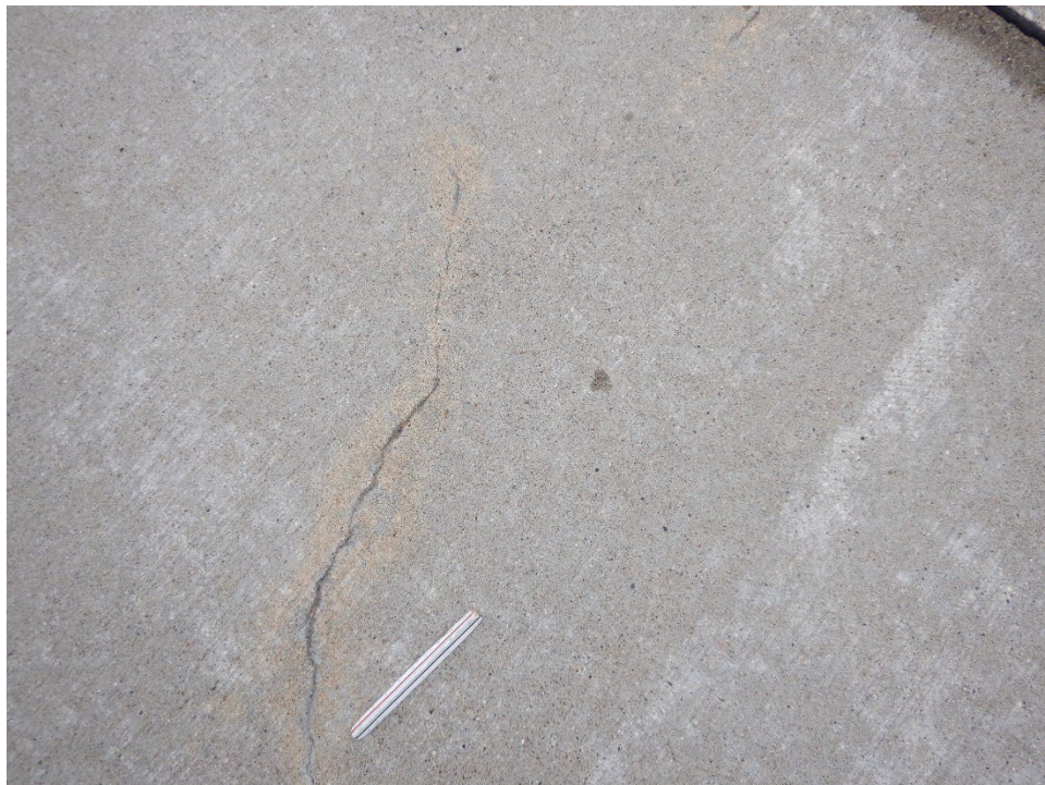
T01KN-01. Shrinkage Cracking (Sample Unit No. 03).
