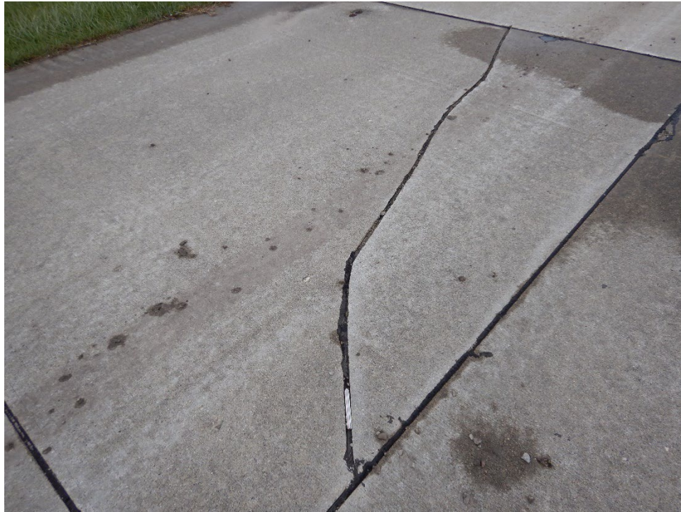
A02KN-01. LTD Cracking (Sample Unit No. 10).
