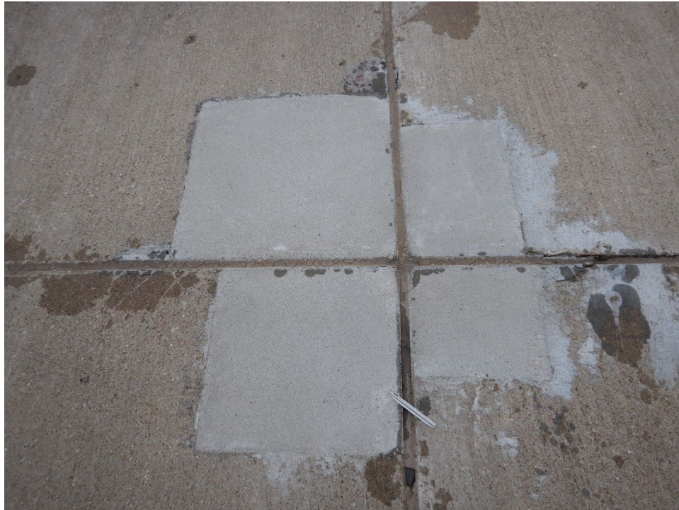
R15KN-02. Small Patching (Sample Unit No. 14).
