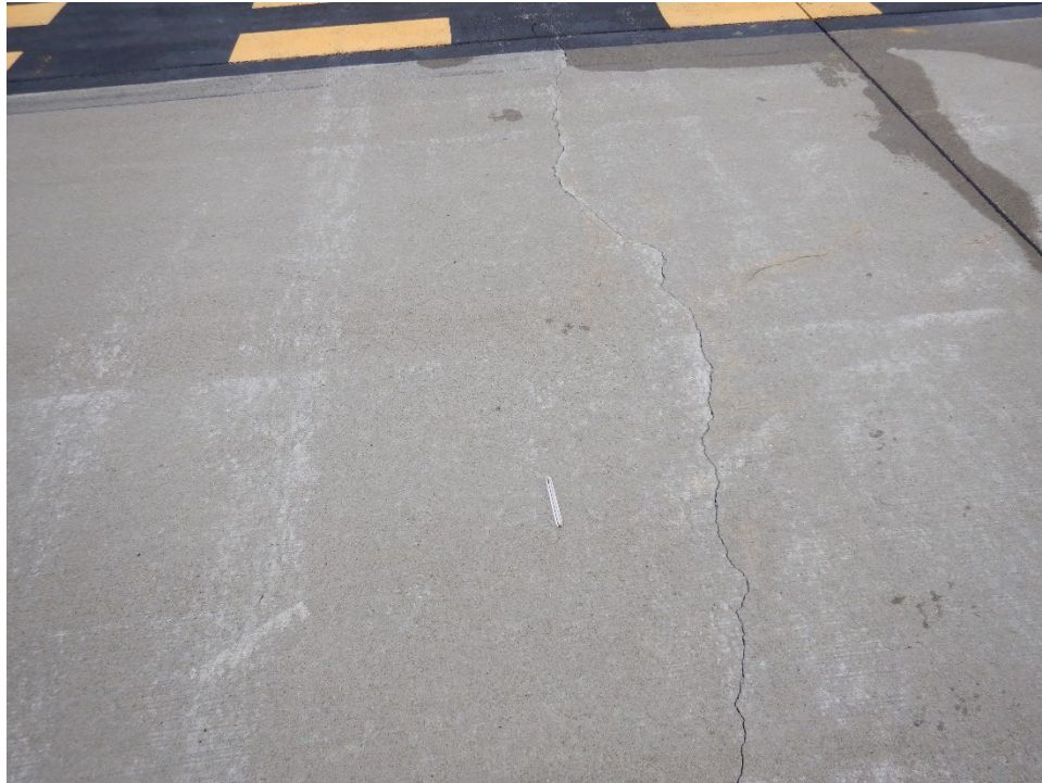
T01KN-01. LTD Cracking (Sample Unit No. 03).
