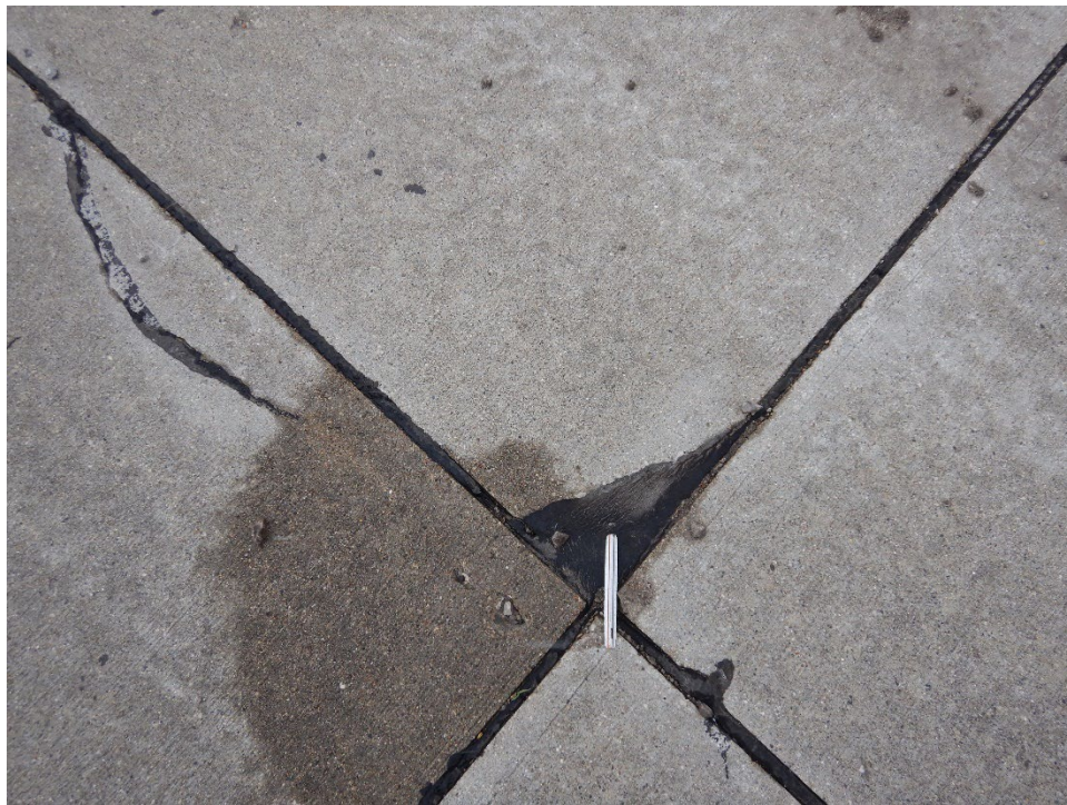
A02KN-01. Corner Spalling (Sample Unit No. 10).
