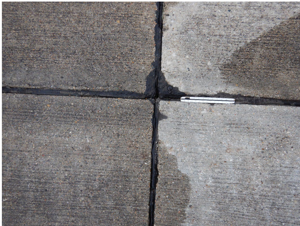
T03KN-01. Joint Seal Damage (Sample Unit No. 02).
