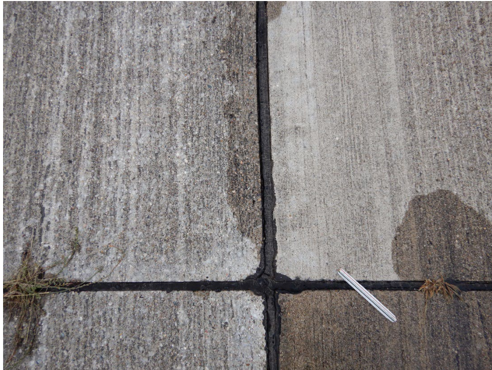
T03KN-02. Joint Seal Damage (Sample Unit No. 20).
