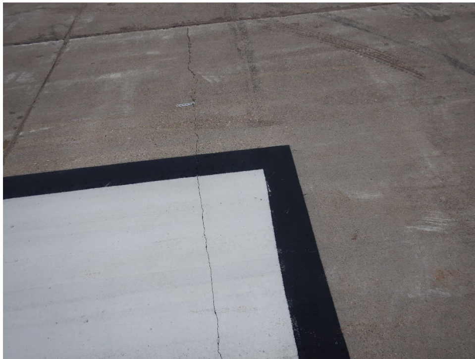
R15KN-02. LTD Cracking (Sample Unit No. 19).
