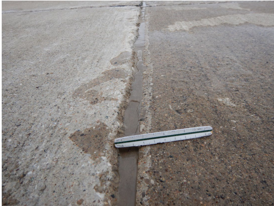
T02KN-01. Faulting (Sample Unit No. 02).
