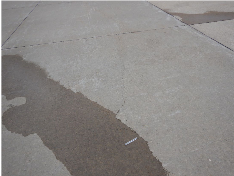
A02KN-02. LTD Cracking (Sample Unit No. 03).
