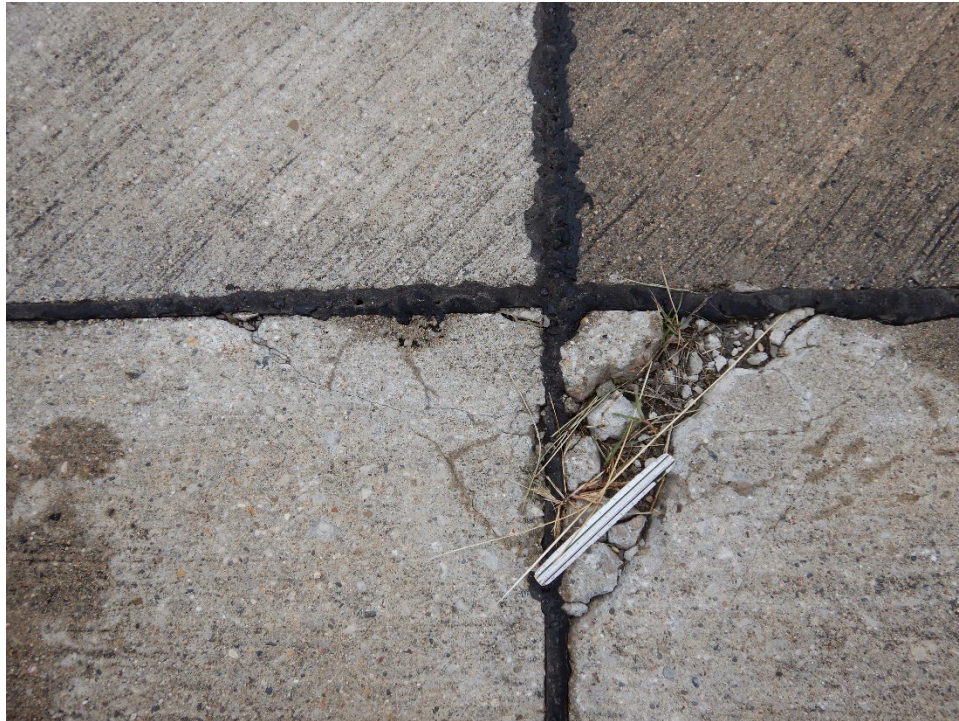
T03KN-03. Durability Cracking (Sample Unit No. 02).
