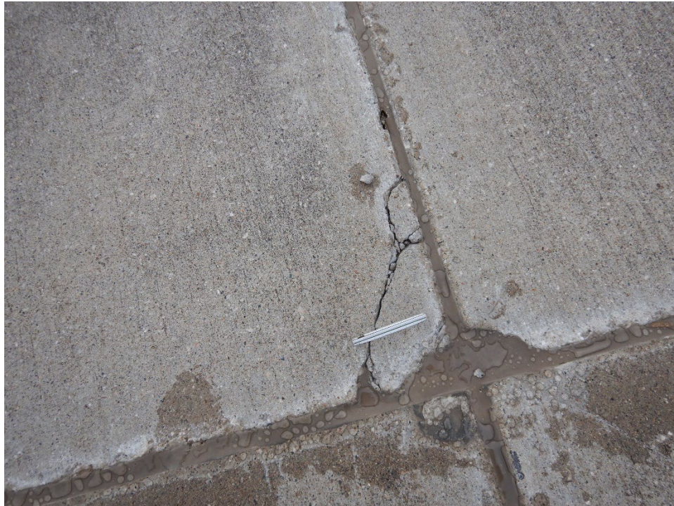
R15KN-02. Joint Spalling (Sample Unit No. 14).
