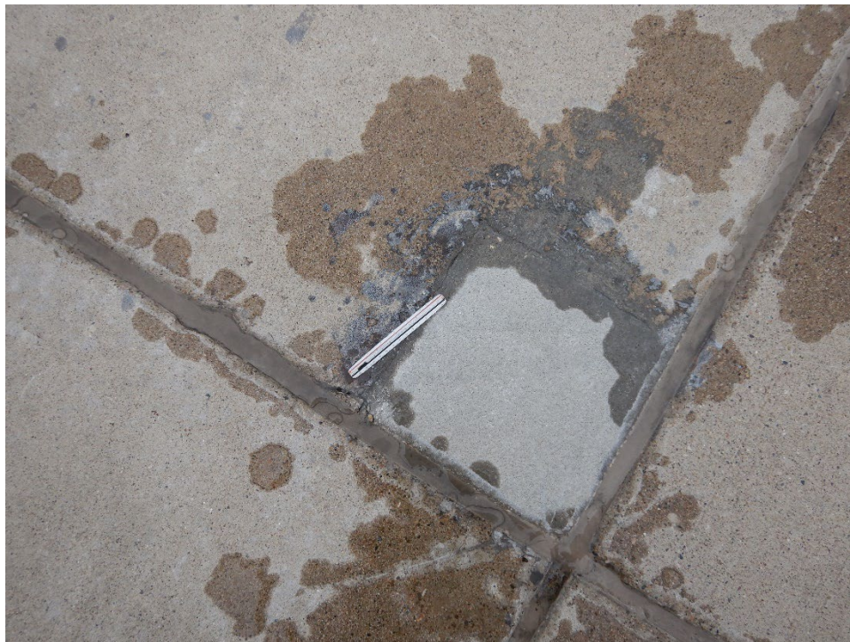
T02KN-01. Small Patching (Sample Unit No. 05).
