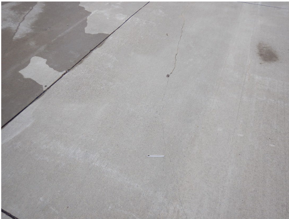
A01KN-01. LTD Cracking (Sample Unit No. 13).
