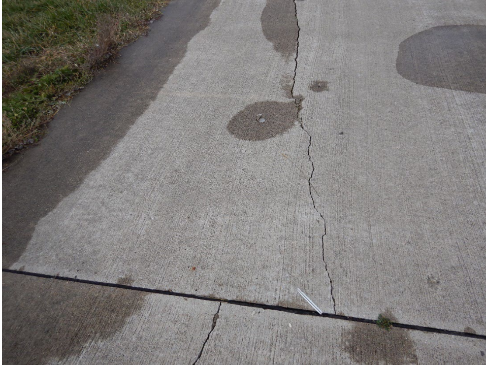
T03KN-01. LTD Cracking (Sample Unit No. 08).
