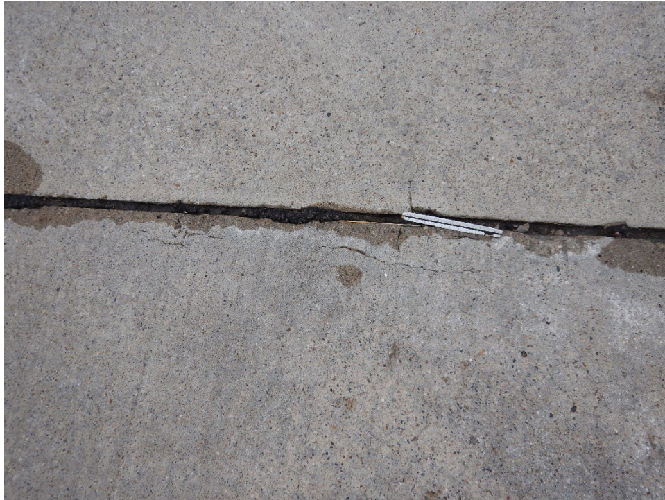
T03KN-04. Durability Cracking (Sample Unit No. 01).
