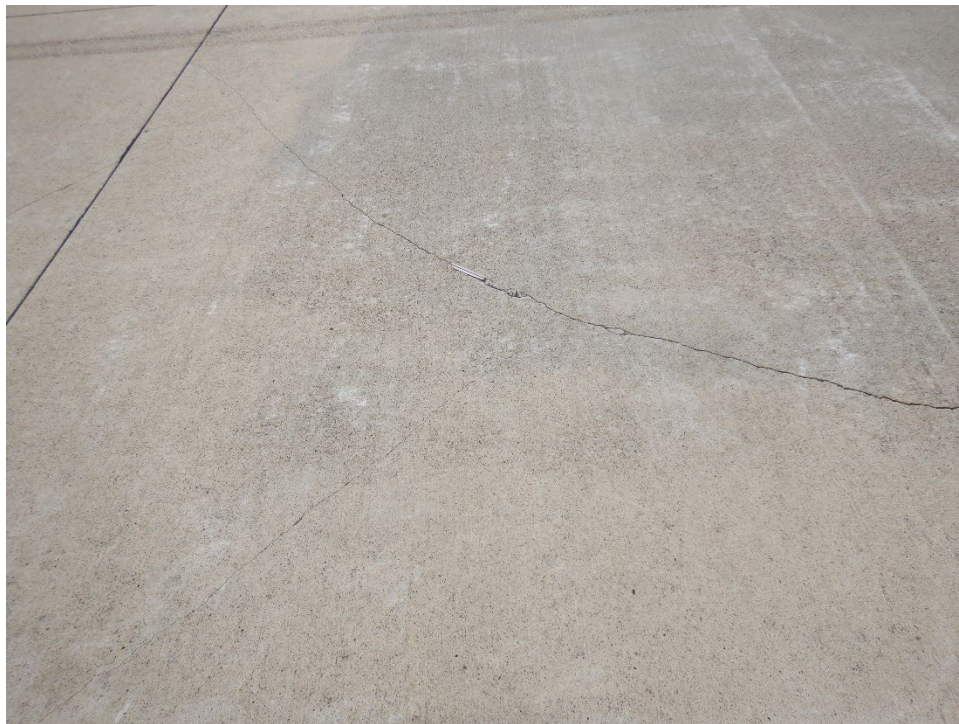
A02KN-02. Shattered Slab (Sample Unit No. 03).
