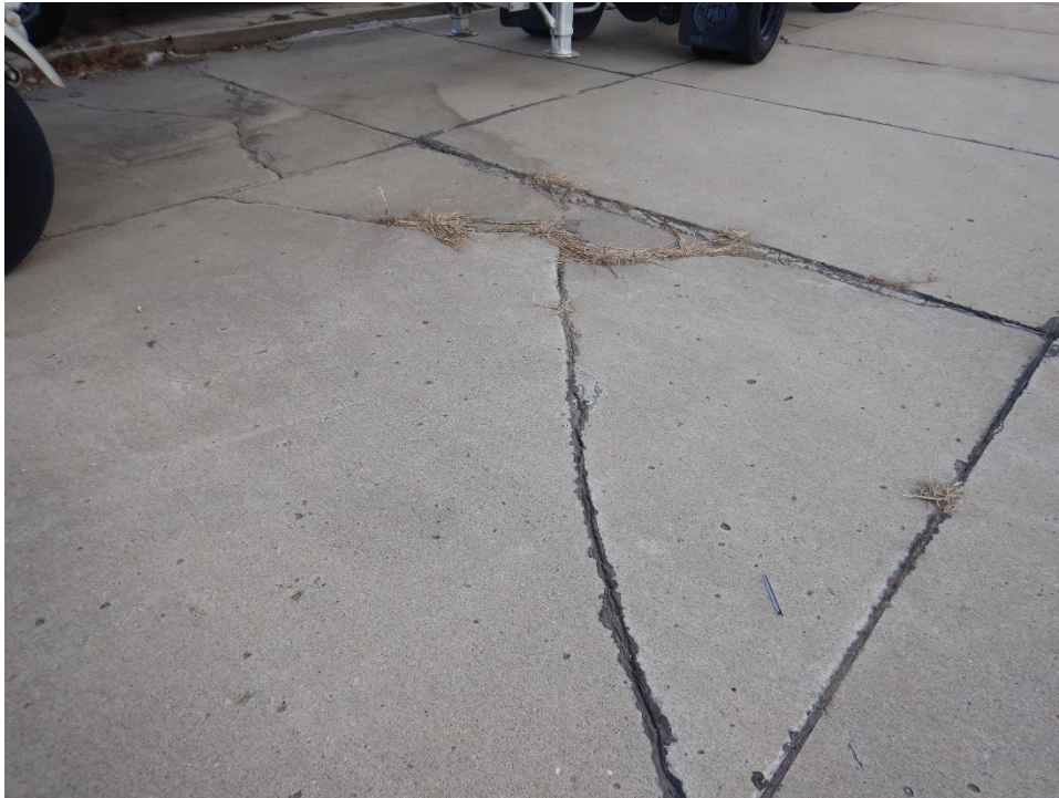
A01LE-02. Shattered Slab (Sample Unit No. 03).
