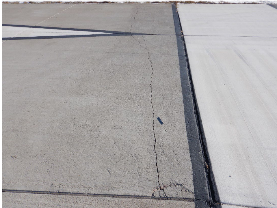
R18LE-07. LTD Cracking (Sample Unit No. 01).
