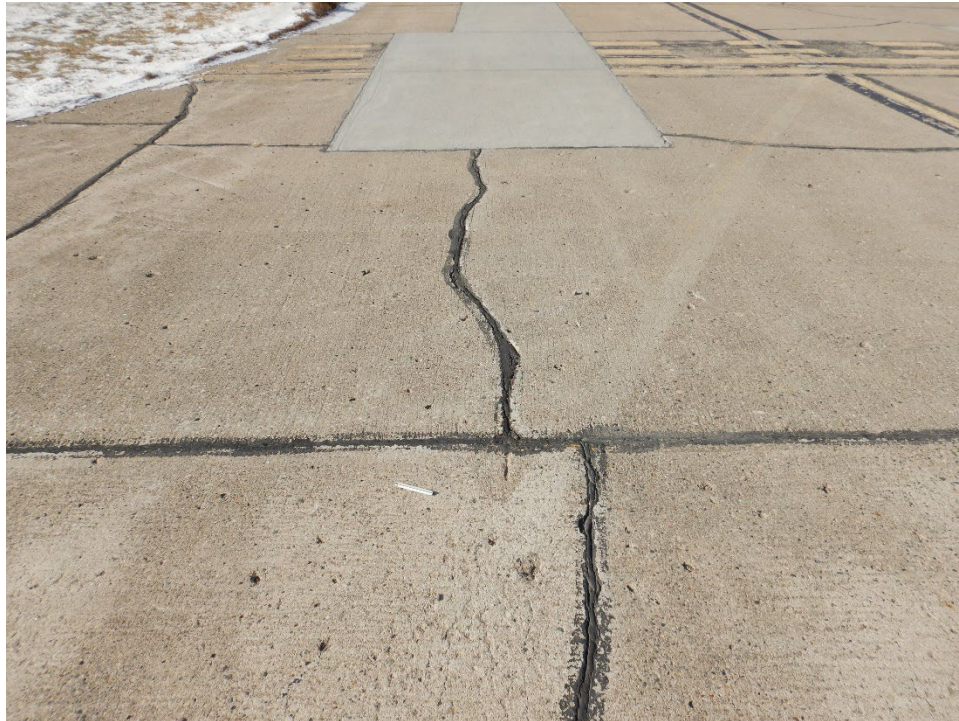
T01LE-01. LTD Cracking (Sample Unit No. 01).
