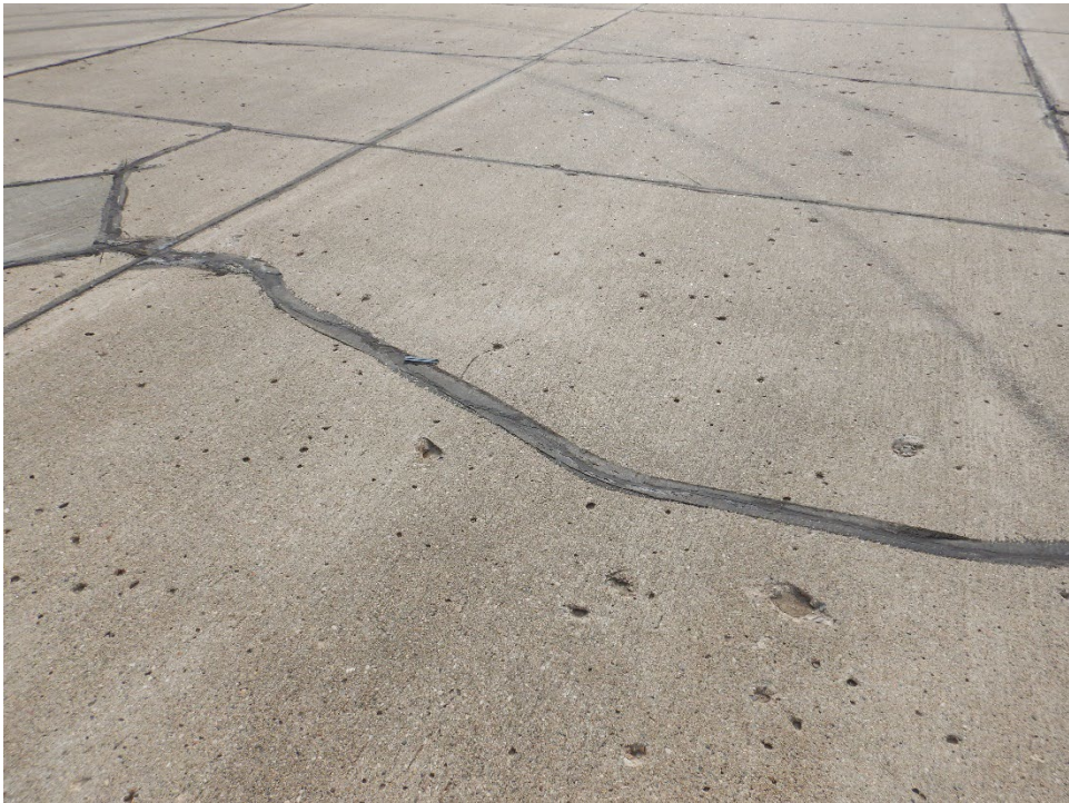
A01LE-01. LTD Cracking (Sample Unit No. 02).
