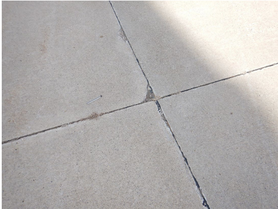
TH01LE-01. Corner Spalling (Sample Unit No. 01).
