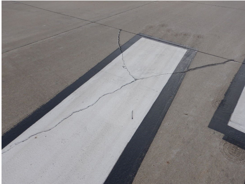
R18LE-05. LTD Cracking (Sample Unit No. 04).
