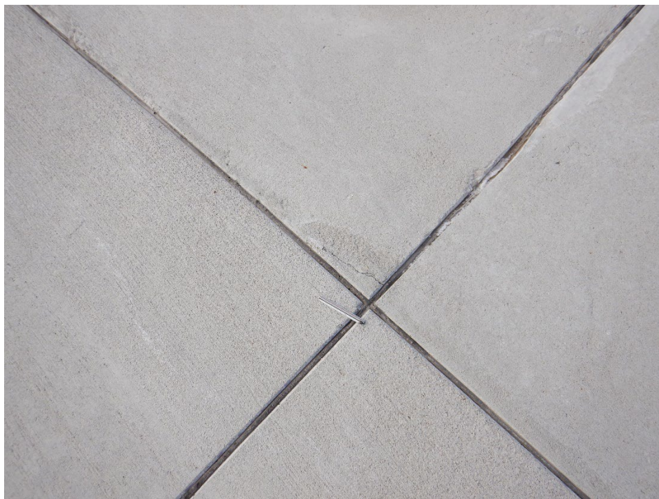
R18LE-07. Joint Spalling (Sample Unit No. 06).
