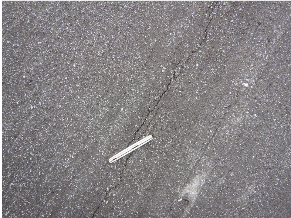
R18C2-01. L&T Cracking (Sample Unit No. 03).
