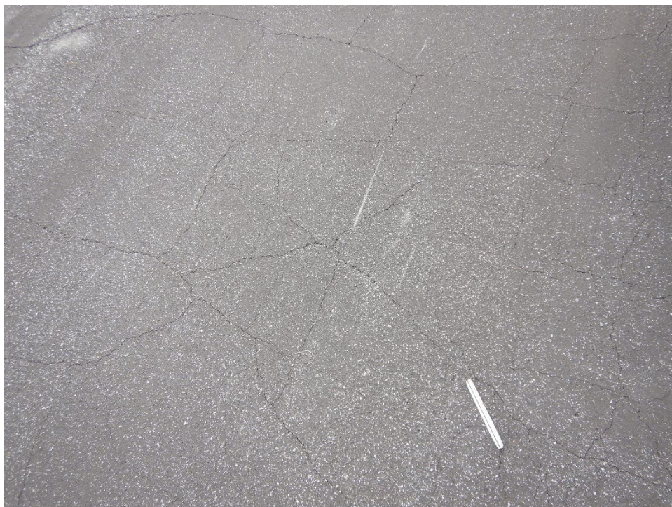
T01C2-01. Alligator Cracking (Sample Unit No. 01).
