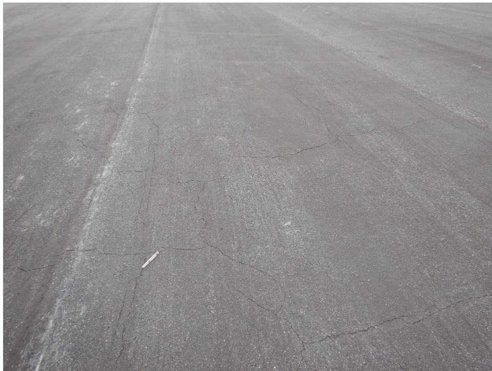
A01C2-01. Block Cracking (Sample Unit No. 02).
