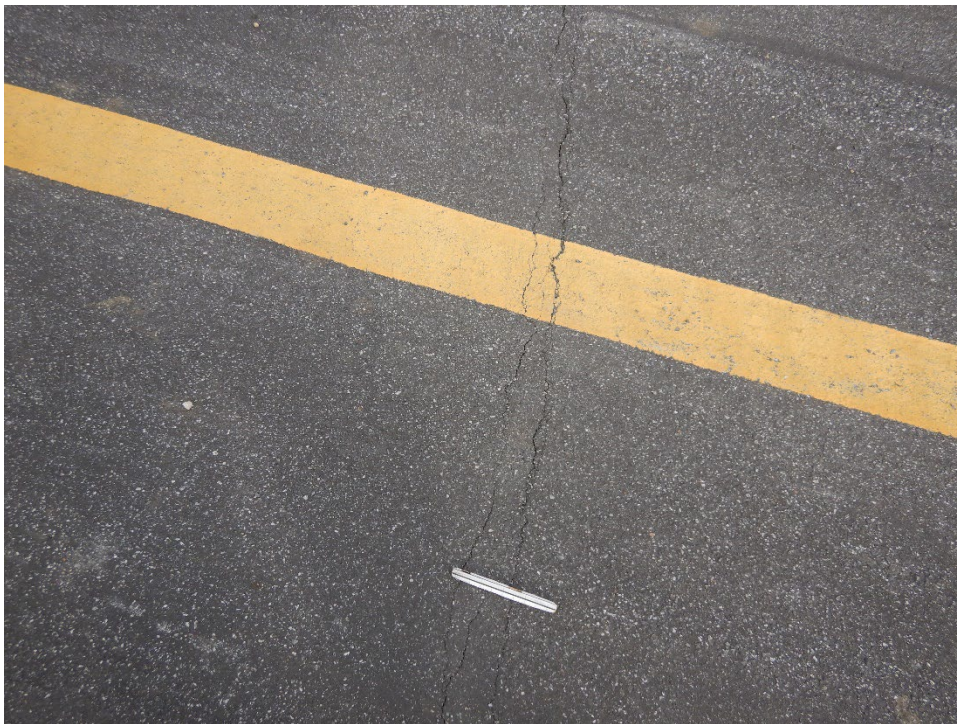
T01C2-02. L&T Cracking (Sample Unit No. 01).
