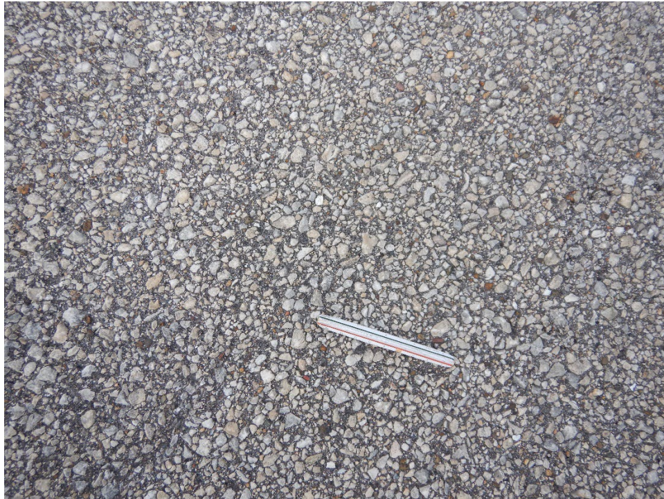
TH01C2-01. Weathering (Sample Unit No. 01).
