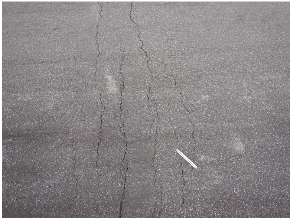
R18C2-02. L&T Cracking (Sample Unit No. 05).
