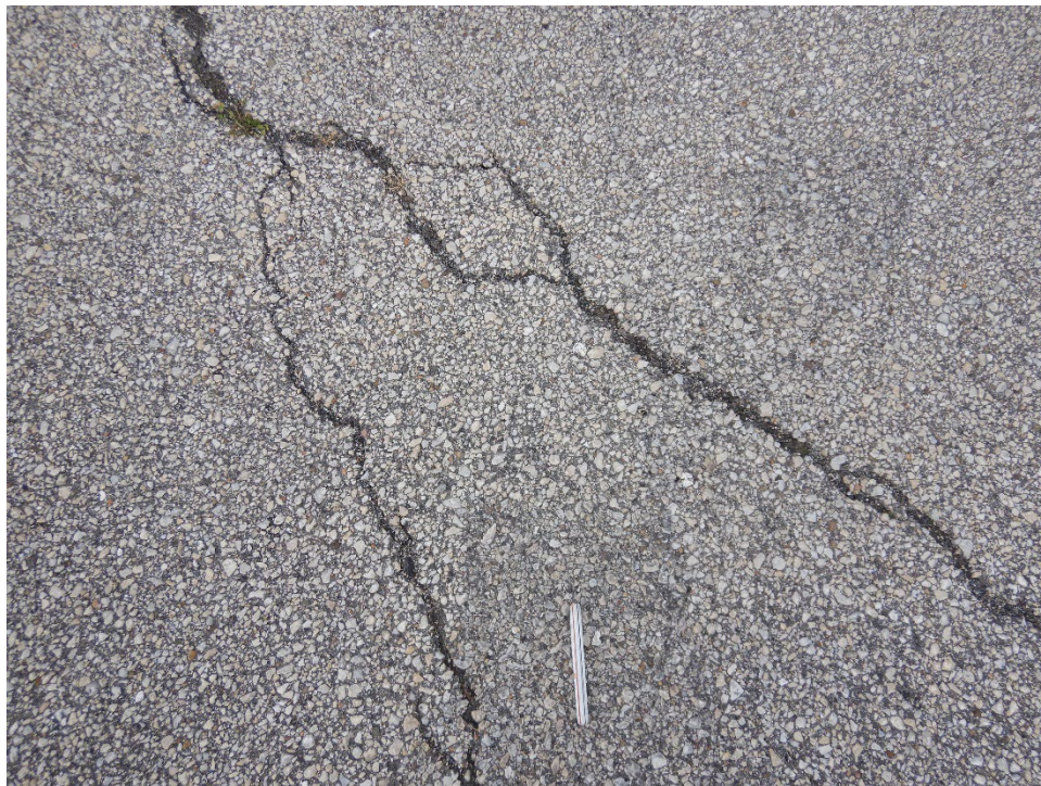
TH01C2-01. L&T Cracking (Sample Unit No. 01).
