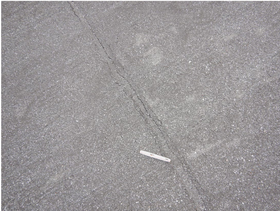
T01C2-01. L&T Cracking (Sample Unit No. 01).
