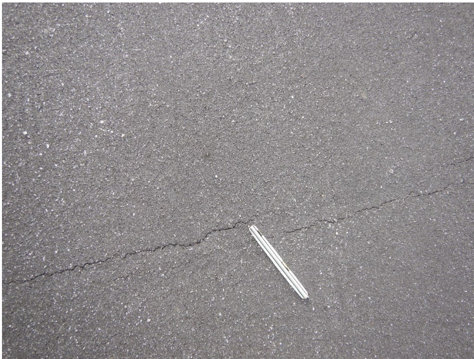
A02C2-01. L&T Cracking (Sample Unit No. 01).
