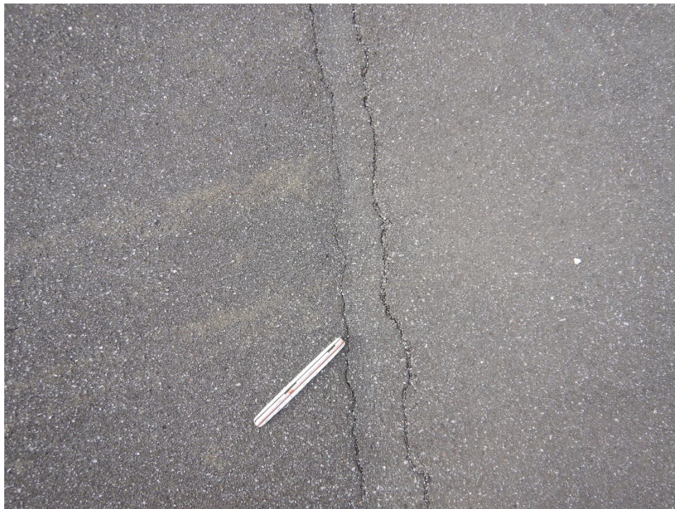
A02C2-02. L&T Cracking (Sample Unit No. 02).
