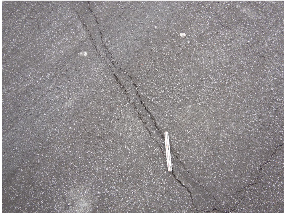
R18C2-02. L&T Cracking (Sample Unit No. 02).
