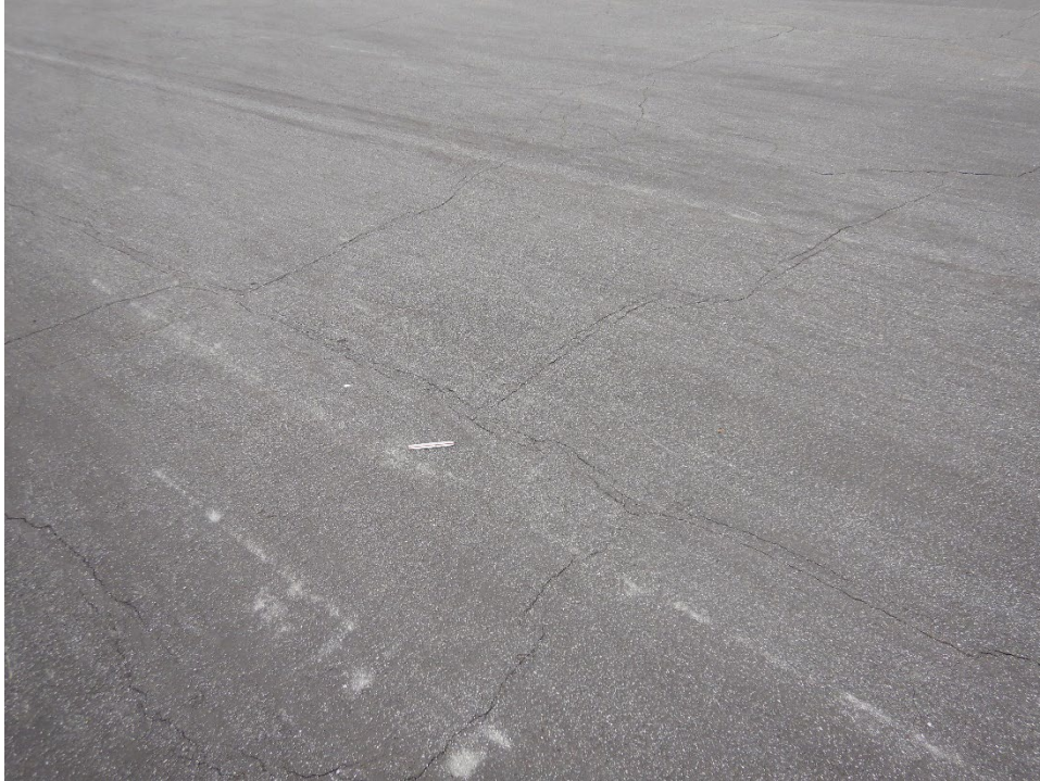
T01C2-01. Block Cracking (Sample Unit No. 02).
