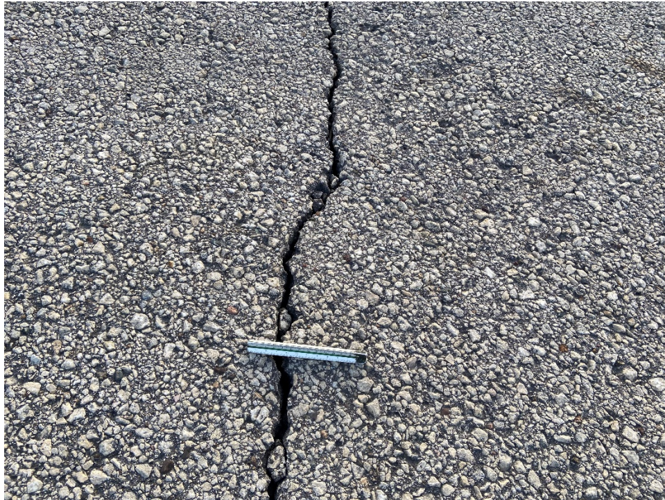
T03MQ-01. L&T Cracking (Sample Unit No. 01).
