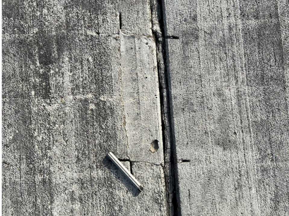
R15MQ-01. Small Patching (Sample Unit No. 06).
