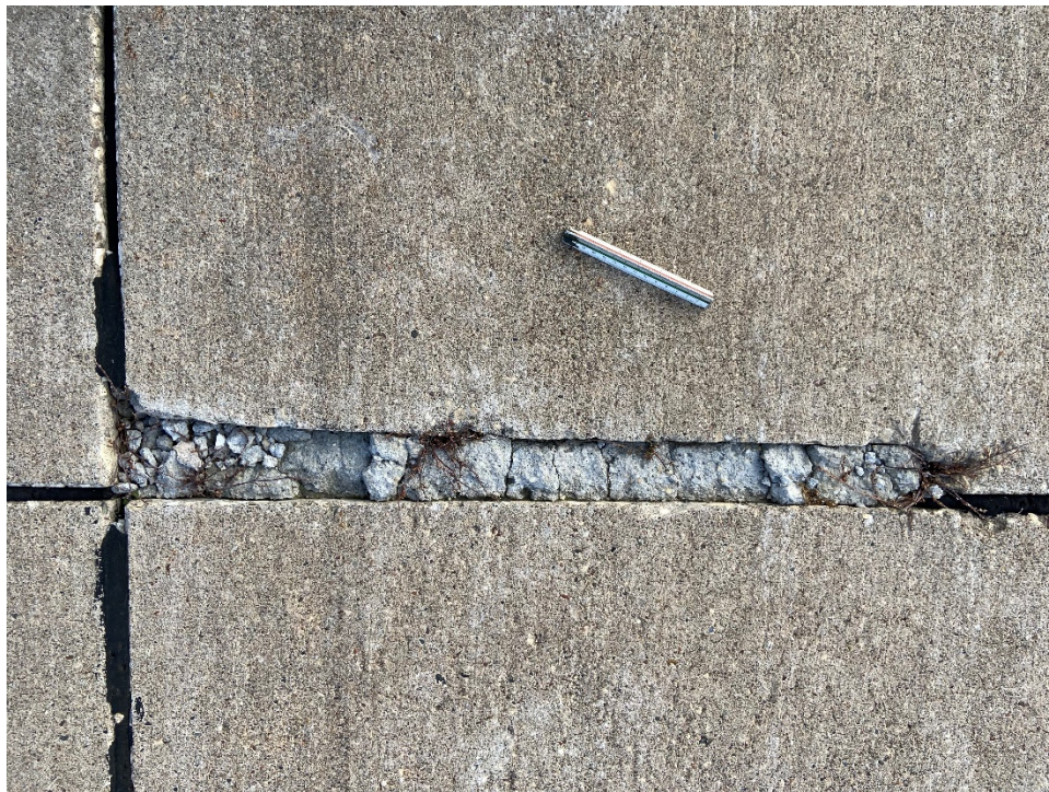
R15MQ-01. Small Patching (Sample Unit No. 60).
