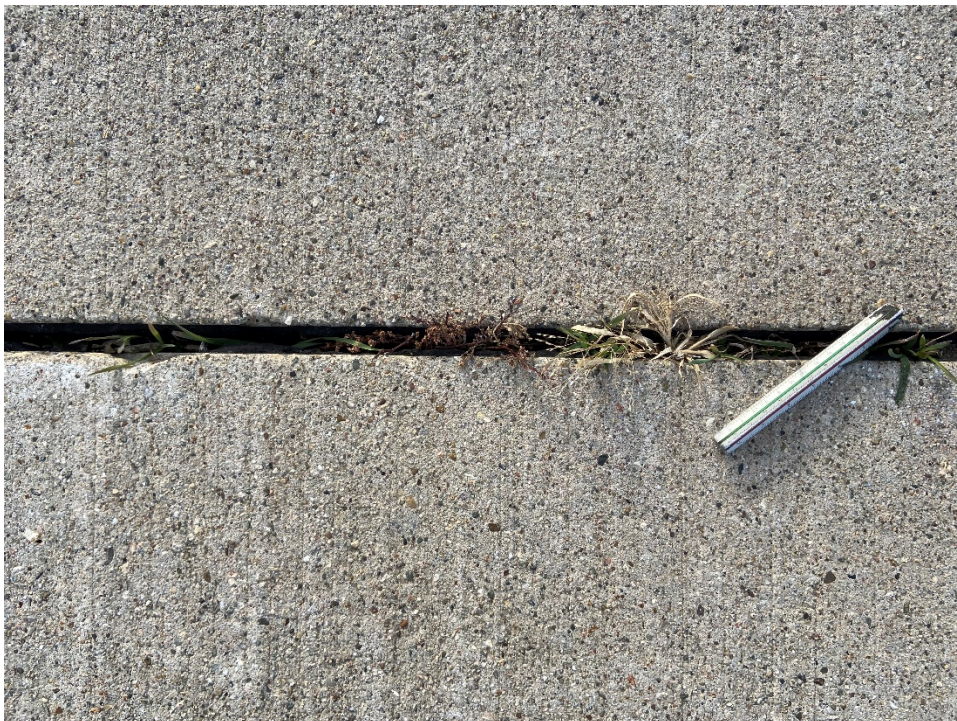
A01MQ-01. Joint Seal Damage (Sample Unit No. 01).
