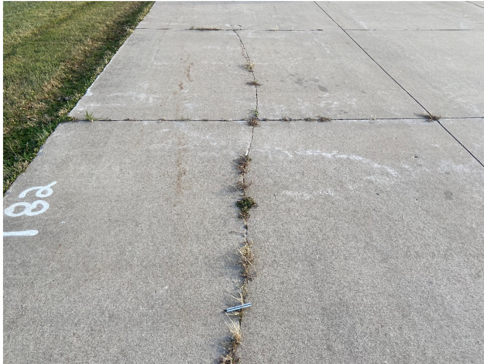
A01MQ-02. LTD Cracking (Additional Sample Unit No. 01).
