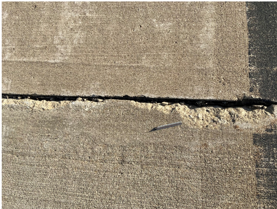
T04MQ-02. Joint Spalling (Sample Unit No. 05) (2).
