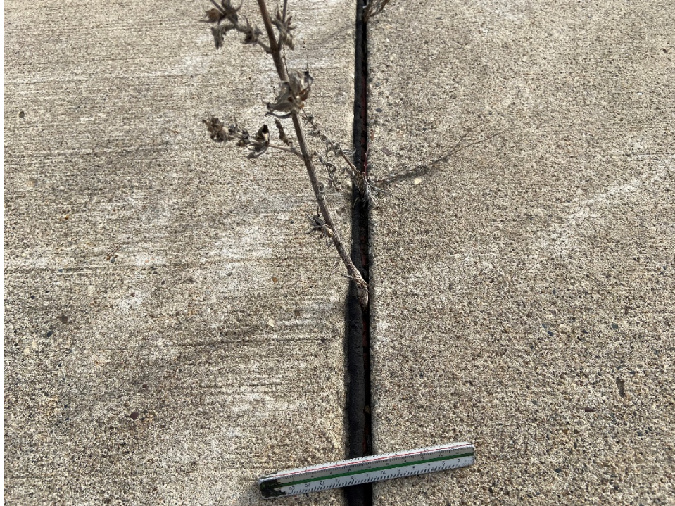
T01MQ-01. Joint Seal Damage (Sample Unit No. 05) (1).
