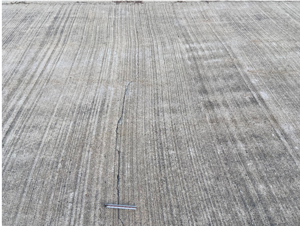
TH01MQ-02. LTD Cracking (Sample Unit No. 03).
