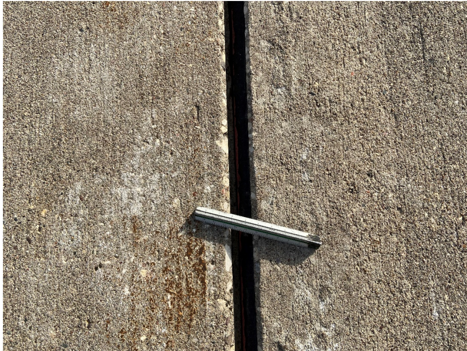
R15MQ-01. Joint Seal Damage (Sample Unit No. 06).
