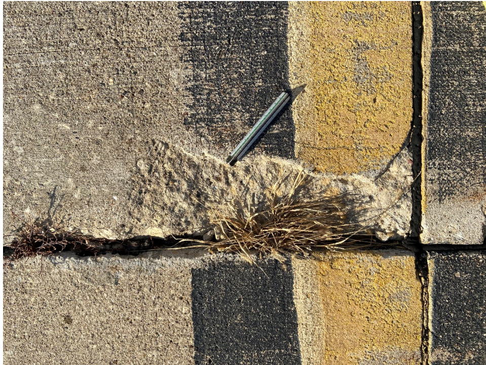
T04MQ-02. Joint Spalling (Sample Unit No. 05) (1).
