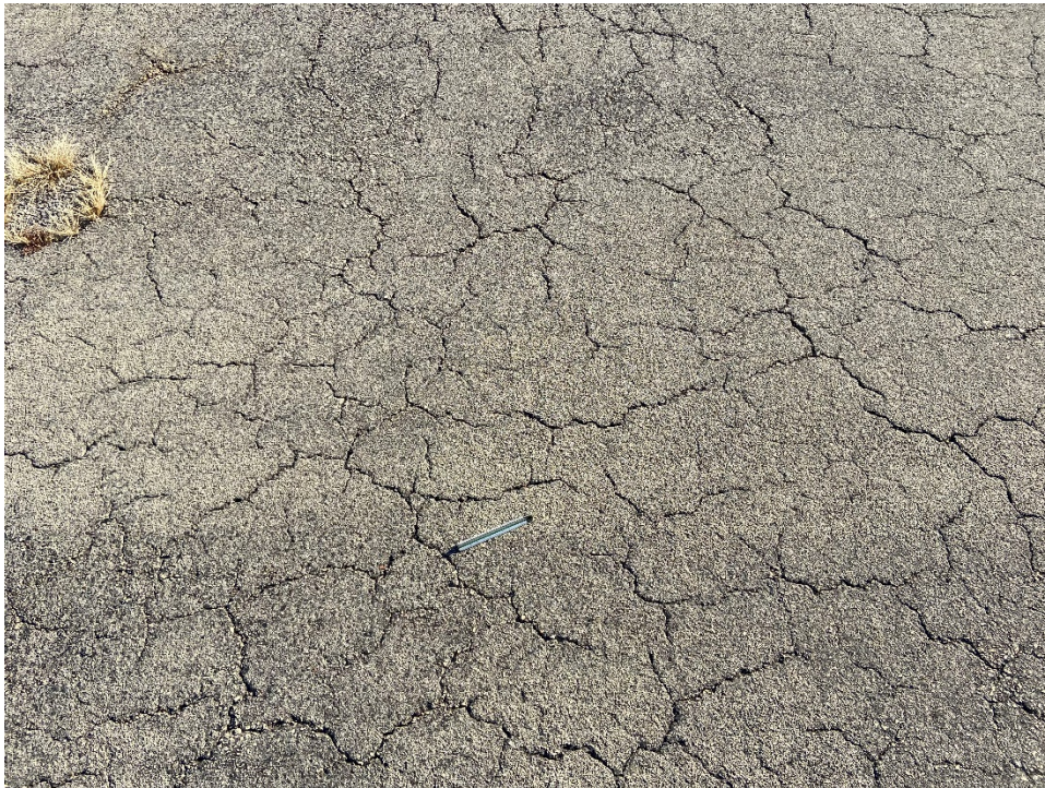
T02MQ-01. Alligator Cracking (Sample Unit No. 01).
