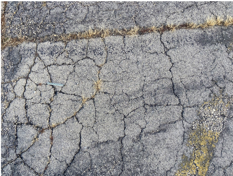
TH01MQ-01. Alligator Cracking (Sample Unit No. 01).
