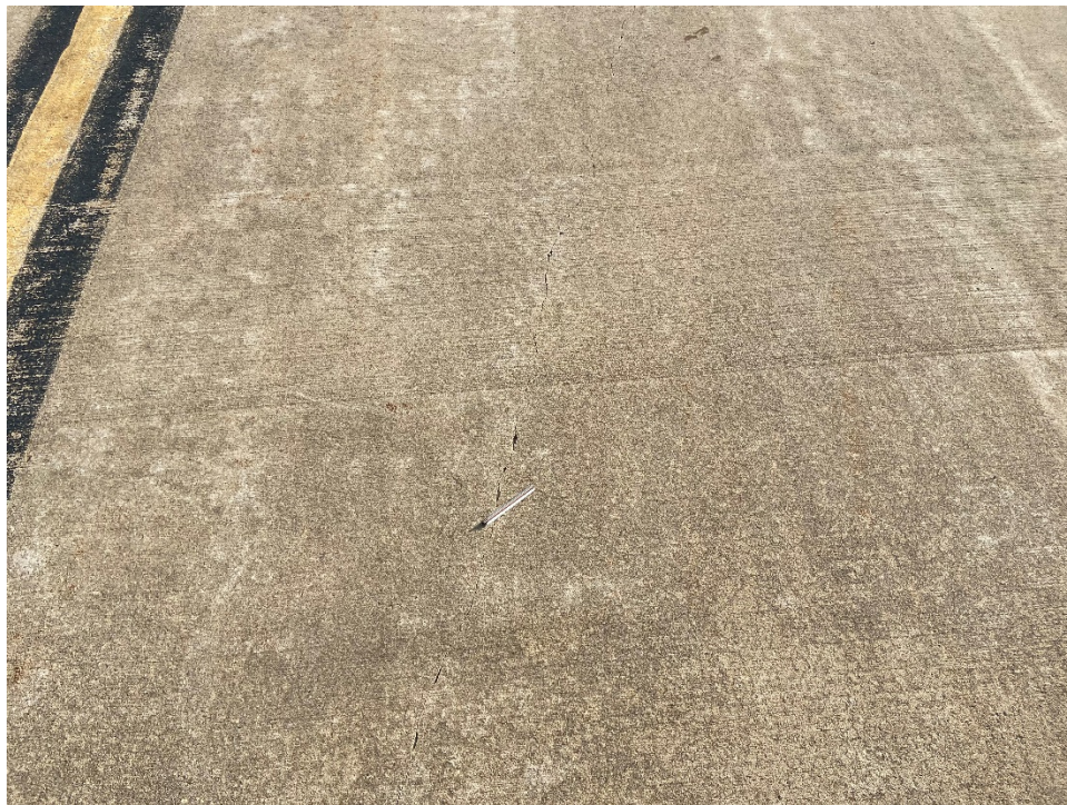
T04MQ-01. LTD Cracking (Sample Unit No. 01).
