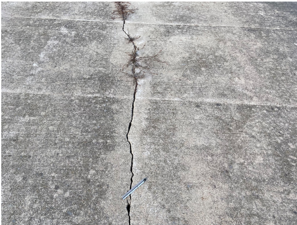
TH01MQ-02. LTD Cracking (Sample Unit No. 01).
