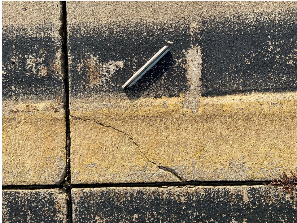
T04MQ-01. Corner Spalling (Sample Unit No. 01).
