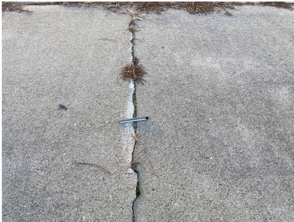
TH01MQ-03. LTD Cracking (Sample Unit No. 03).
