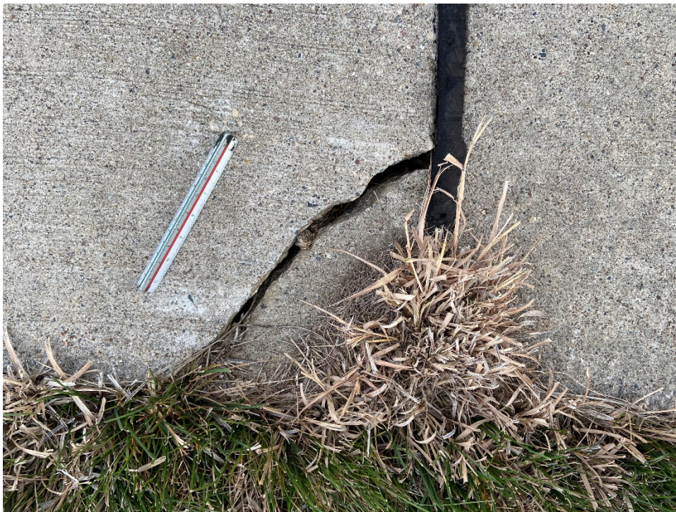
T01MQ-01. Corner Spalling (Sample Unit No. 05).
