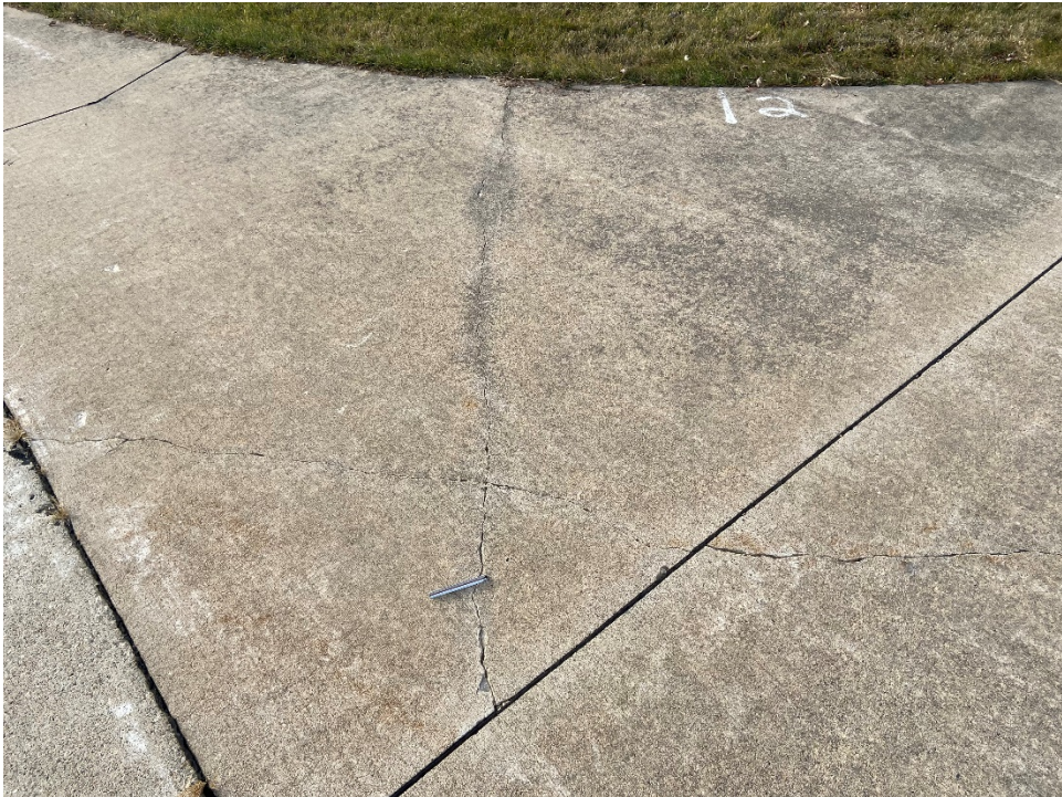
T04MQ-01. Shattered Slab (Sample Unit No. 01).
