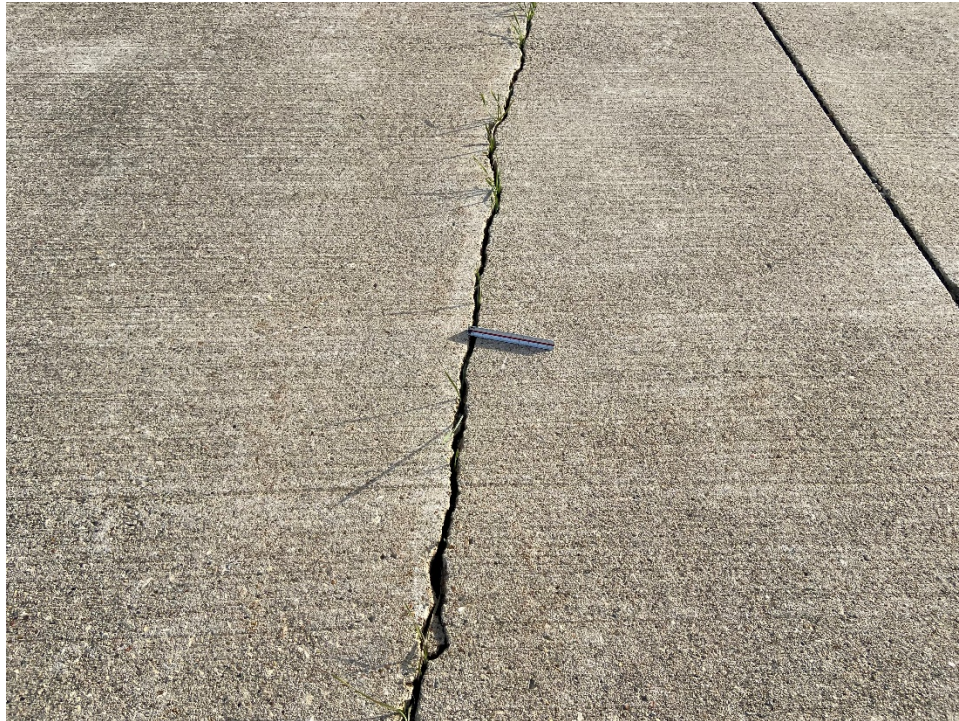
A01MQ-01. LTD Cracking (Sample Unit No. 01).
