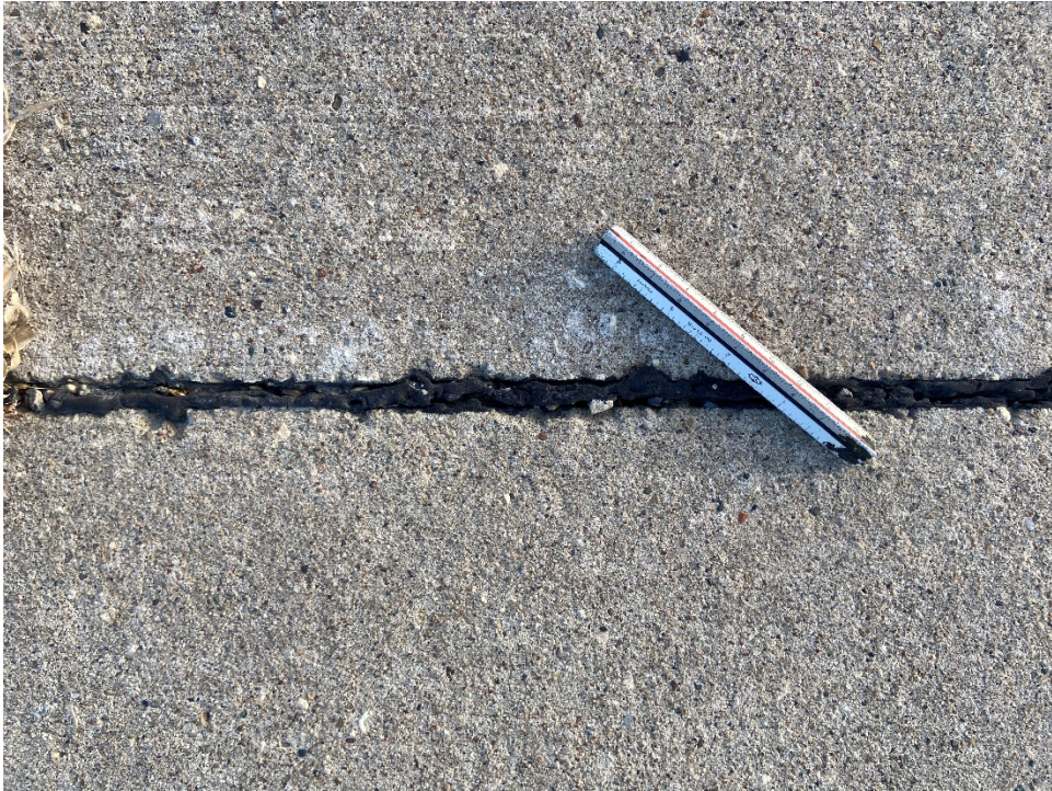
A01MQ-02. Joint Seal Damage (Sample Unit No. 02).
