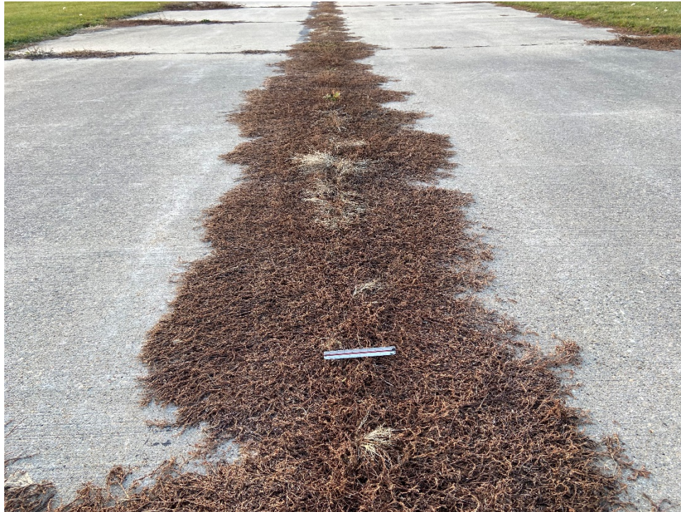
TH01MQ-03. Joint Seal Damage (Sample Unit No. 01).
