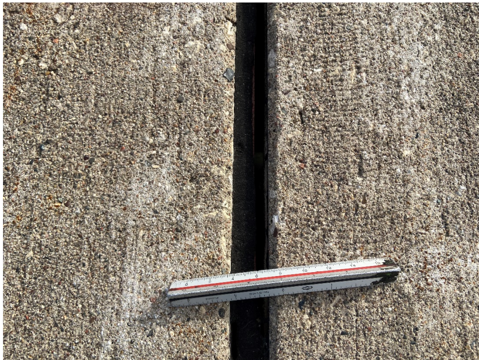
R15MQ-01. Joint Seal Damage (Sample Unit No. 69).
