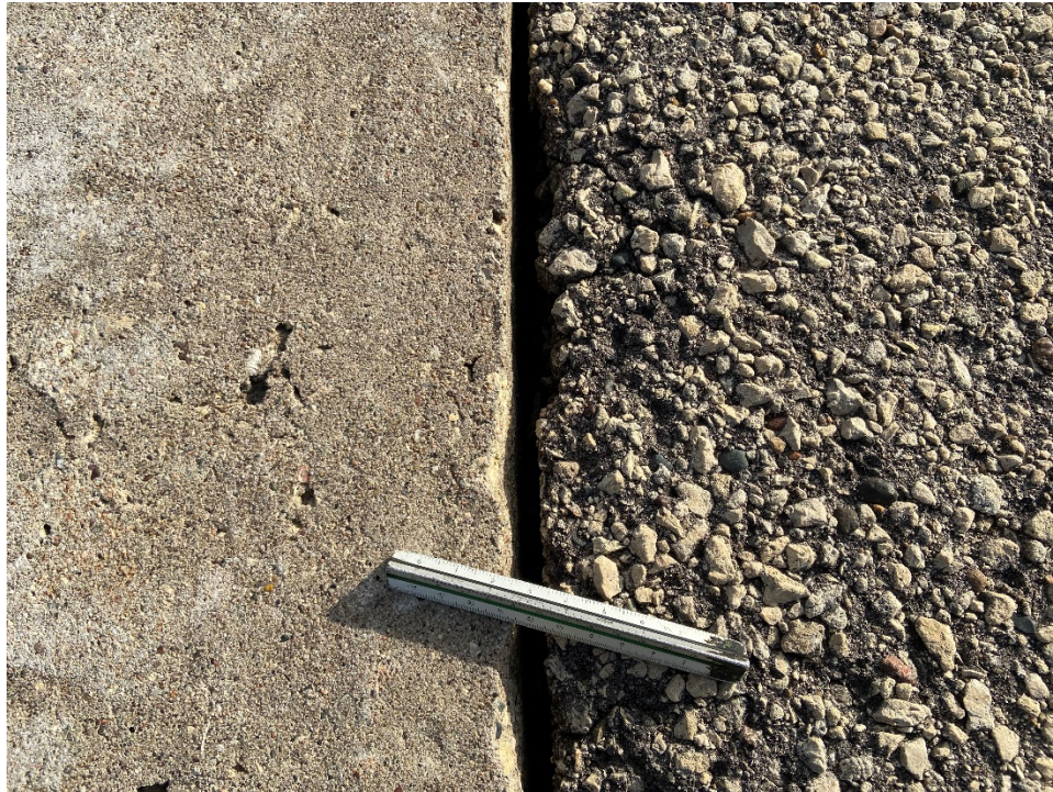
T02MQ-02. L&T Cracking (Sample Unit No. 01) (2).
