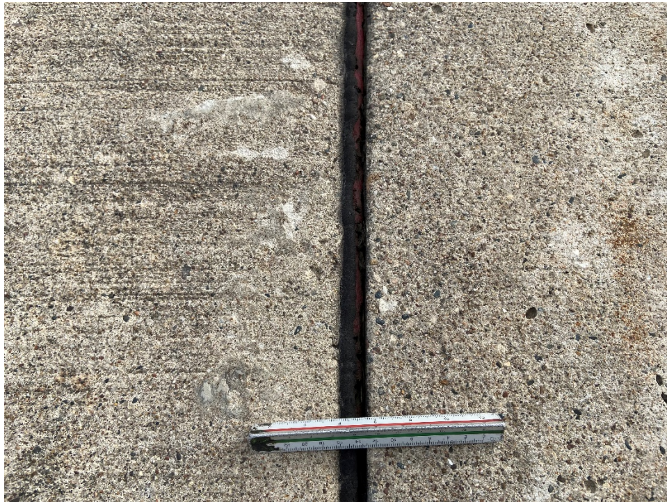
T01MQ-01. Joint Seal Damage (Sample Unit No. 05) (2).
