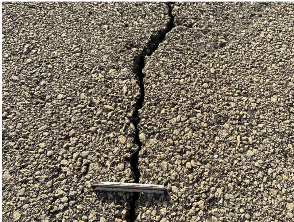
T02MQ-02. L&T Cracking (Sample Unit No. 01) (1).
