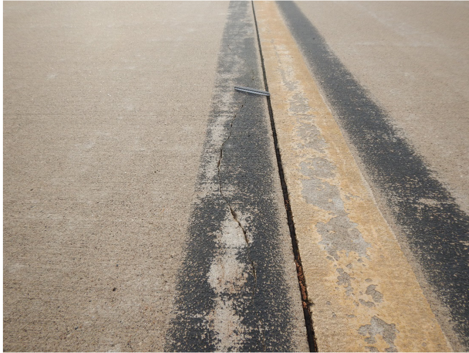
TBMQ-01. Joint Spalling (Sample Unit No. 01).
