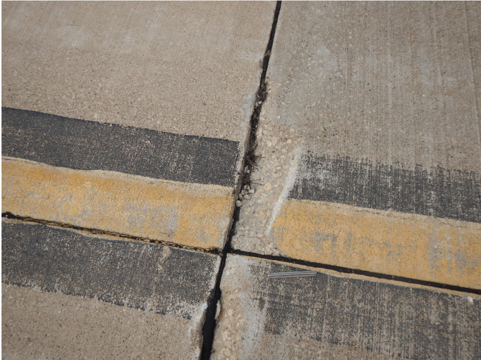
TBMQ-02. Joint Spalling (Sample Unit No. 05).
