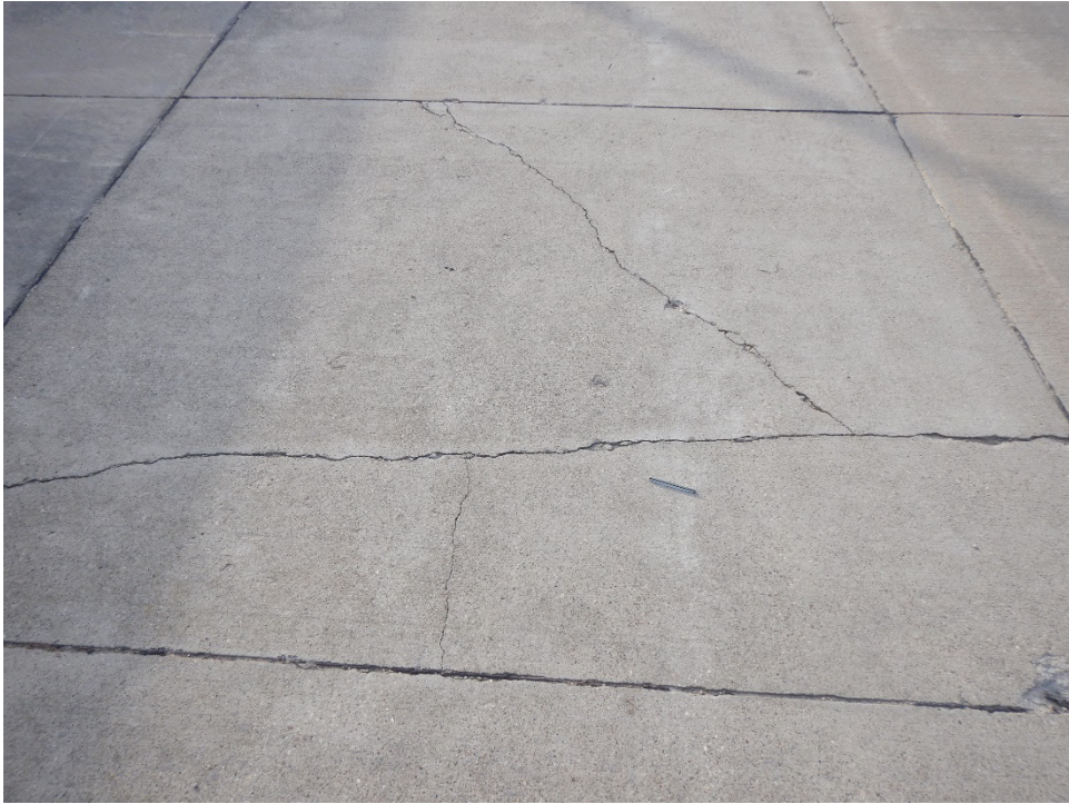
TH01MQ-03. Shattered Slab (Sample Unit No. 03).
