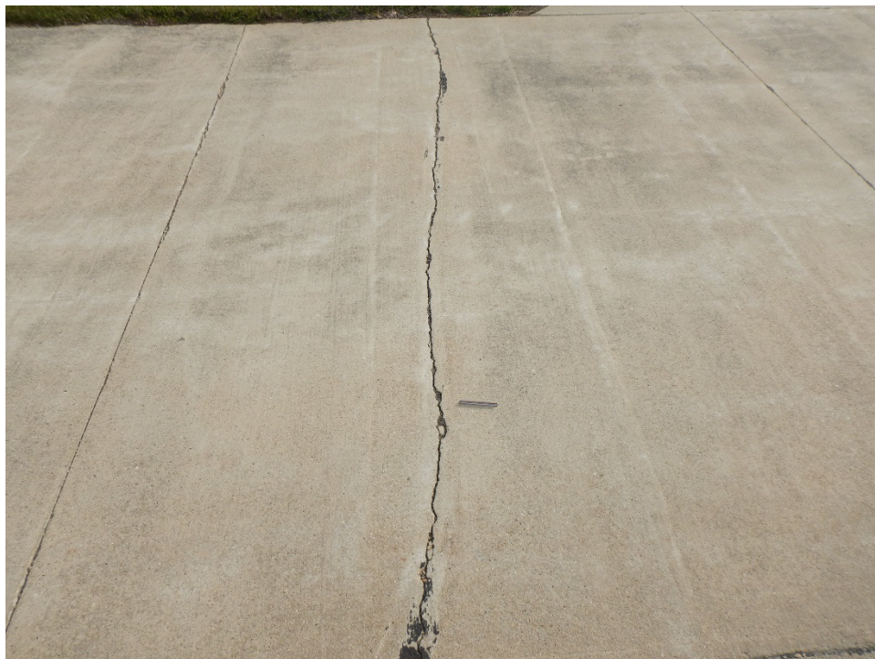
TH01MQ-02. LTD Cracking (Sample Unit No. 02).
