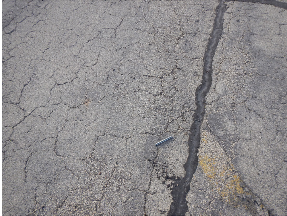
TH01MQ-01. Alligator Cracking (Sample Unit No. 01).
