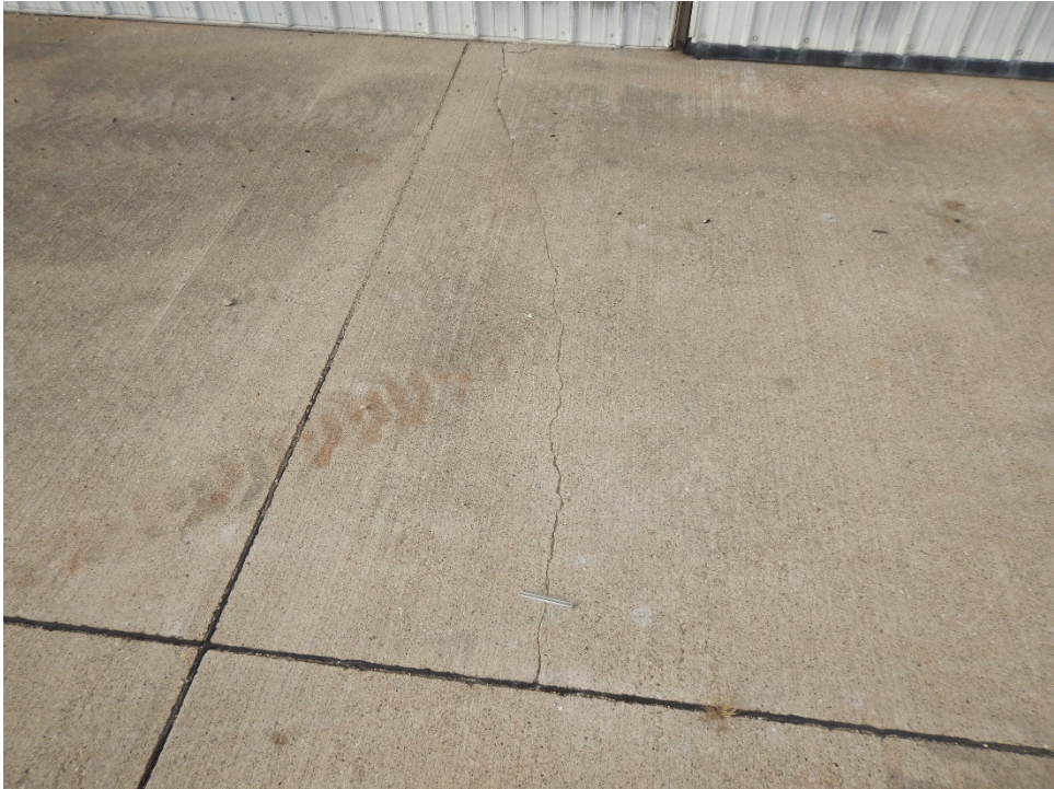
A01MQ-01. LTD Cracking (Sample Unit No. 11).
