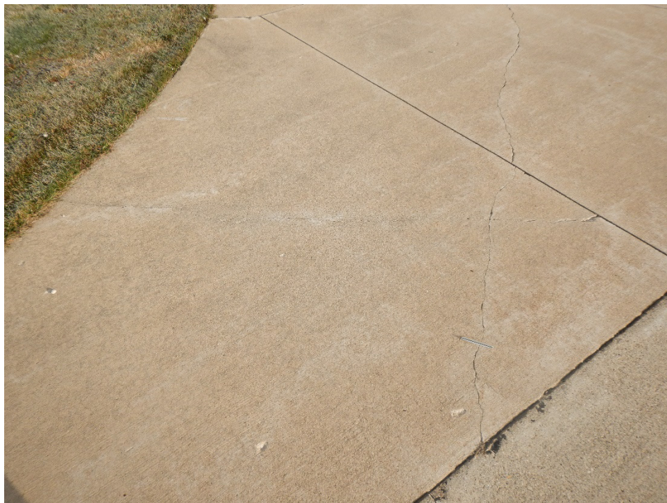
TBMQ-01. Shattered Slab (Sample Unit No. 01).
