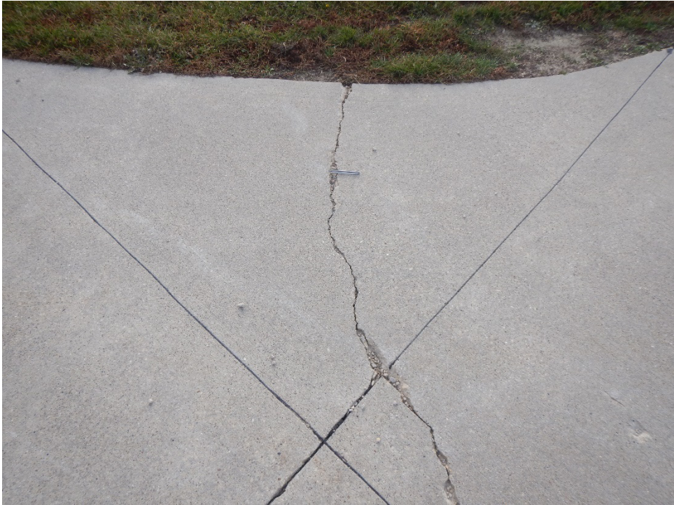
TH01MQ-03. LTD Cracking (Sample Unit No. 02).
