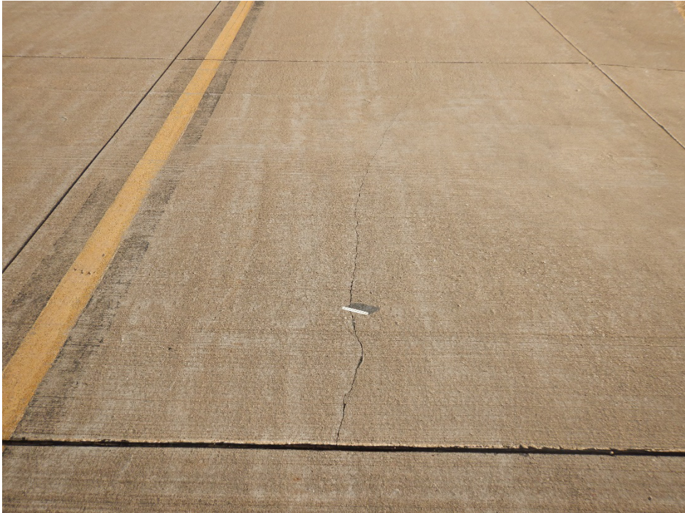
T01MQ-01. LTD Cracking (Sample Unit No. 02).
