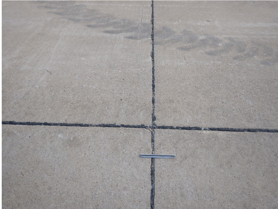
A01MQ-02. Joint Seal Damage (Sample Unit No. 07).
