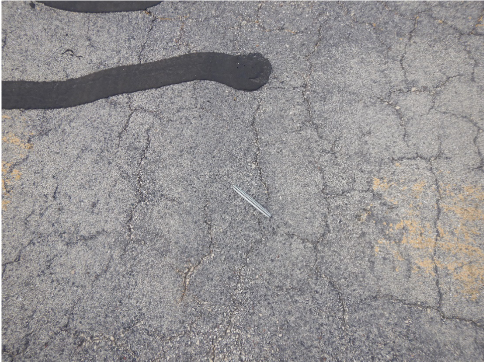
TAMQ-01. Alligator Cracking (Sample Unit No. 01).
