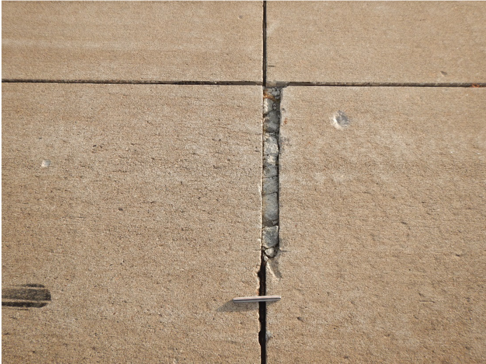
R15MQ-01. Small Patching (Sample Unit No. 60).
