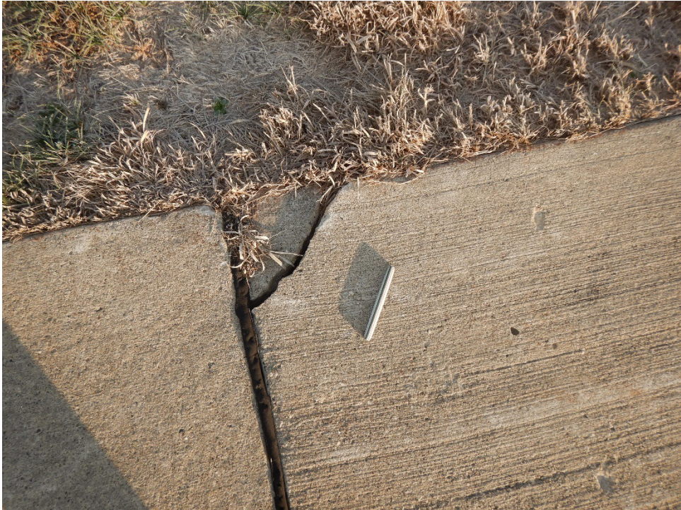
T01MQ-01. Corner Spalling (Sample Unit No. 05).
