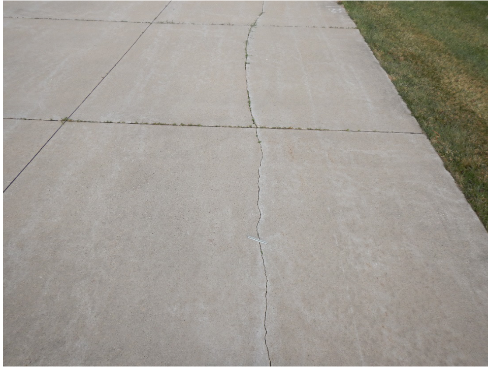
A01MQ-02. LTD Cracking (Additional Sample Unit No. 01).
