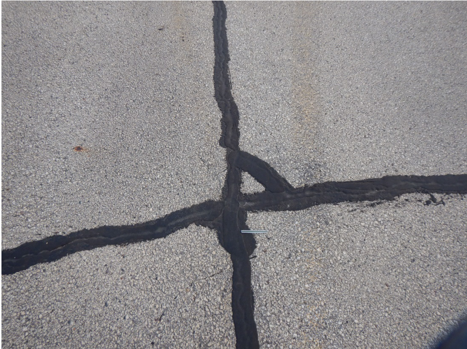
TAMQ-02. L&T Cracking (Sample Unit No. 01).
