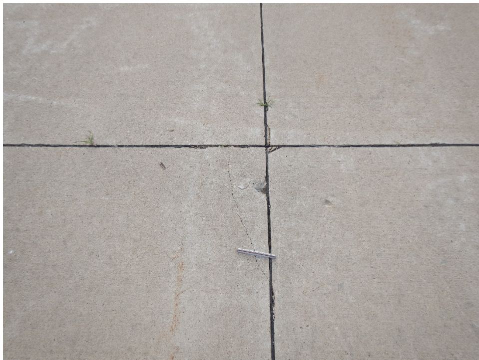
A01MQ-02. Joint Spalling (Sample Unit No. 02).
