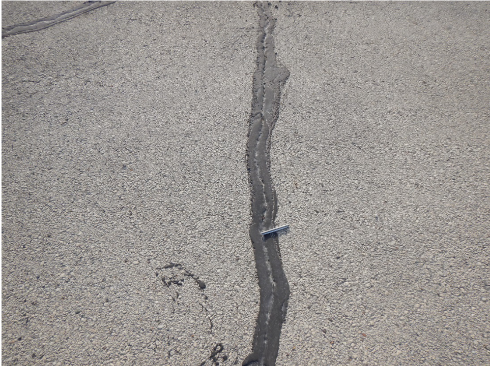
T03MQ-01. L&T Cracking (Sample Unit No. 01).
