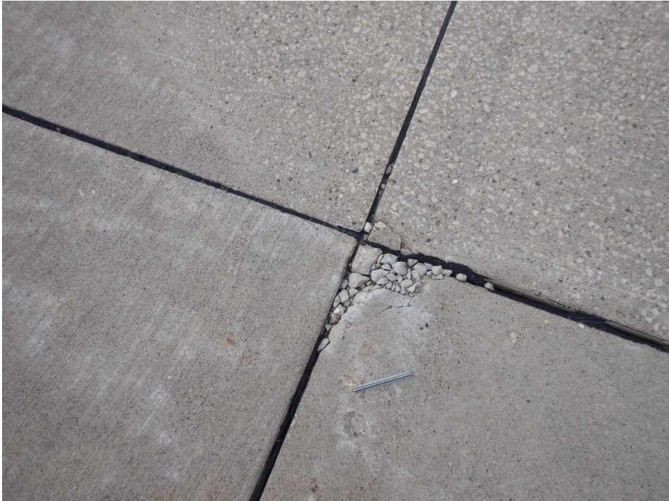
TBMQ-02. Corner Spalling (Sample Unit No. 03).
