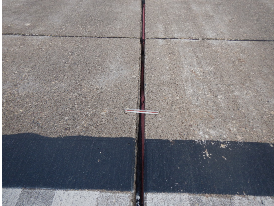
R15MQ-01. Joint Seal Damage (Sample Unit No. 06).
