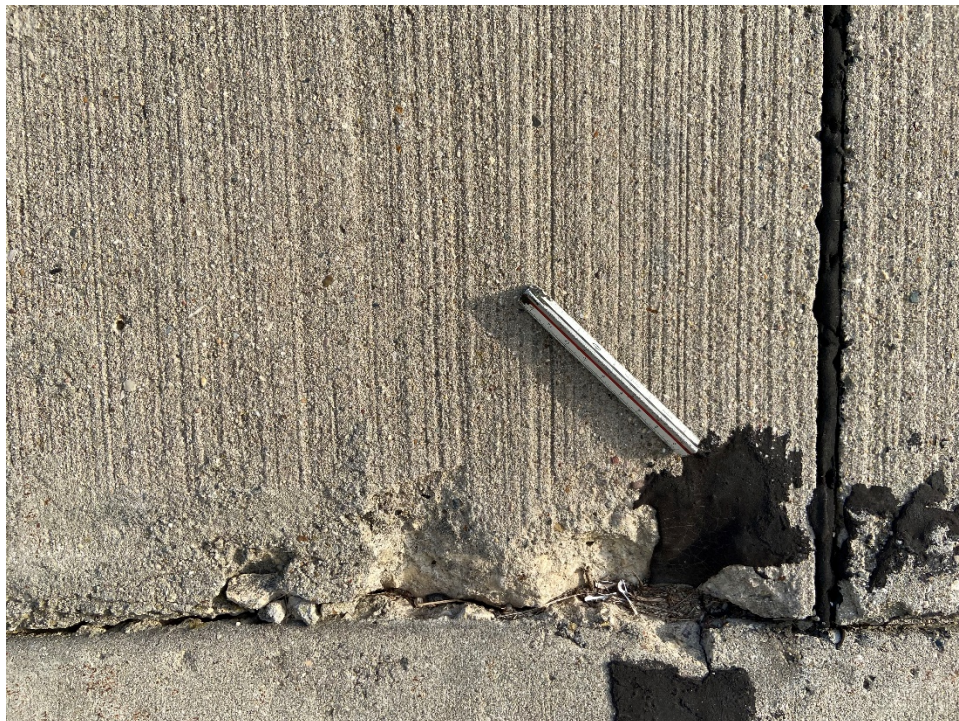
TH01MO-02. Joint Spalling (Sample Unit No. 03).
