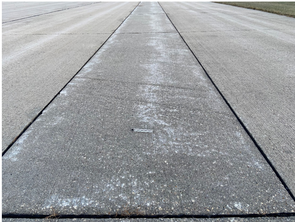
R15MO-01. Large Patching (Sample Unit No. 35).
