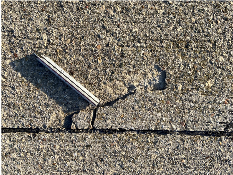
TH01MO-03. Joint Spalling (Sample Unit No. 04).
