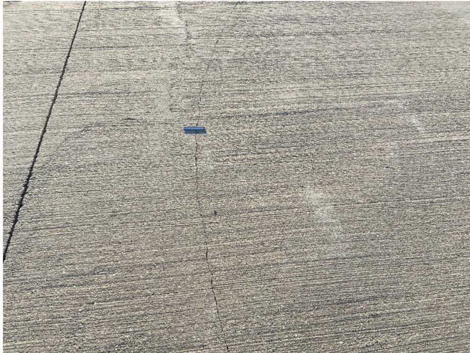
TH01MO-01. LTD Cracking (Sample Unit No. 03).
