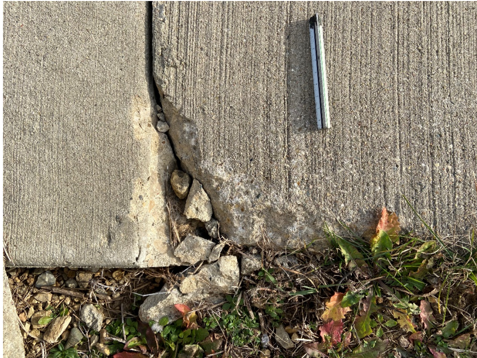
TH01MO-02. Corner Spalling (Sample Unit No. 04).
