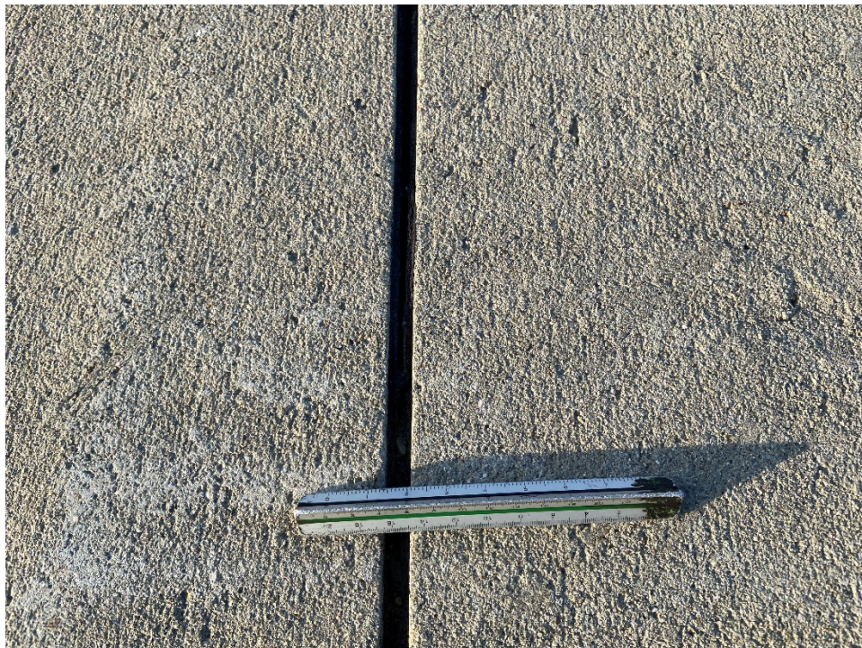
TH01MO-05. Joint Seal Damage (Sample Unit No. 06).
