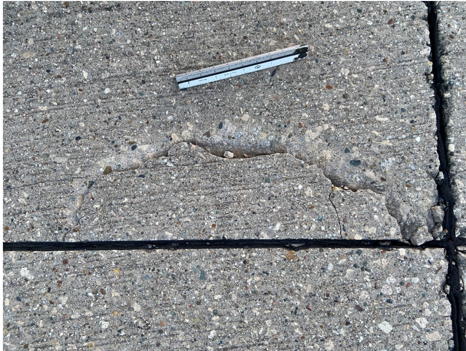
R15MO-01. Joint Spalling (Sample Unit No. 05).
