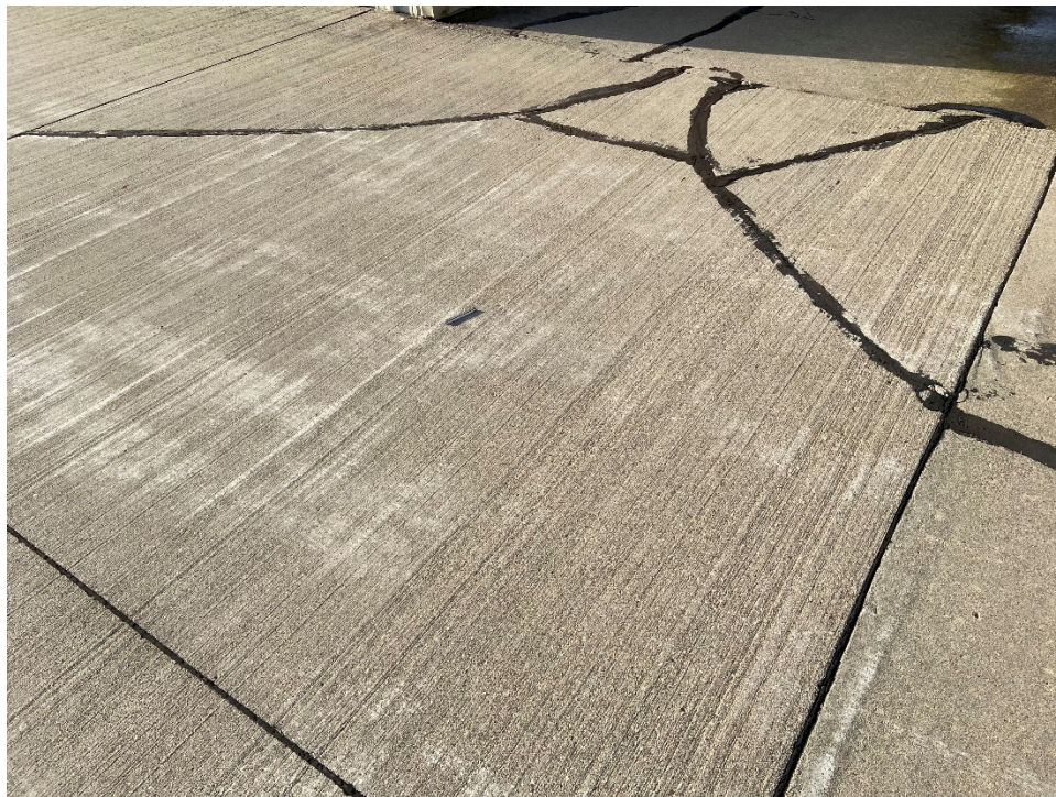
TH01MO-02. Shattered Slab (Sample Unit No. 01).
