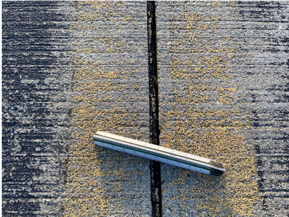
TH01MO-01. Joint Seal Damage (Sample Unit No. 01) (1).
