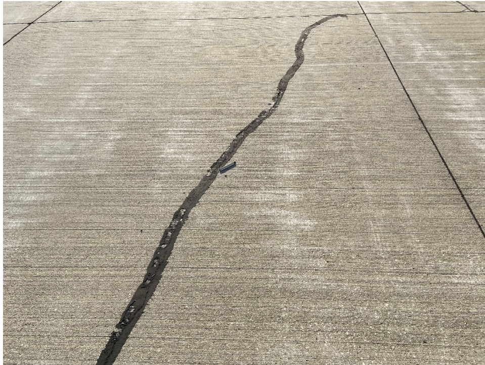
TH01MO-02. LTD Cracking (Sample Unit No. 01).
