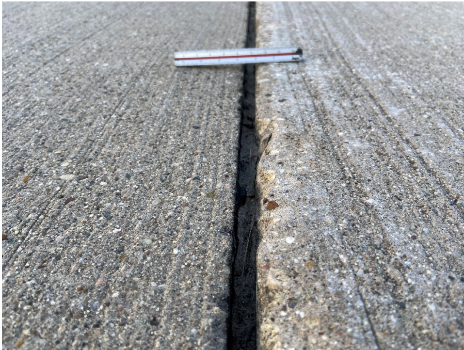
TH01MO-01. Faulting (Sample Unit No. 02).
