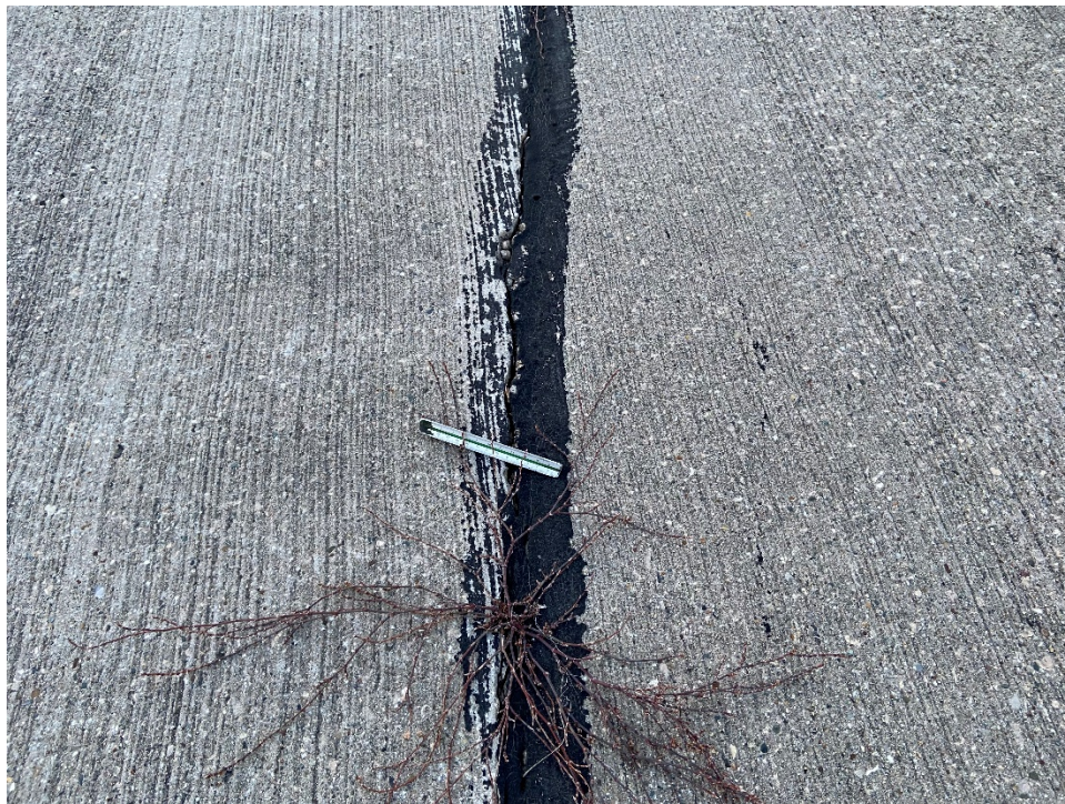
R15MO-01. LTD Cracking (Sample Unit No. 05).
