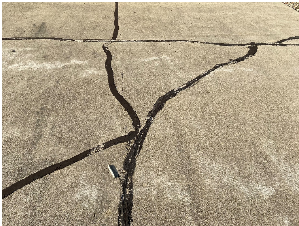
TH01MO-04. Shattered Slab (Sample Unit No. 01).
