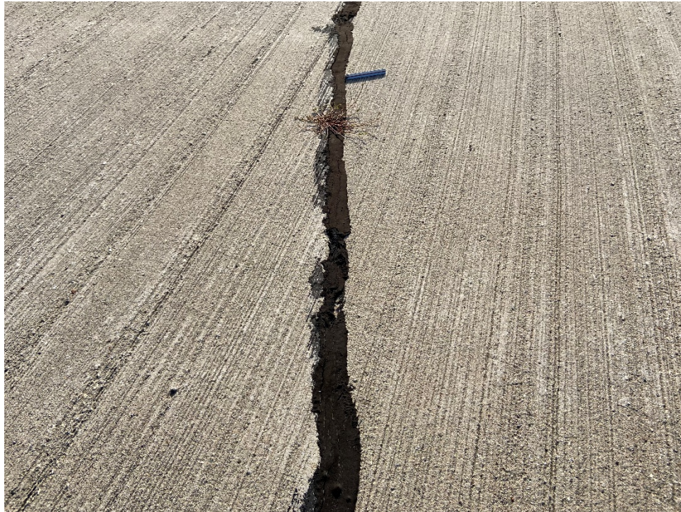
A01MO-01. LTD Cracking (Sample Unit No. 44).
