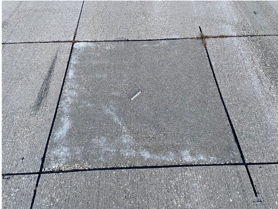
R15MO-01. Large Patching (Sample Unit No. 05).
