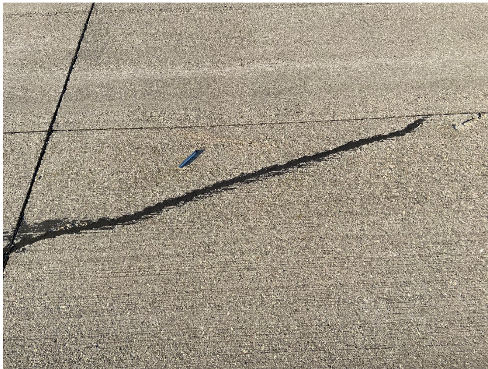
TH01MO-03. Corner Break (Sample Unit No. 04).
