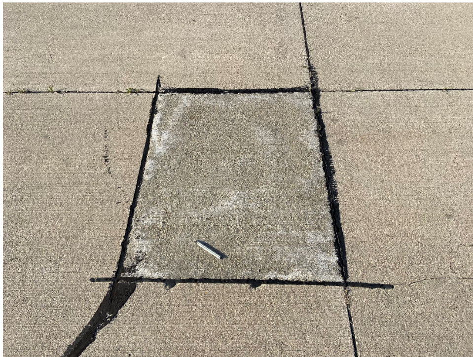
A01MO-01. Large Patching (Sample Unit No. 44).
