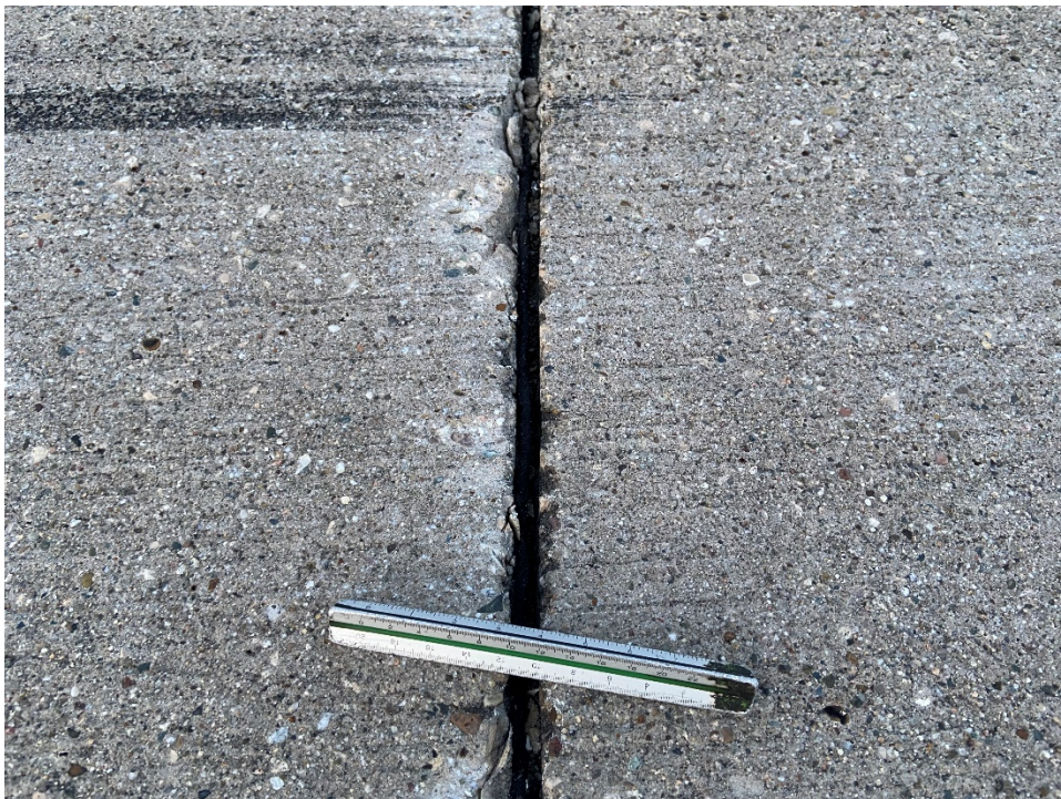
R15MO-01. Joint Seal Damage (Sample Unit No. 05).
