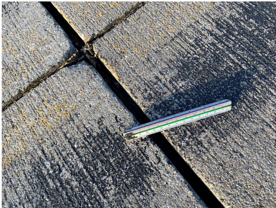
TH01MO-01. Joint Seal Damage (Sample Unit No. 01) (2).
