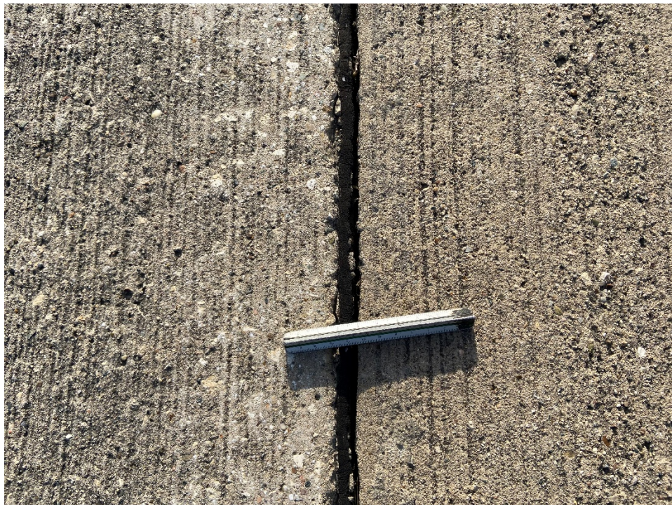
A01MO-01. Joint Seal Damage (Sample Unit No. 36).
