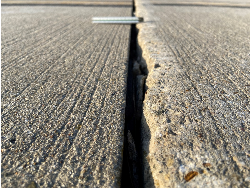
TH01MO-01. Faulting (Sample Unit No. 01).
