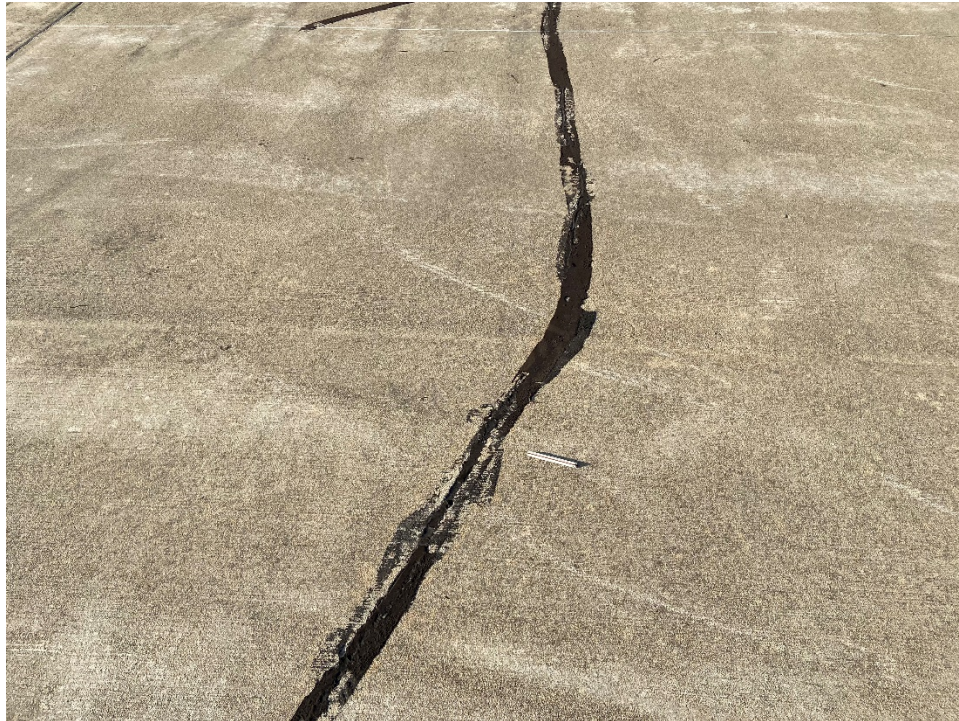
TH01MO-04. LTD Cracking (Sample Unit No. 01).
