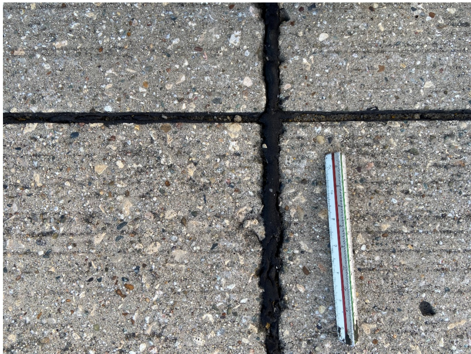
T01MO-01. Joint Seal Damage (Sample Unit No. 48).
