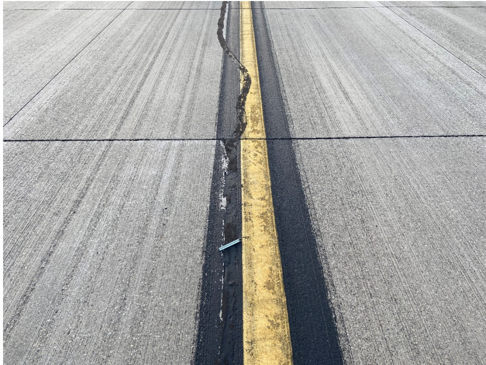
T01MO-01. LTD Cracking (Sample Unit No. 48).
