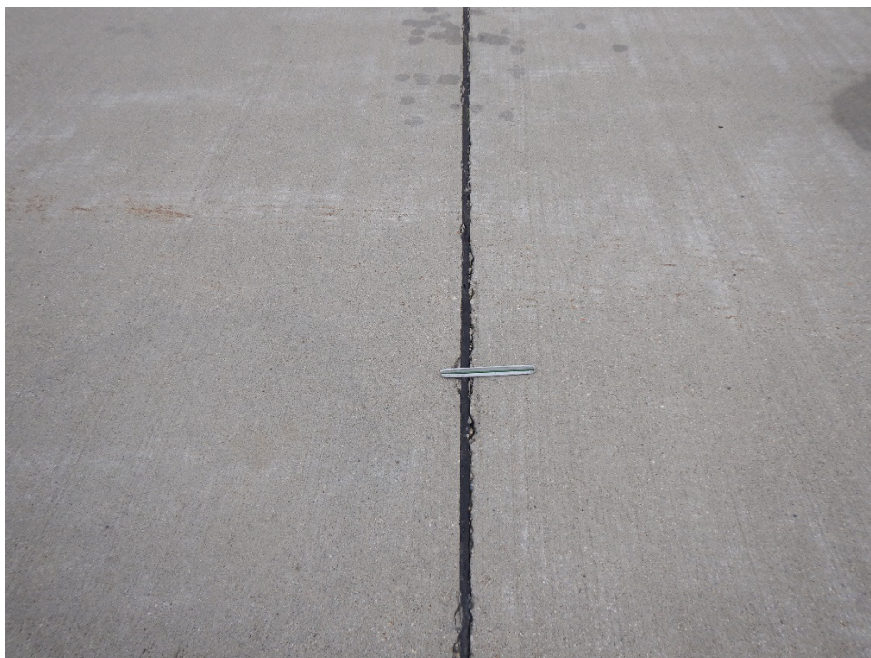
TH01MO-02. Joint Seal Damage (Sample Unit No. 02).
