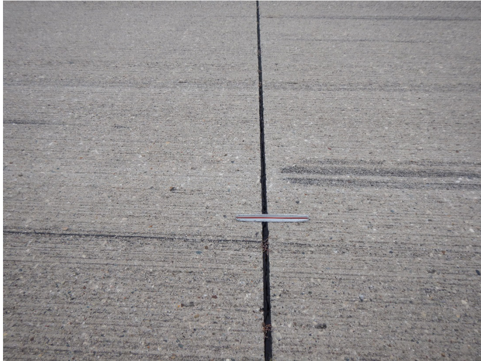
R15MO-01. Joint Seal Damage (Sample Unit No. 75).
