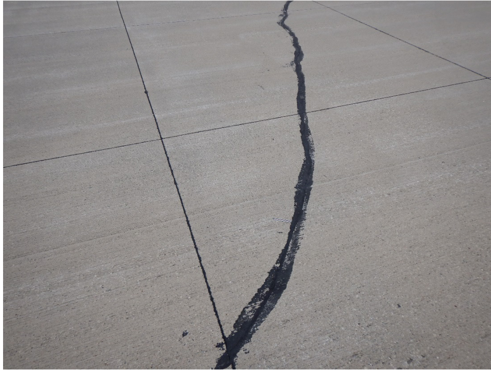
A01MO-01. LTD Cracking (Sample Unit No. 16).
