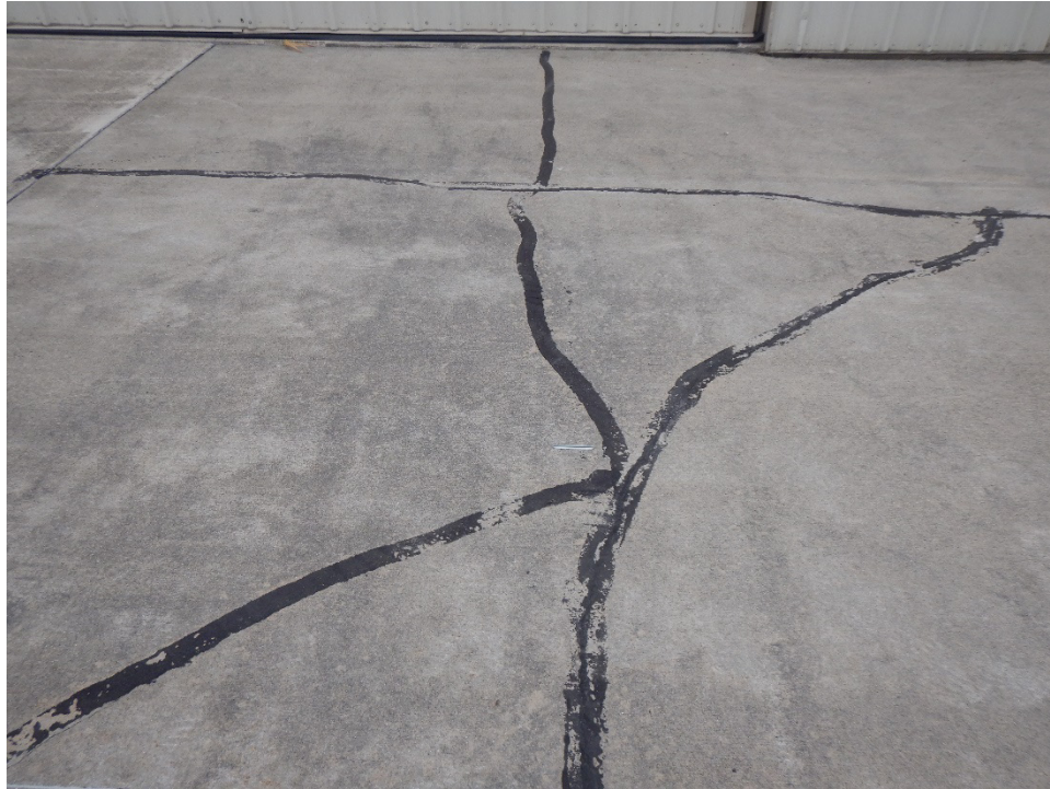
TH01MO-04. Shattered Slab (Sample Unit No. 01).
