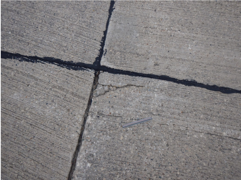
TH01MO-03. Joint Spalling (Sample Unit No. 02).
