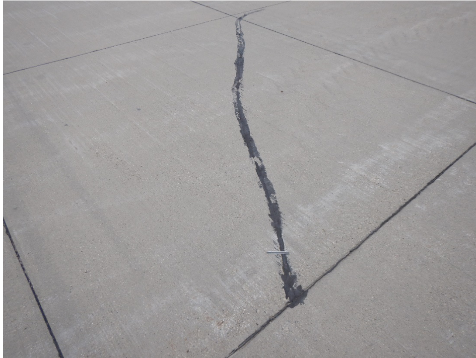
TH01MO-02. LTD Cracking (Sample Unit No. 04).
