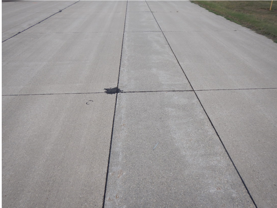
R15MO-01. Large Patching (Sample Unit No. 55).
