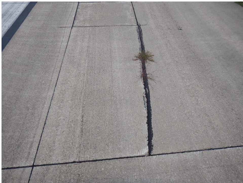
R15MO-01. LTD Cracking (Sample Unit No. 05).
