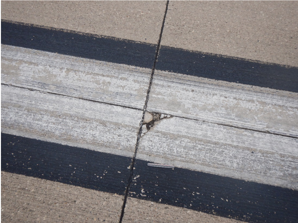
R15MO-01. Corner Spalling (Sample Unit No. 25).
