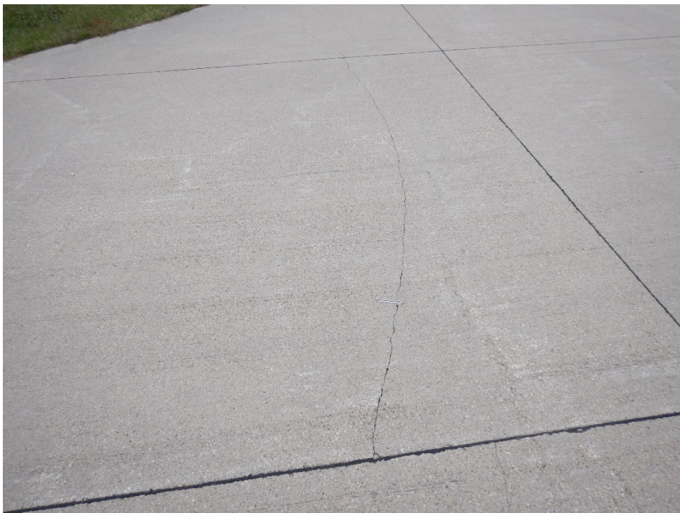
TH01MO-01. LTD Cracking (Sample Unit No. 03).
