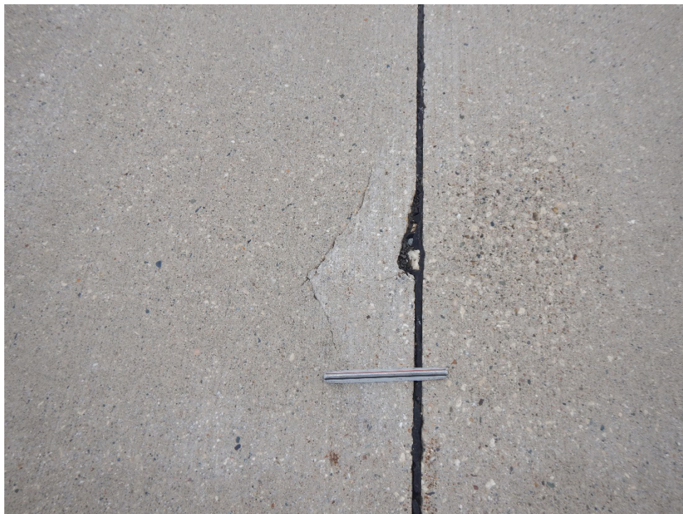
T01MO-01. Joint Spalling (Sample Unit No. 33).
