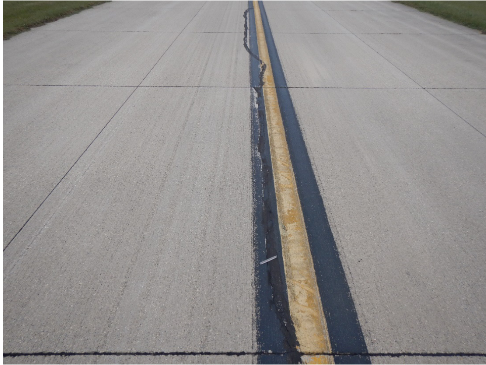
T01MO-01. LTD Cracking (Sample Unit No. 48).
