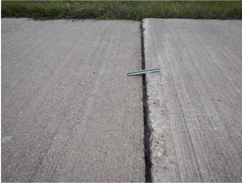
TH01MO-01. Faulting (Sample Unit No. 02).
