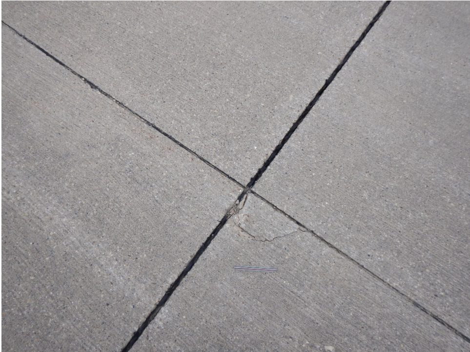
TH01MO-03. Corner Spalling (Sample Unit No. 08).
