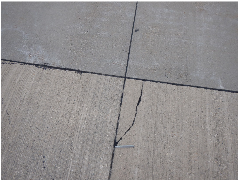
A01MO-01. Joint Spalling (Sample Unit No. 32).
