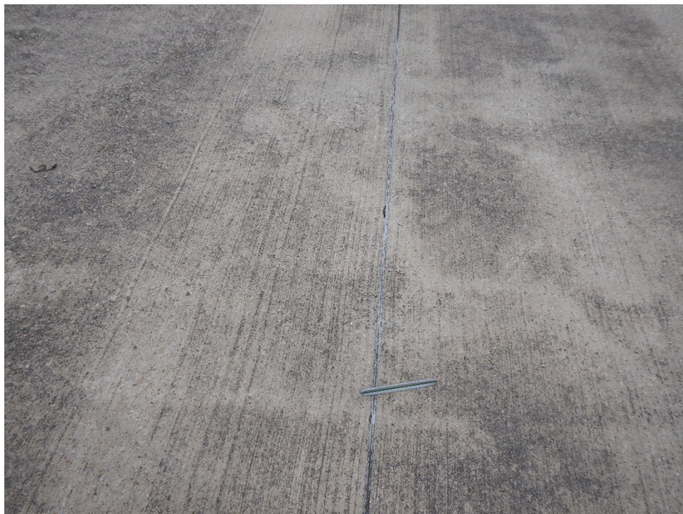
TH01MO-04. Joint Seal Damage (Sample Unit No. 01).
