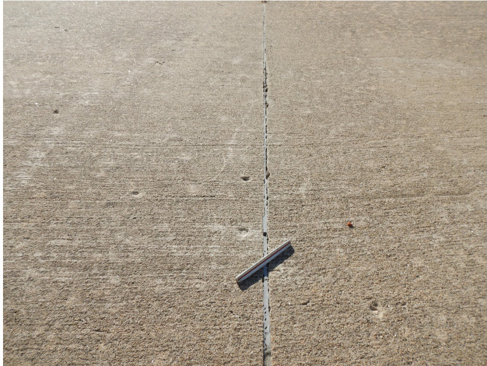
TH01MP-02. Joint Seal Damage (Sample Unit No. 01).
