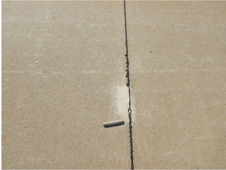
TH01MP-01. Small Patching (Sample Unit No. 07).
