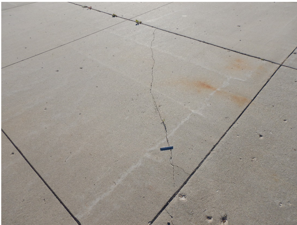
A02MP-02. LTD Cracking (Sample Unit No. 01).
