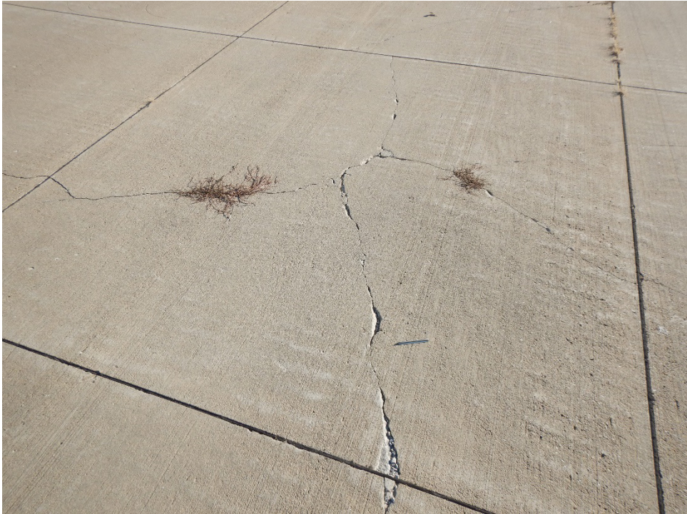
A02MP-01. Shattered Slab (Sample Unit No. 06).
