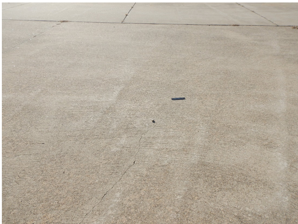
TH01MP-02. LTD Cracking (Sample Unit No. 01).
