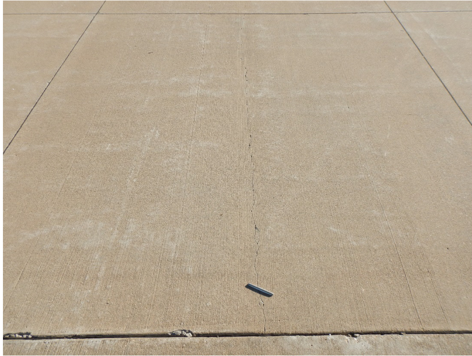
A02MP-03. LTD Cracking (Sample Unit No. 06).
