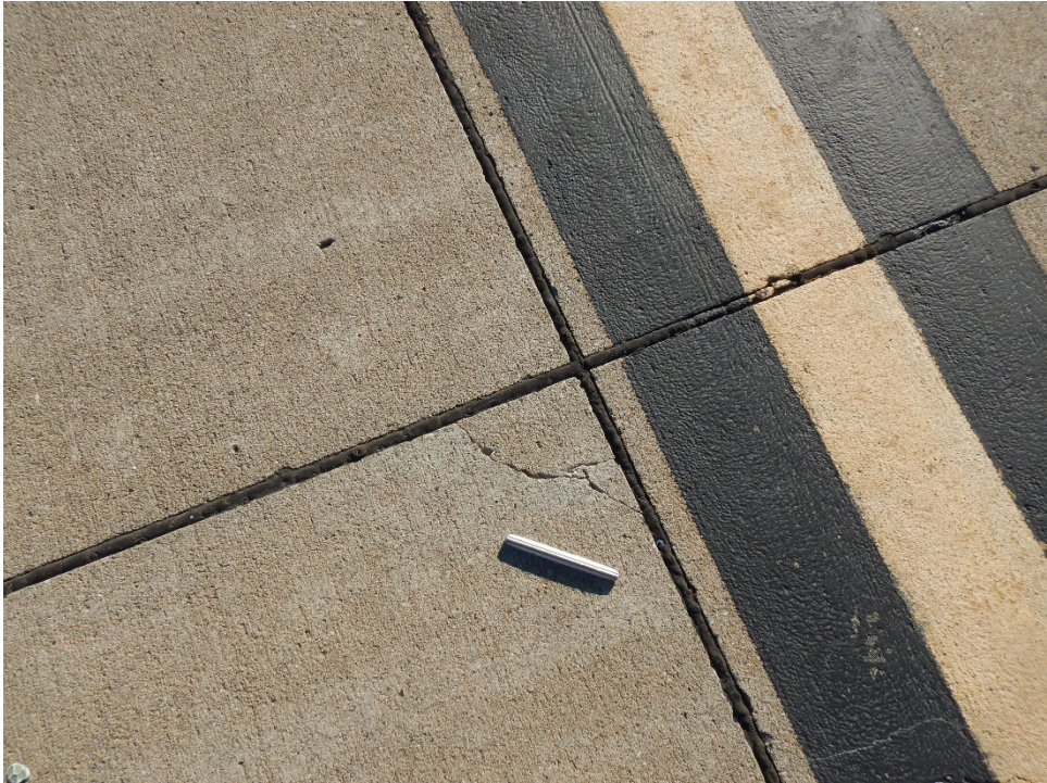
A02MP-01. Corner Spalling (Sample Unit No. 18).
