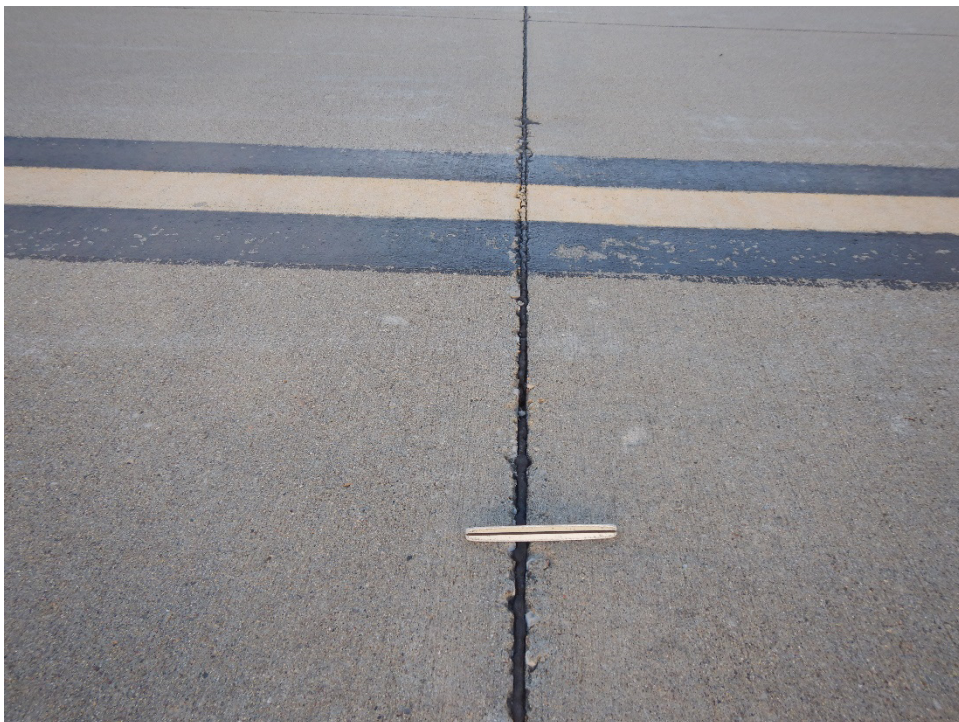
TH01MP-01. Joint Seal Damage (Sample Unit No. 08).
