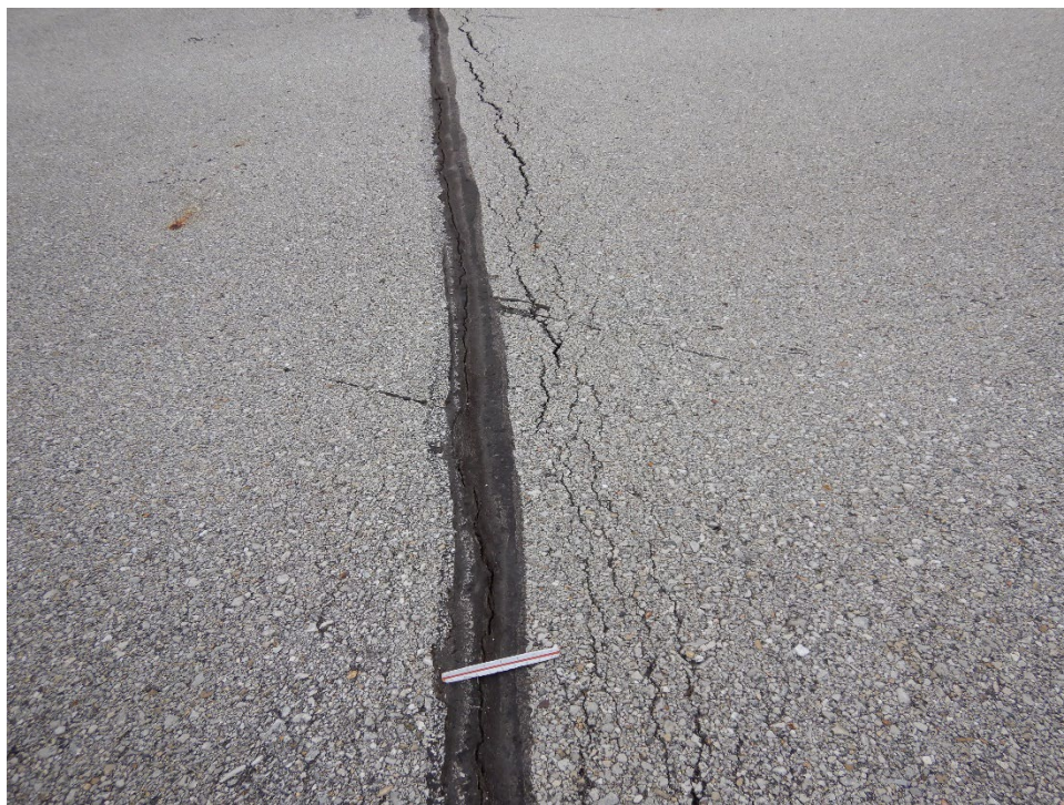
T05NE-01. L&T Cracking (Sample Unit No. 20) (2).
