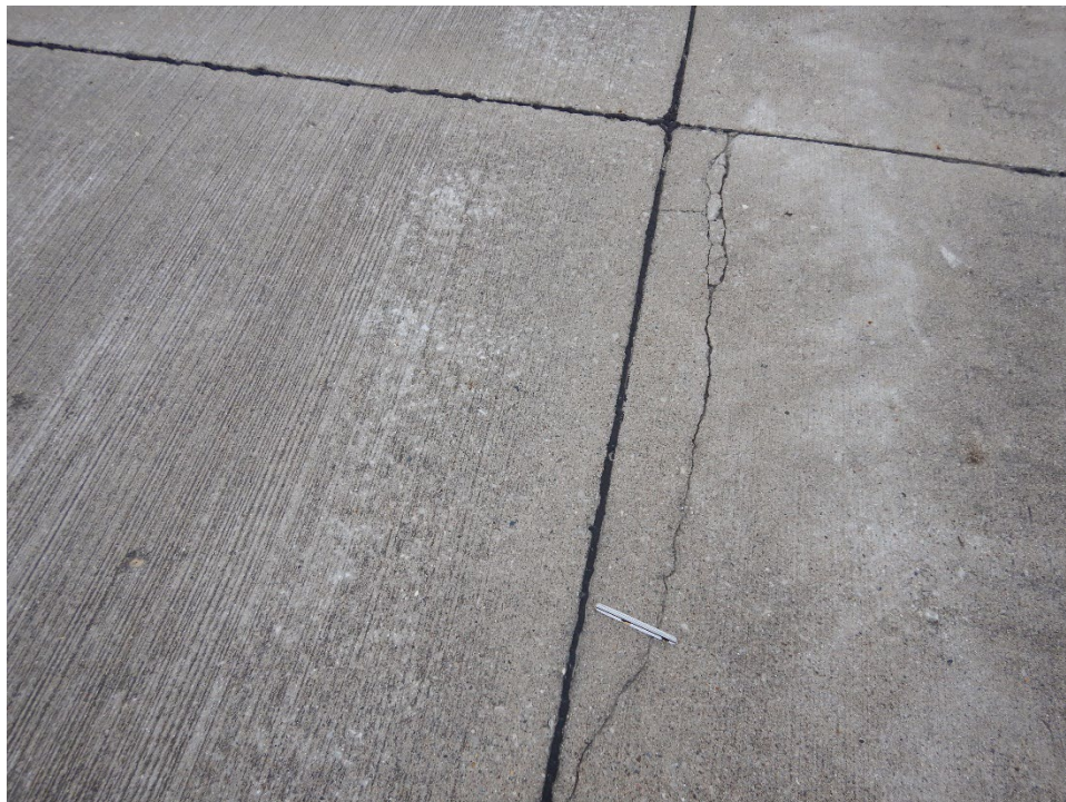
A01NE-01. Joint Spalling (Sample Unit No. 17).
