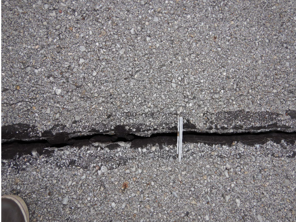
T02NE-02. L&T Cracking (Sample Unit No. 01).
