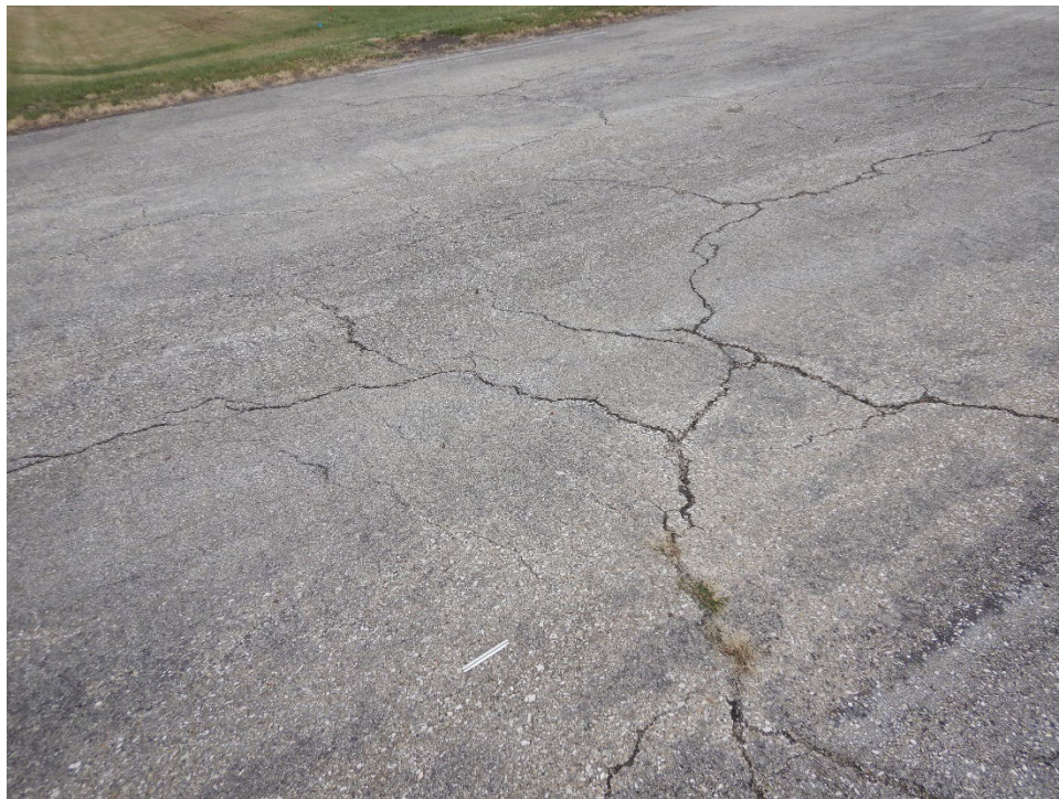
A02NE-01. Block Cracking (Sample Unit No. 02).
