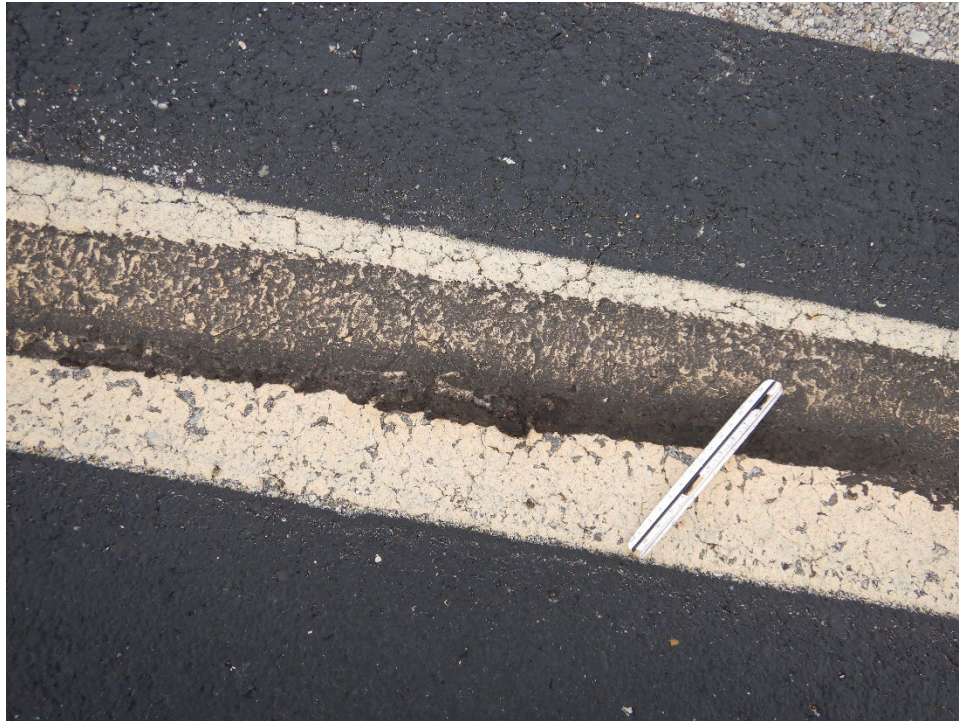
T05NE-01. L&T Cracking (Sample Unit No. 20) (1).
