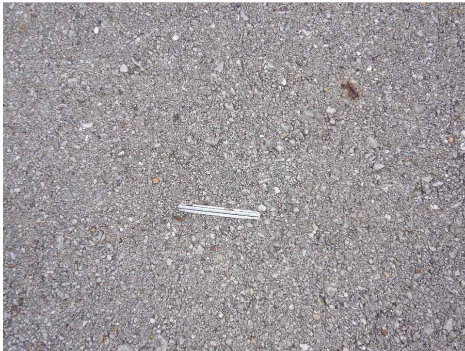
T06NE-01. Weathering (Sample Unit No. 02).
