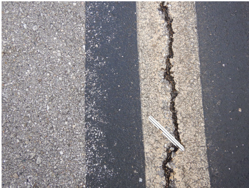
T07NE-01. L&T Cracking (Sample Unit No. 02) (1).
