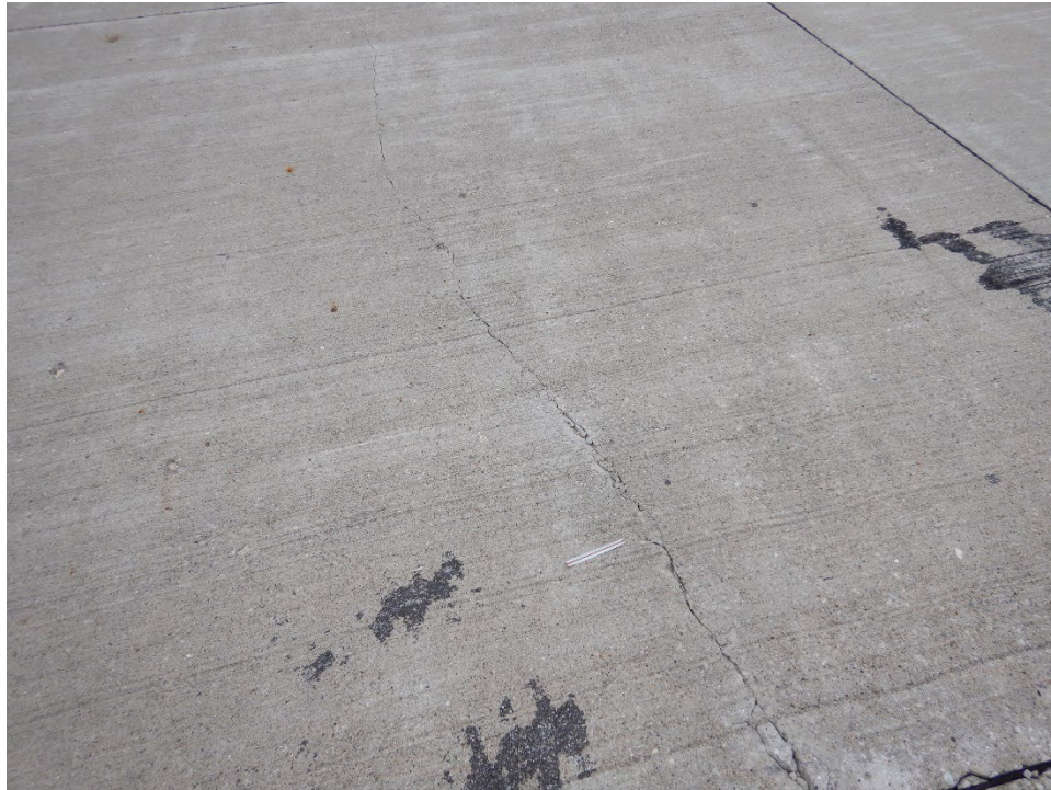
T02NE-01. LTD Cracking (Sample Unit No. 01).
