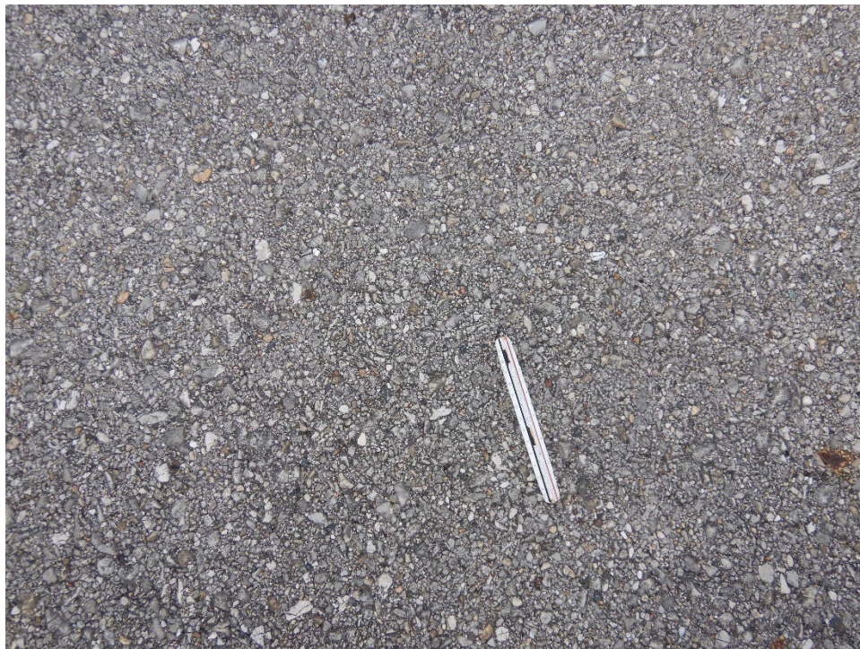
T07NE-01. Weathering (Sample Unit No. 02).
