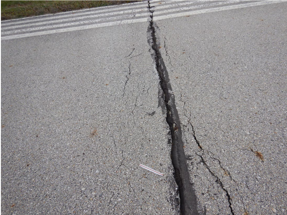
R14NE-02. L&T Cracking (Sample Unit No. 14) (2).
