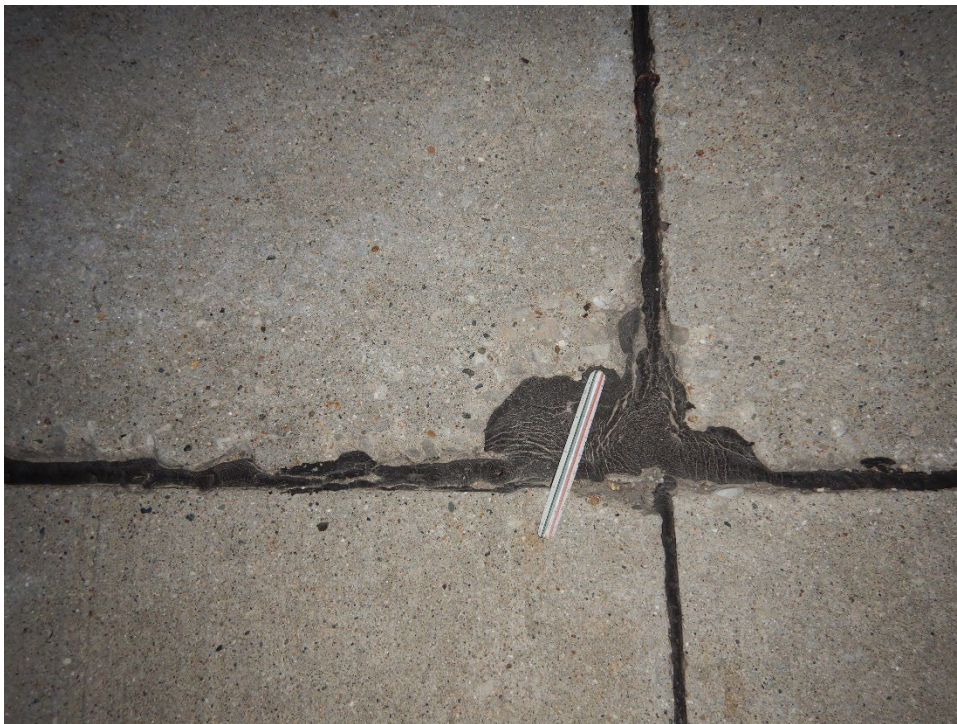
T08NE-01. Corner Spalling (Sample Unit No. 01).
