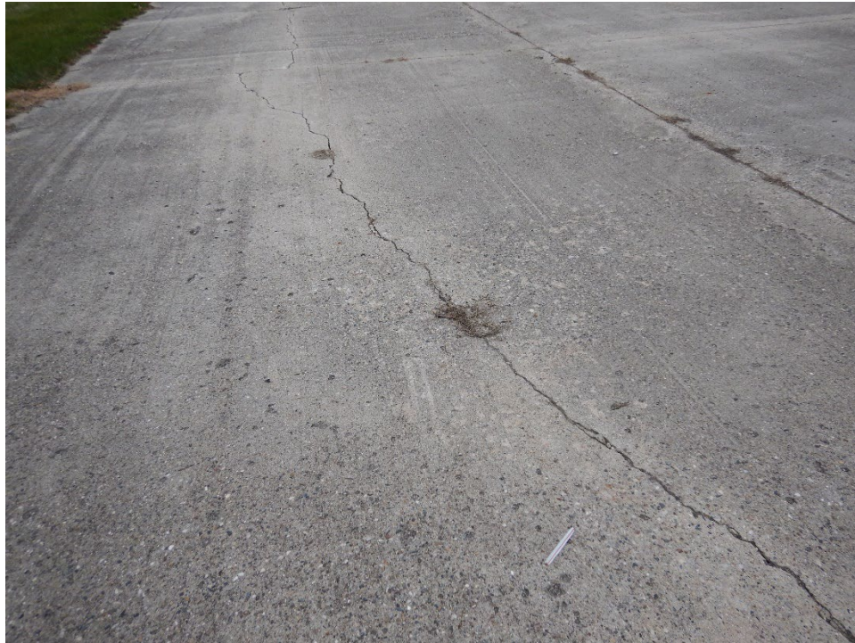
T04NE-01. LTD Cracking (Sample Unit No. 01).
