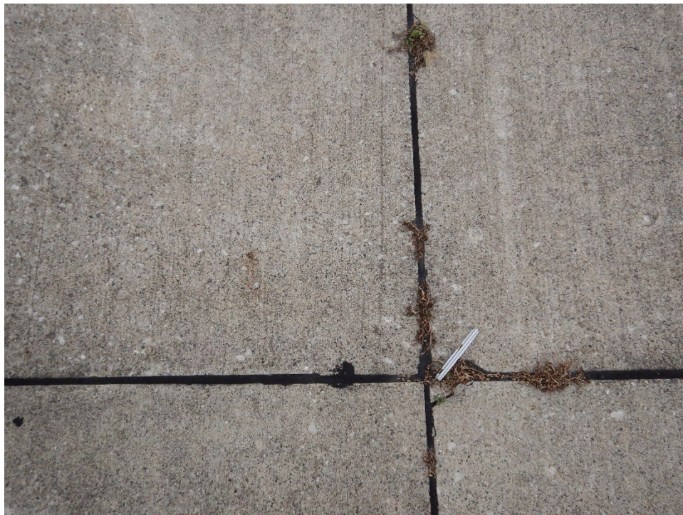
TH01NE-01. Joint Seal Damage (Sample Unit No. 02).
