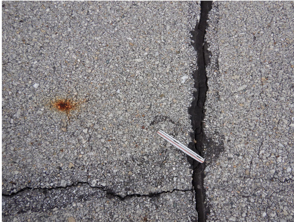
R14NE-01. L&T Cracking (Sample Unit No. 01).
