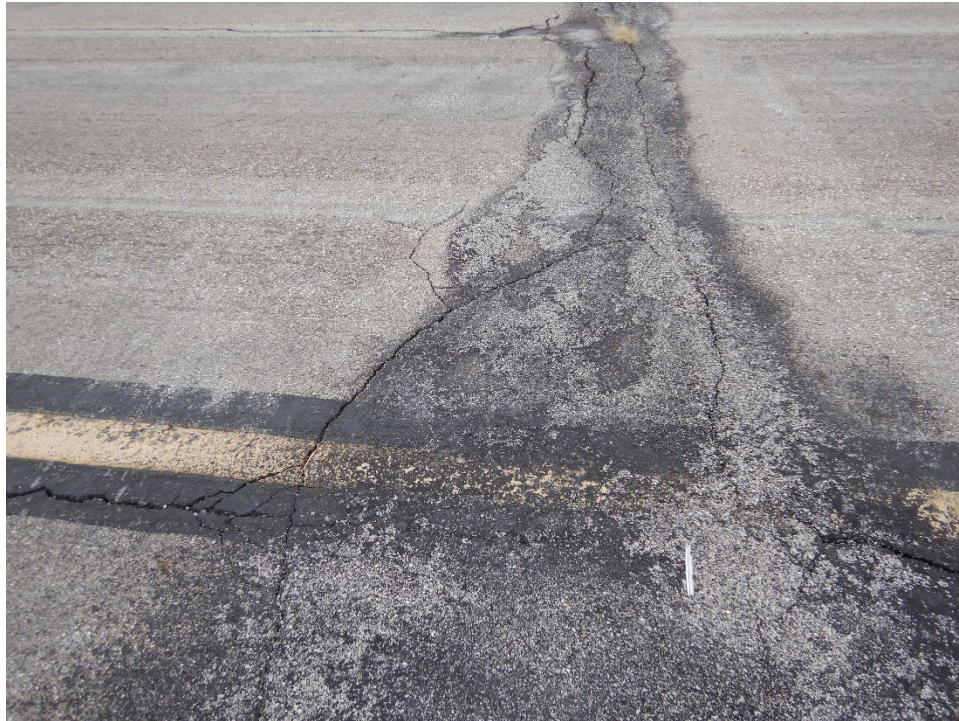
T01NE-01. Patching (Sample Unit No. 08).
