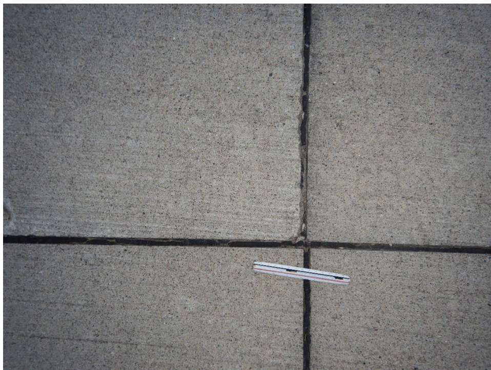
A03NE-02. Joint Seal Damage (Sample Unit No. 10).
