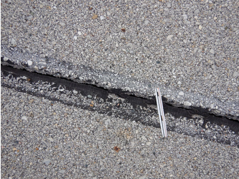
R14NE-02. L&T Cracking (Sample Unit No. 14) (1).
