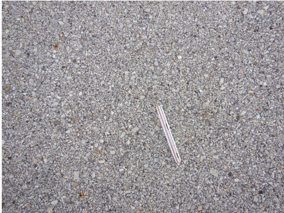
R14NE-01. Weathering (Sample Unit No. 01).
