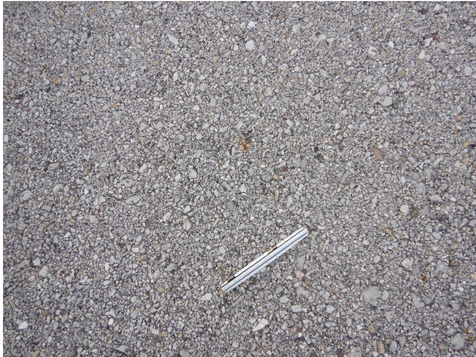
T05NE-01. Weathering (Sample Unit No. 20).
