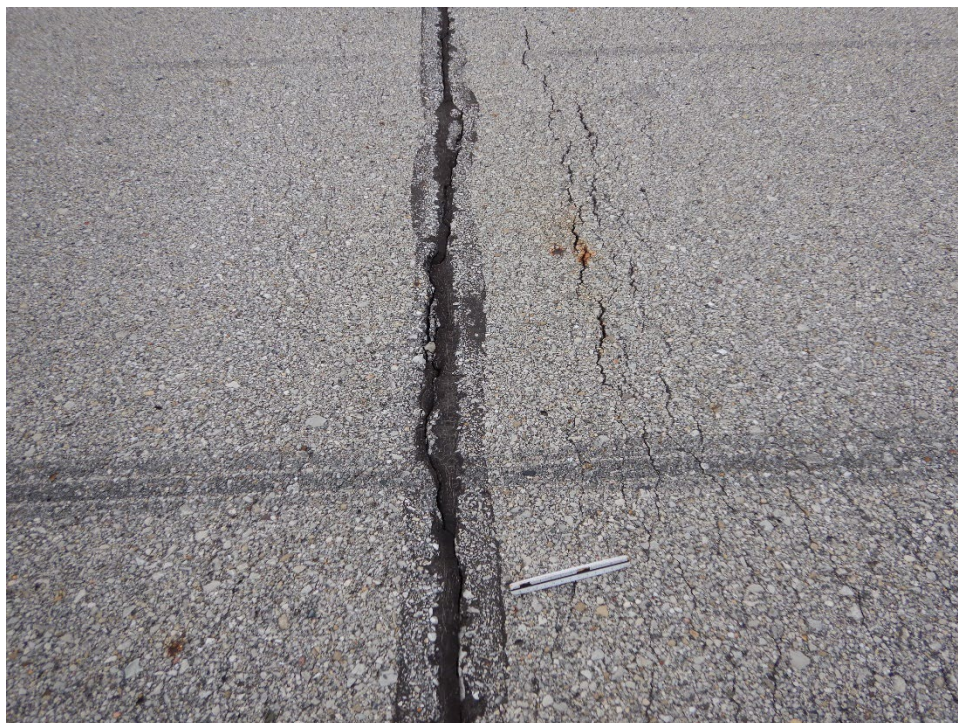
R14NE-01. L&T Cracking (Sample Unit No. 08).
