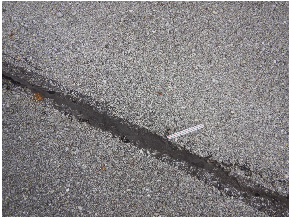
T06NE-01. L&T Cracking (Sample Unit No. 02).
