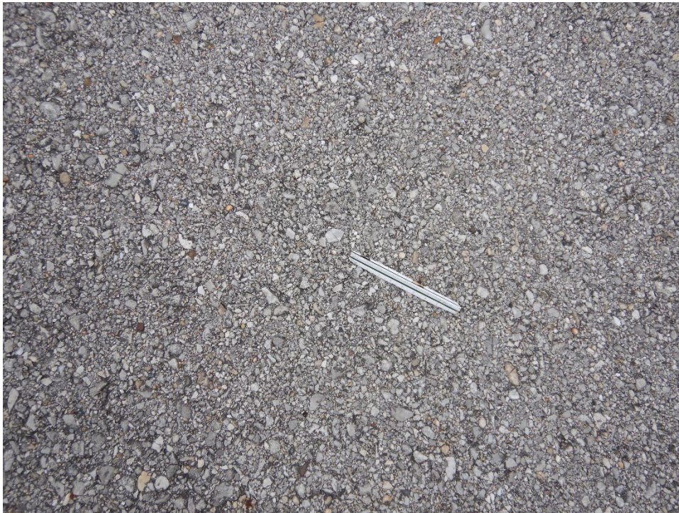
T02NE-02. Weathering (Sample Unit No. 01).
