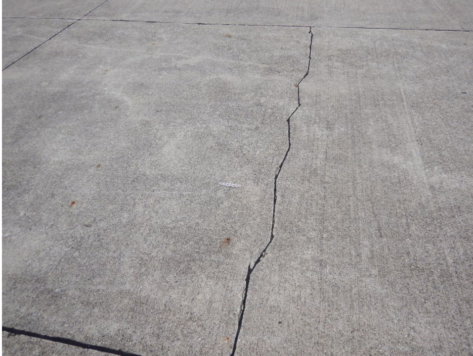
TH01NE-01. LTD Cracking (Sample Unit No. 02).
