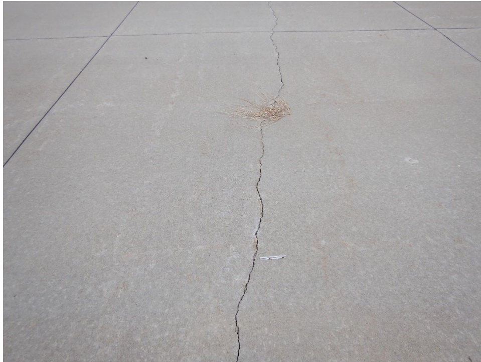
TH02NE-01. LTD Cracking (Sample Unit No. 01).
