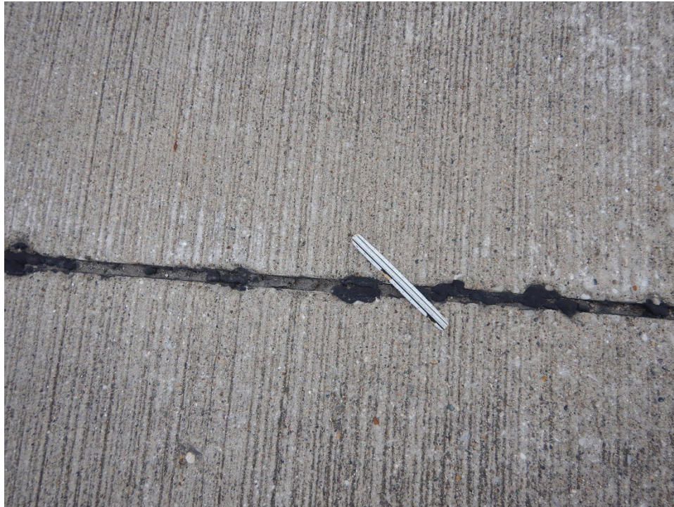
A01NE-01. Joint Seal Damage (Sample Unit No. 17).
