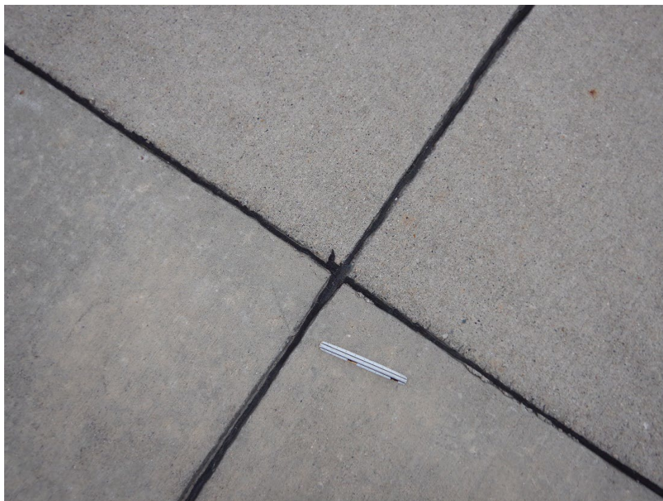
A03NE-03. Joint Seal Damage (Sample Unit No. 10).
