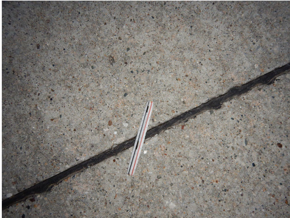
A03NE-01. Joint Seal Damage (Sample Unit No. 15).
