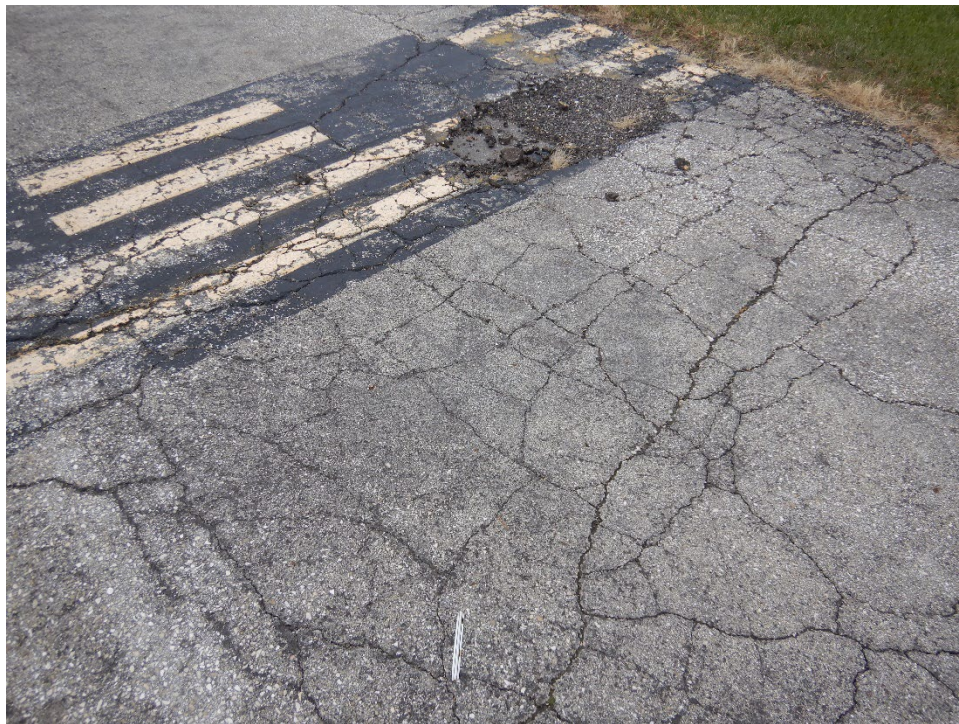
T01NE-01. Alligator Cracking (Sample Unit No. 08).
