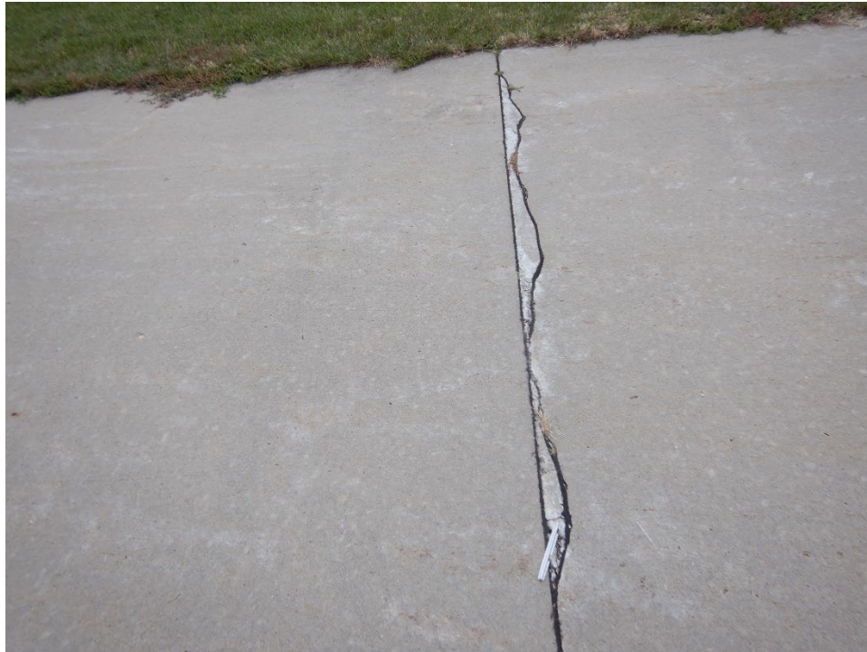
TH03NE-01 Joint Spalling (Sample Unit No. 09).
