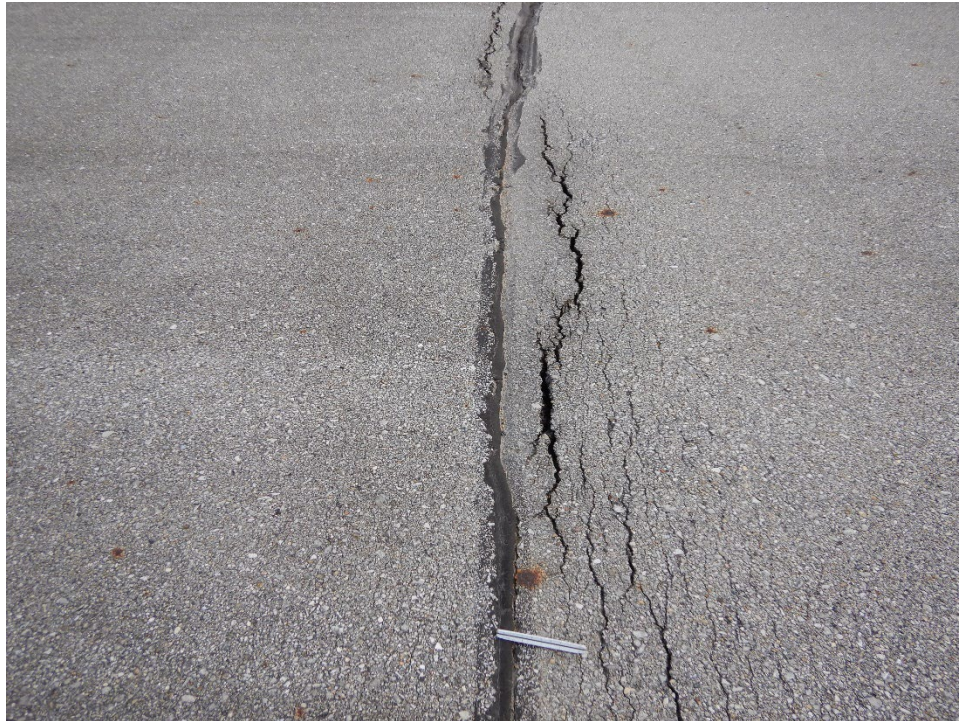
T07NE-01. L&T Cracking (Sample Unit No. 02) (2).
