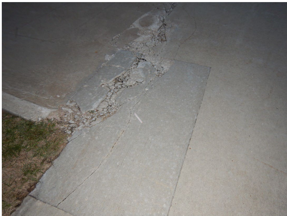
A03NE-01. Large Patching (Additional Sample Unit No. 16).
