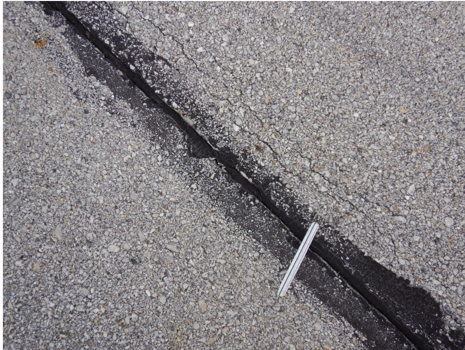
R14NE-03. L&T Cracking (Sample Unit No. 11).
