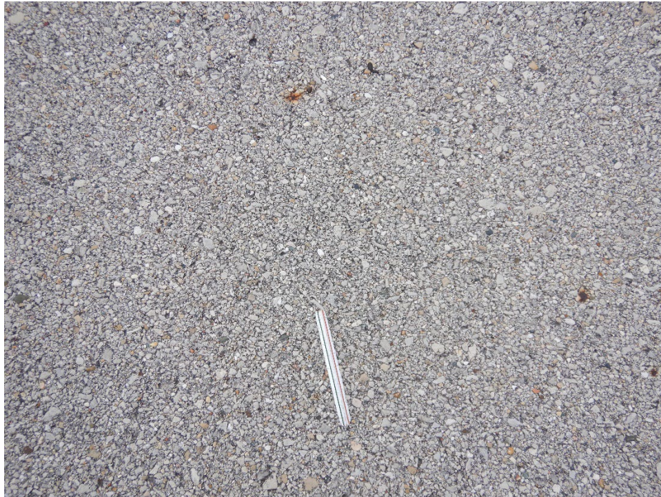
R14NE-02. Weathering (Sample Unit No. 14).
