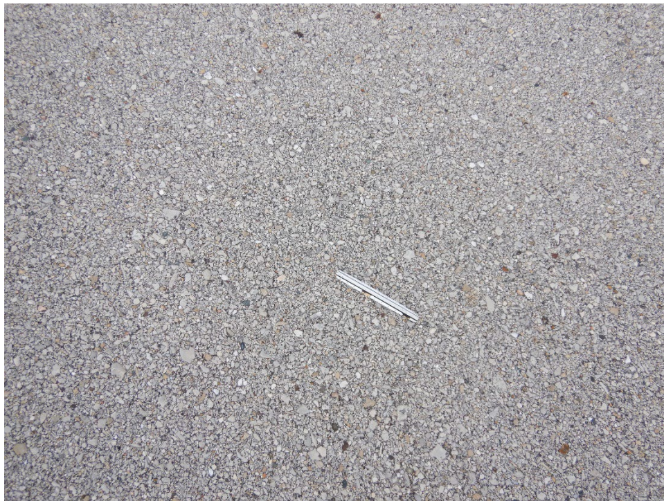
R14NE-03. Weathering (Sample Unit No. 11).
