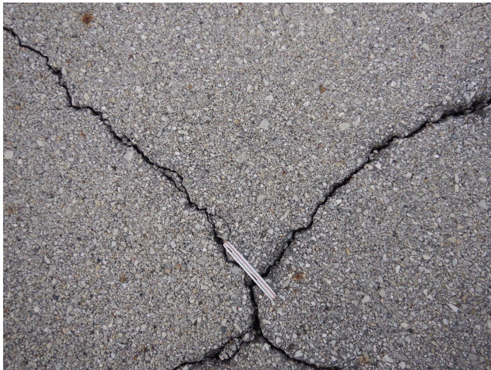
T03NE-01. L&T Cracking (Sample Unit No. 06).
