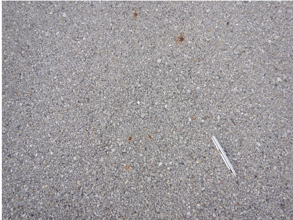
T03NE-01. Weathering (Sample Unit No. 06).
