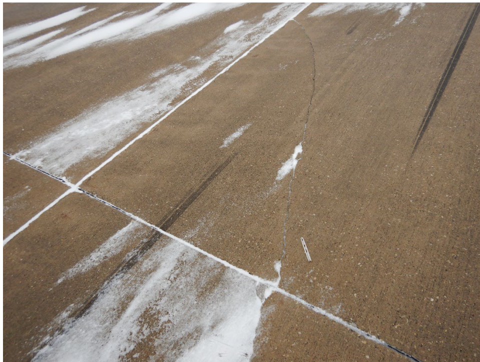
R12CC-01. LTD Cracking (Sample Unit No. 20).
