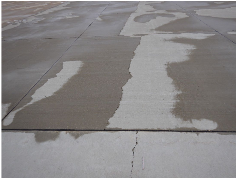
A04CC-01. LTD Cracking (Sample Unit No. 02).
