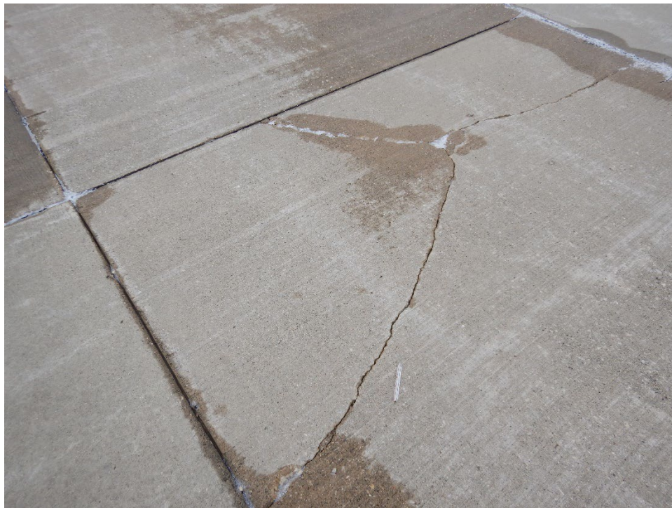
A01CC-01. LTD Cracking (Sample Unit No. 05).
