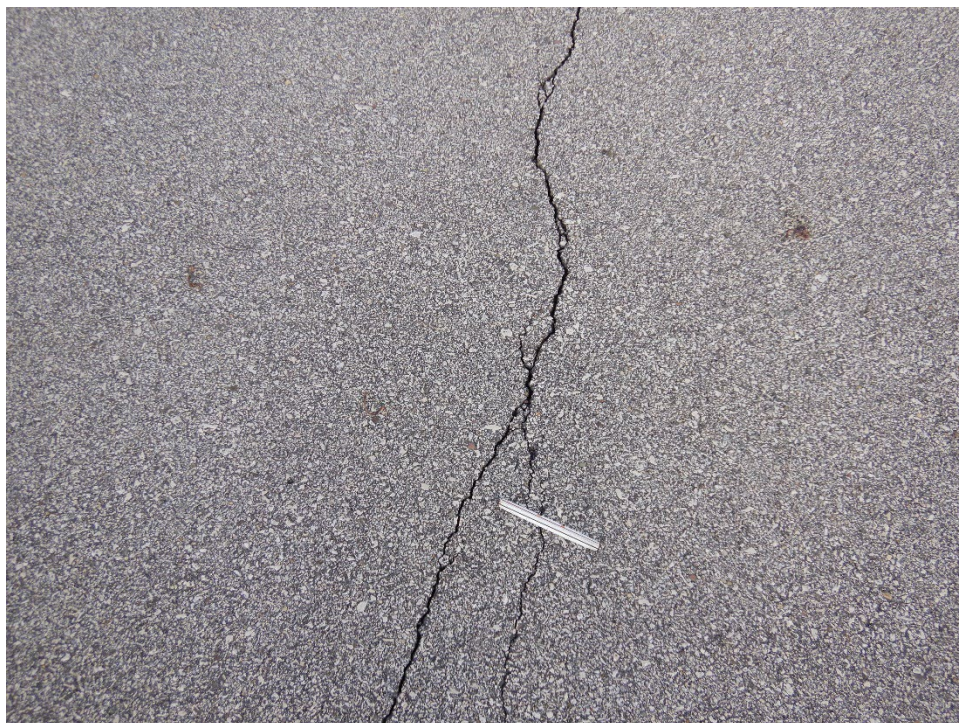
T01OE-02. L&T Cracking (Sample Unit No. 05).
