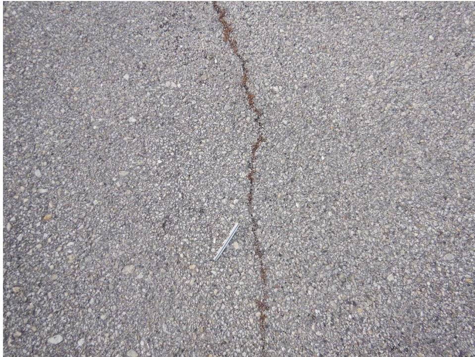
TH01OE-02. L&T Cracking (Sample Unit No. 02).
