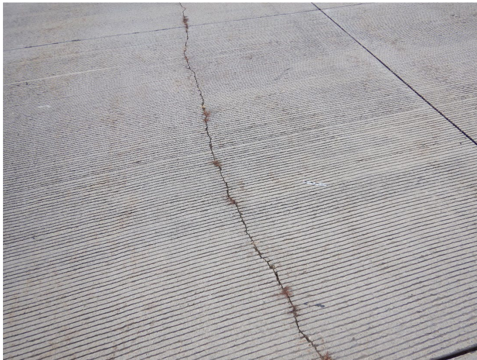
A01OE-01. LTD Cracking (Sample Unit No. 03).
