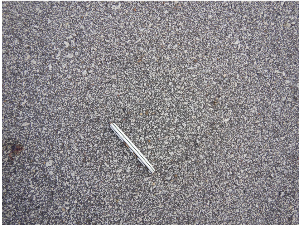
T01OE-02. Weathering (Sample Unit No. 05).
