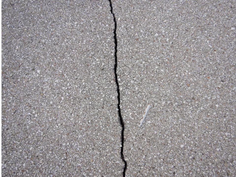
TH01OE-01. L&T Cracking (Sample Unit No. 02).
