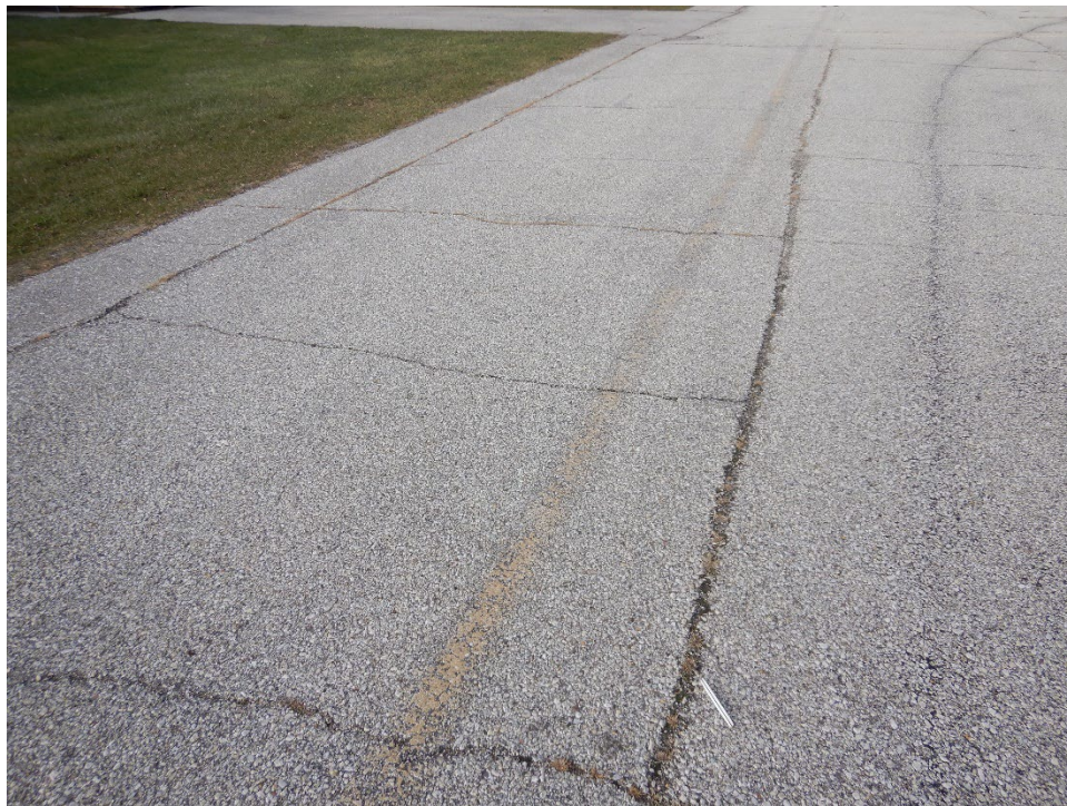
TH01OE-03. Block Cracking (Sample Unit No. 01).
