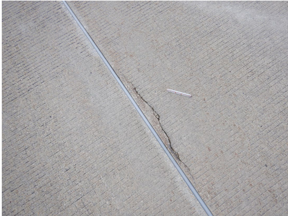
T01OE-01. Joint Spalling (Sample Unit No. 07).
