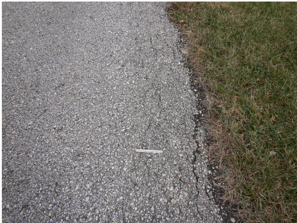
TH01OE-02. Alligator Cracking (Sample Unit No. 02).
