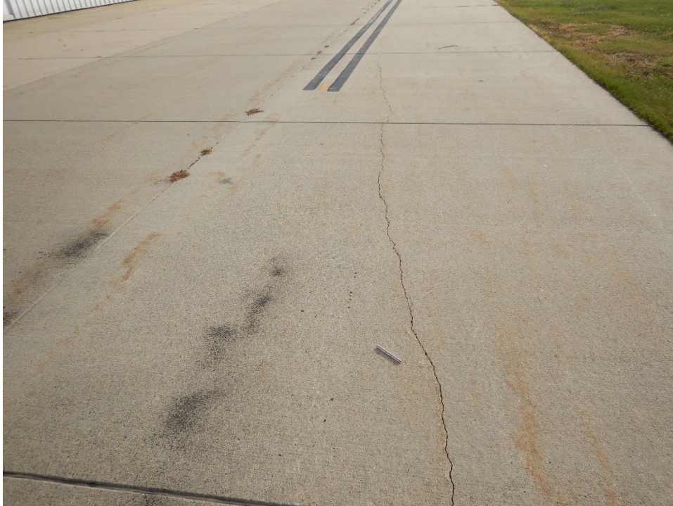
TH01OE-04. LTD Cracking (Sample Unit No. 01).
