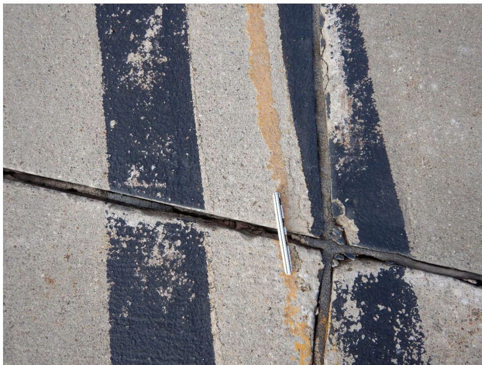
TH01OE-04. Joint Seal Damage (Sample Unit No. 01).
