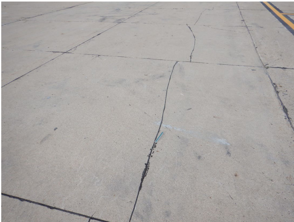
A010A-01. LTD Cracking (Sample Unit No. 01).
