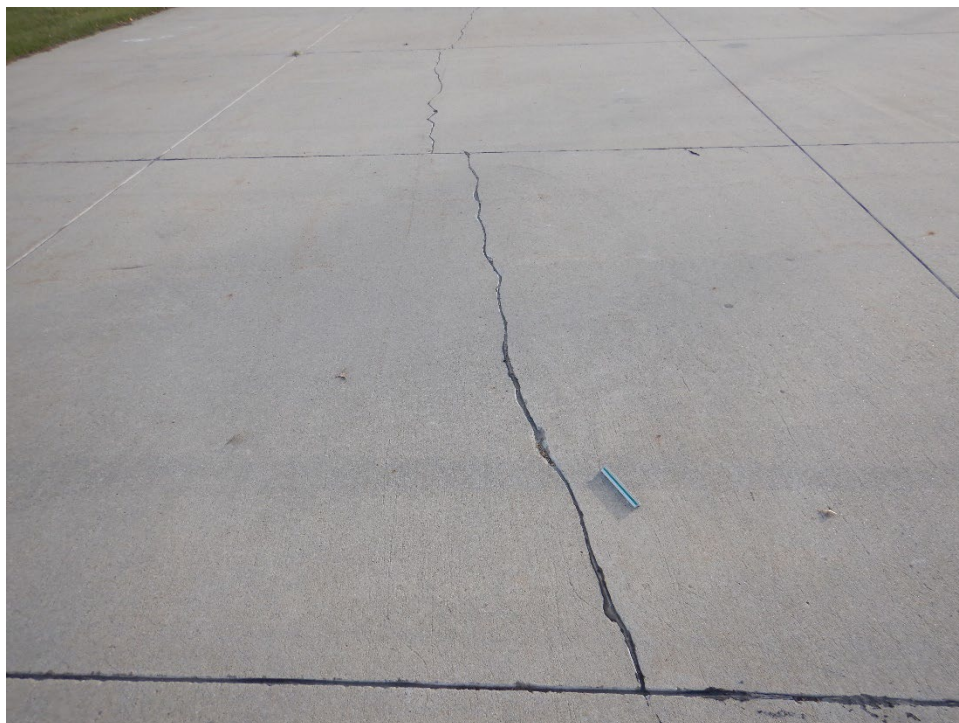
A010A-02. LTD Cracking (Sample Unit No. 06).
