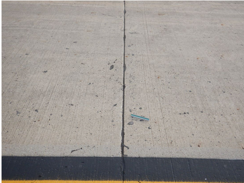
T01OA-01. Joint Seal Damage (Sample Unit No. 04).
