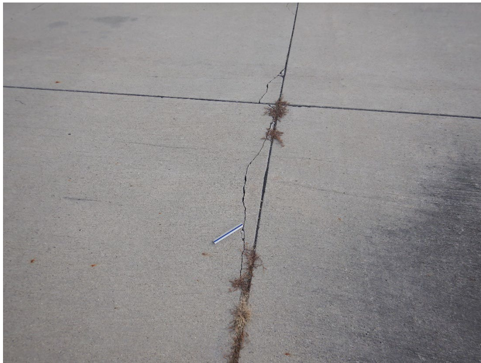
TH01OA-02. Joint Spalling (Additional Sample Unit No. 07).
