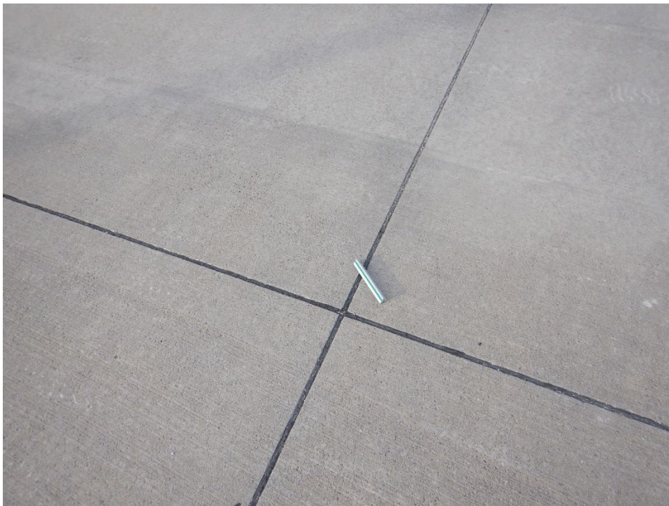
TH02OA-02. Joint Seal Damage (Sample Unit No. 01).
