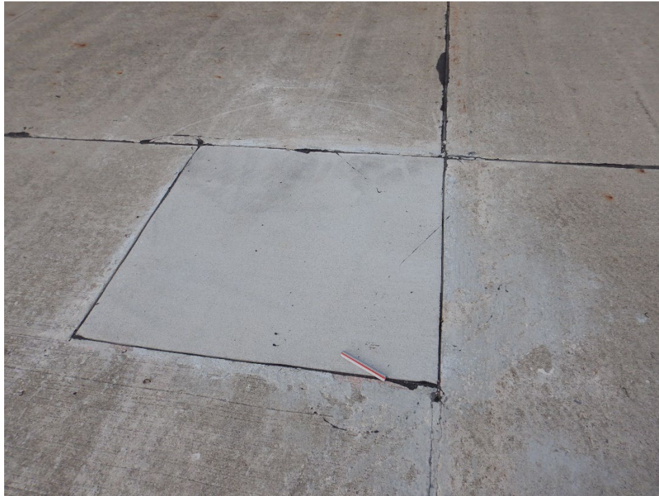
R180A-01. Large Patching (Sample Unit No. 50).
