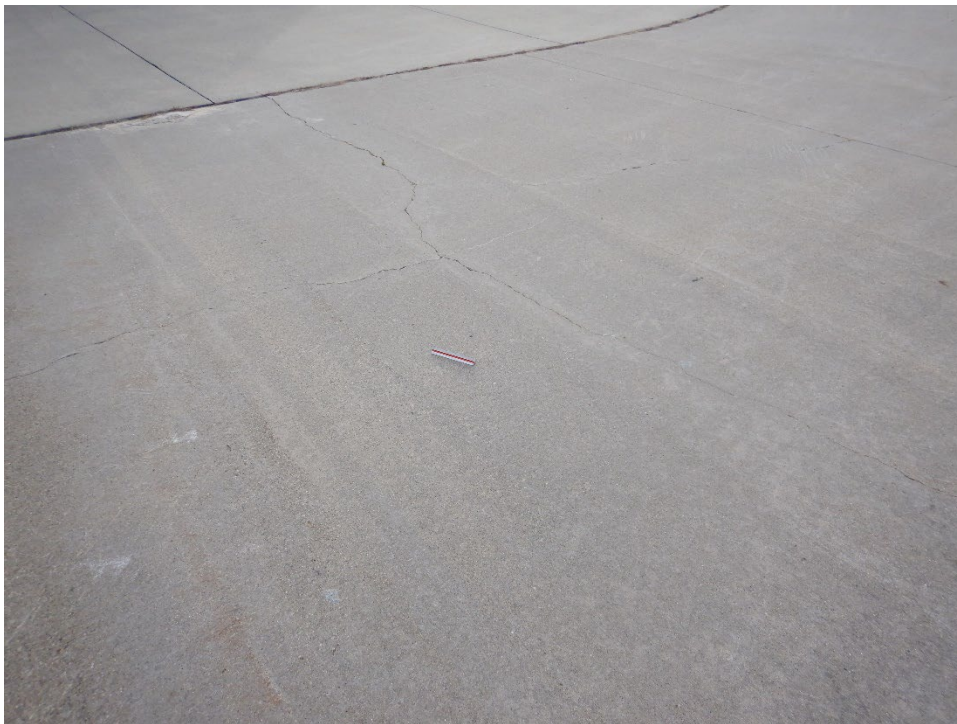
TH02OA-01. Shattered Slab (Sample Unit No. 01).
