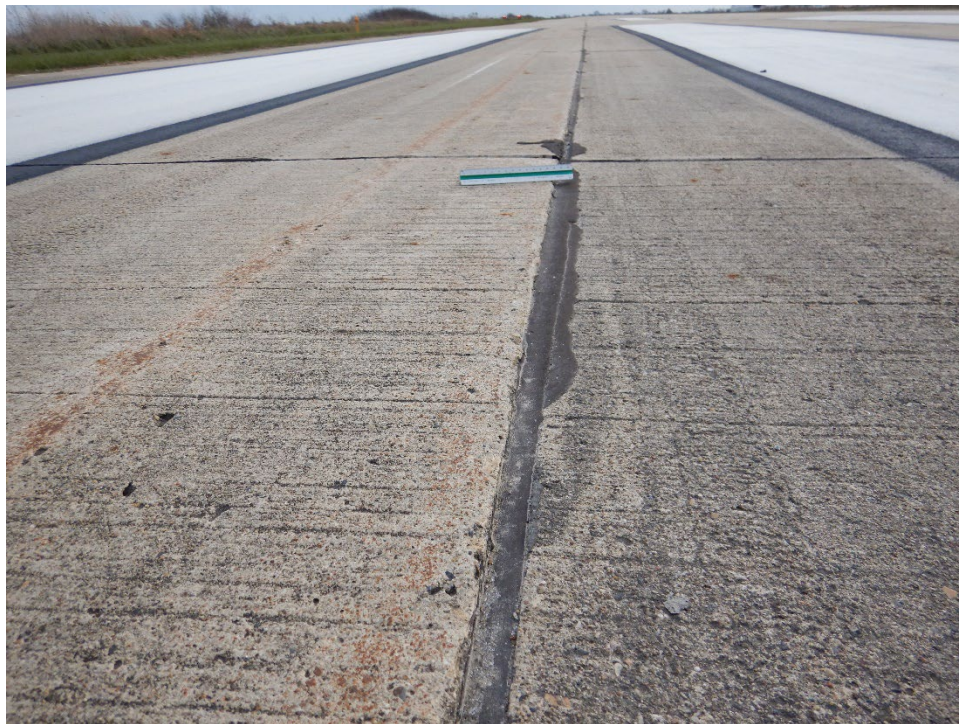
R18OA-01. Faulting (Sample Unit No. 05).
