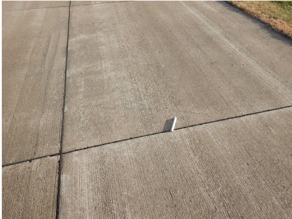
T02OK-01. Corner Break (Sample Unit No. 04).
