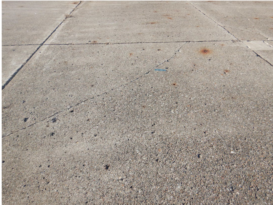
T01OK-01. LTD Cracking (Sample Unit No. 02).
