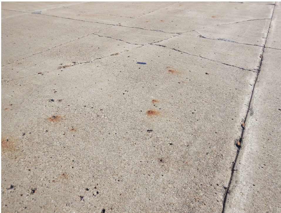
TH01OK-01. Shattered Slab (Sample Unit No. 01).
