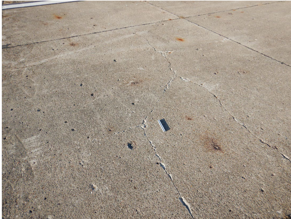
R04OK-01. Shattered Slab (Sample Unit No. 03).
