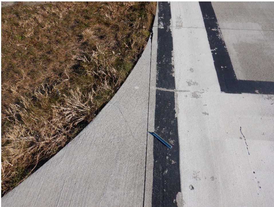
T01OK-02. Corner Break (Sample Unit No. 01).
