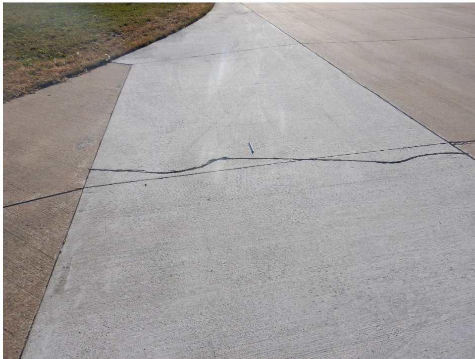
T01OK-02. LTD Cracking (Sample Unit No. 01).
