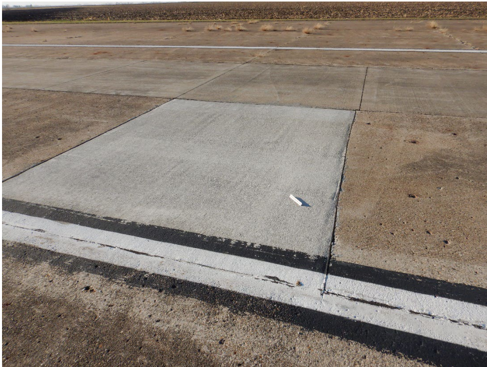
R04OK-01. Large Patching (Sample Unit No. 16).
