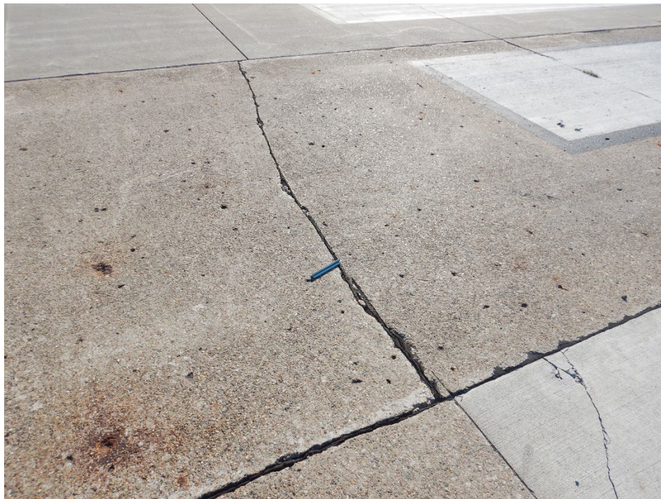
T04OK-01. LTD Cracking (Sample Unit No. 01).
