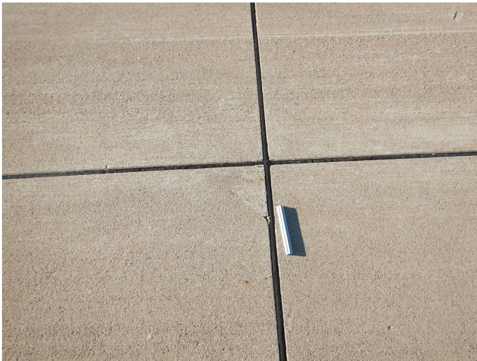
T05OK-01. Corner Spalling (Sample Unit No. 06).
