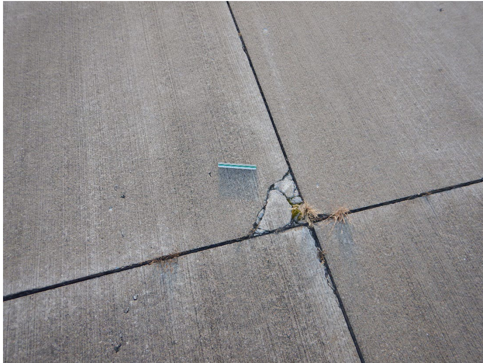
T03OK-01. Corner Spalling (Sample Unit No. 05).
