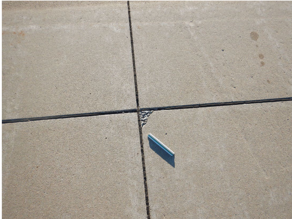
T05OK-03. Corner Spalling (Sample Unit No. 07).
