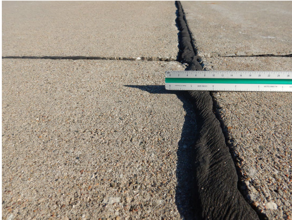
T01OK-02. Faulting (Sample Unit No. 04).
