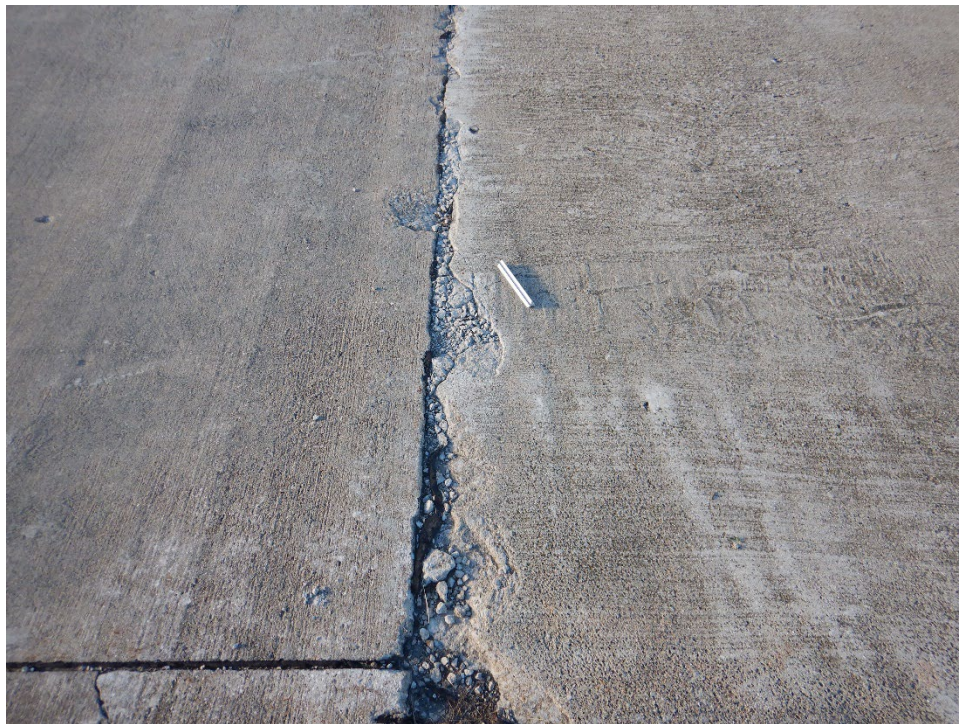
T05OK-03. Joint Spalling (Additional Sample Unit No. 01).
