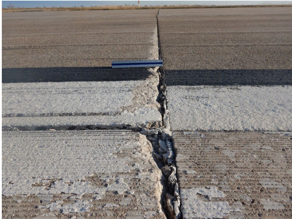
R13OK-01. Faulting (Additional Sample Unit No. 66).
