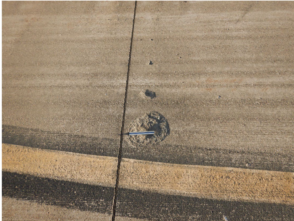
R13OK-01. Small Patching (Sample Unit No. 24).
