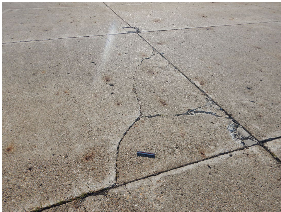
T01OK-01. Shattered Slab (Sample Unit No. 14).
