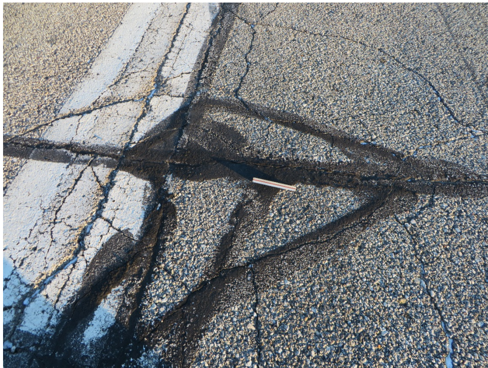
R171Y-03. Alligator Cracking (Sample Unit No. 04).
