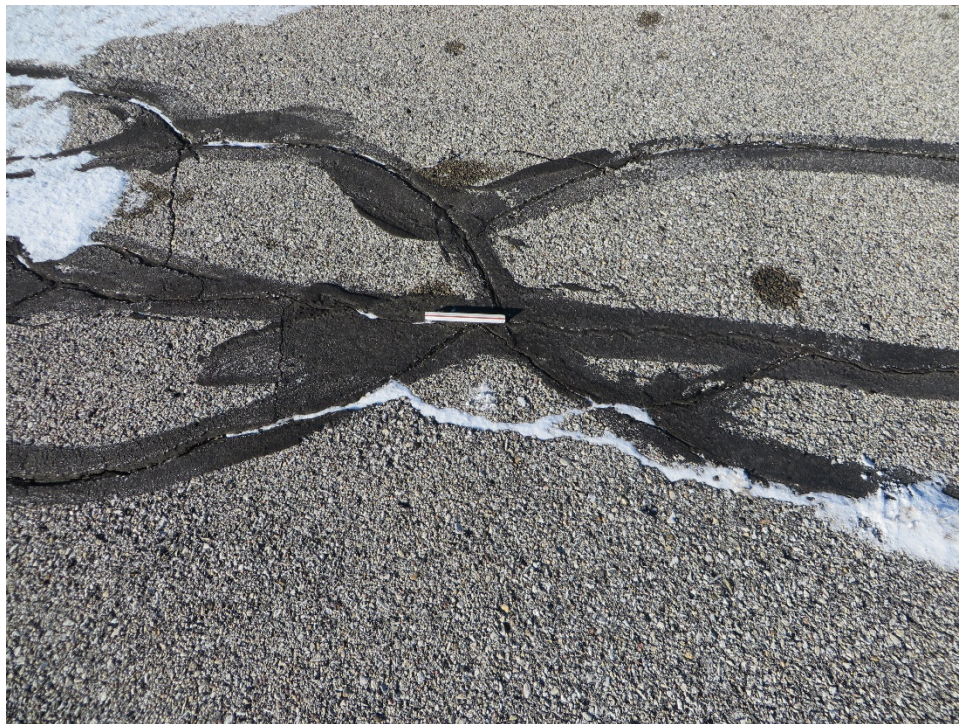
T011Y-03. Alligator Cracking (Sample Unit No. 01).
