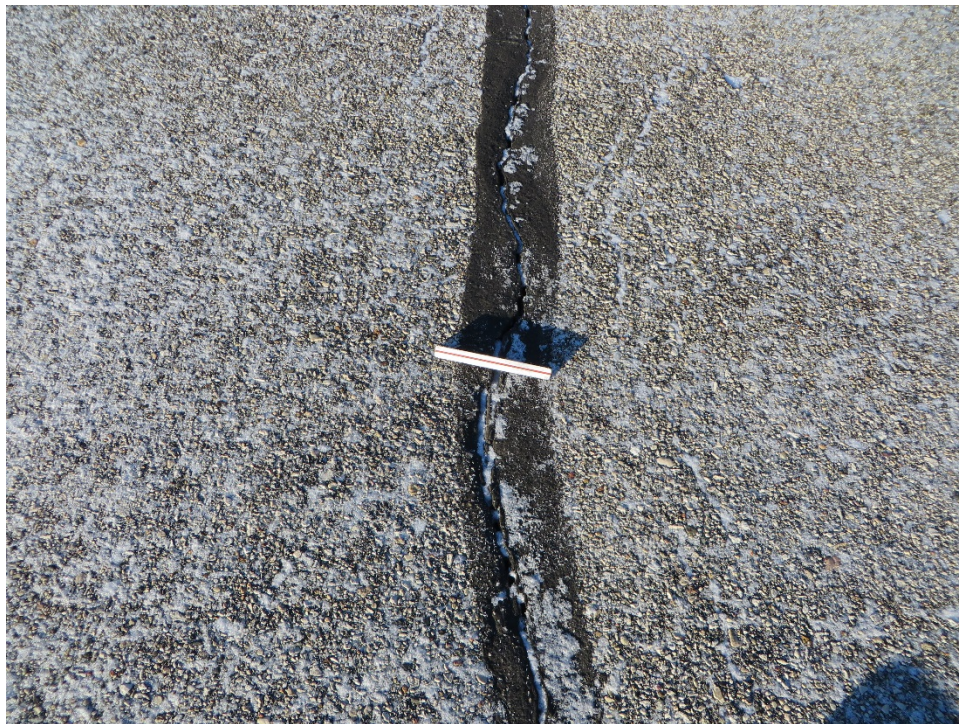
R171Y-02. L&T Cracking (Sample Unit No. 08).
