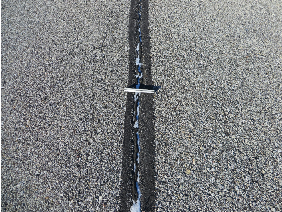
T011Y-02. L&T Cracking (Sample Unit No. 01).
