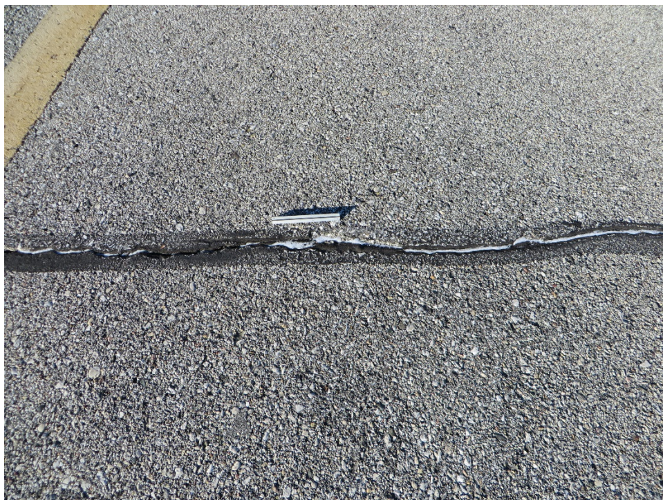
T011Y-01. L&T Cracking (Sample Unit No. 01).
