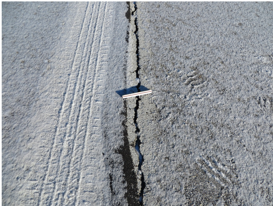
R171Y-01. L&T Cracking (Sample Unit No. 02).
