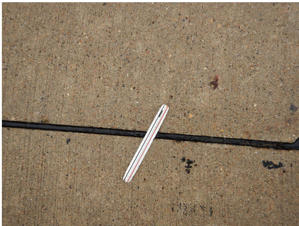
R16PE-08. Joint Seal Damage (Sample Unit No. 01).
