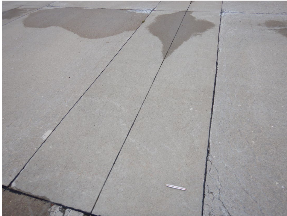
A01PE-01. Large Patching (Sample Unit No. 15).
