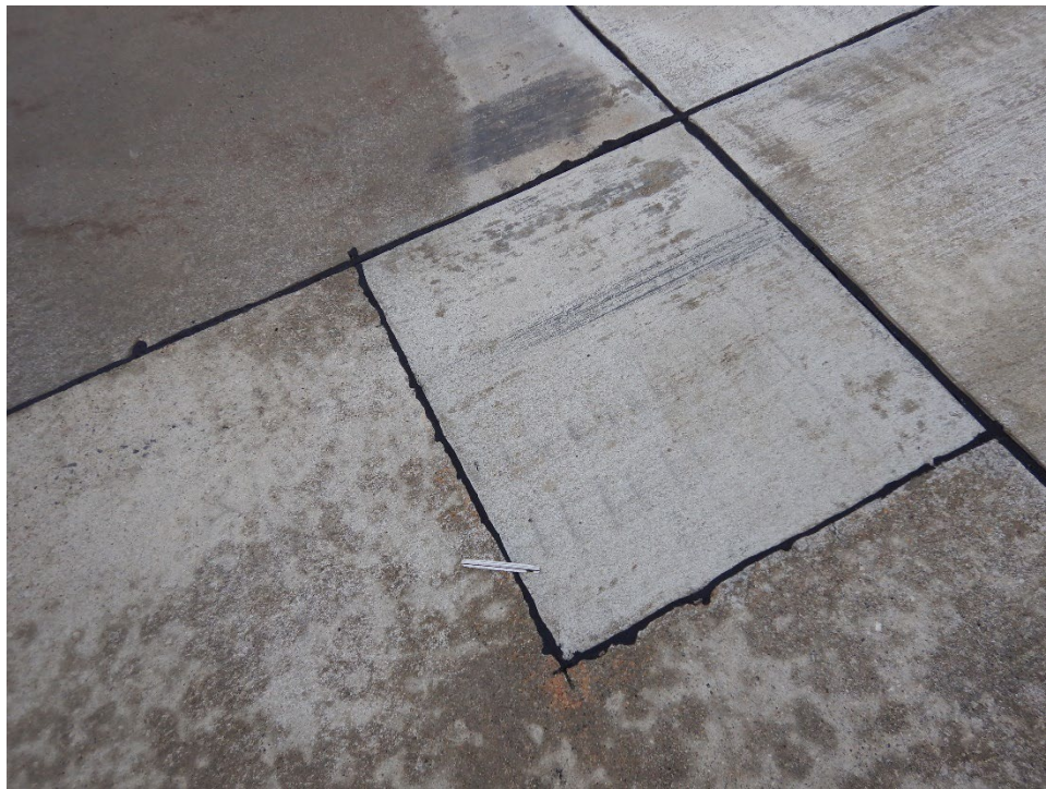
R16PE-10. Large Patching (Sample Unit No. 02).
