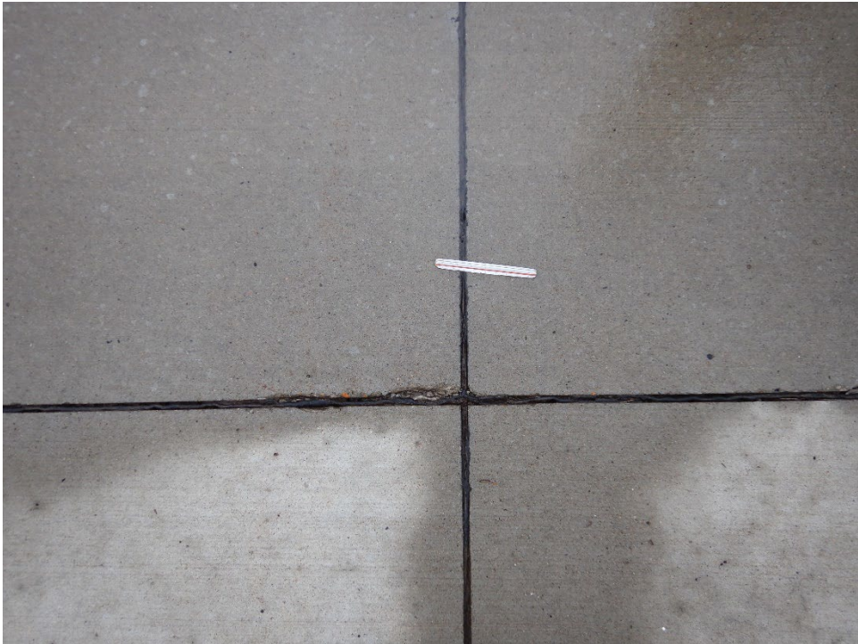
TH01PE-02. Joint Seal Damage (Sample Unit No. 02).
