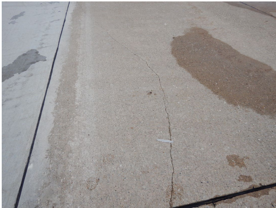
R16PE-03. LTD Cracking (Sample Unit No. 27).
