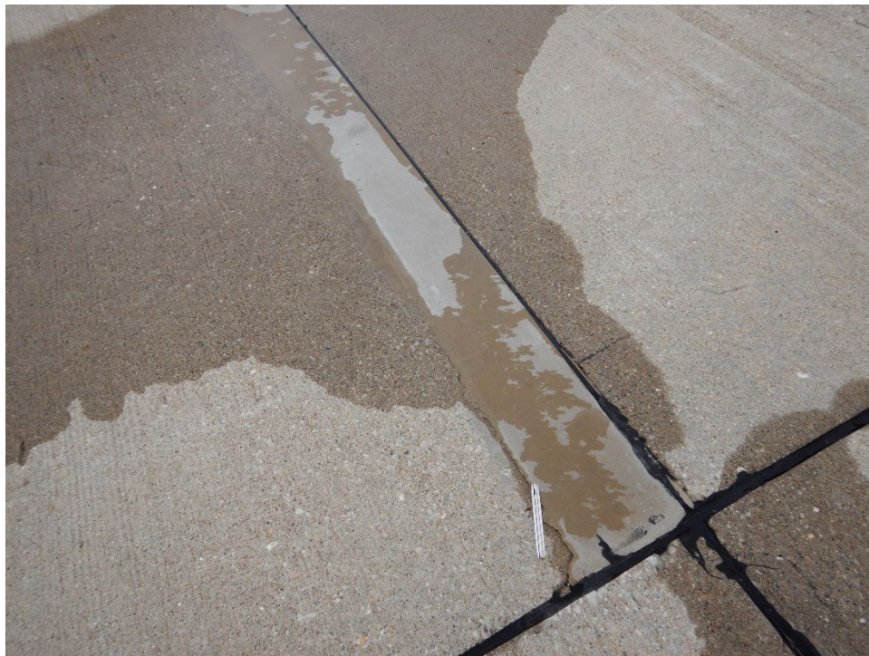
R16PE-05. Large Patching (Sample Unit No. 01).
