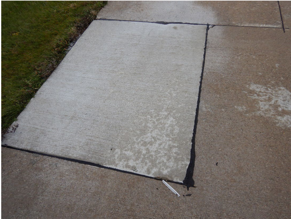
R16PE-07. Large Patching (Sample Unit No. 04).
