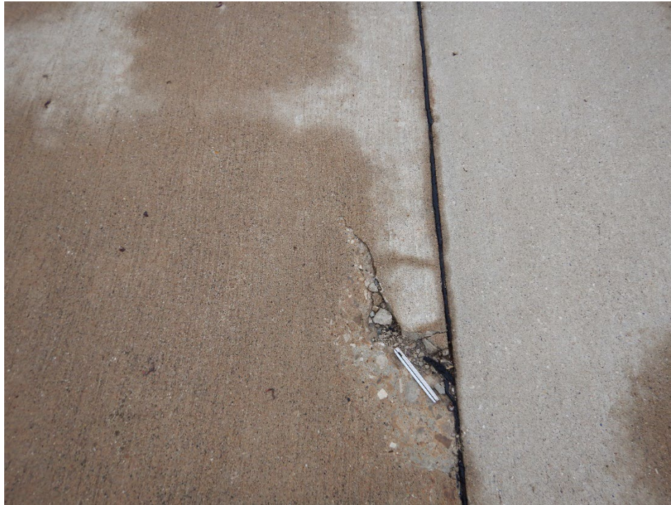
A01PE-04. Joint Spalling (Sample Unit No. 02).
