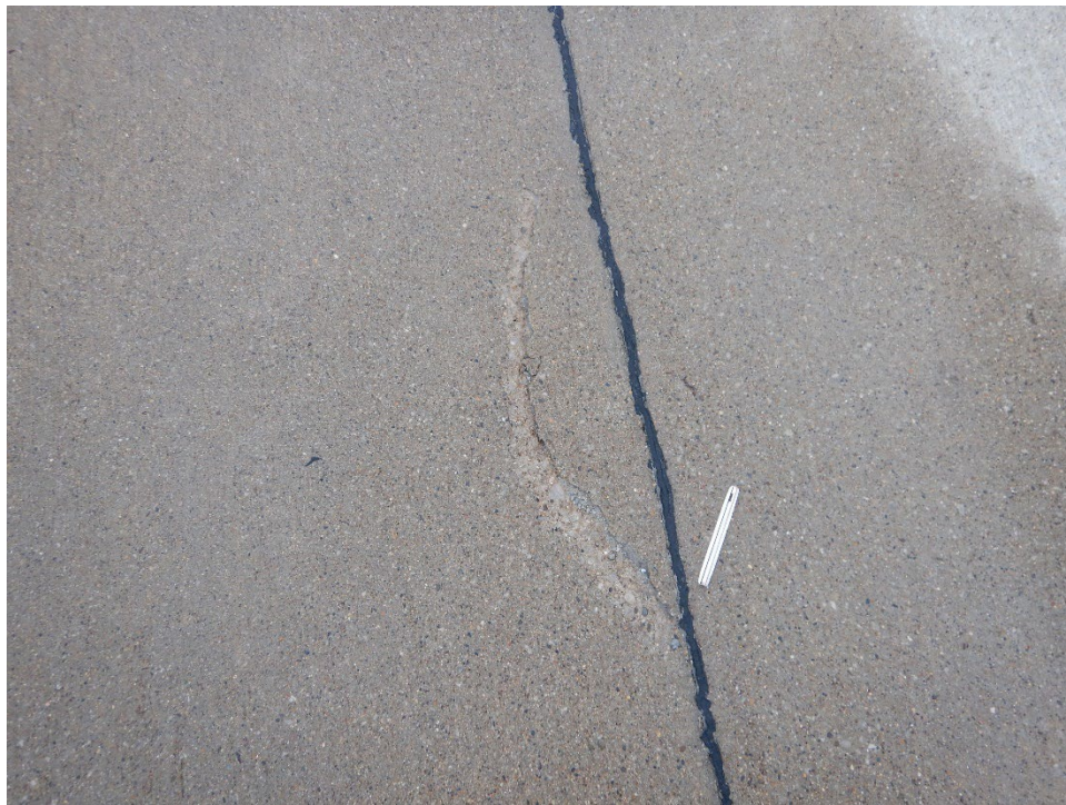
A01PE-03. Joint Spalling (Sample Unit No. 02).
