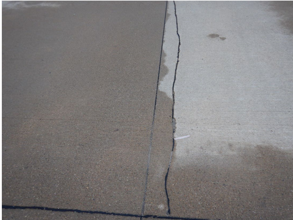
A01PE-03. LTD Cracking (Sample Unit No. 03).
