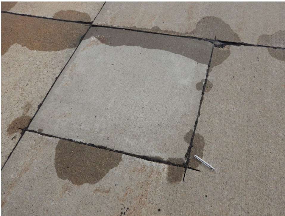
R16PE-06. Large Patching (Sample Unit No. 02).
