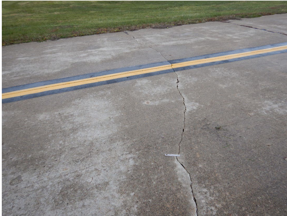
TH01PE-01. LTD Cracking (Sample Unit No. 01).
