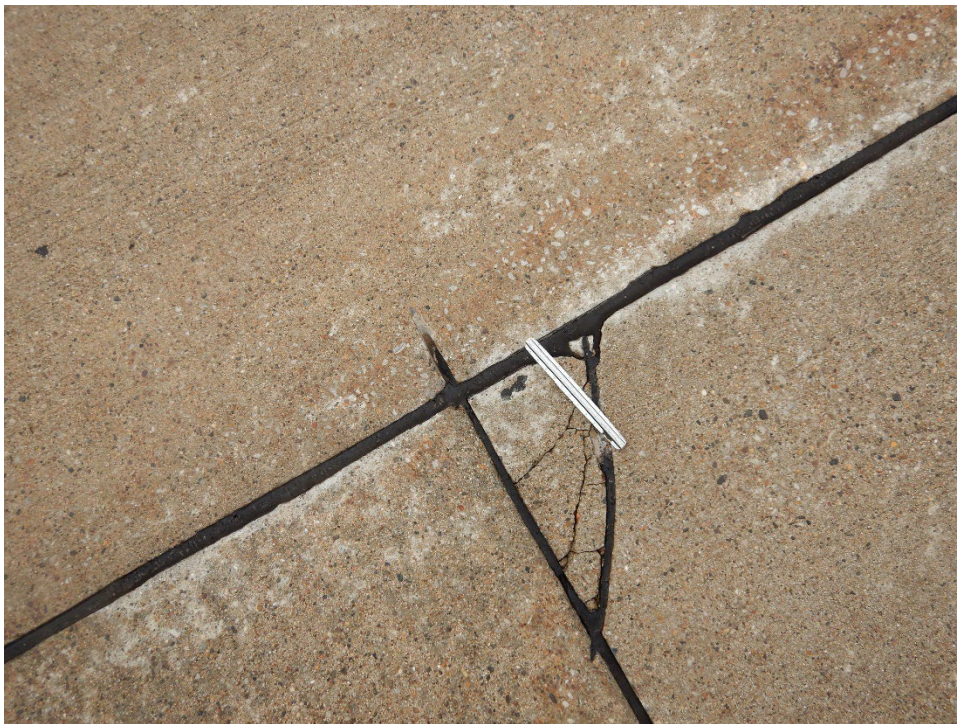
R16PE-07. Corner Spalling (Sample Unit No. 04).
