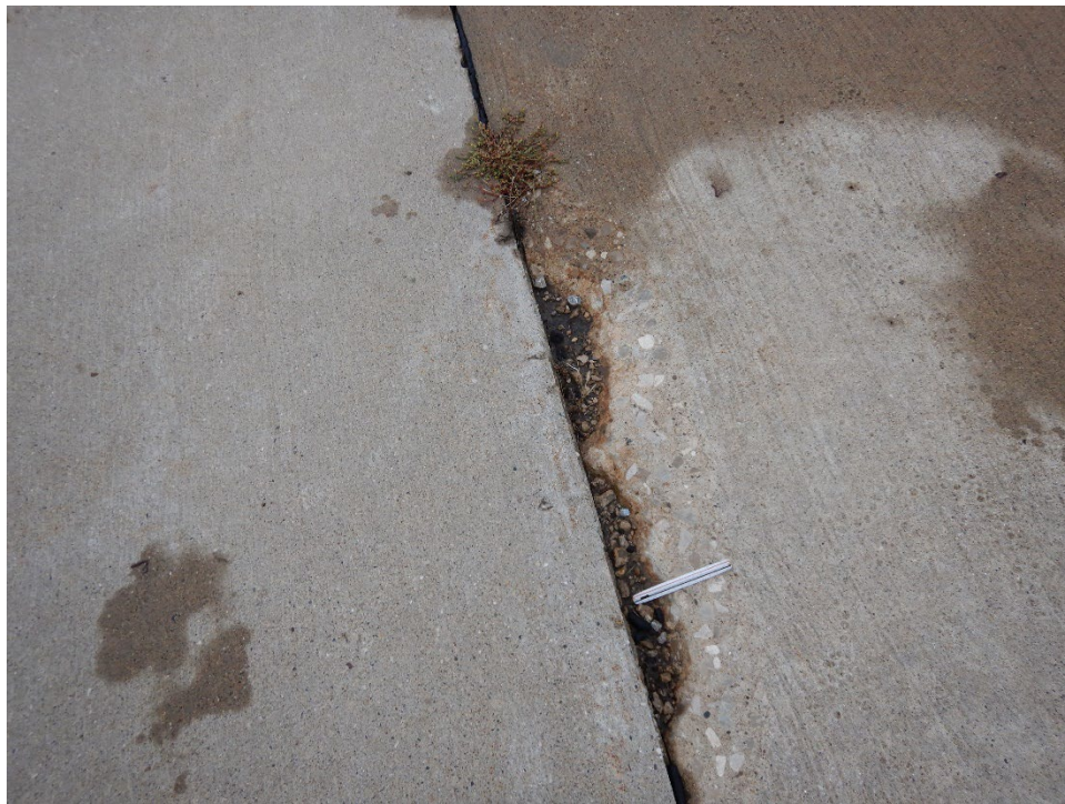
A01PE-04. Joint Spalling (Sample Unit No. 03).
