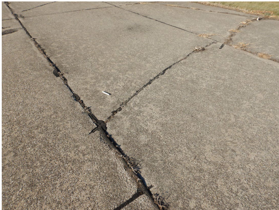
R12PO-04. LTD Cracking (Sample Unit No. 01).
