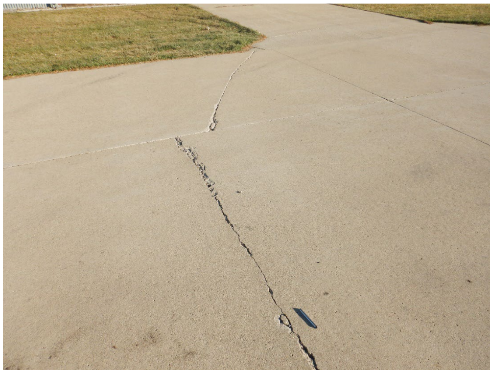
TH01PO-02. LTD Cracking (Sample Unit No. 01).
