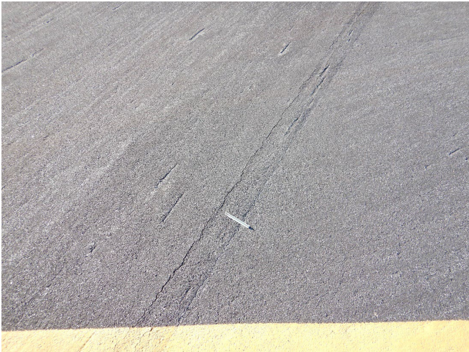
T01PO-03. L&T Cracking (Sample Unit No. 01).
