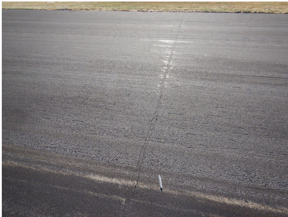
R12PO-01. L&T Cracking (Sample Unit No. 04).
