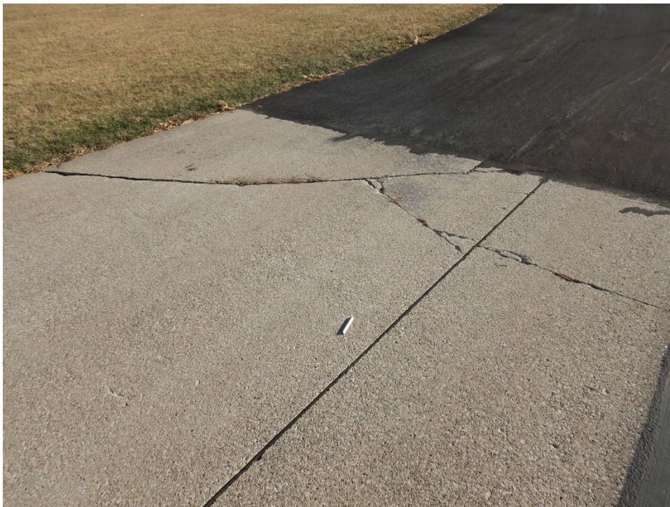
T01PO-01. Shattered Slab (Sample Unit No. 01).
