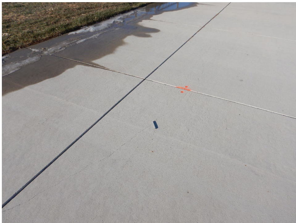
TH01PO-04. LTD Cracking (Sample Unit No. 05).
