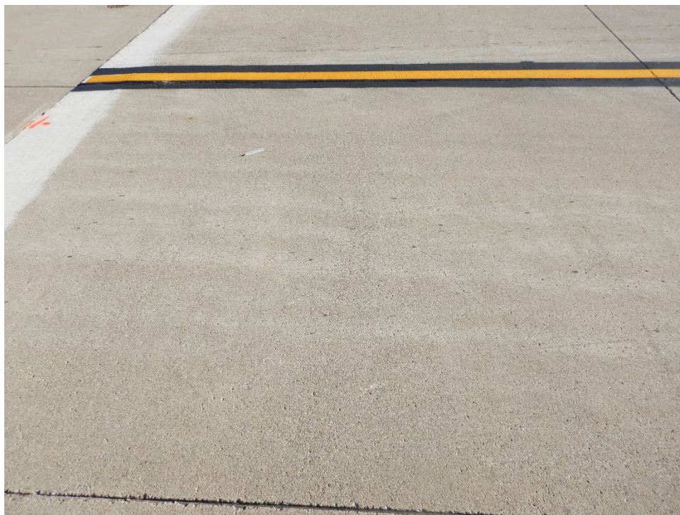
T02PO-02. LTD Cracking (Sample Unit No. 03).
