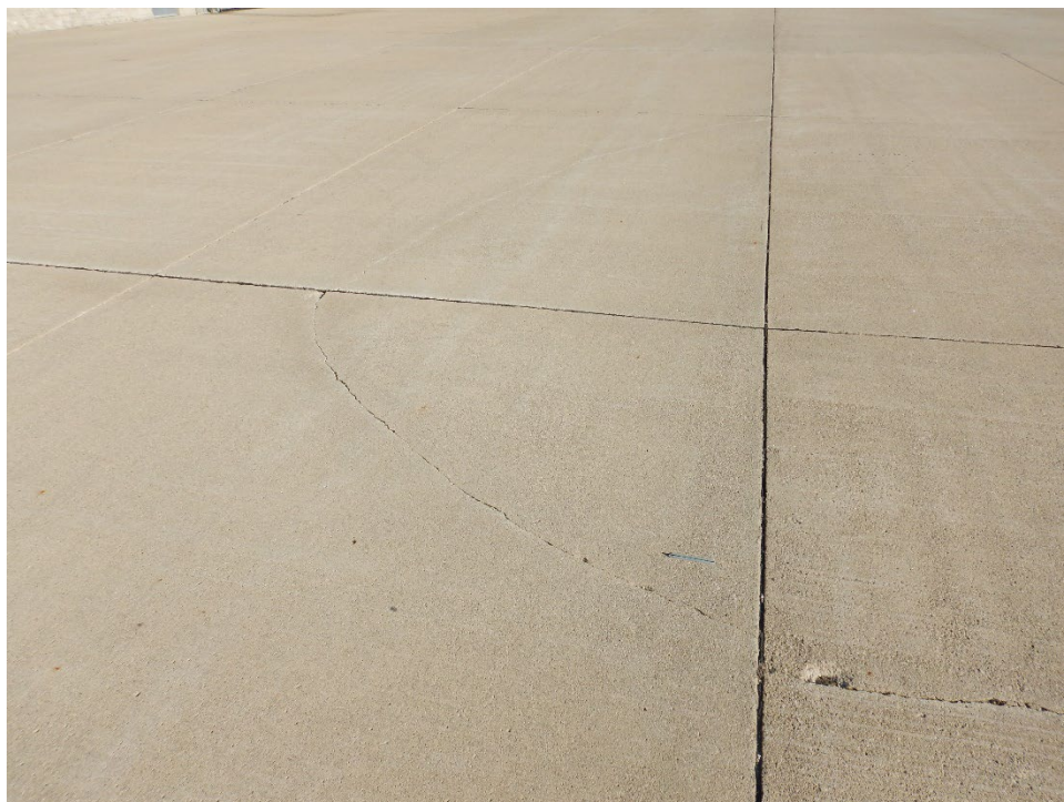
A01PO-01. LTD Cracking (Sample Unit No. 15).
