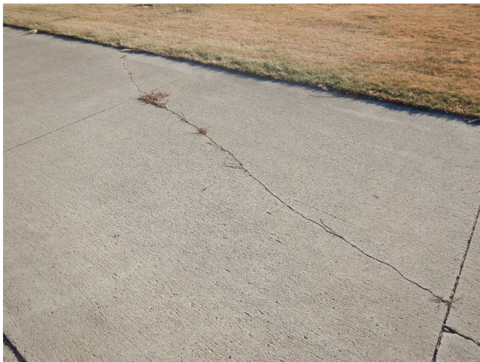
T01PO-02. LTD Cracking (Sample Unit No. 04).
