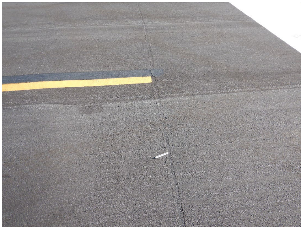
T02PO-03. Joint Reflection Cracking (Sample Unit No. 01).
