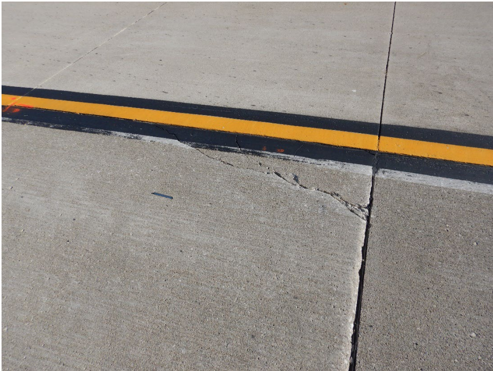
T02PO-01. Joint Spalling (Sample Unit No. 01).
