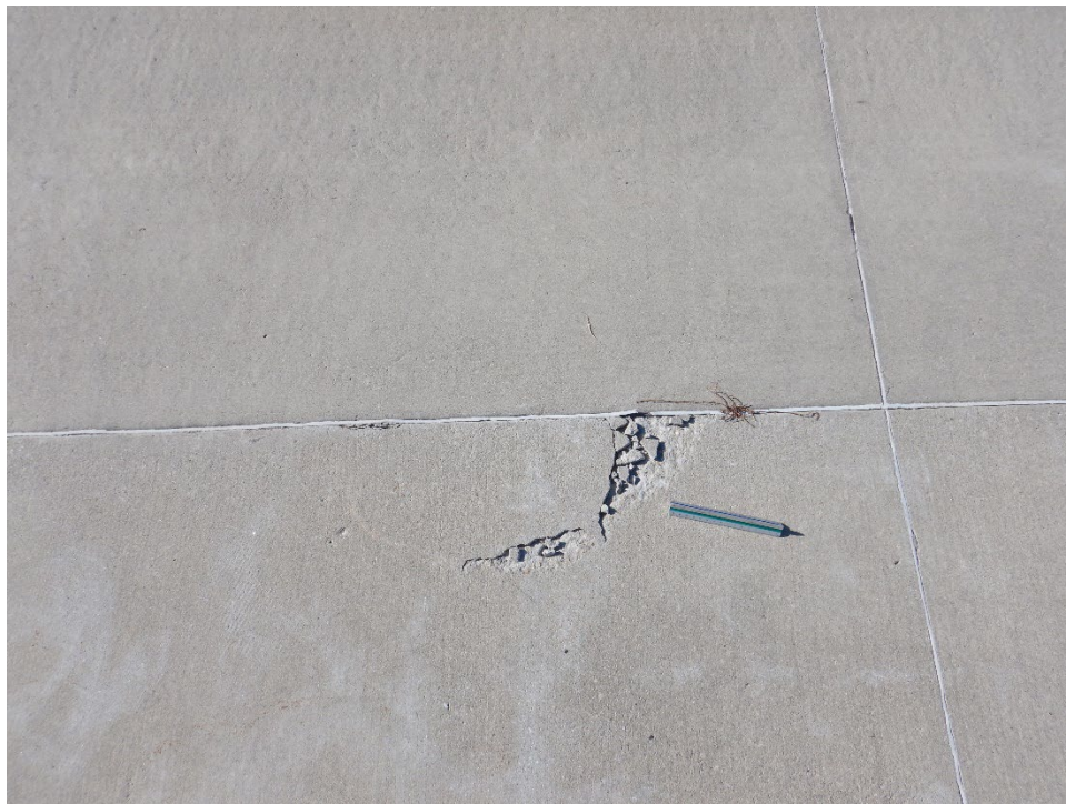
TH01RO-03. Joint Spalling (Sample Unit No. 01).
