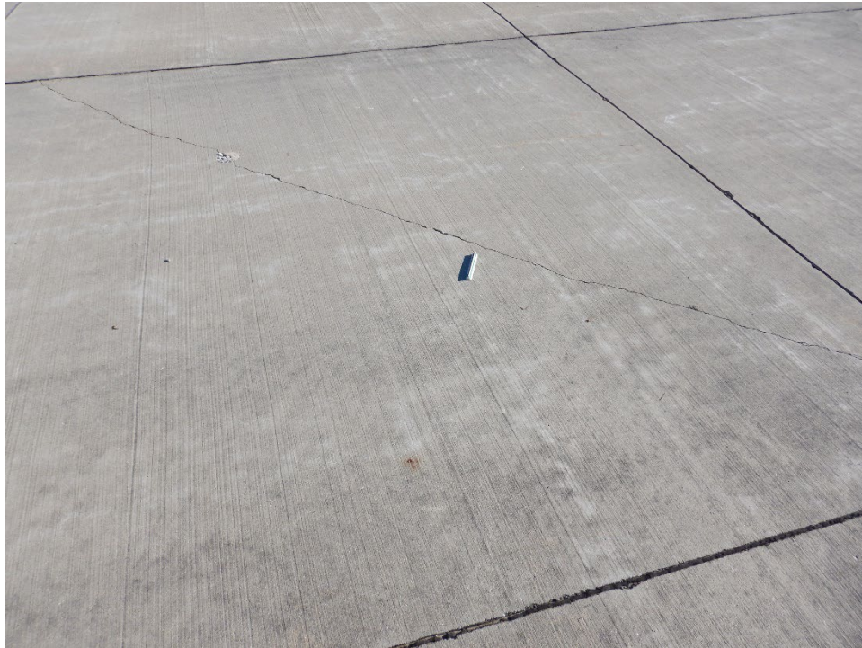
T04RO-01. LTD Cracking (Sample Unit No. 03).
