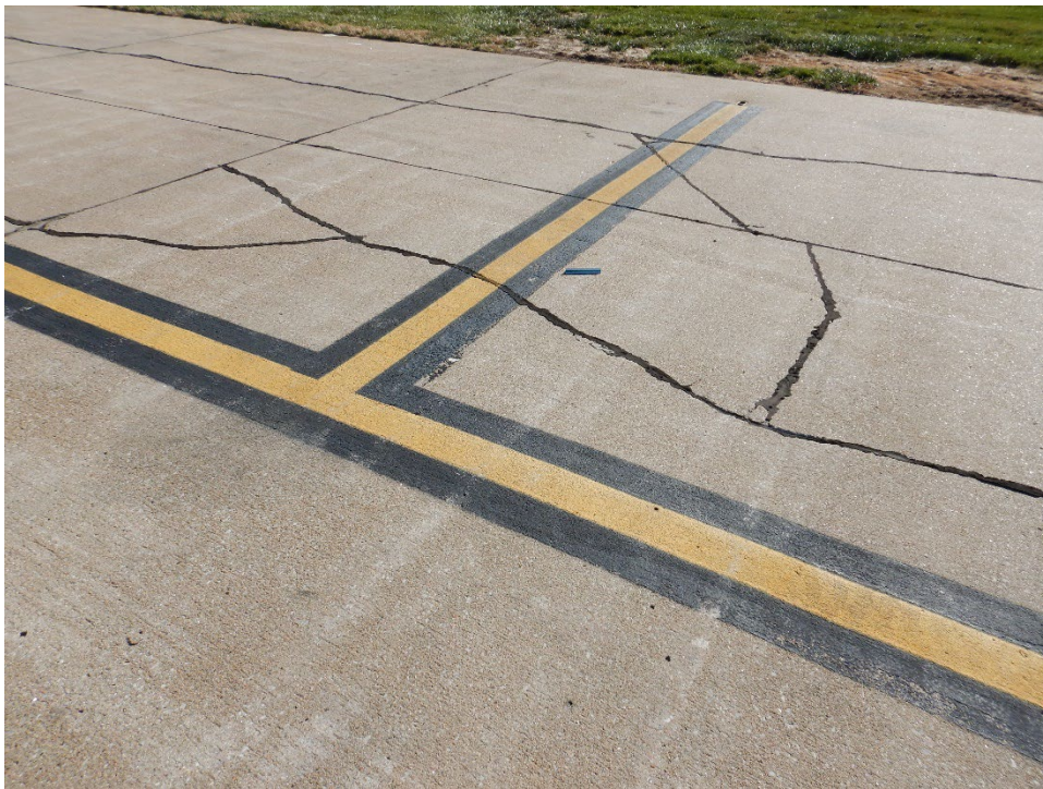
A02RO-01. Shattered Slab (Sample Unit No. 06).
