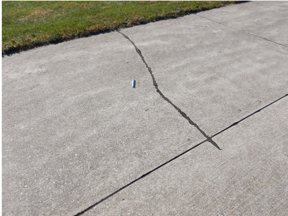
T02RO-01. LTD Cracking (Sample Unit No. 09).
