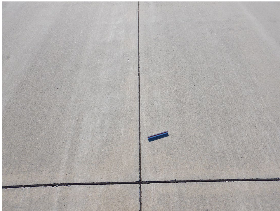
T06RO-01. Joint Seal Damage (Sample Unit No. 13).
