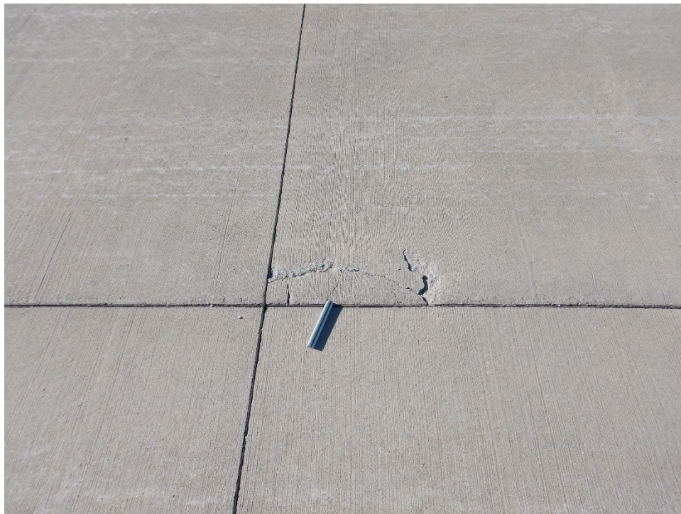
TH01RO-02. Joint Spalling (Sample Unit No. 01).
