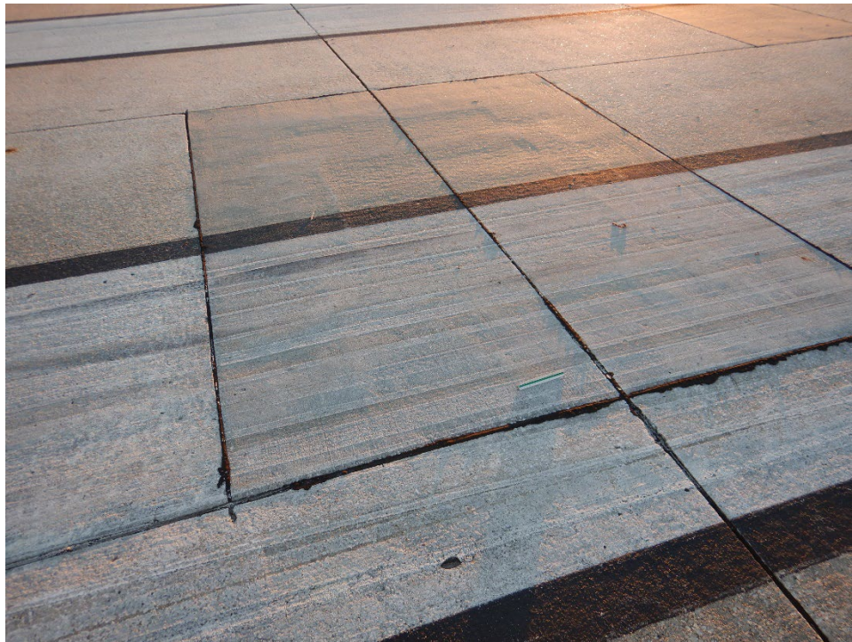
R17RO-02. Large Patching (Sample Unit No. 02).
