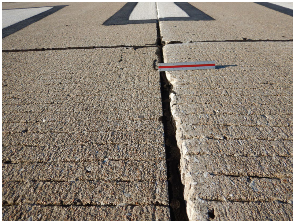
R05RO-01. Faulting (Sample Unit No. 16).
