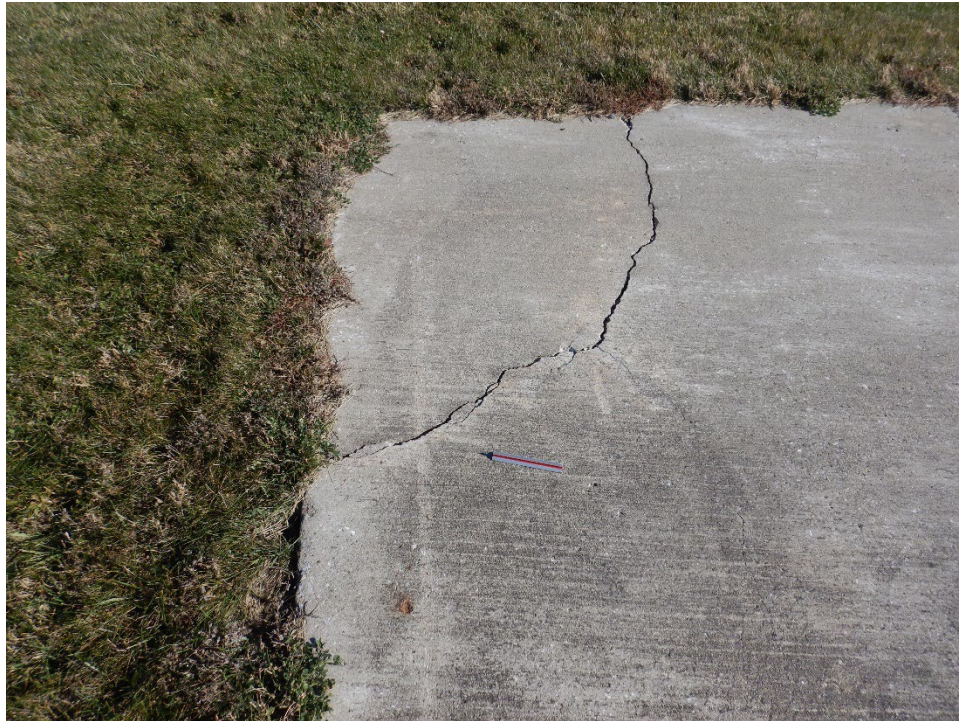
T03RO-01. Corner Break (Sample Unit No. 02).
