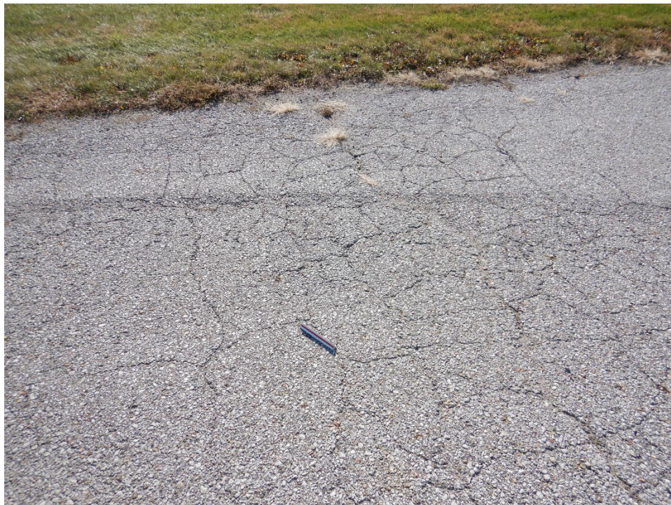
TH01RO-01. Alligator Cracking (Sample Unit No. 02).
