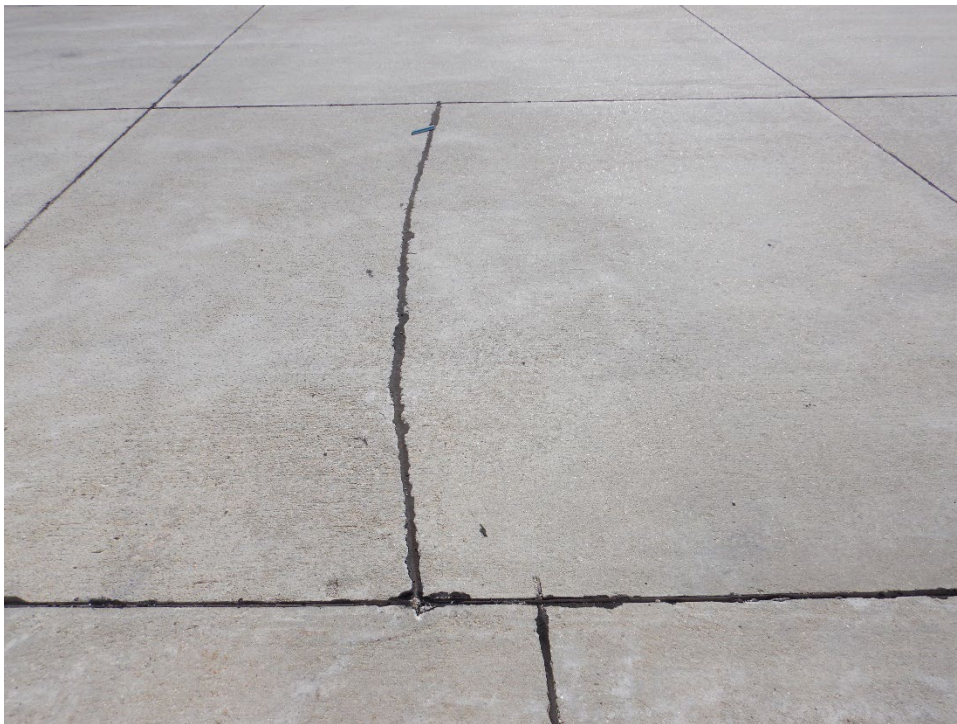
A01RO-01. LTD Cracking (Sample Unit No. 05).
