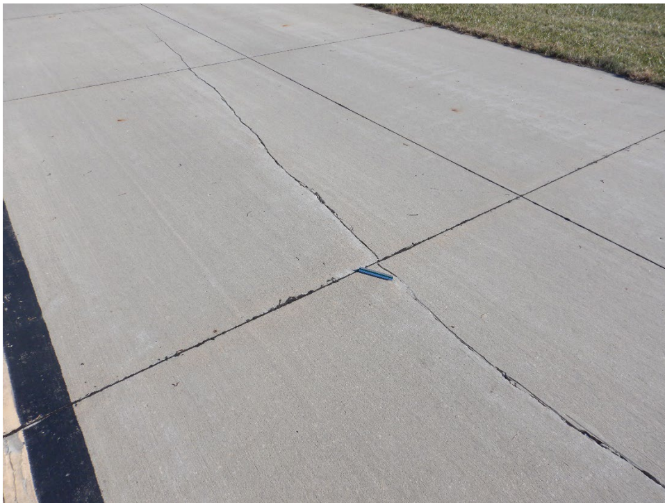
T07RO-01. LTD Cracking (Sample Unit No. 09).
