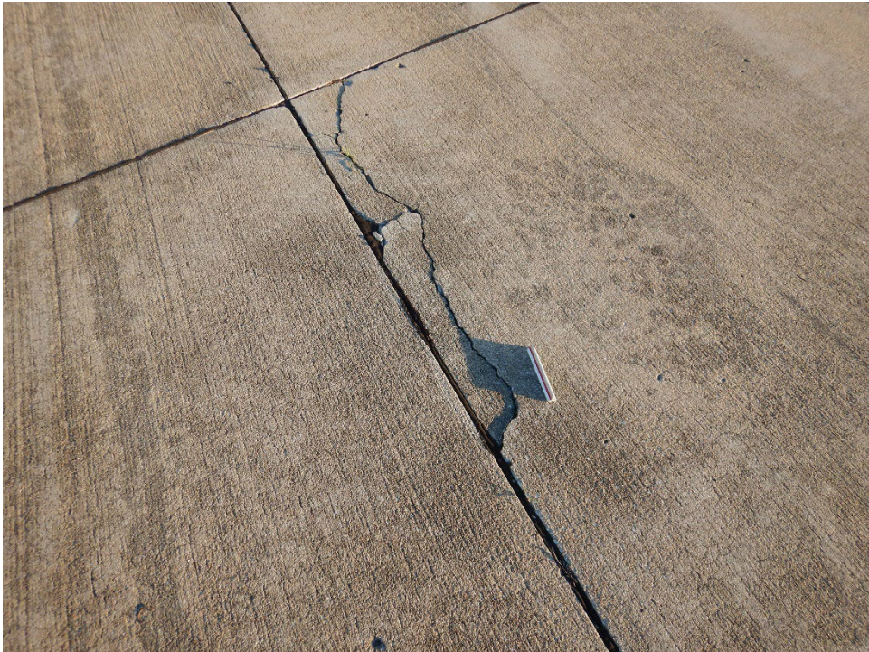
R17RO-03. Joint Spalling (Sample Unit No. 02).
