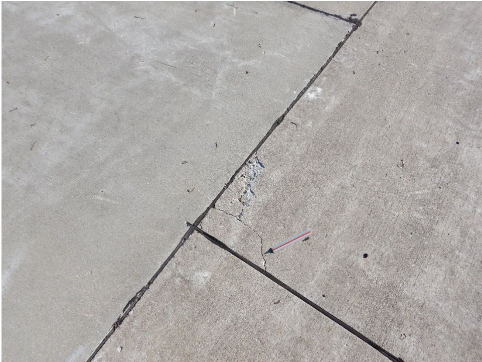
T01RO-01. Corner Spalling (Sample Unit No. 06).
