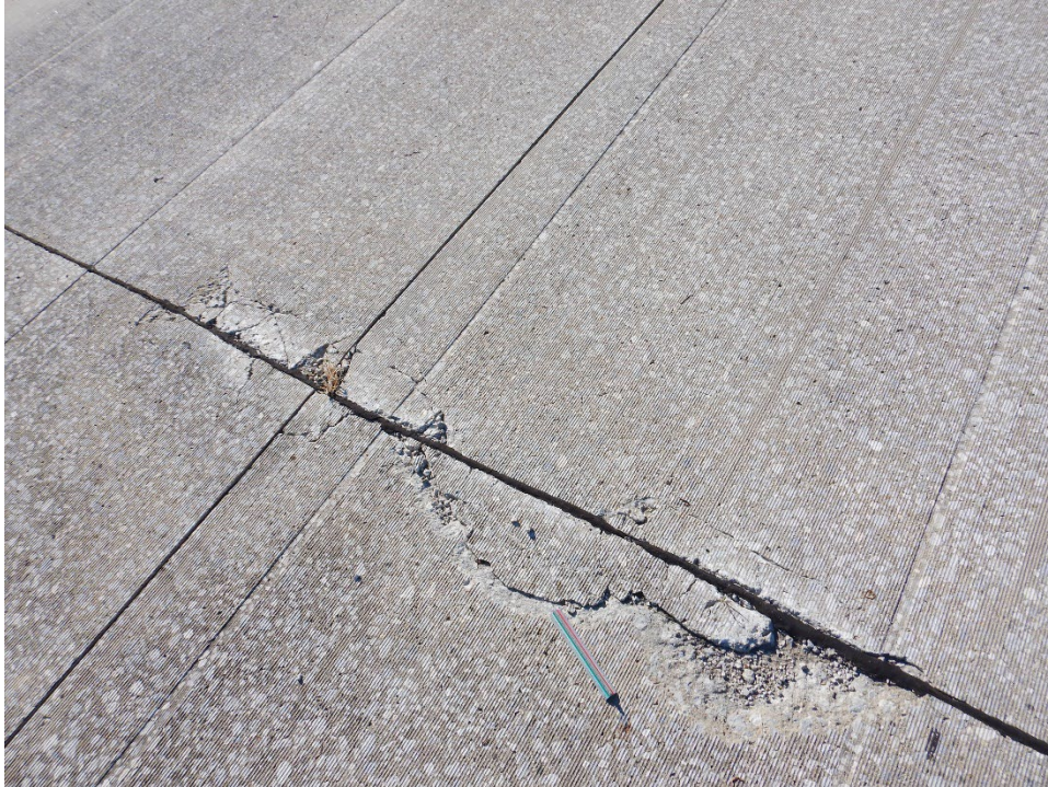
T07RO-01. Joint Spalling (Additional Sample Unit No. 16).
