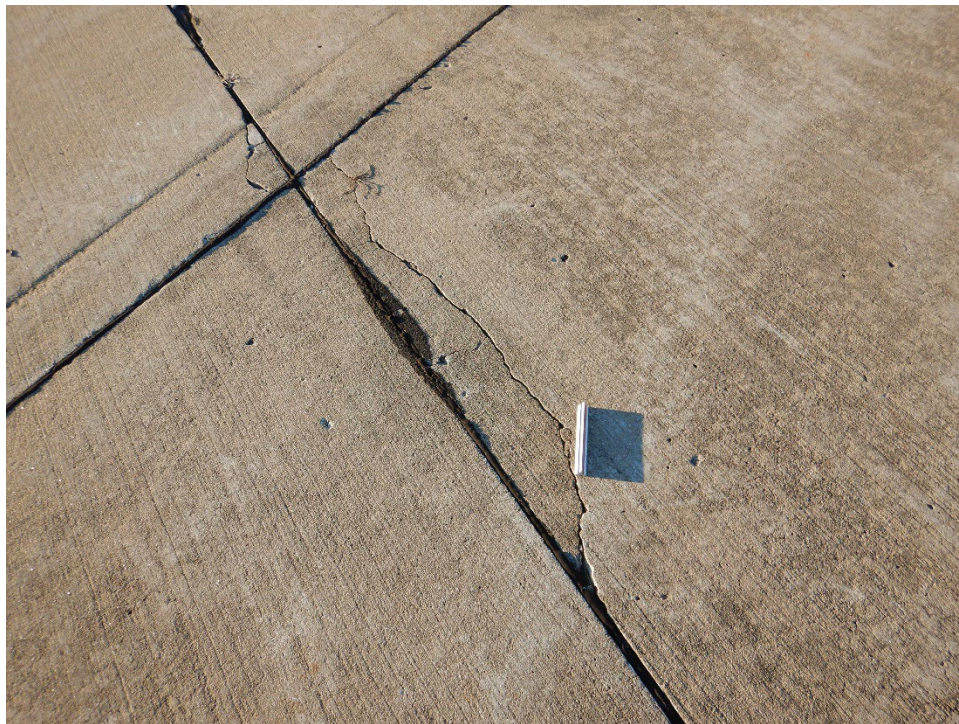
R17RO-04. Joint Spalling (Sample Unit No. 02).
