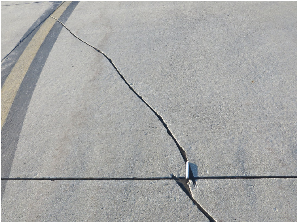
T01RC-02. LTD Cracking (Sample Unit No. 03).
