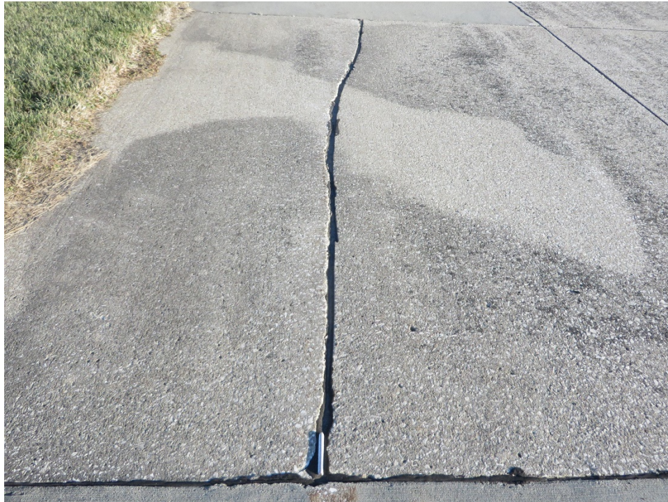
R12RC-01. LTD Cracking (Sample Unit No. 51).
