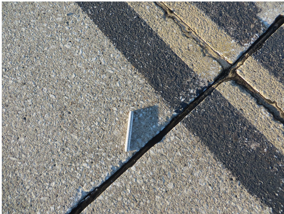
T01RC-01. Joint Seal Damage (Sample Unit No. 03).
