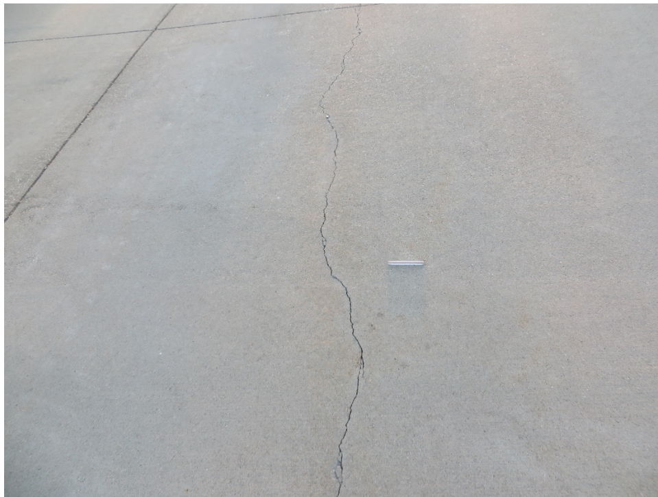
A01RC-02. LTD Cracking (Sample Unit No. 03).
