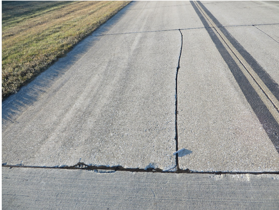
T01RC-01. LTD Cracking (Sample Unit No. 03).
