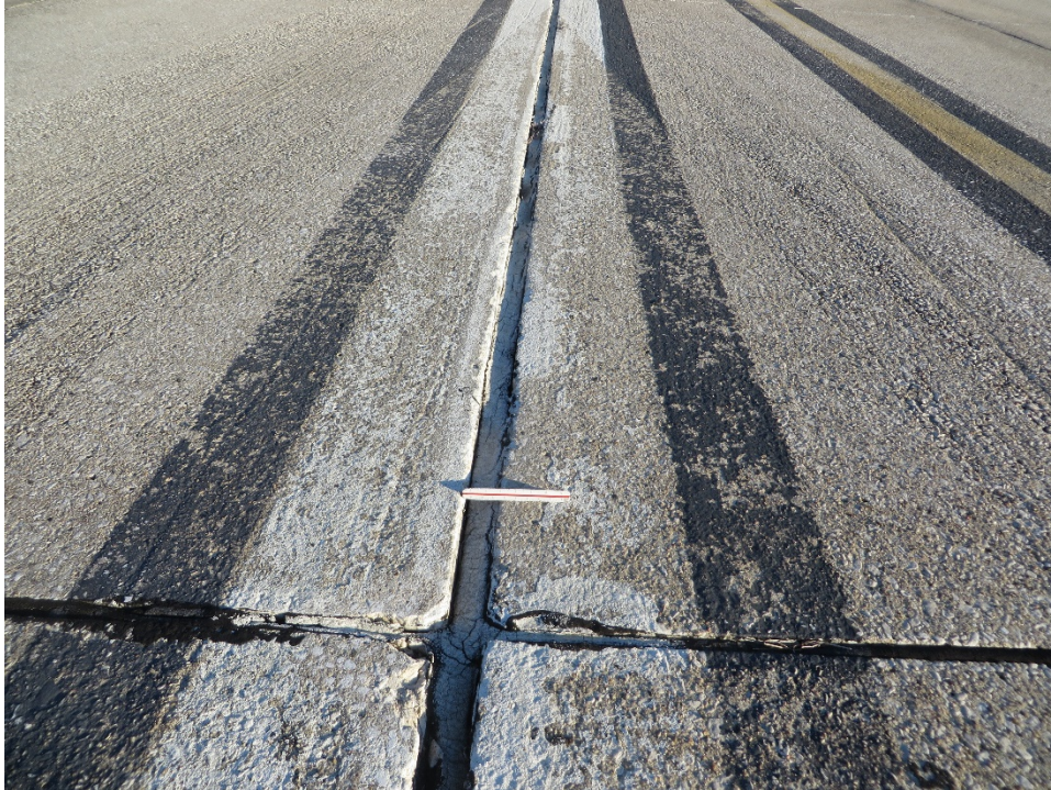
R12RC-01. Faulting (Sample Unit No. 05).
