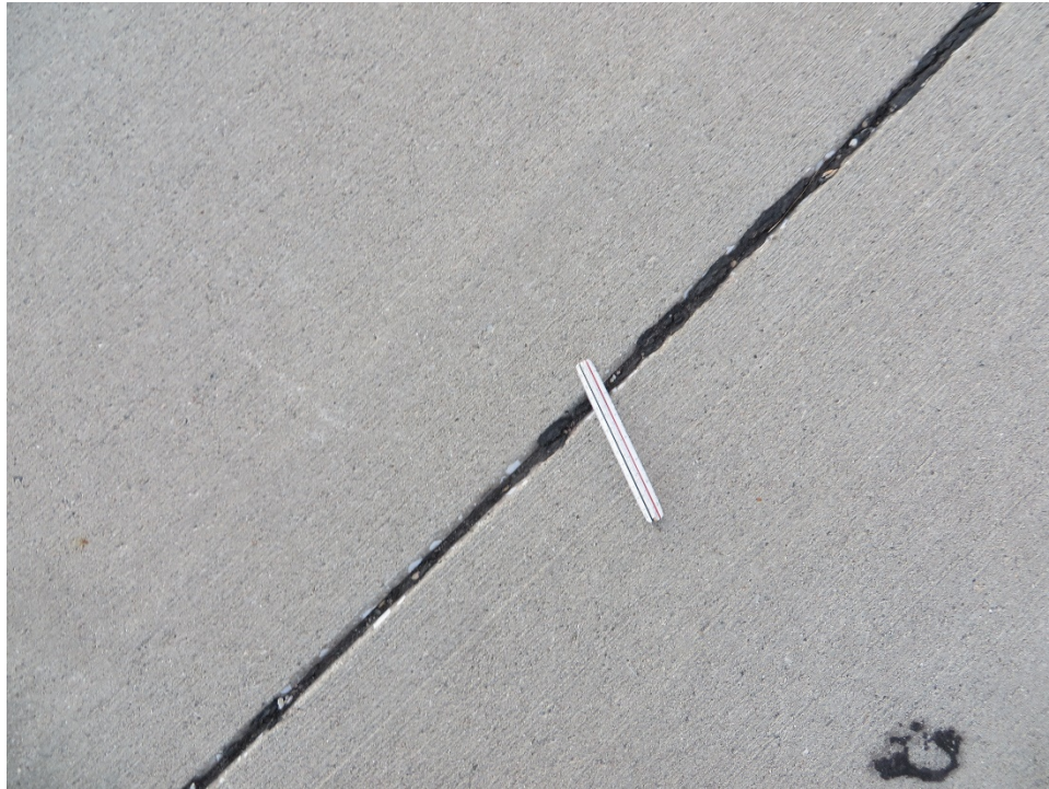
A01RC-01. Joint Seal Damage (Sample Unit No. 04).
