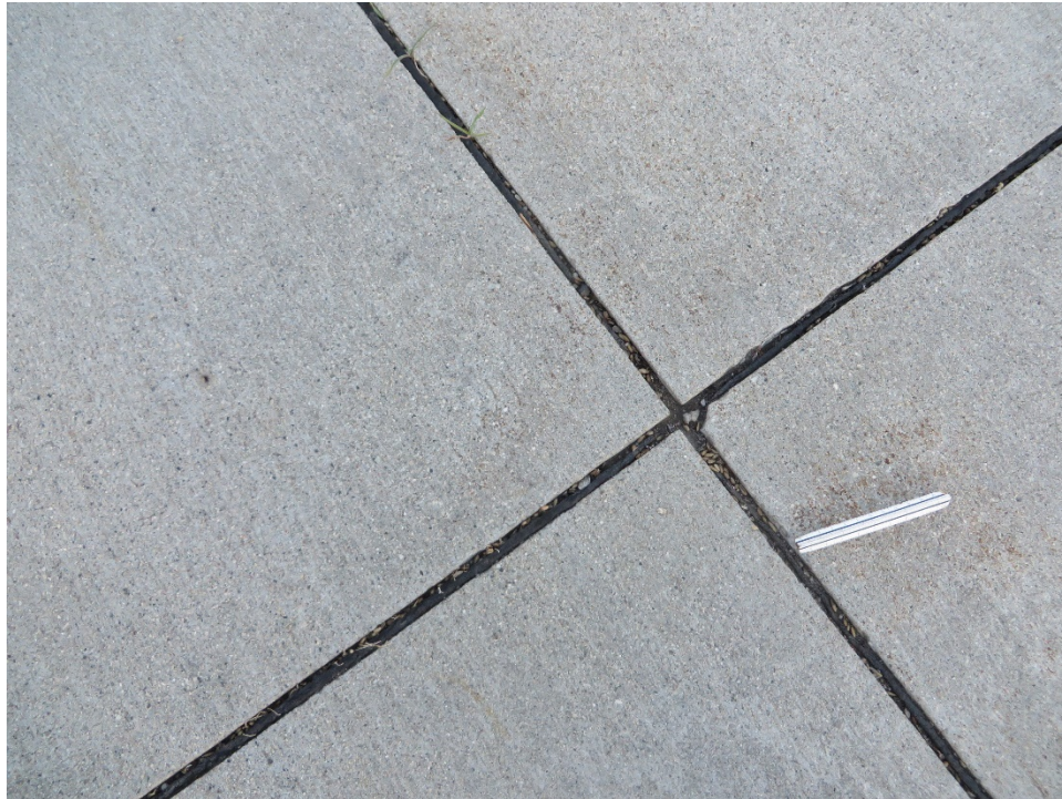
A02RC-01. Joint Seal Damage (Sample Unit No. 14).
