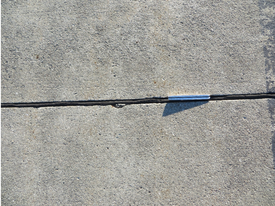
T02RC-01. Joint Seal Damage (Sample Unit No. 01).
