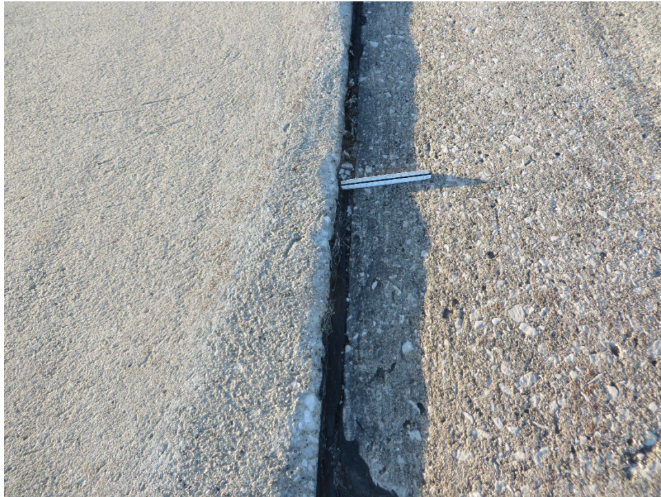
T01RC-01. Faulting (Sample Unit No. 02).
