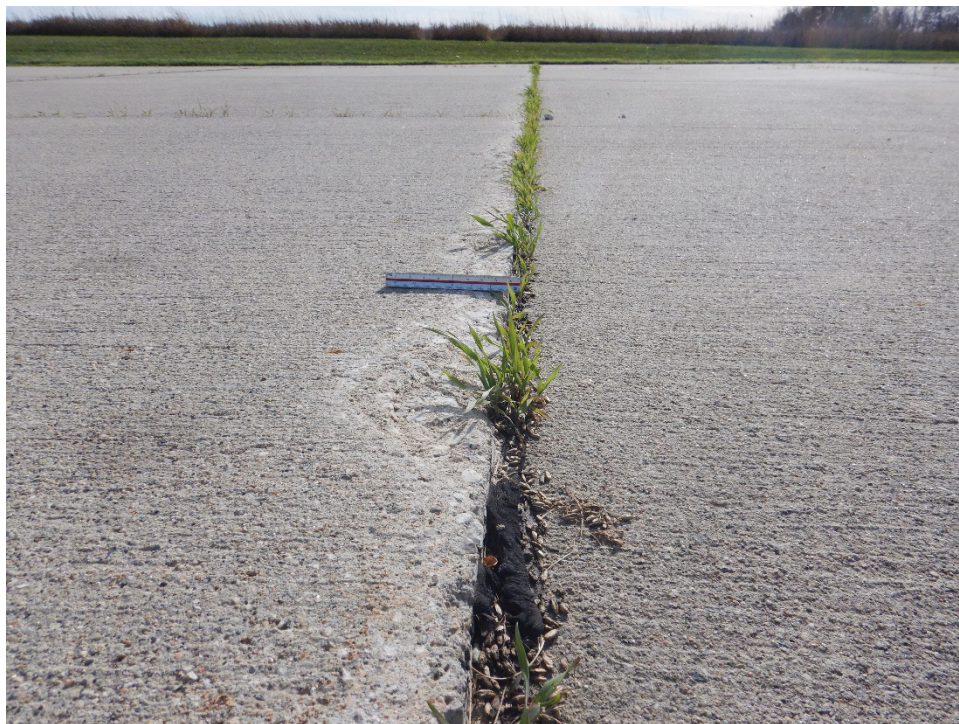
A02RC-01. Faulting (Sample Unit No. 11).
