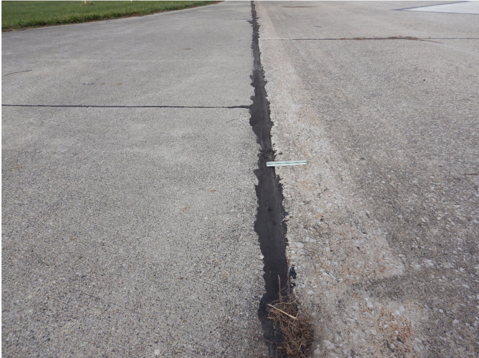
T02RC-01. Faulting (Sample Unit No. 01).
