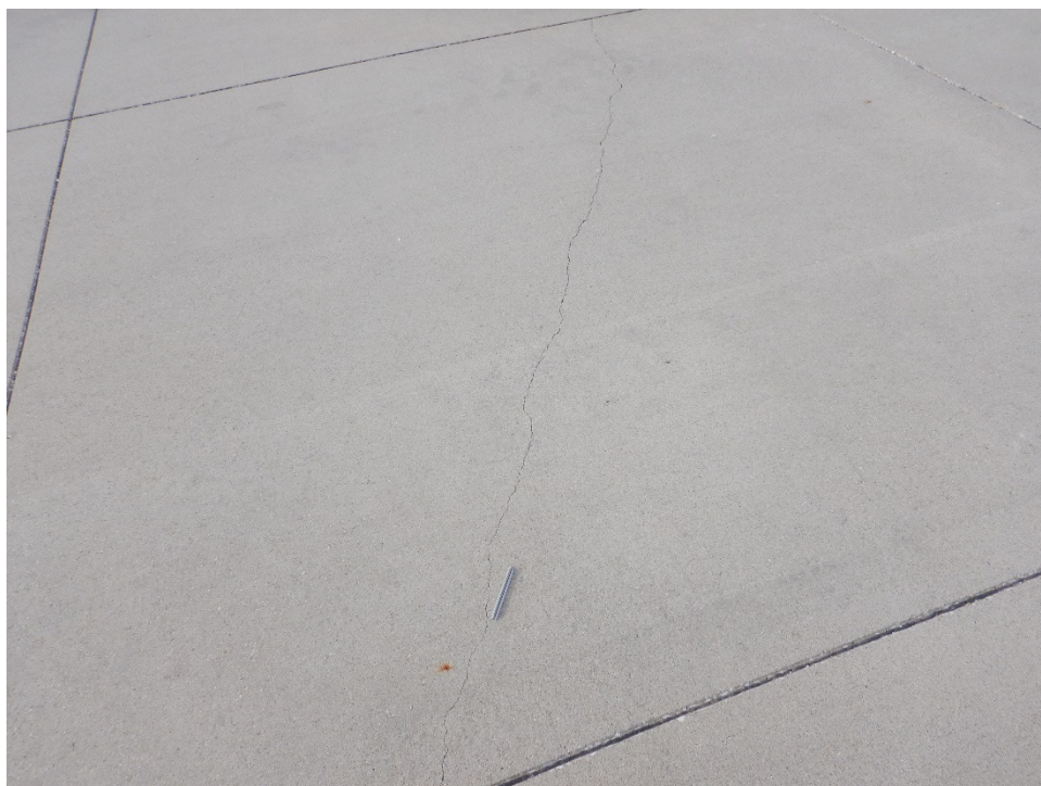
A01RC-01. LTD Cracking (Sample Unit No. 04).
