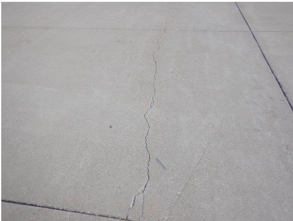
A01RC-02. LTD Cracking (Sample Unit No. 03).
