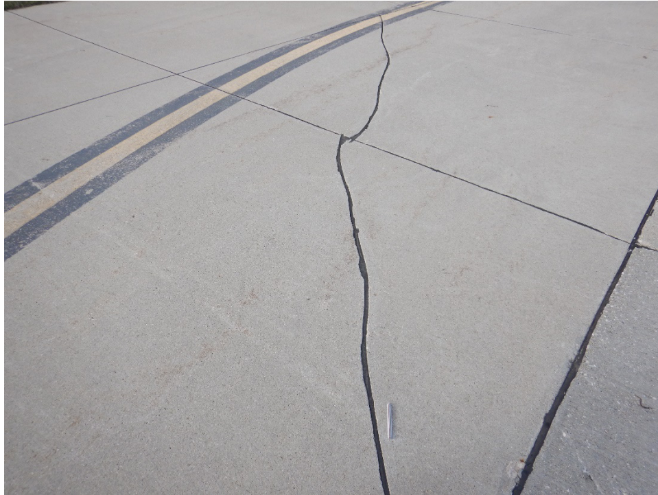
T01RC-02. LTD Cracking (Sample Unit No. 03).
