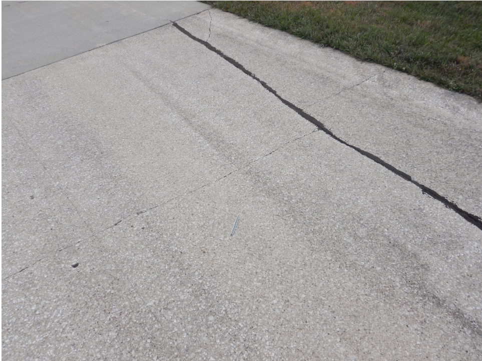
T01RC-01. Shattered Slab (Sample Unit No. 03).
