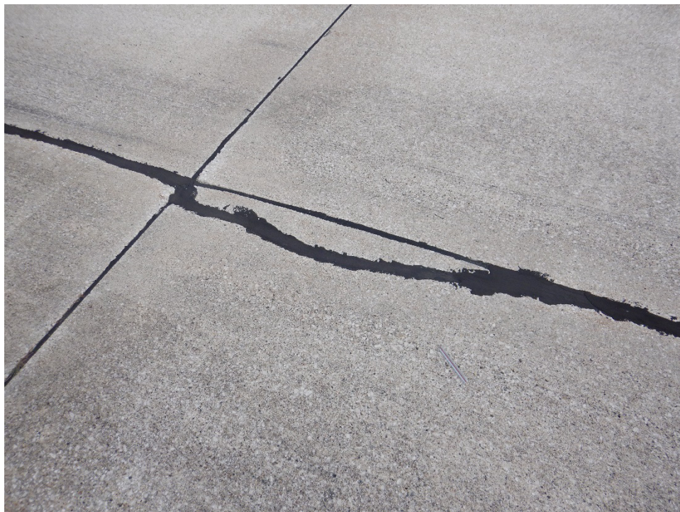
R12RC-01. Joint Spalling (Sample Unit No. 25).
