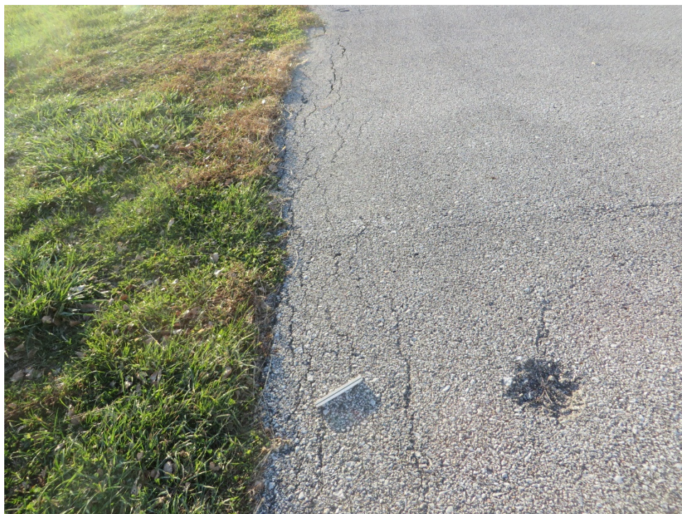
TH01SH-04. Alligator Cracking (Sample Unit No. 01).
