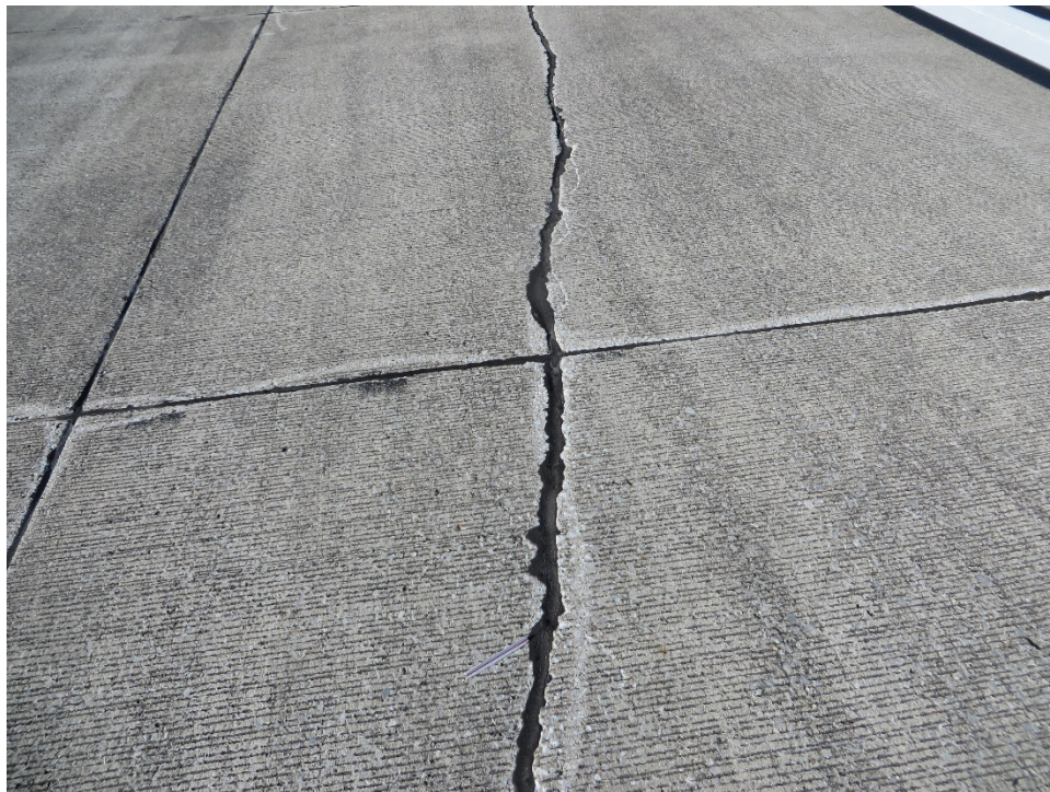
R12SH-02. LTD Cracking (Sample Unit No. 01).
