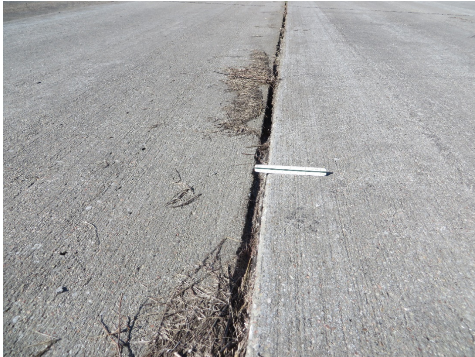
R12SH-01. Faulting (Sample Unit No. 05).
