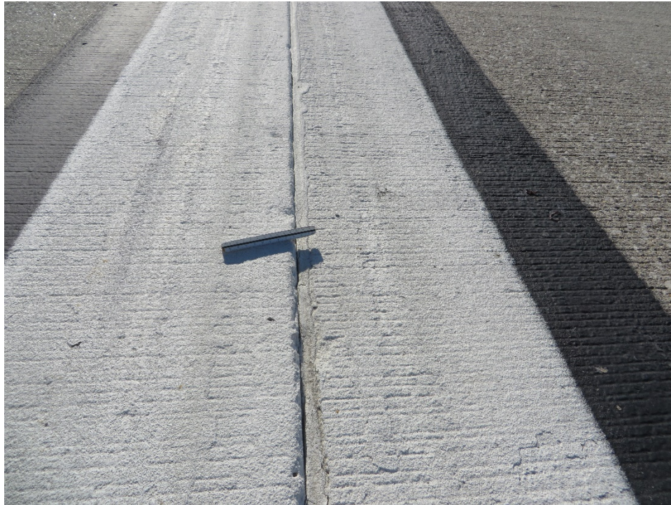
R04SH-01. Faulting (Sample Unit No. 07).
