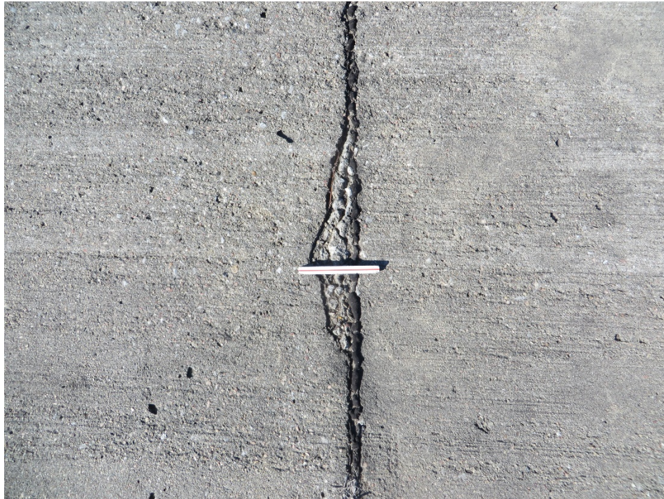
T01SH-01. Joint Spalling (Sample Unit No. 05).
