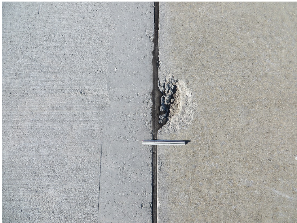
R12SH-04. Joint Spalling (Sample Unit No. 01).
