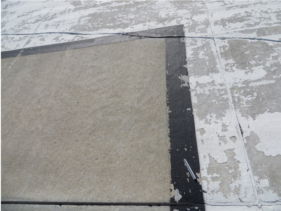
R12SH-04. LTD Cracking (Sample Unit No. 03).
