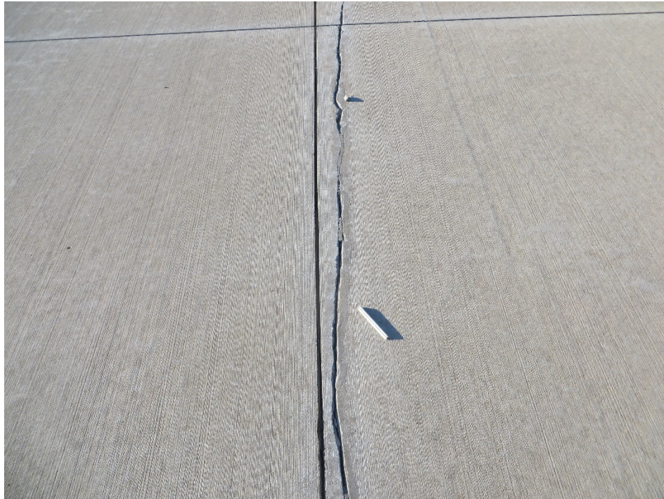
T03SH-02. Joint Spalling (Sample Unit No. 26).
