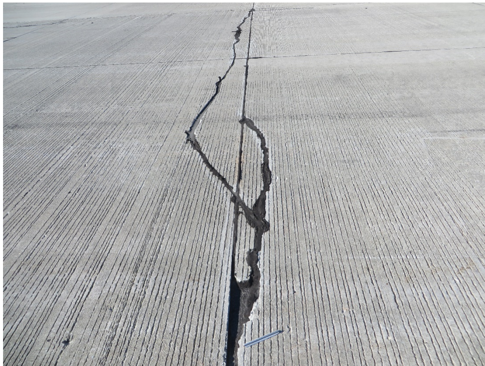
R04SH-02. Joint Spalling (Sample Unit No. 05).
