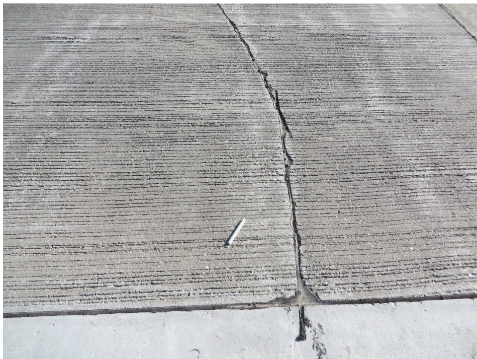
R12SH-03. LTD Cracking (Sample Unit No. 02).
