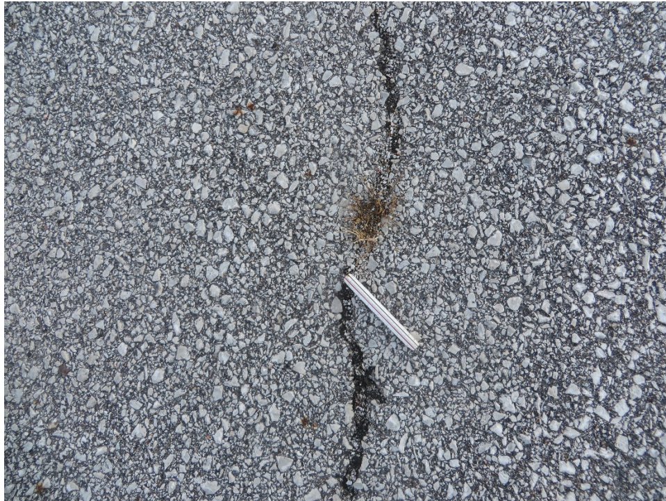
TH01SH-03. L&T Cracking (Sample Unit No. 01).
