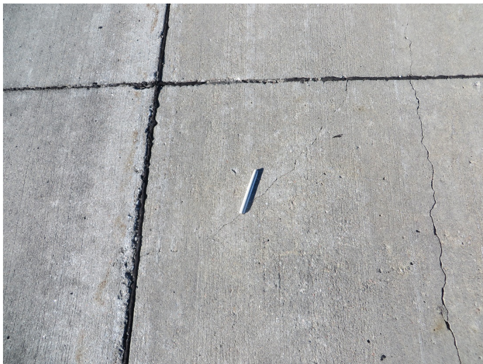
R12SH-01. Corner Break (Sample Unit No. 55).
