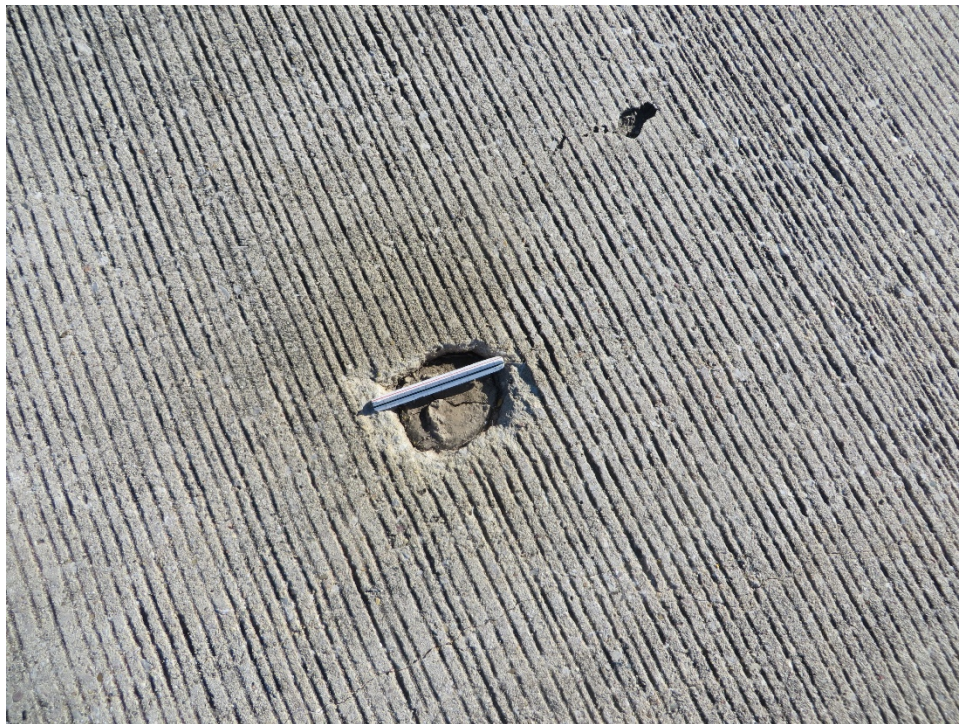
R04SH-01. Small Patching (Sample Unit No. 70).
