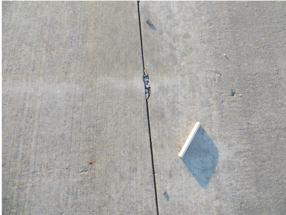
TH01SH-02. Joint Seal Damage (Sample Unit No. 01).
