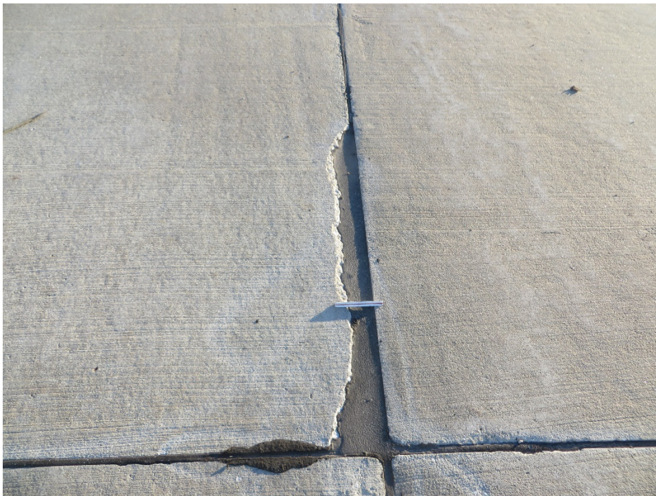
A02SH-03. Joint Spalling (Sample Unit No. 07).
