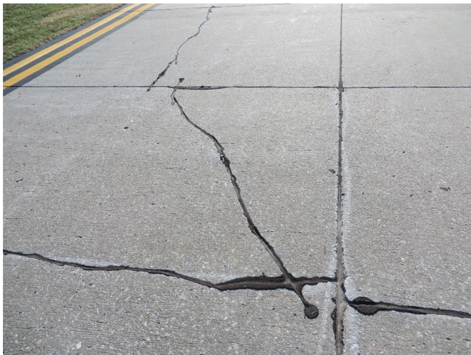
T03SH-03. LTD Cracking (Sample Unit No. 06).
