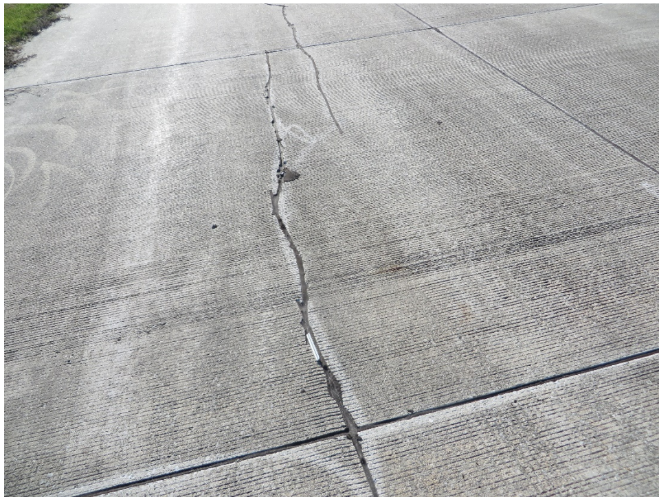
R04SH-01. LTD Cracking (Sample Unit No. 51).
