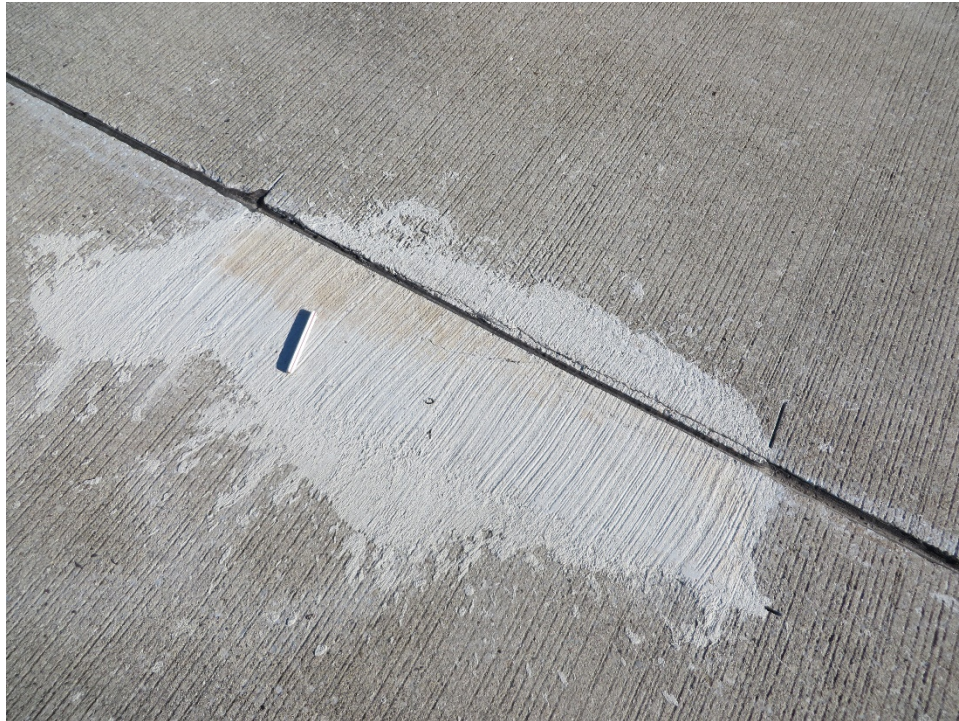
R04SH-01. Small Patching (Sample Unit No. 51).
