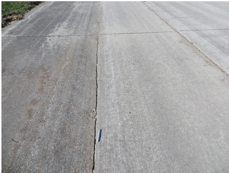
R12SH-01. LTD Cracking (Sample Unit No. 05).
