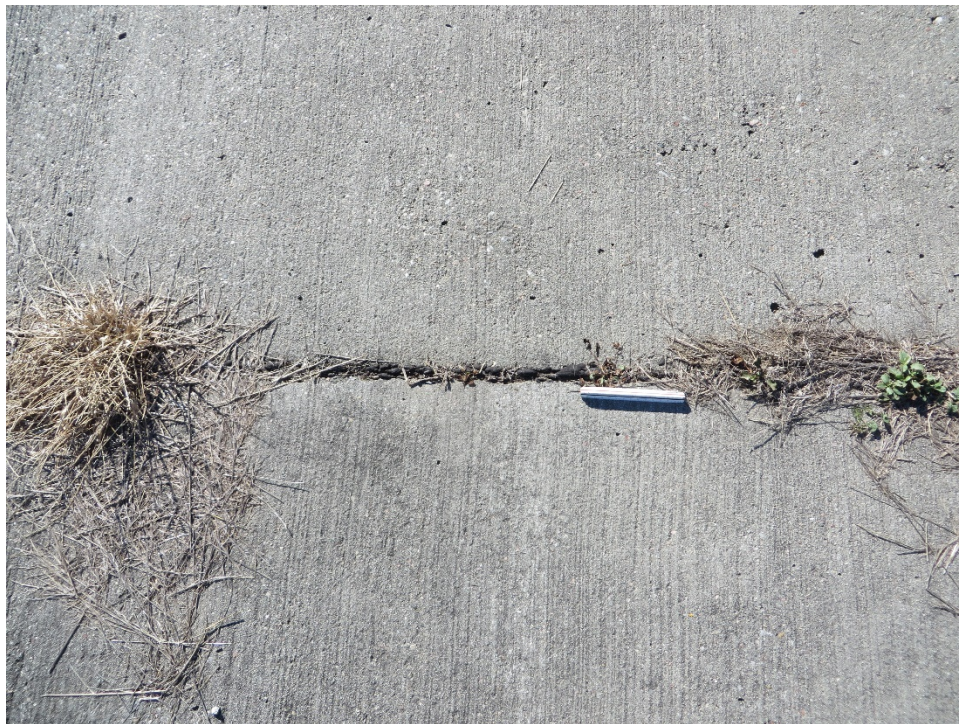
T01SH-01. Joint Seal Damage (Sample Unit No. 04).
