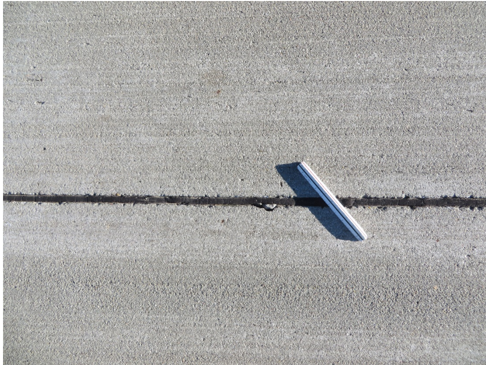
T03SH-01. Joint Seal Damage (Sample Unit No. 14).
