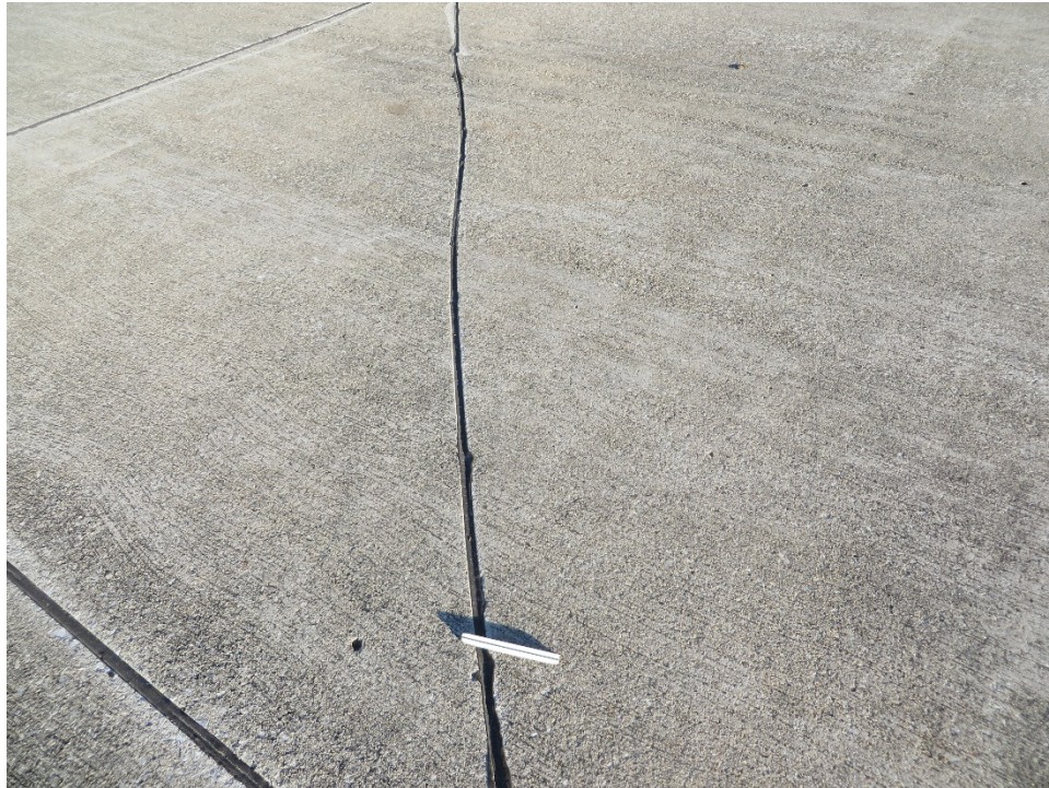
A02SH-01. LTD Cracking (Sample Unit No. 03).
