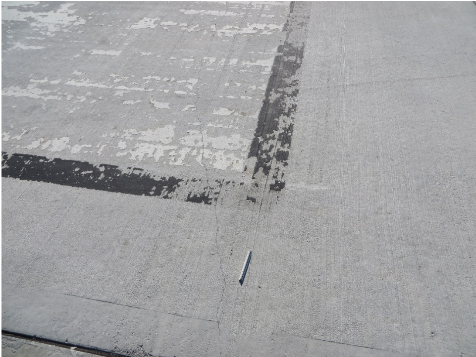
R12SH-04. LTD Cracking (Sample Unit No. 02).
