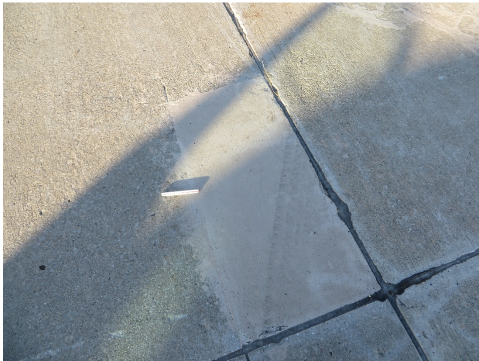
A02SH-02. Small Patching (Sample Unit No. 01).
