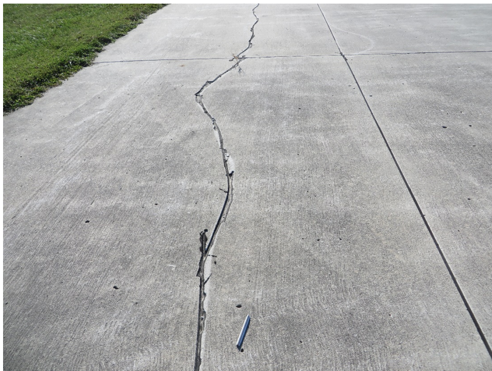
T04SH-01. LTD Cracking (Sample Unit No. 08).
