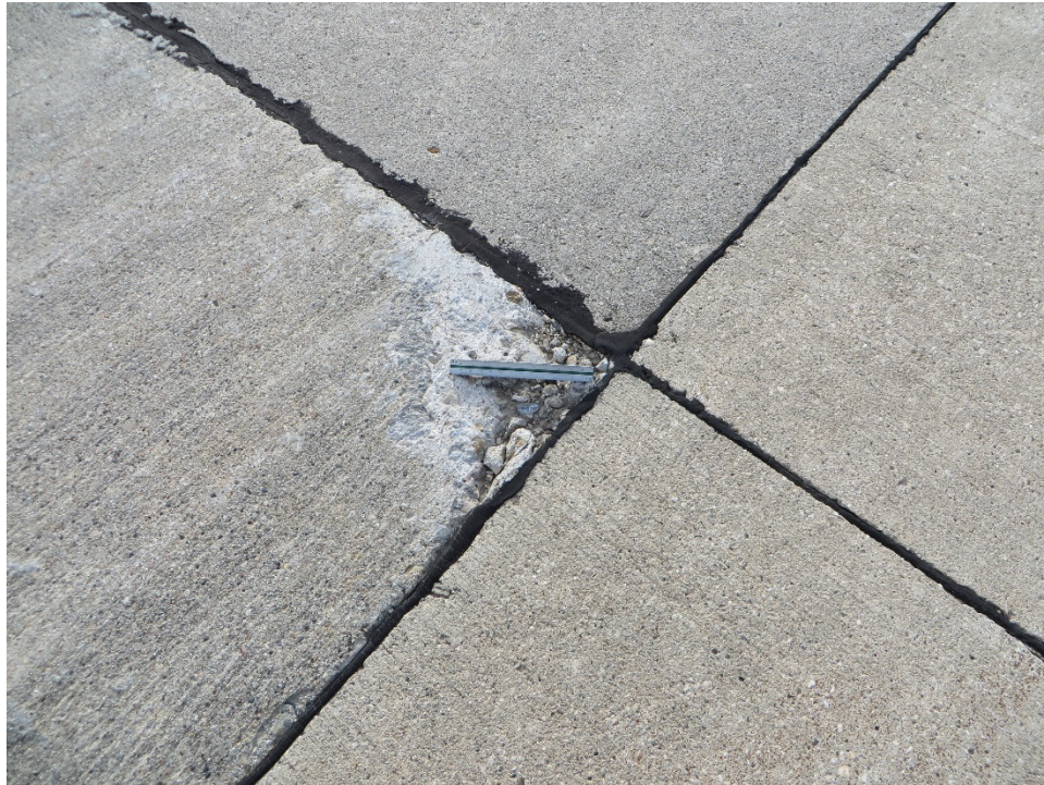
T01IS-01. Corner Spalling (Sample Unit No. 01).
