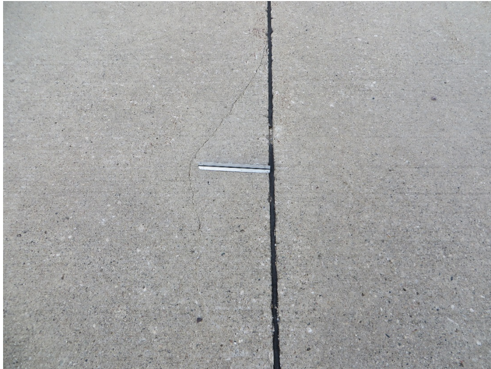
T02IS-01. Joint Spalling (Sample Unit No. 03).
