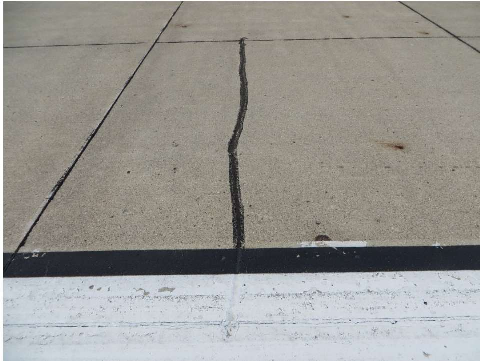
R17IS-01. LTD Cracking (Sample Unit No. 32).
