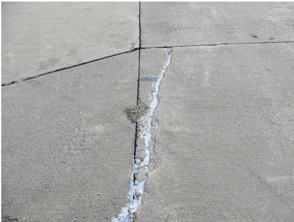
A01IS-01. Joint Spalling (Sample Unit No. 05).
