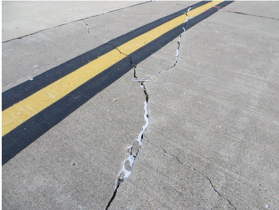
T03IS-04. Shattered Slab (Sample Unit No. 03).
