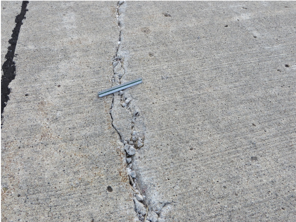
T03IS-03. LTD Cracking (Sample Unit No. 03).
